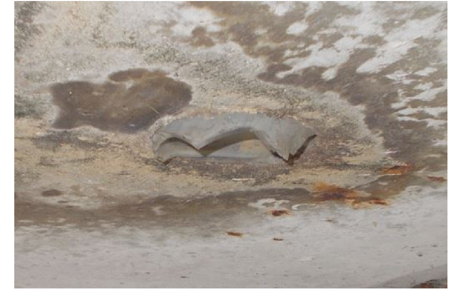
BROKEN 3" Ø P. V. C. PIPE DRAIN
