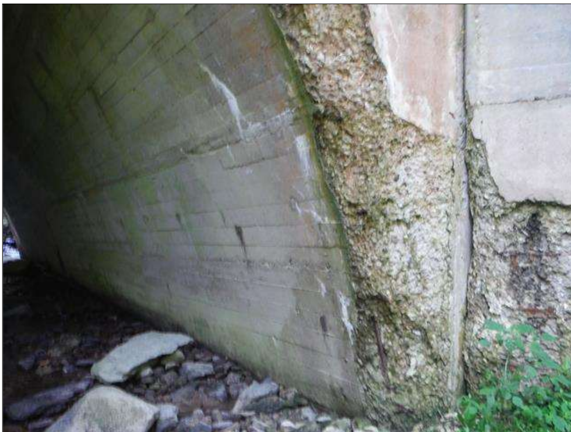
150 SF. X UP TO 4" DEEP SPALL WITH EXPOSED REBAR IN DOWNSTREAM HEADWALL (PM)
