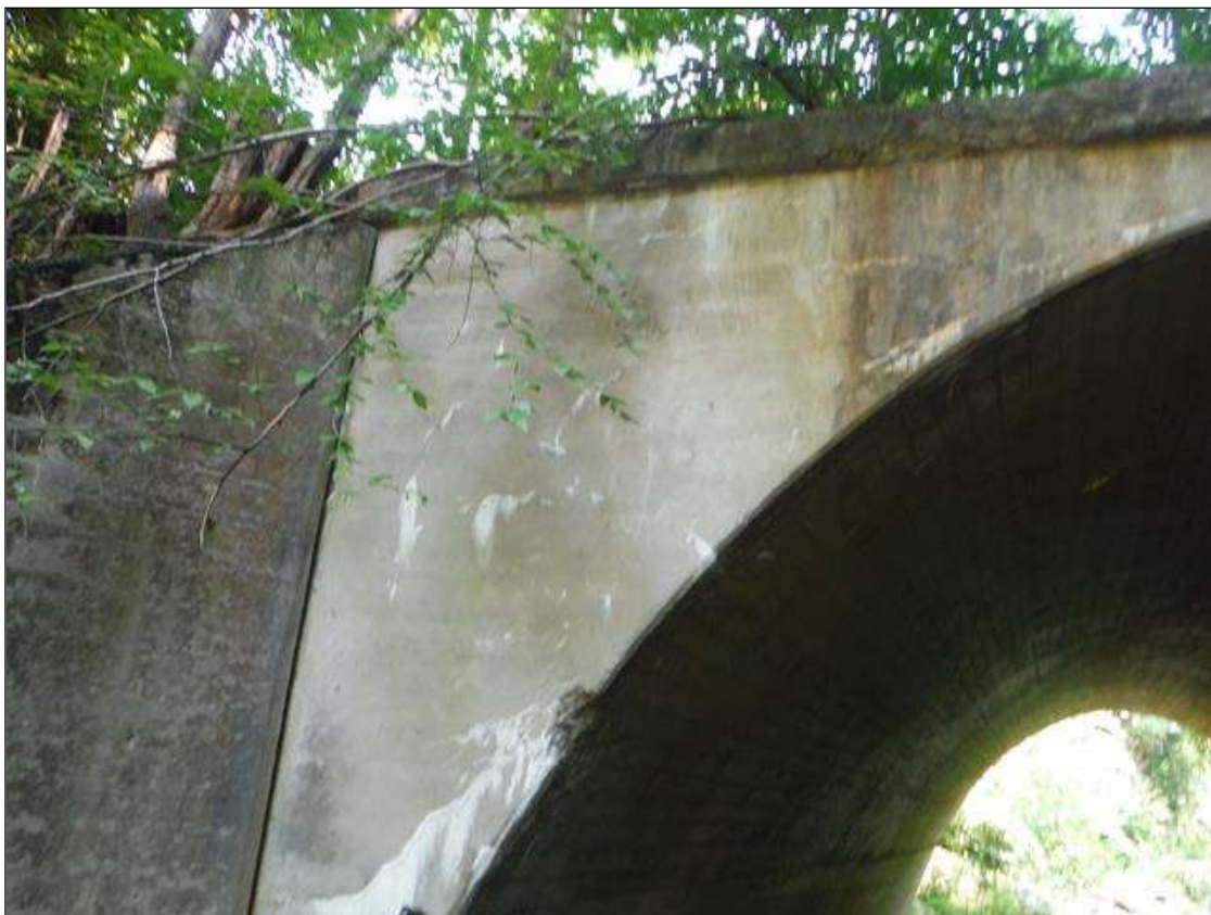
100 SF. OF VERTICAL AND LONGITUDINAL CRACKING WITH EFFLORESCENCE IN UPSTREAM HEADWALL
