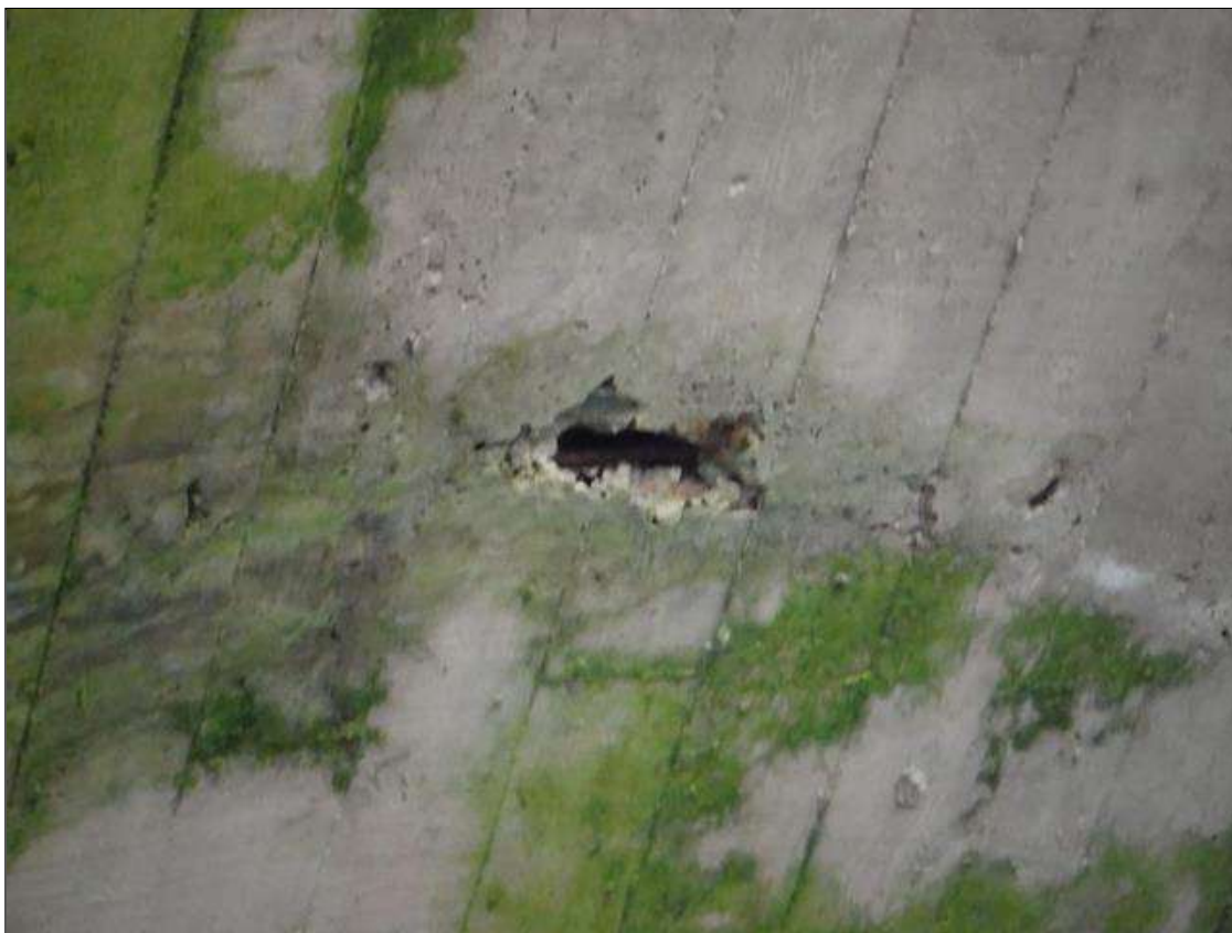
Barrel 1 Section 1: 6" X 1" X 4" DEEP SPALL WITH EXPOSED REBAR IN TOP OF PIPE 25 FT. FROM DOWNSTREAM END
