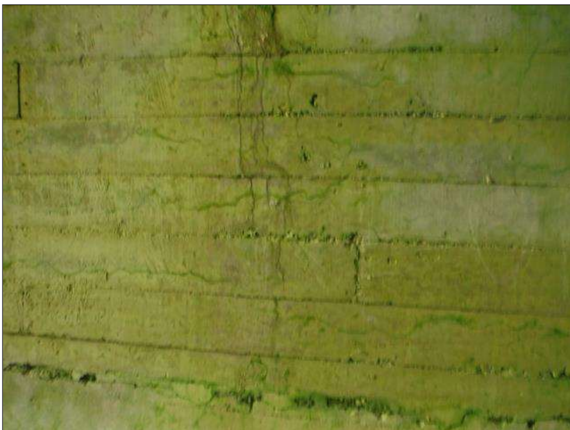
2300 SF. OF LONGITUDINAL CRACKING AND MAP CRACKING UP TO 1/32" WIDE
