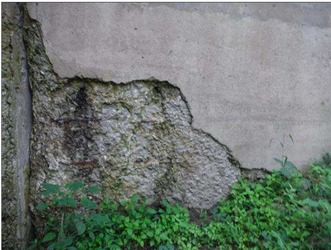
5 FT. X 4 FT. X 2" DEEP SPALL WITH EXPOSED REBAR IN NORTHEAST WINGWALL
