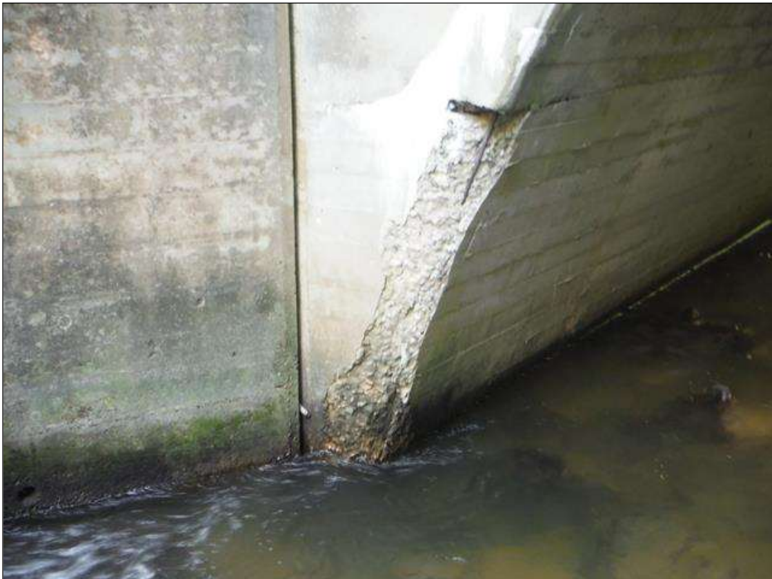
5 FT. X 1 FT. X 4" DEEP SPALL WITH EXPOSED REBAR IN UPSTREAM HEADWALL (PM)
