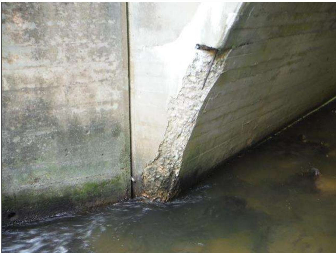
5 FT. X 1 FT. X 4" DEEP SPALL WITH EXPOSED REBAR IN UPSTREAM HEADWALL (PM)
