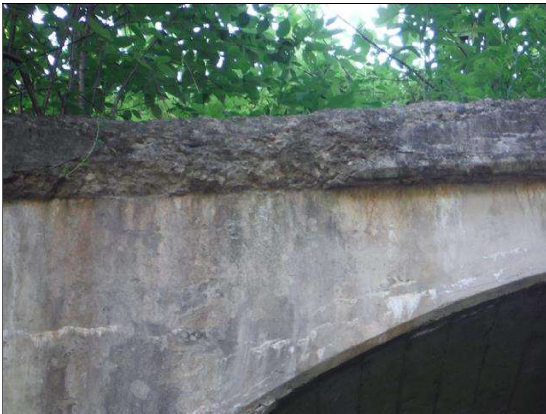
36 FT. X 1 FT. X 2" DEEP SPALL IN UPSTREAM HEADWALL
