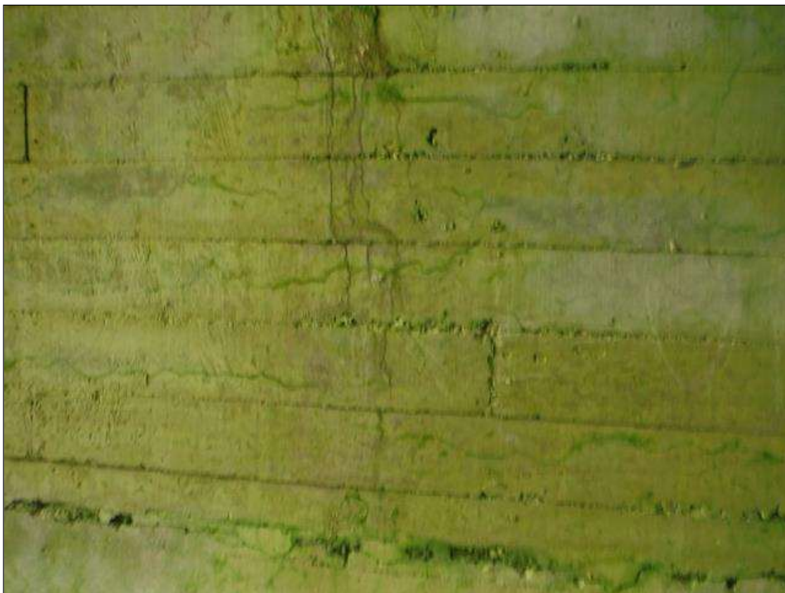
Barrel 1 Section 1: 2300 SF. OF LONGITUDINAL CRACKING AND MAP CRACKING UP TO 1/32" WIDE
