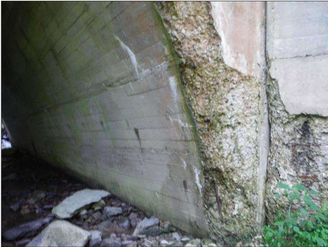
150 SF. X UP TO 4" DEEP SPALL WITH EXPOSED REBAR IN DOWNSTREAM HEADWALL (PM)
