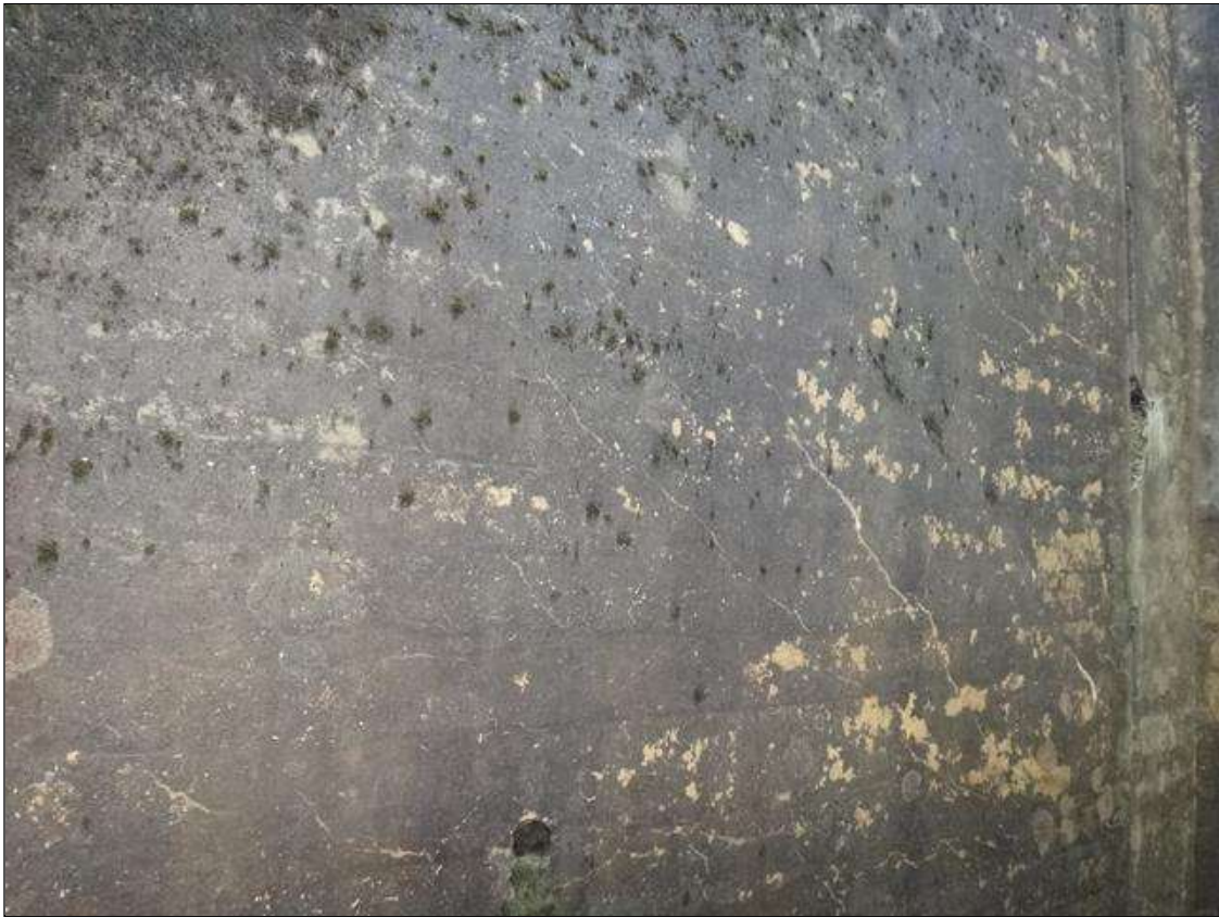
southeast wingwall, multiple diagonal cracks (up to 6ft x hairline)
