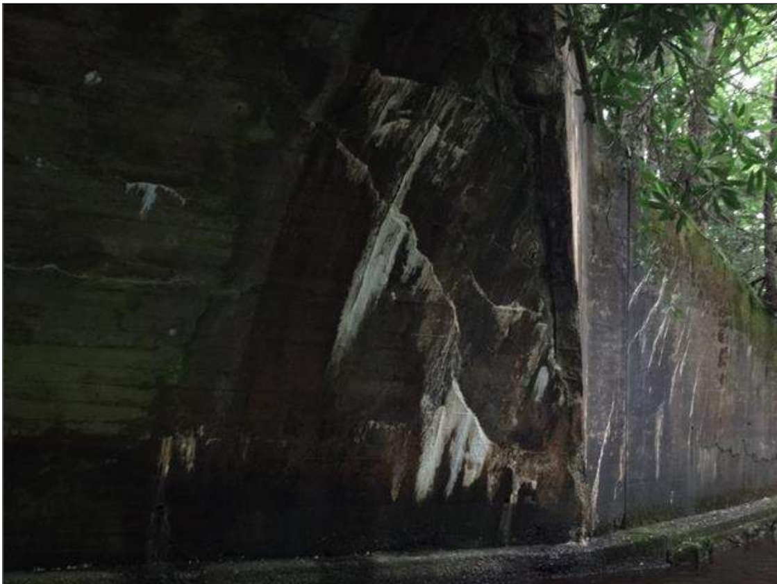
Barrel 1 Section 1: south wall at west end of barrel 1, cracking (12ft x up to 1/8in) with efflorescence
