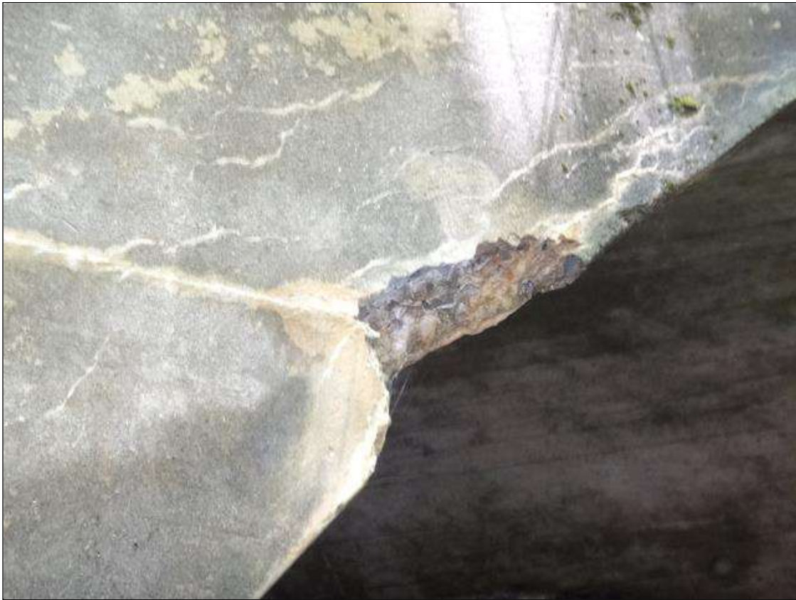
east headwall at south end, spall (10in x 5in x up to 4in)
