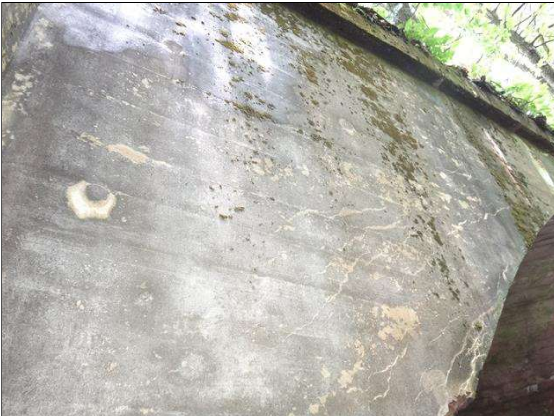
east headwall at south end, multiple diagonal cracks (up to 10ft x hairline)
