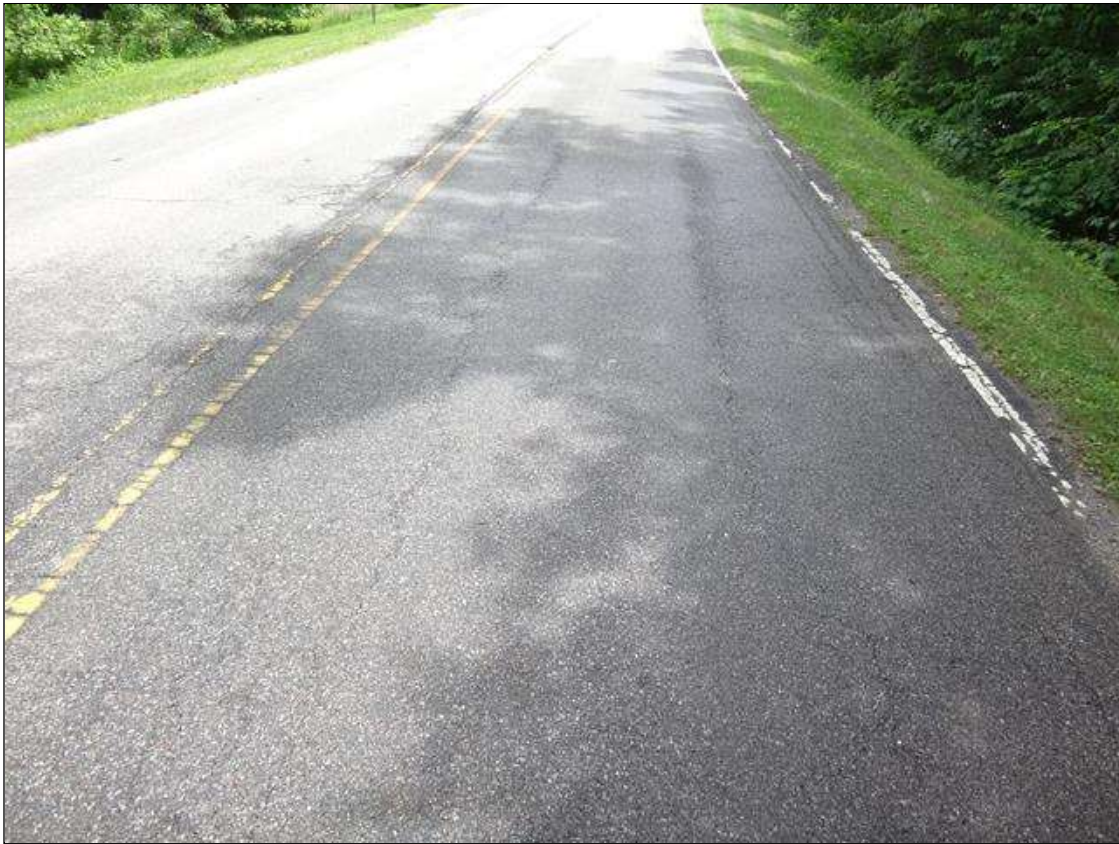
northbound lane over culvert, (2) longitudinal cracks (full length x up to 1/8in)
