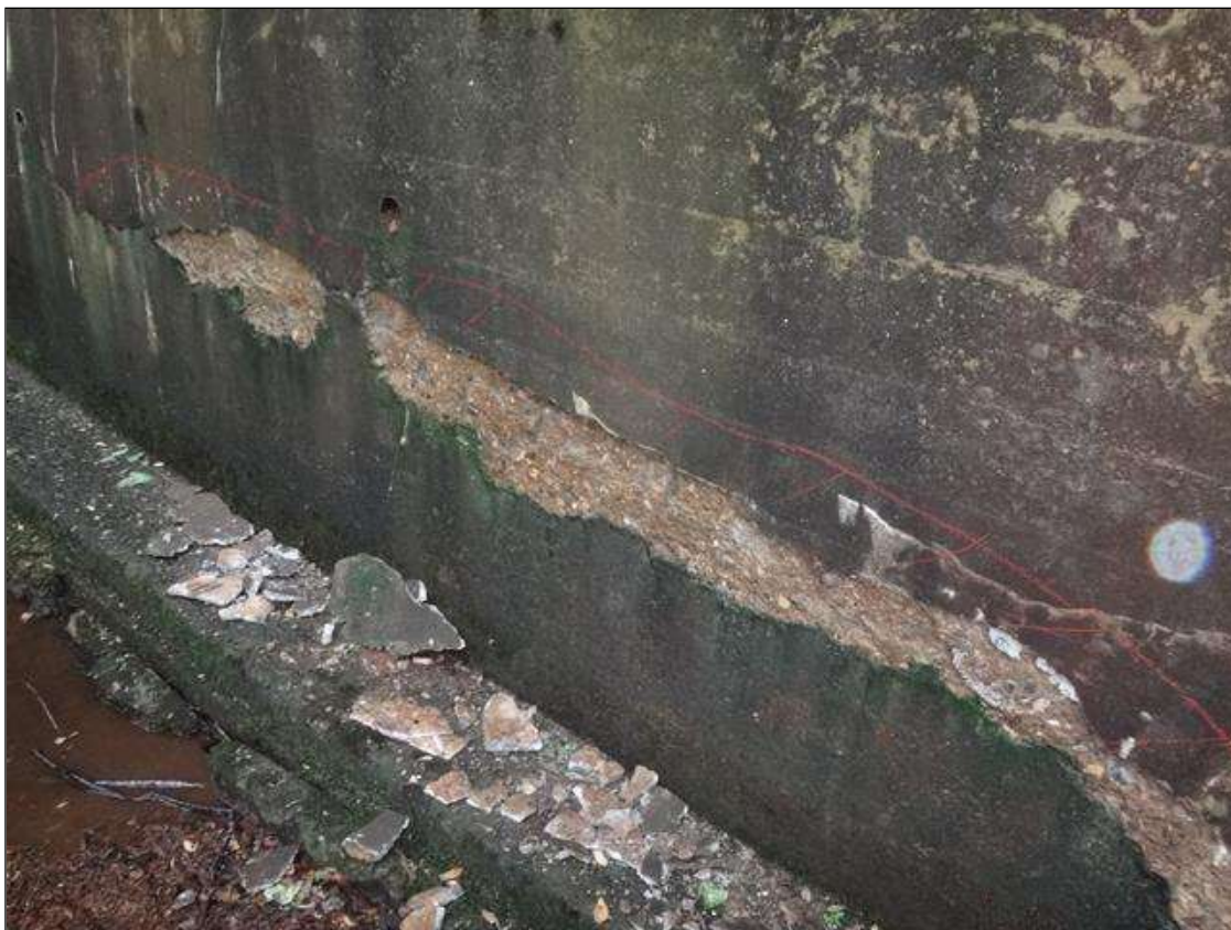
southwest wingwall, spall (13ft x up to 1ft x up to 1in) with adjacent delamination (13ft x up to 1ft)
