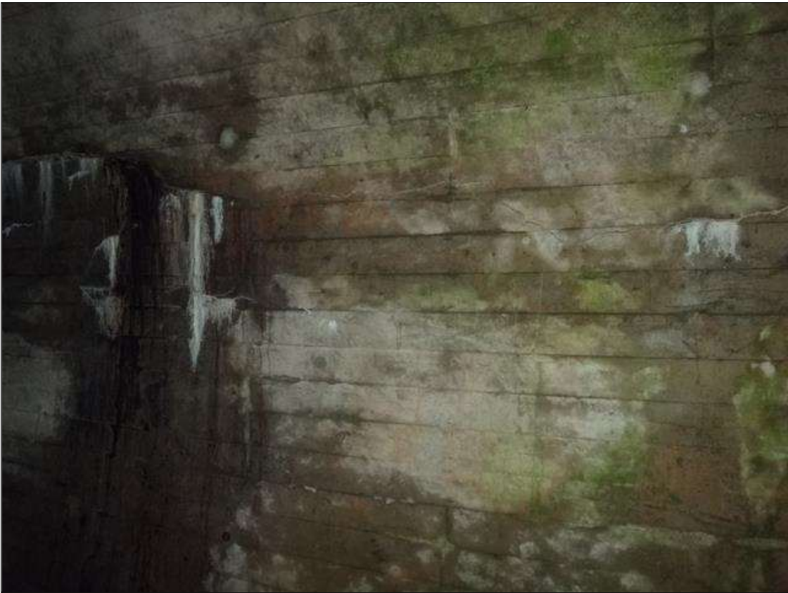
Barrel 1 Section 1: near top of north wall, (2) longitudinal cracks (24ft x up to 1/4in) at east end
