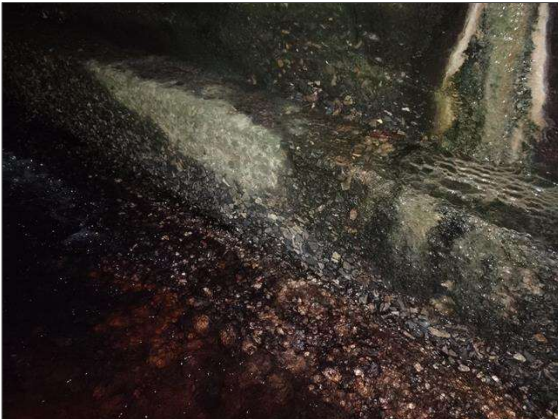
south footing at waterline, abrasion (full length) with exposed aggregate
