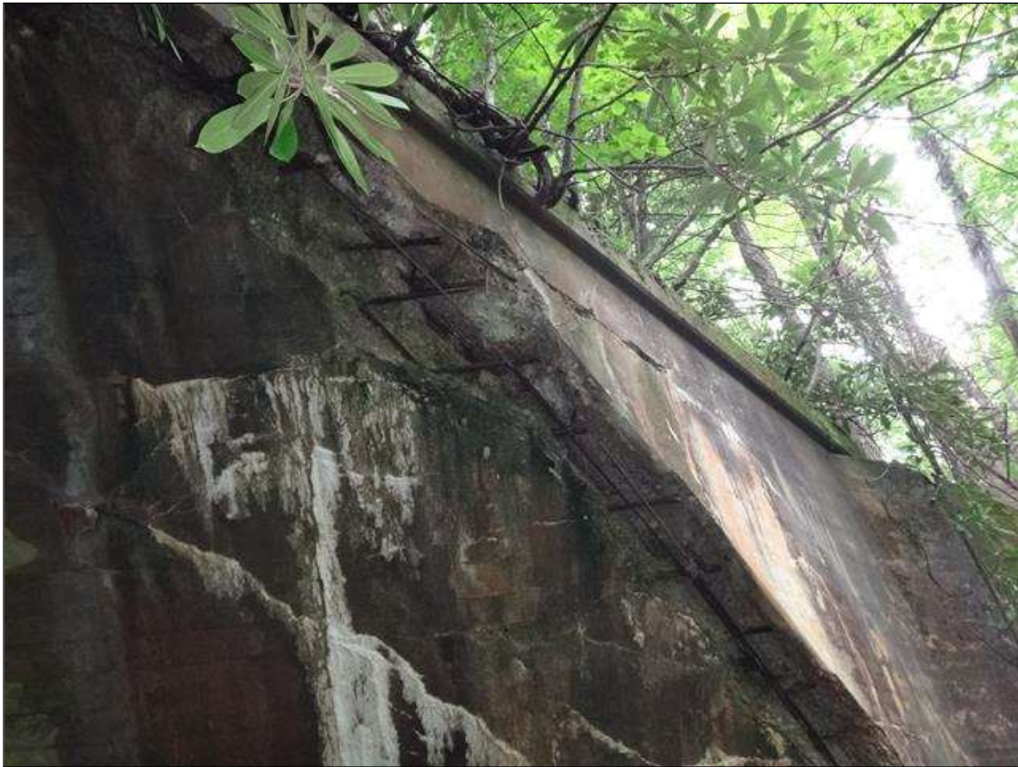
WEST HEADWALL ALONG SOUTHERN HALF OF SPANDREL, SPALL (18FT X 30IN X UP TO 16IN) WITH EXPOSED RUSTED REBAR
