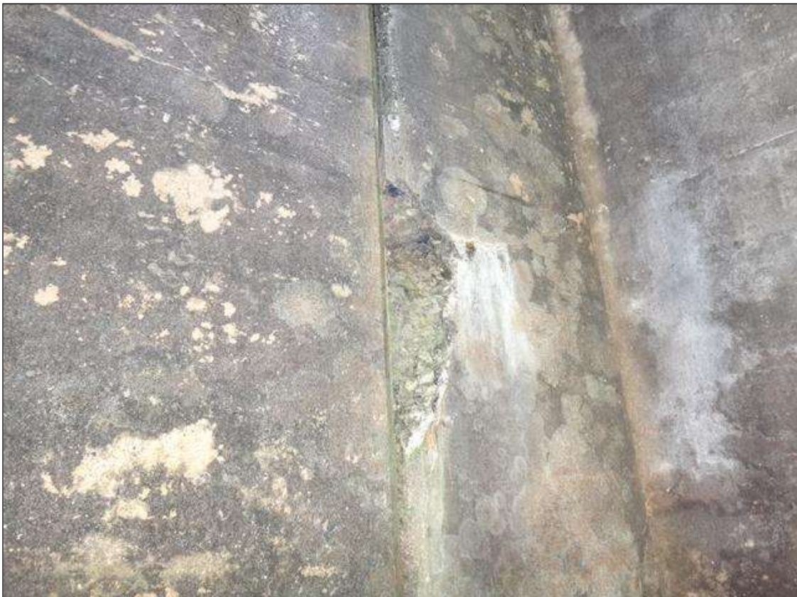
southeast wingwall, spall (4in x 1ft x up to 2in)
