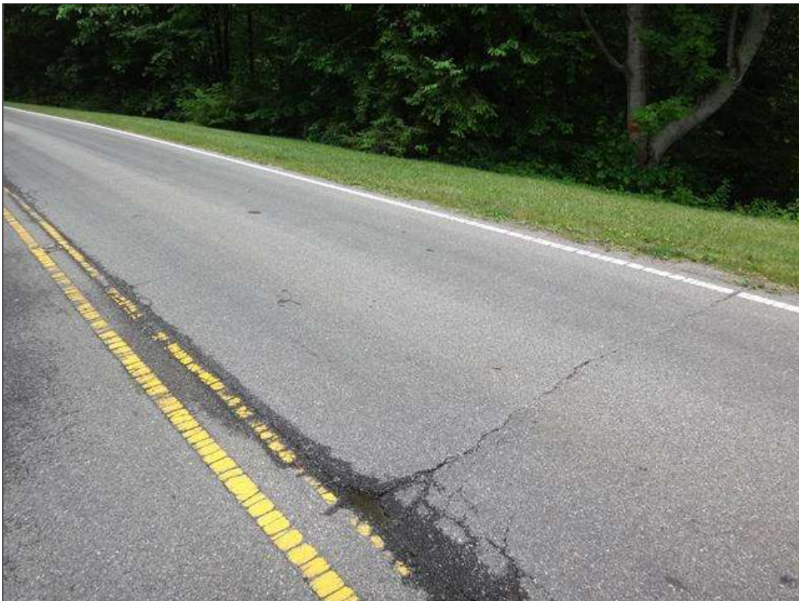
southbound lane over culvert, (5) transverse cracks (12ft x up to 1/8in)
