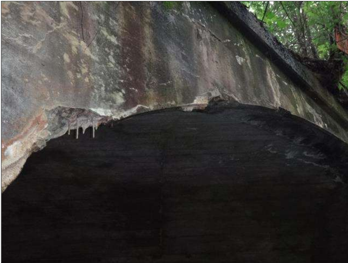
west headwall, (3) spalls (up to 24in x 6in x up to 5in)
