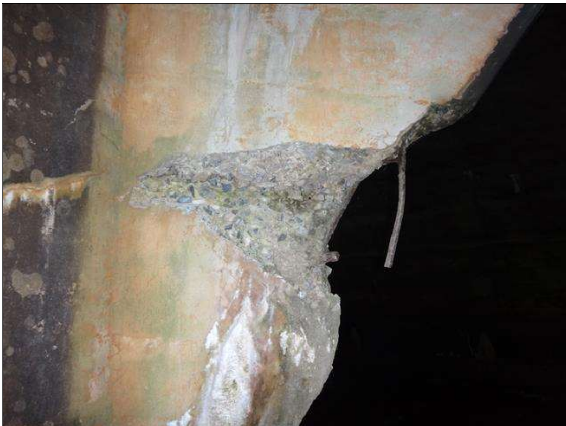
WEST HEADWALL AT NORTH WALL, SPALL (20IN X 14IN X 4-1/2IN) WITH EXPOSED RUSTED REBAR
