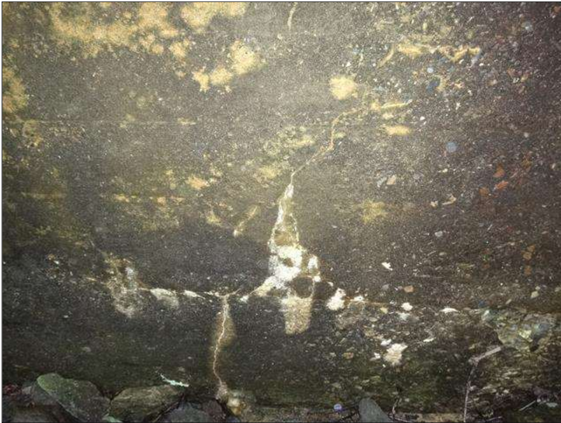
northeast wingwall at midpoint, vertical crack (5ft x hairline) with efflorescence
