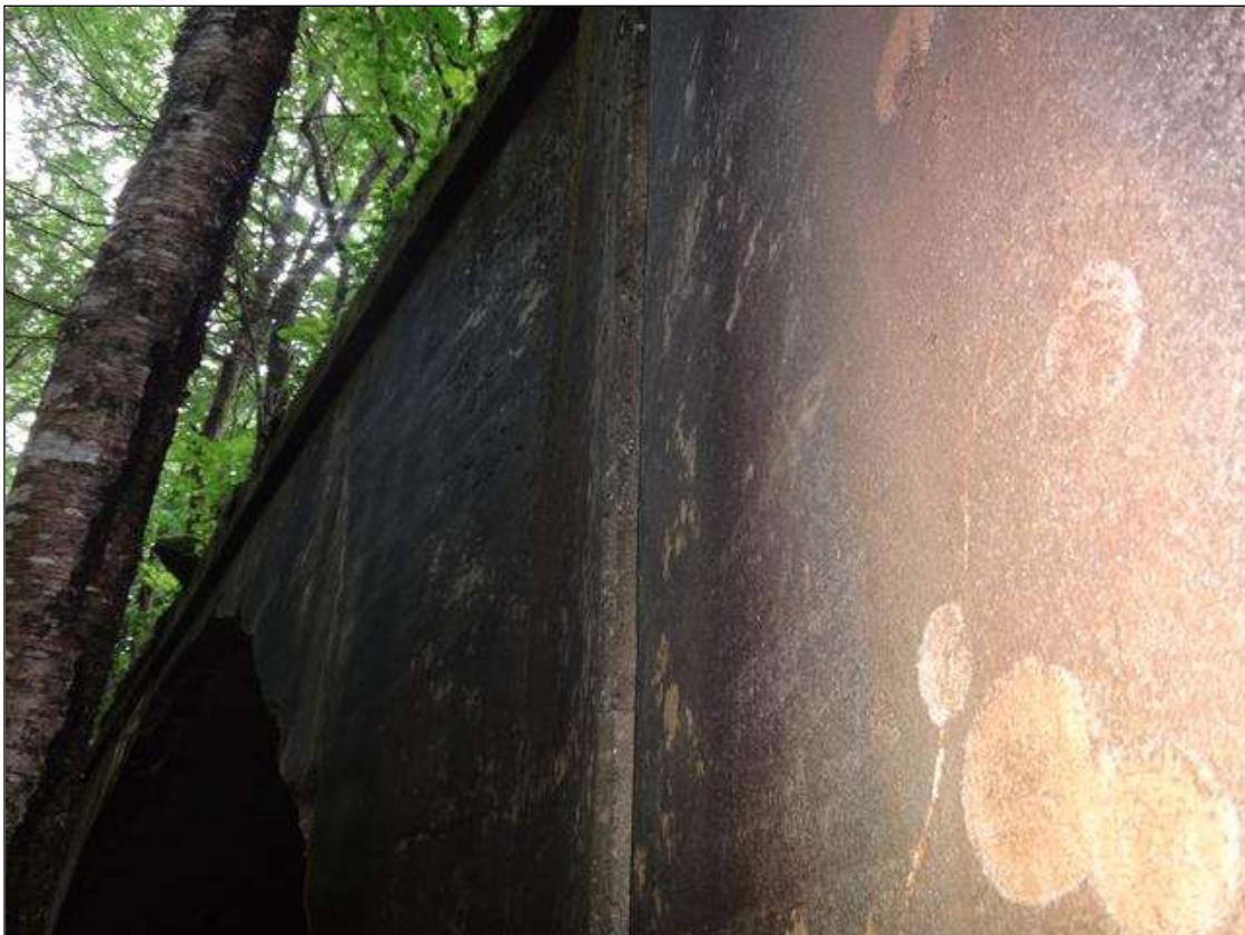
northeast wingwall, rotated west (up to 1-1/2in)
