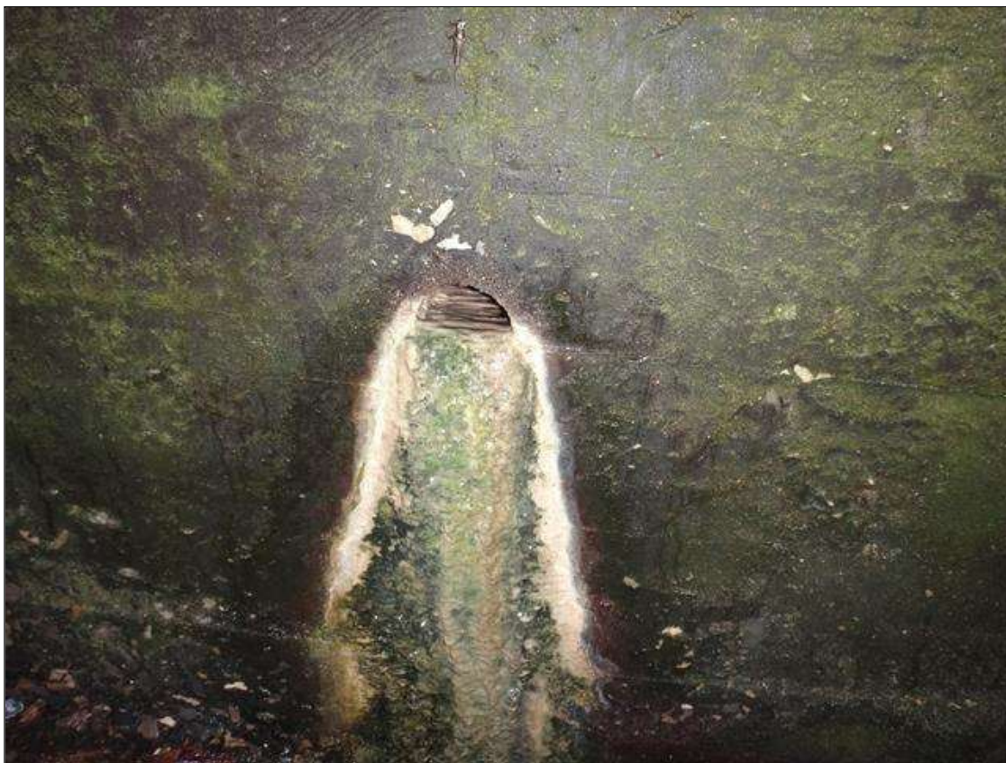
south wall at west end, partially clogged weep drain
