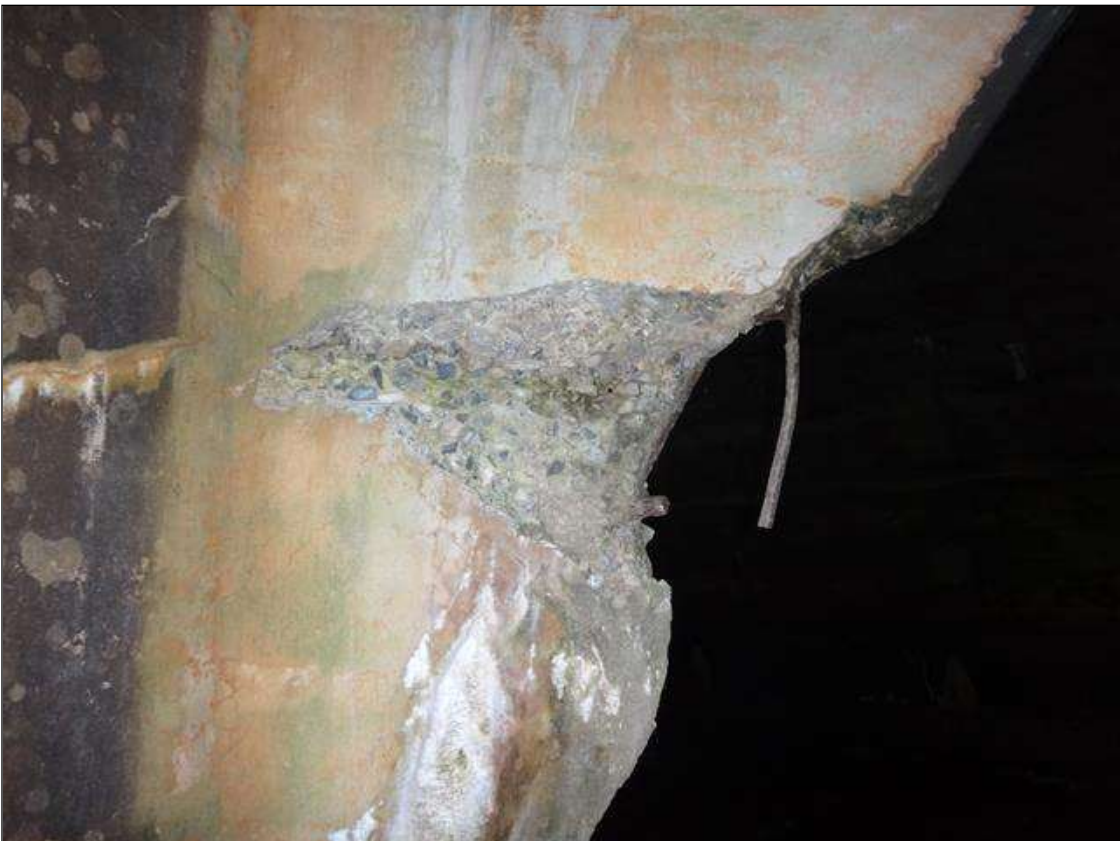
west headwall at north side, spall (20in x 14in x 4-1/2in) with exposed rusted rebar
