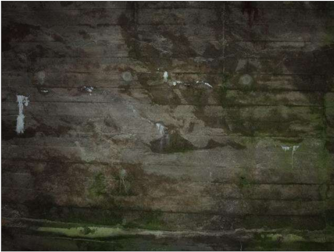
Barrel 1 Section 1: south wall near top at west end, (2) horizontal cracks (up to 30ft x up to 1/4in)
