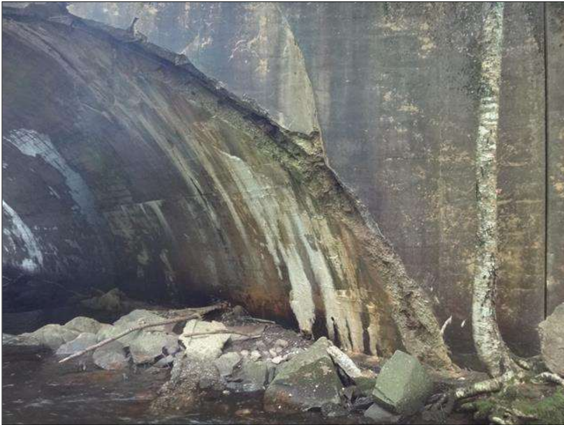
EAST HEADWALL ALONG NORTHERN HALF OF SPANDREL, SPALL (16FT X 18IN X UP TO 1FT) WITH EXPOSED RUSTED REBAR
