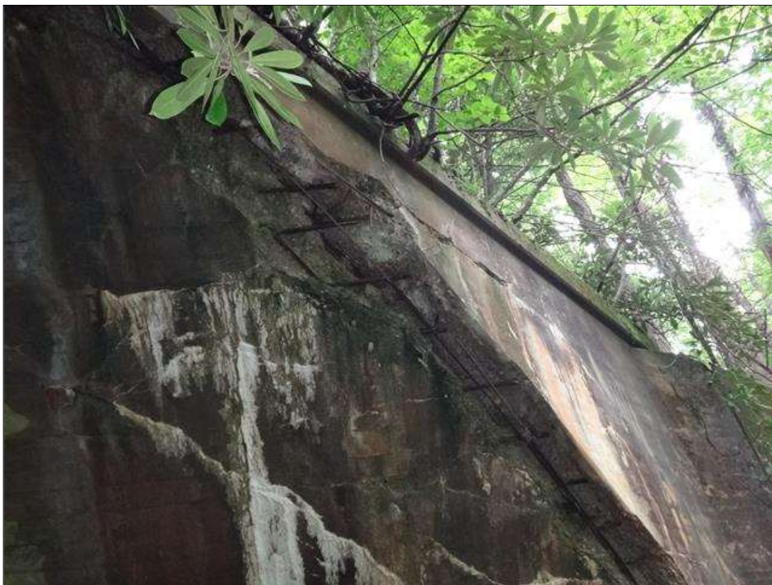
west headwall along southside, spall (18ft x 30in x up to 16in) with exposed rusted rebar
