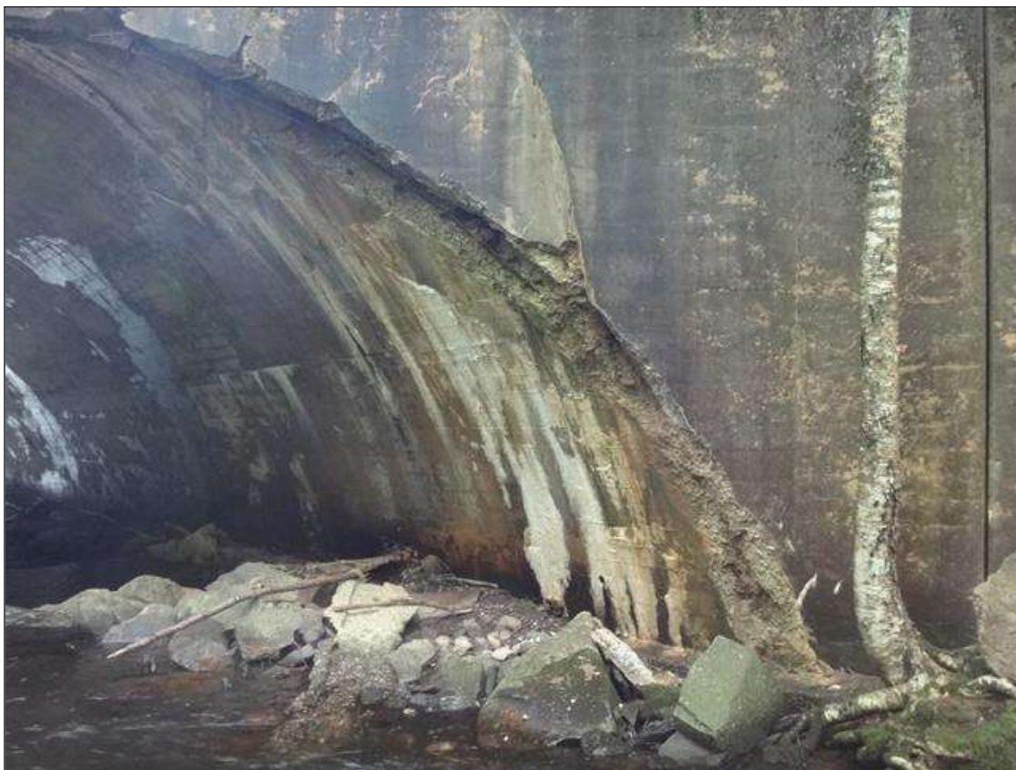
east headwall along northside, spall (16ft x 18in x up to 1ft) with exposed rusted rebar
