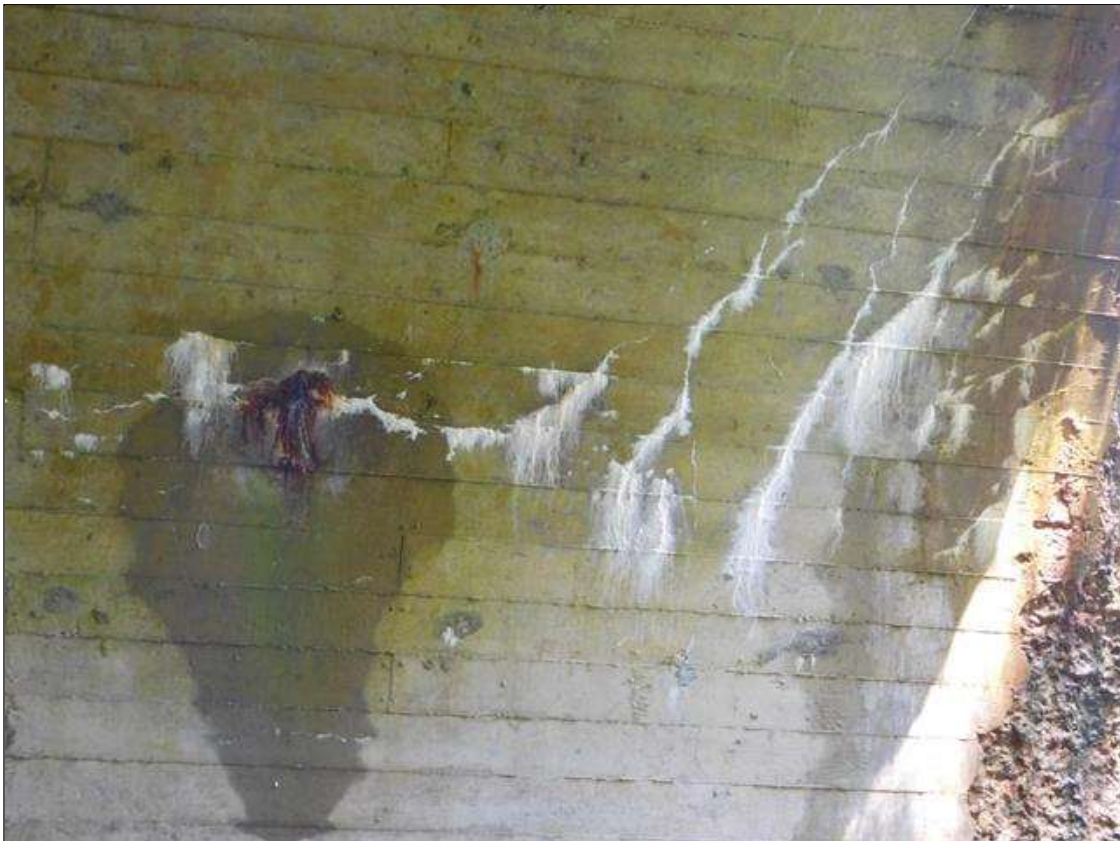
Barrel 1 Section 1: BARREL 1 HAS SCATTERED HORIZONTAL AND DIAGONAL CRACKS WITH HEAVY RUST STAINS AND EFFLO VISIBLE. LOCATED AT: 50' FROM UPSTREAM END.
