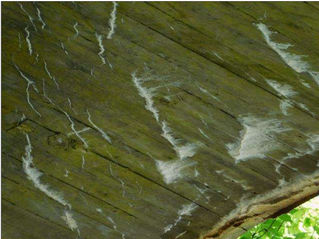
Barrel 2 Section 1: BARREL 2 INTERIOR WALL 1 AND 2 AND BOTTOM OF ARCH HAS SCATTERED DIAGONAL CRACKS WITH HEAVY EFFLO VISIBLE.
