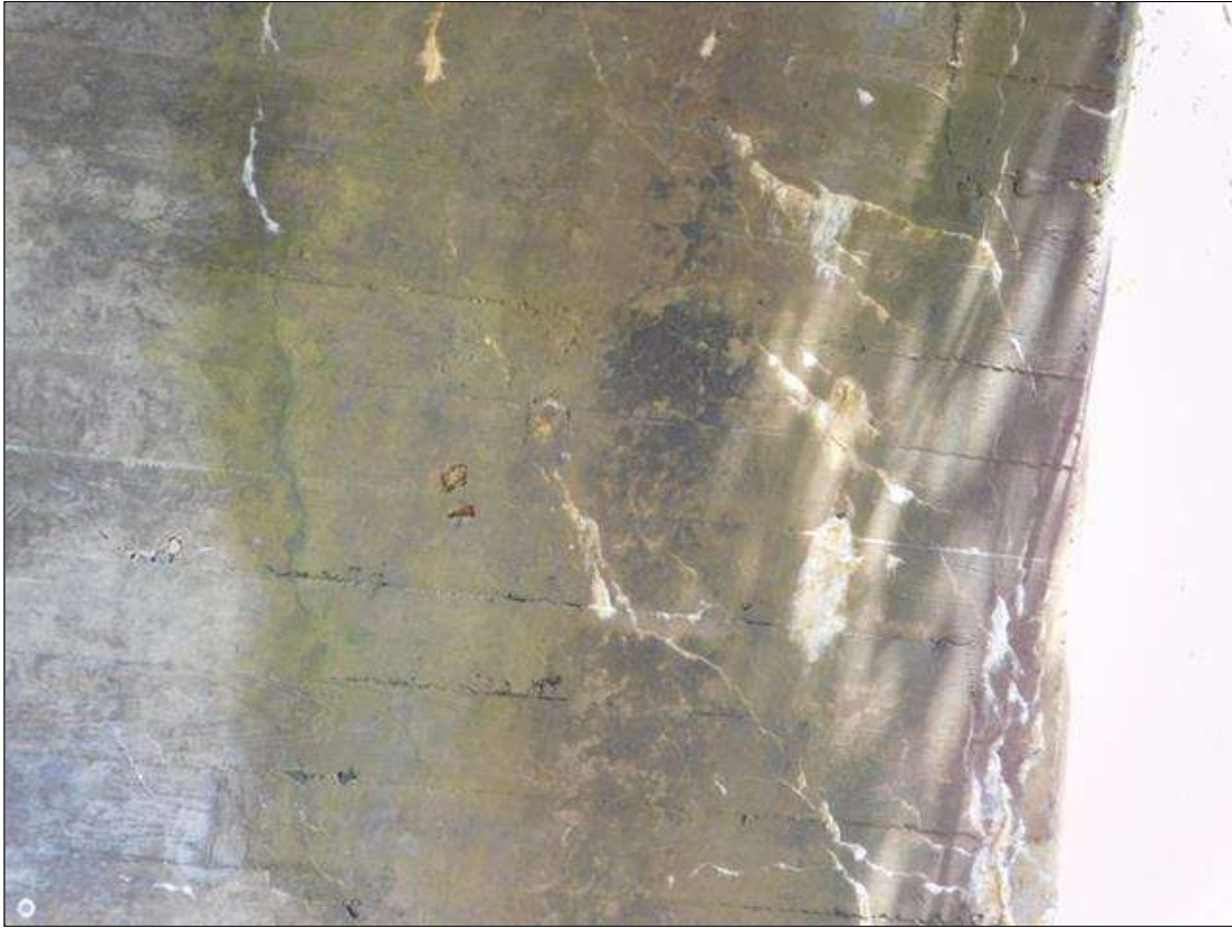
Barrel 2 Section 1: BARREL 2 INTERIOR WALL 1 AND 2 AND BOTTOM OF ARCH HAS SCATTERED DIAGONAL CRACKS WITH HEAVY EFFLO VISIBLE.
