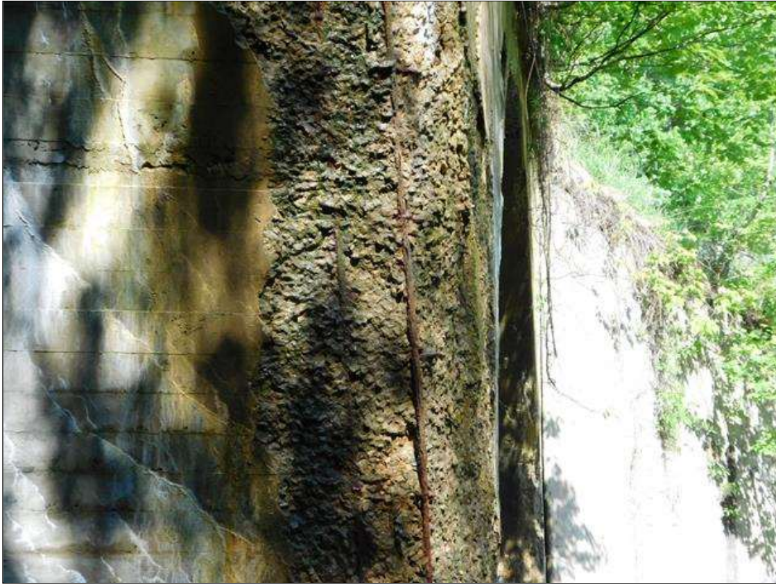
Barrel 1 Section 1: BARREL 1 DOWNSTREAM END HAS A LARGE AREA OF HEAVY DELAMINATION AND SPALL WITH REBAR EXPOSED. AREA IS: FULL CIRCUMFERENCE OF BARREL. A "PM" HAS BEEN ISSUED FOR THIS CONDITION.
