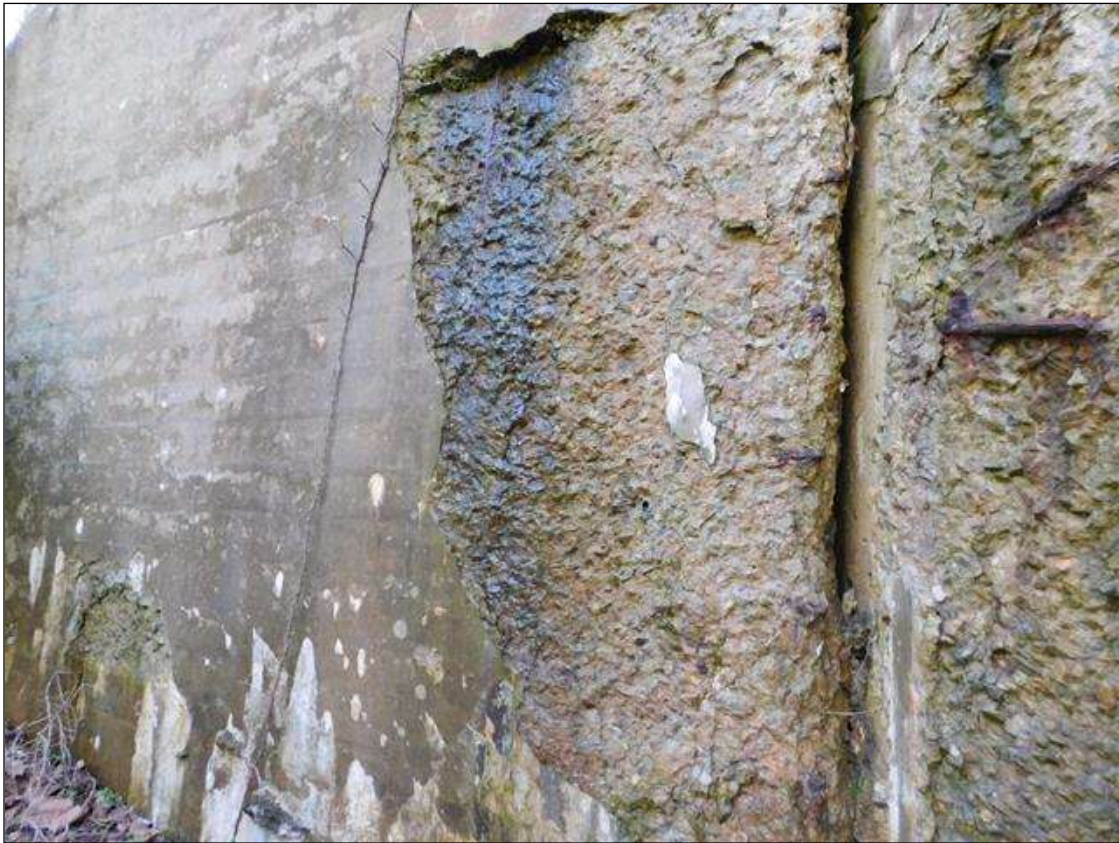
SOUTH EAST WINGWALL HEAVY SPALL & DELAMINATION WITH RE-BAR EXPOSED AREA IS 3' X 7' X 4" DEEP
