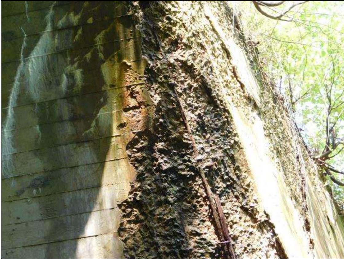
Barrel 1 Section 1: BARREL 1 DOWNSTREAM END HAS A LARGE AREA OF HEAVY DELAMINATION AND SPALL WITH REBAR EXPOSED. AREA IS: FULL CIRCUMFERENCE OF BARREL. A "PM" HAS BEEN ISSUED FOR THIS CONDITION.
