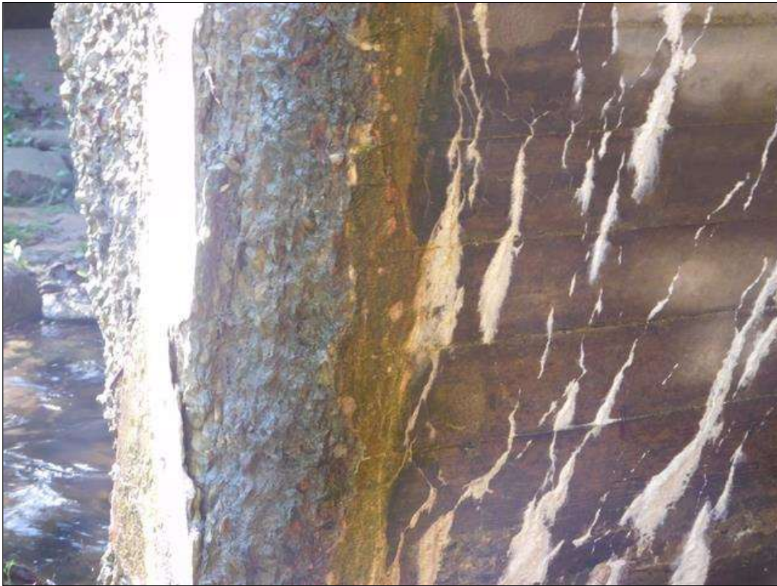
Barrel 2 Section 1: BARREL 2 DOWNSTREAM END OF BOTH INTERIOR WALLS AND BOTTOM OF ARCH HAS SCATTERED AREAS OF HEAVY SPALL AND DELAMINATION WITH REBAR EXPOSED. A "PM" HAS BEEN ISSUED FOR THIS CONDITION.
