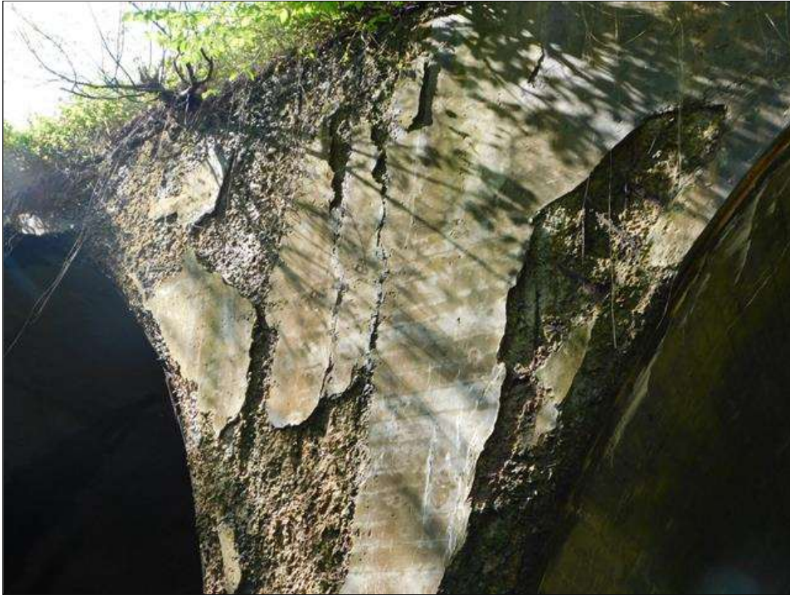
EAST HEADWALL HAS A LARGE AREA OF HEAVY SPALL AND DELAMINATION WITH REBAR AND EFFLO EXPOSED. AREA IS: 20' x 45'. TOTAL MAINTENANCE QUANTITY IS: 900 SQ FEET. A "PM" HAS BEEN ISSUED FOR THIS CONDITION.
