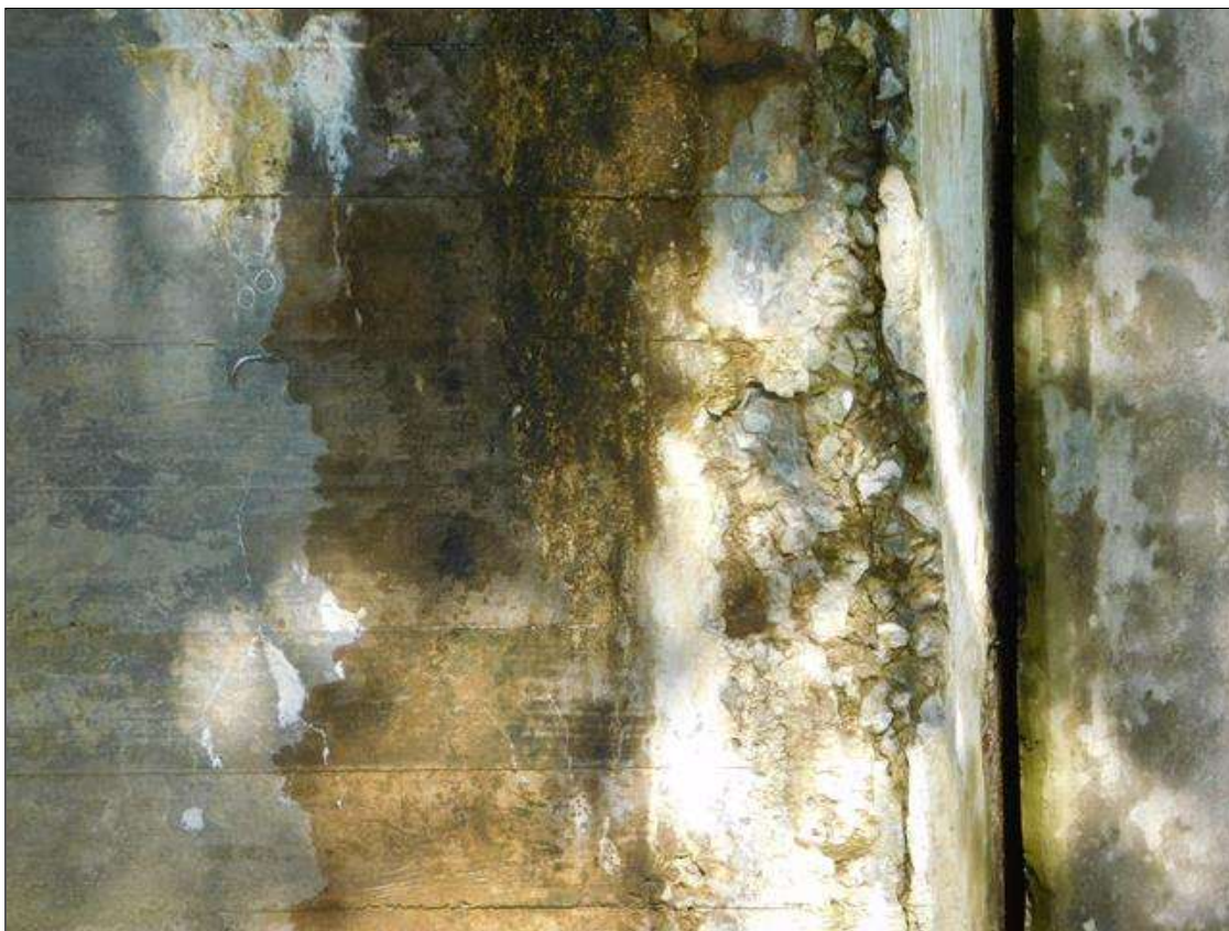
Barrel 2 Section 1: BARREL 2 DOWNSTREAM END OF BOTH INTERIOR WALLS AND BOTTOM OF ARCH HAS SCATTERED AREAS OF HEAVY SPALL AND DELAMINATION WITH REBAR EXPOSED. A "PM" HAS BEEN ISSUED FOR THIS CONDITION.
