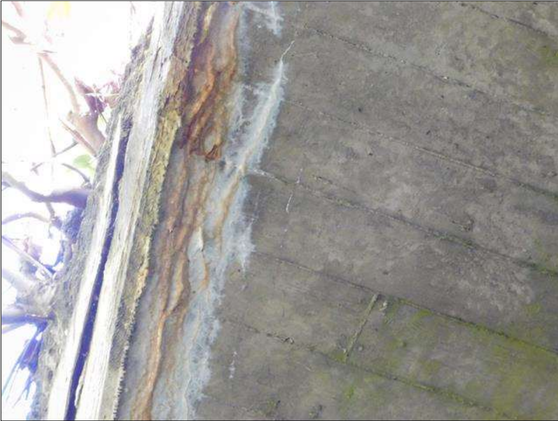
Barrel 1 Section 1: BARREL 1 BOTTOM OF TOP SLAB AND NORTHWEST CORNER. HAS A LARGE AREA THAT IS CRACKED/DELAMINATED AND SPALLED WITH REBAR AND HEAVY EFFLO VISIBLE. A "PM" HAS BEEN ISSUED FOR THIS CONDITION.
