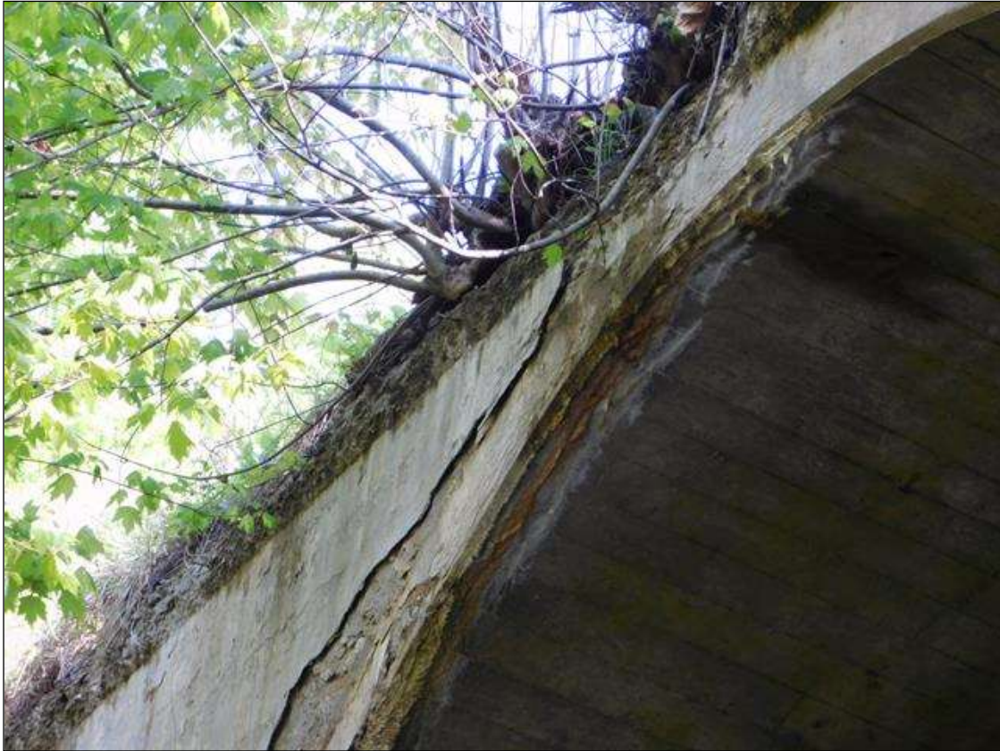
WEST HEADWALL HAS A LARGE AREA THAT IS CRACKED, SPALLED & DELAMINATED WITH RE-BAR & EFFLO EXPOSED. AREA IS 16' X 40' X 6" DEEP.
