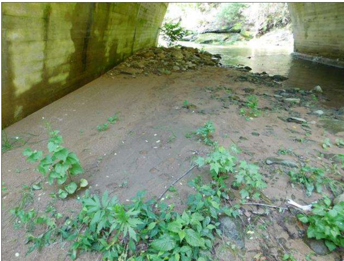
EXCESS SAND AND ROCKS IN BARREL 1. AREA IS: 15' x 56' x UP TO 3' HIGH. TOTAL MAINTENANCE QUANTITY IS 840' SQ FEET
