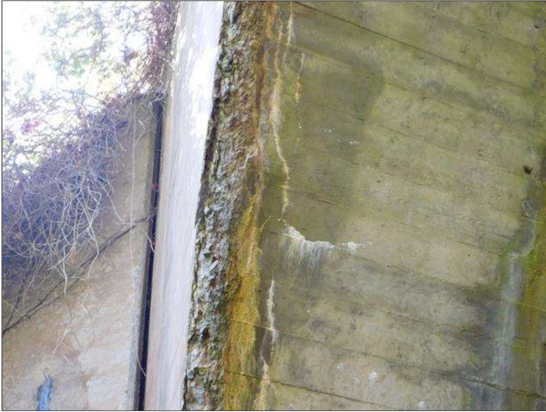
Barrel 1 Section 1: BARREL 1 DOWNSTREAM END HAS A LARGE AREA OF HEAVY DELAMINATION AND SPALL WITH REBAR EXPOSED. AREA IS: FULL CIRCUMFERENCE OF BARREL. A "PM" HAS BEEN ISSUED FOR THIS CONDITION.
