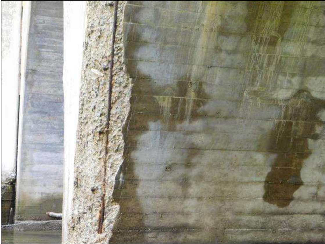
Barrel 1 Section 1: BARREL 1 BOTTOM OF TOP SLAB AND NORTHWEST CORNER. HAS A LARGE AREA THAT IS CRACKED/DELAMINATED AND SPALLED WITH REBAR AND HEAVY EFFLO VISIBLE. A "PM" HAS BEEN ISSUED FOR THIS CONDITION.
