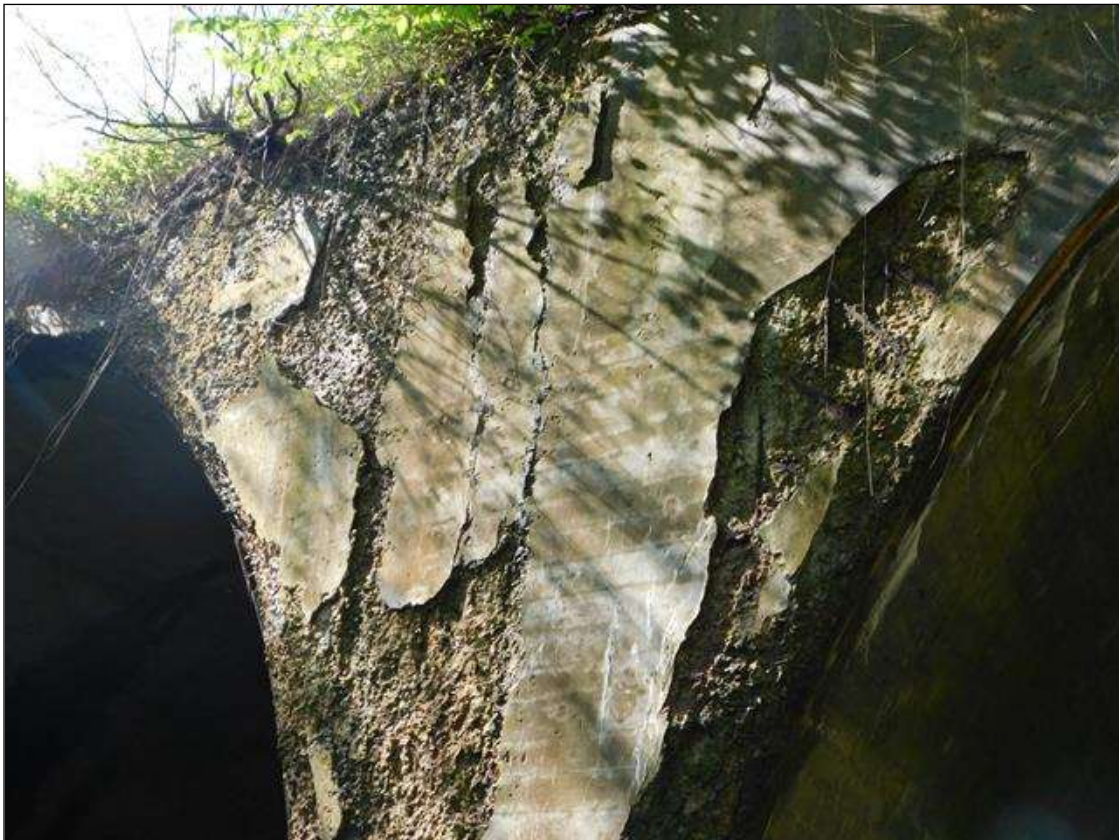
EAST HEADWALL HAS A LARGE AREA WITH HEAVY SPALL & DELAMINATION WITH RE-BAR & EFFLO EXPOSED. AREA IS 20' X 45' X 3" DEEP.
