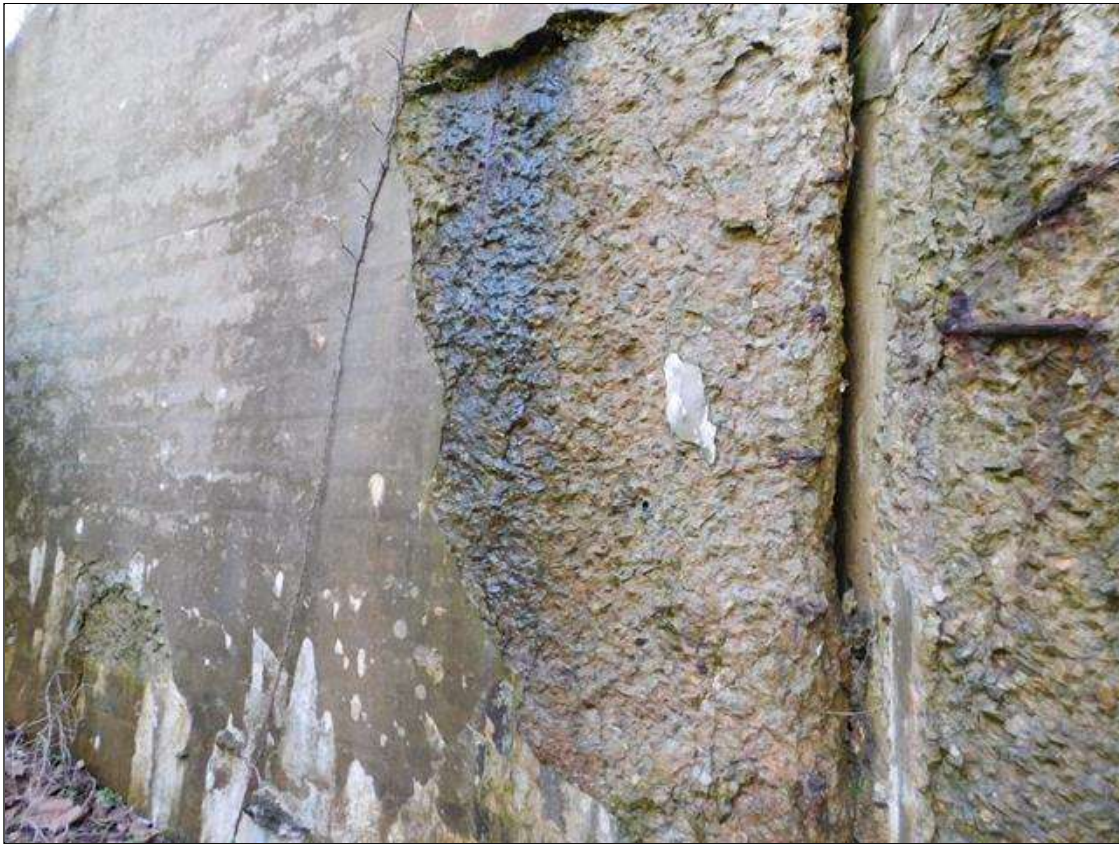
SOUTHEAST WING WALL HAS A AREA OF HEAVY SPALL AND DELAMINATION WITH REBAR EXPOSED. AREA IS: 3' x 7' x 4" DEEP. A "PM" HAS BEEN ISSUED FOR THIS CONDITION.
