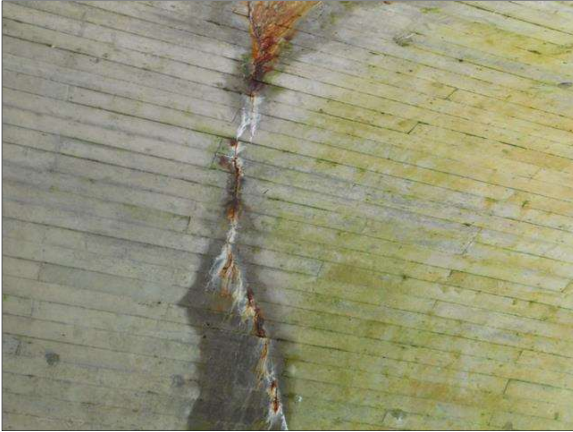
Barrel 1 Section 1: BARREL 1 HAS 2 CRACKS WITH HEAVY RUST STAINS AND EFFLO VISIBLE IN BOTTOM OF TOP SLAB AND DOWN BOTH INTERIOR WALLS. LOCATED AT: 27' AND 39' FROM UPSTREAM END.
