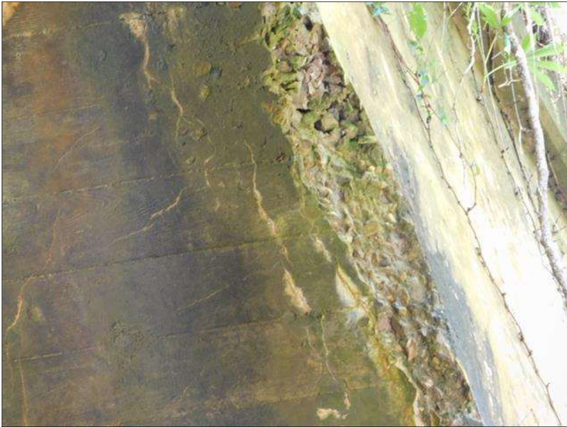
Barrel 2 Section 1: BARREL 2 DOWNSTREAM END OF BOTH INTERIOR WALLS AND BOTTOM OF ARCH HAS SCATTERED AREAS OF HEAVY SPALL AND DELAMINATION WITH REBAR EXPOSED. A "PM" HAS BEEN ISSUED FOR THIS CONDITION.
