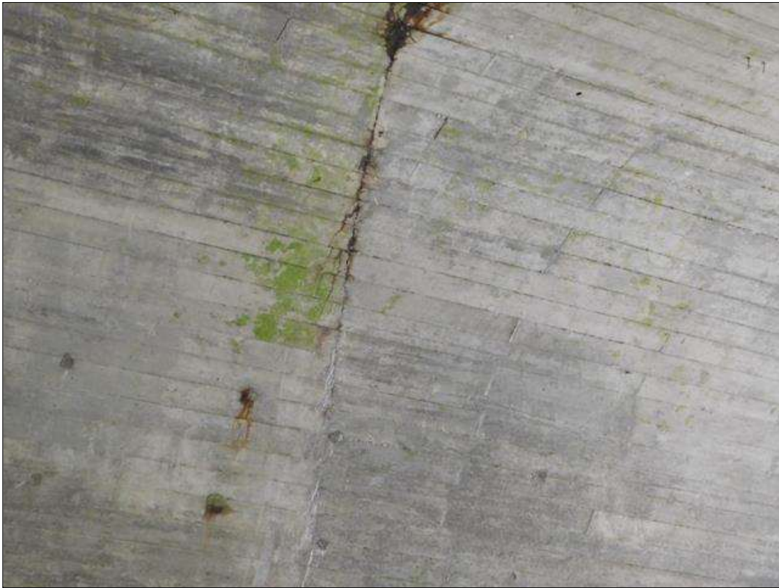
Barrel 2 Section 1: BARREL 2 INTERIOR WALL 2 AND BOTTOM OF ARCH HAS A CRACK WITH HEAVY RUST STAINS AND SOME EFFLO VISIBLE. LOCATED AT: 26' FROM UPSTREAM END.
