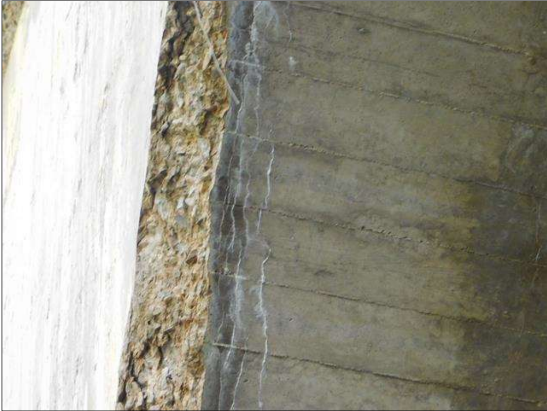
Barrel 1 Section 1: BARREL 1 BOTTOM OF TOP SLAB AND NORTHWEST CORNER. HAS A LARGE AREA THAT IS CRACKED/DELAMINATED AND SPALLED WITH REBAR AND HEAVY EFFLO VISIBLE. A "PM" HAS BEEN ISSUED FOR THIS CONDITION.
