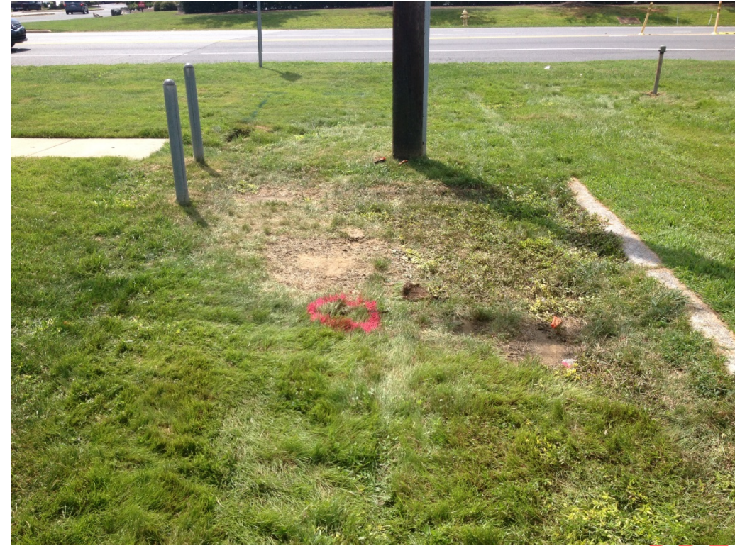
D. Photo of circled location of 6-inch pipe found at south end of property, looking west.
