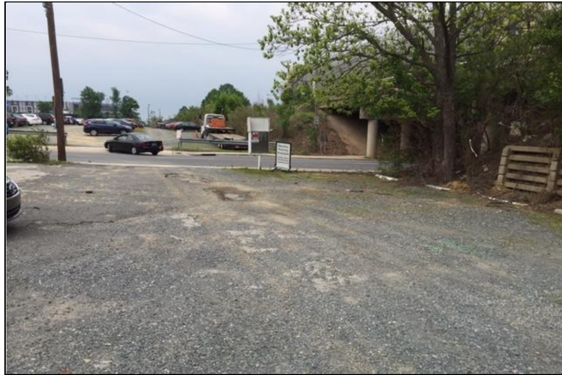
PHOTOGRAPH NO. 1: EAST APPROACH TO END BENT NO. 1 ON -S2- ALIGNMENT, LOOKING WEST
