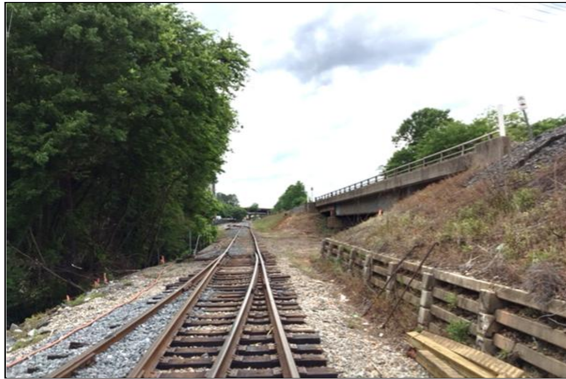
PHOTOGRAPH NO. 1: EAST APPROACH TO END BENT NO. 1 ON -A1- ALIGNMENT, LOOKING WEST
