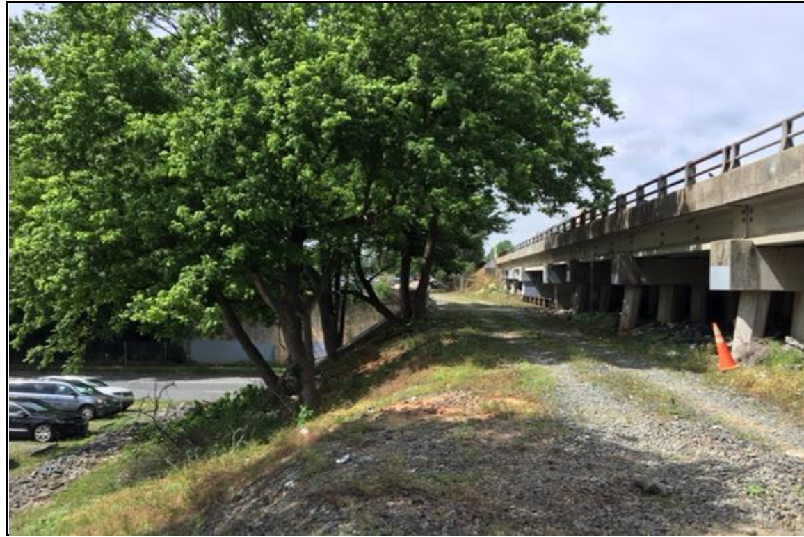
PHOTOGRAPH NO. 1: EAST APPROACH TO END BENT NO. 1 ON -S1- ALIGNMENT, LOOKING WEST
