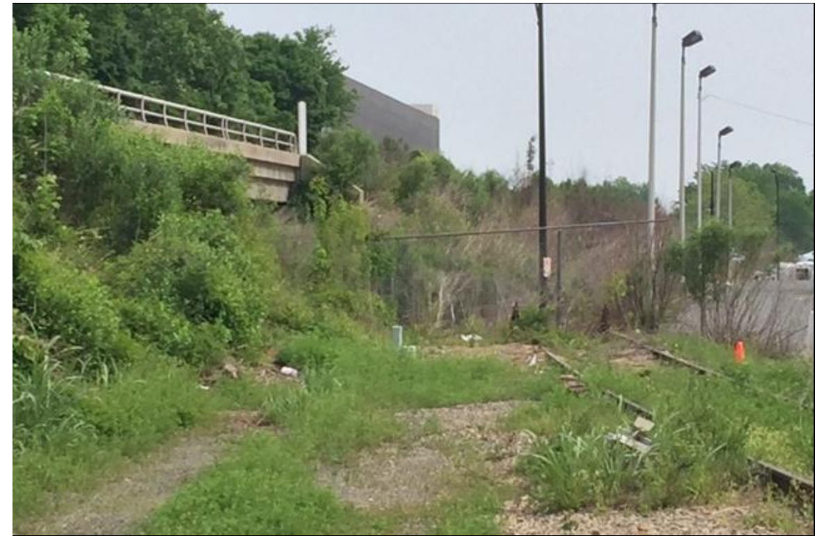
PHOTOGRAPH NO. 4: WEST APPROACH TO END BENT NO.2 ON -S2- ALIGNMENT, LOOKING EAST
