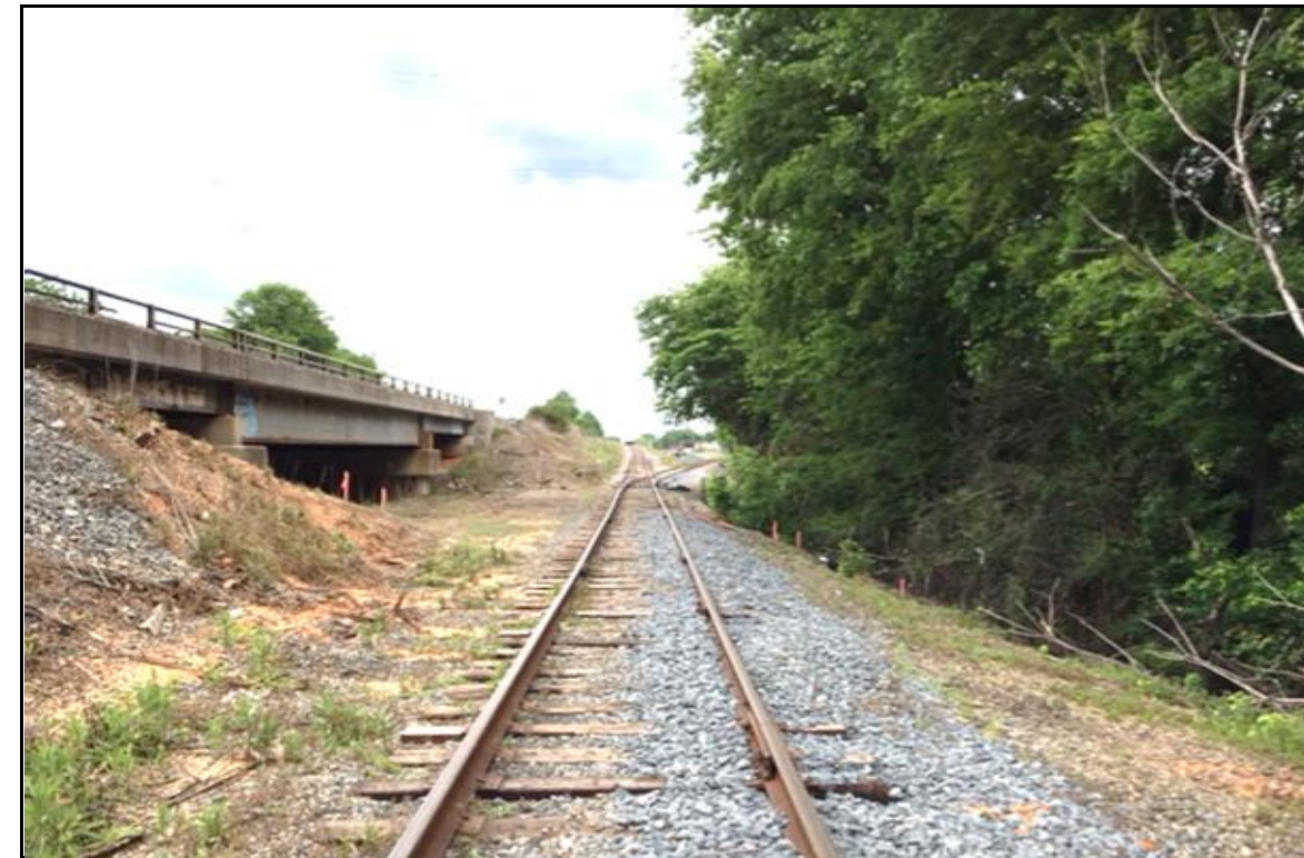
PHOTOGRAPH NO. 4: WEST APPROACH TO END BENT NO.2 ON -A1- ALIGNMENT, LOOKING EAST
