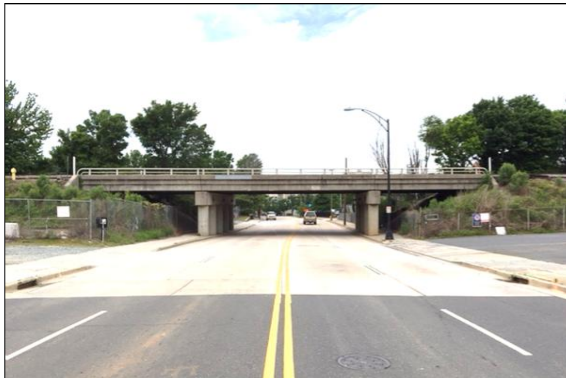
PHOTOGRAPH NO. 2: ON WEST 4th STREET (-Y-), SOUTHEAST OF -S1- ALIGNMENT, LOOKING NORTHWEST
