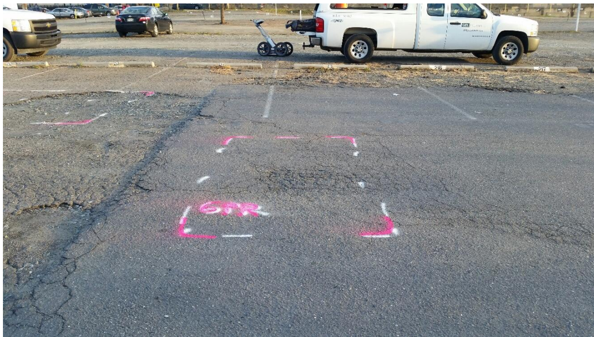
Photo 9: Showing GPR anomaly and "Possible UST" (upper left) in Parcel 4B.
