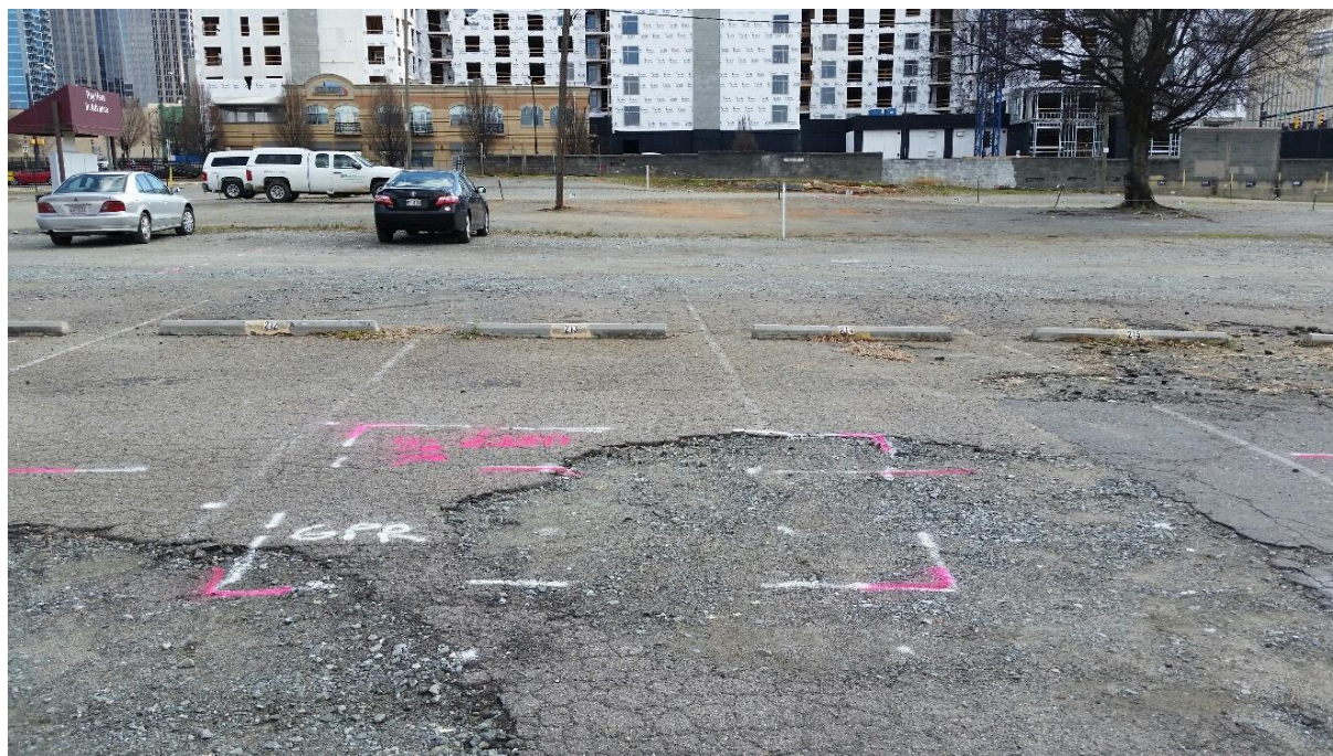
Photo 12: Showing "Possible UST" in Parcel 4B.
