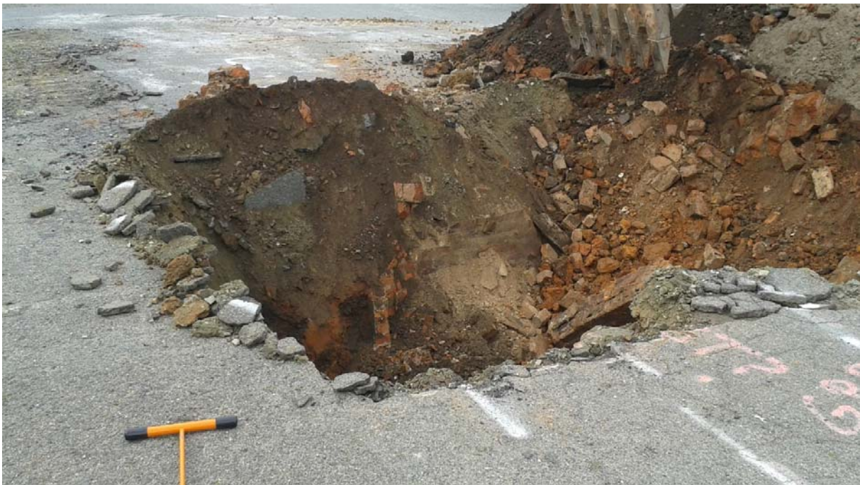
Photograph 2: View of brick debris in excavation.
