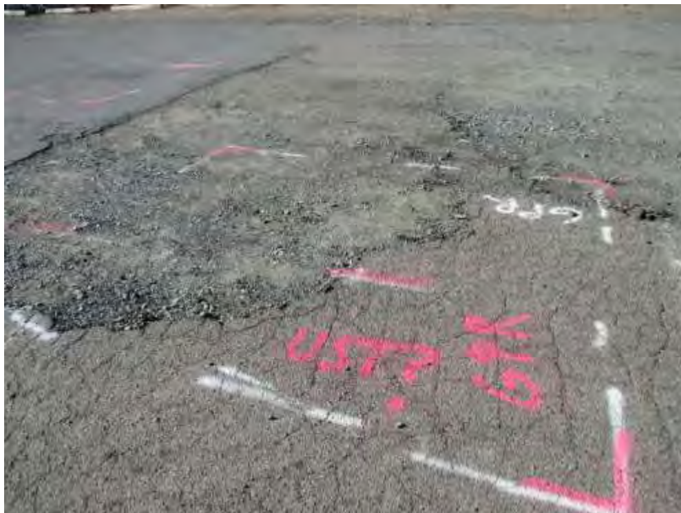
Photo 6 View of typical GPR/EM markings indicating possible UST in the western portion of site.
