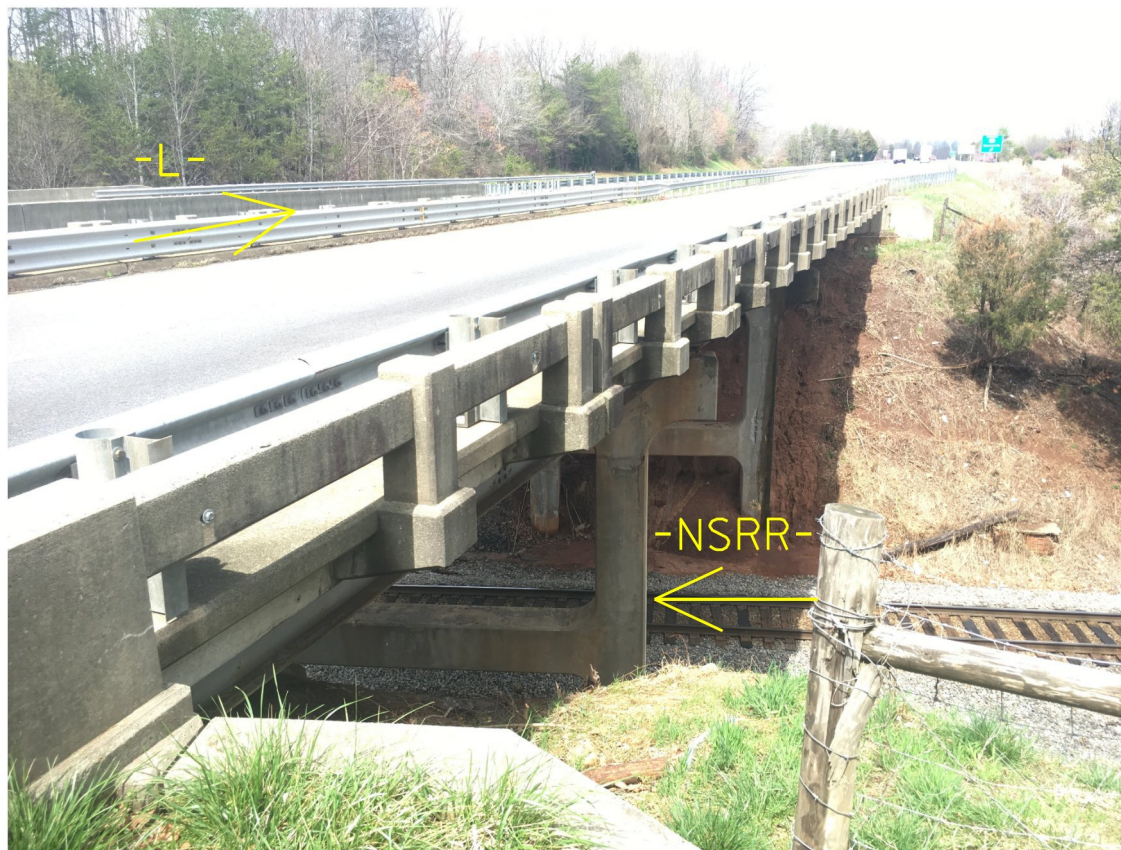
Photo No. 2: View at End Bent 1 looking north (upstation) on -L- (US 220 Bypass) over the Norfolk Southern RailWay
