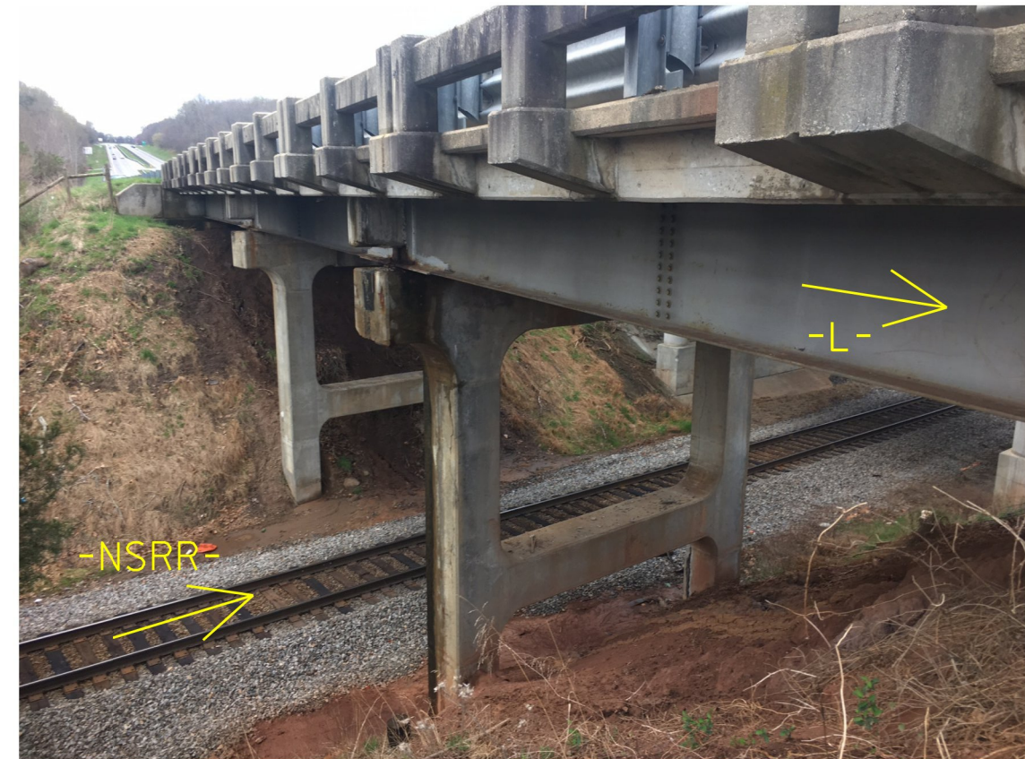
Photo No. 3: View at End Bent 2 looking south (downstation) on -L- (US 220 Bypass) over the Norfolk Southern RailWay
