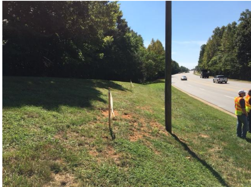
Photograph No. 1: Right of the I-85 Bypass -L- alignment, looking South along proposed End Bent No. 1
