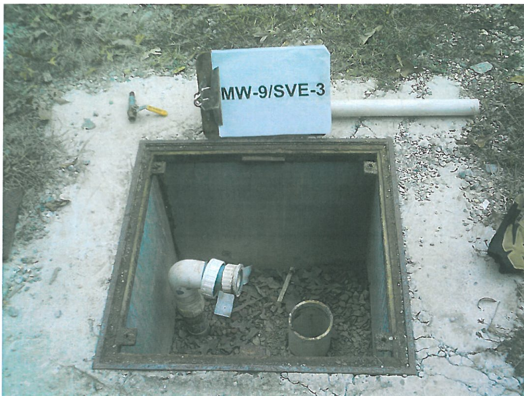
Photograph 7: Typical remediation system well prior to abandonment
