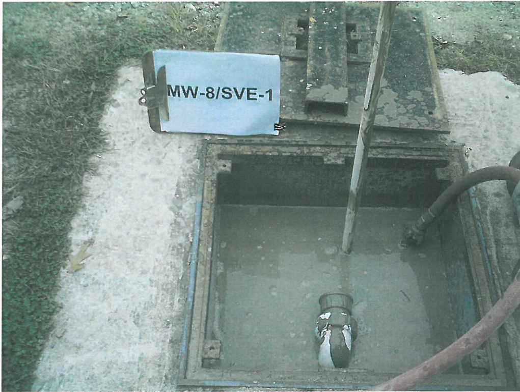
Photograph 9: Typical remediation system well after abandonment
