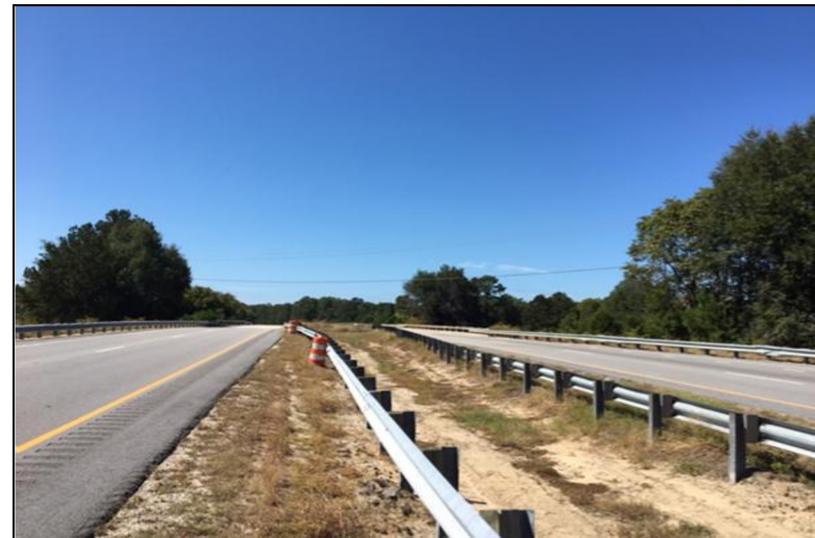
PHOTOGRAPH NO. 4: EAST APPROACH TO END BENT NO.2 BETWEEN -L1- AND -L2- ALIGNMENTS, LOOKING WEST
