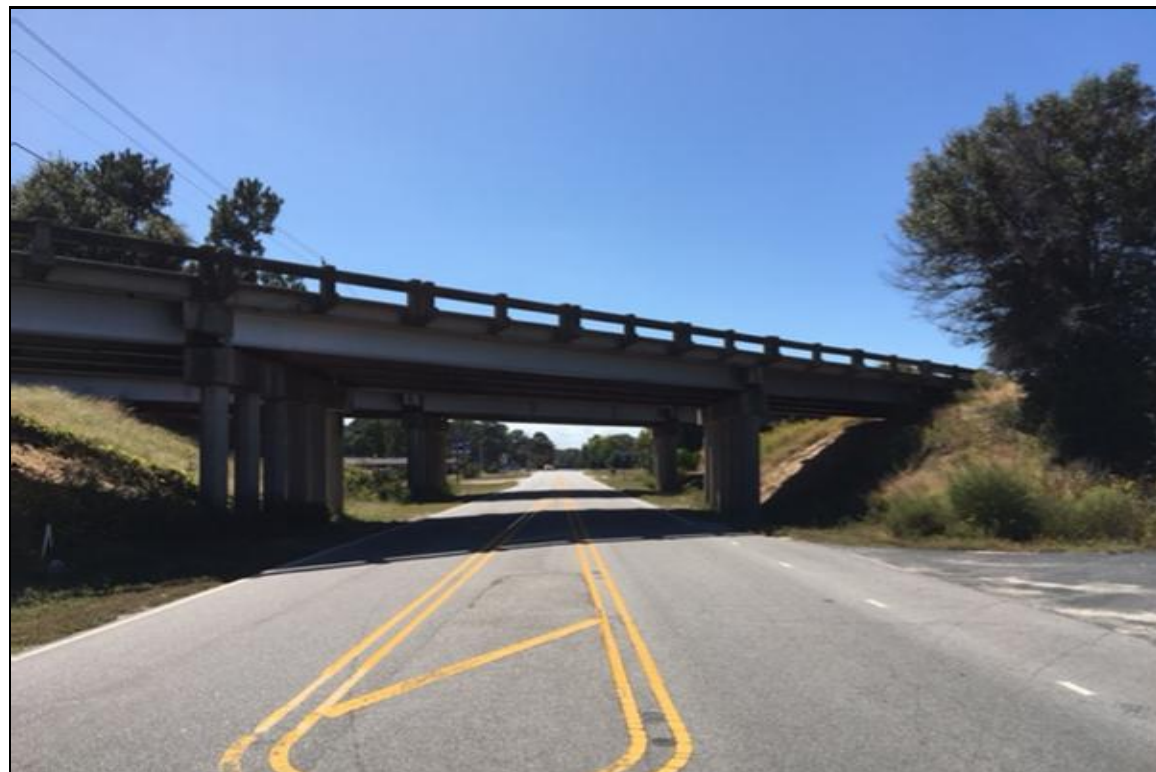
PHOTOGRAPH NO. 2: ON -Y- ALIGNMENT, NORTH OF -L1- AND -L2- ALIGNMENTS, LOOKING SOUTH
