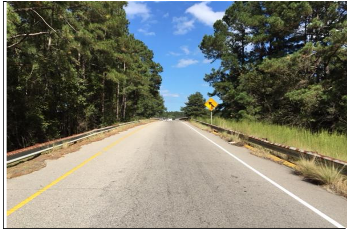
PHOTOGRAPH NO. 1: WEST APPROACH TO END BENT NO. 1 ON -L- ALIGNMENT, LOOKING EAST
