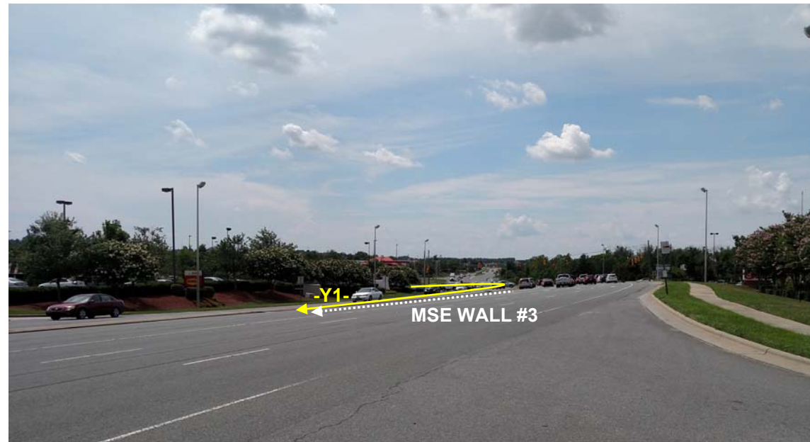
Photograph No. 1: Looking west at -L- (Concord Mills Blvd.) and walls on -Y1-
