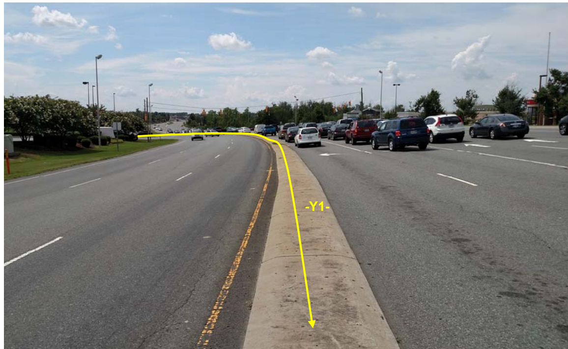
Photograph No. 2: On -L- (Concord Mills Blvd.) looking northwest towards End Bent 2
