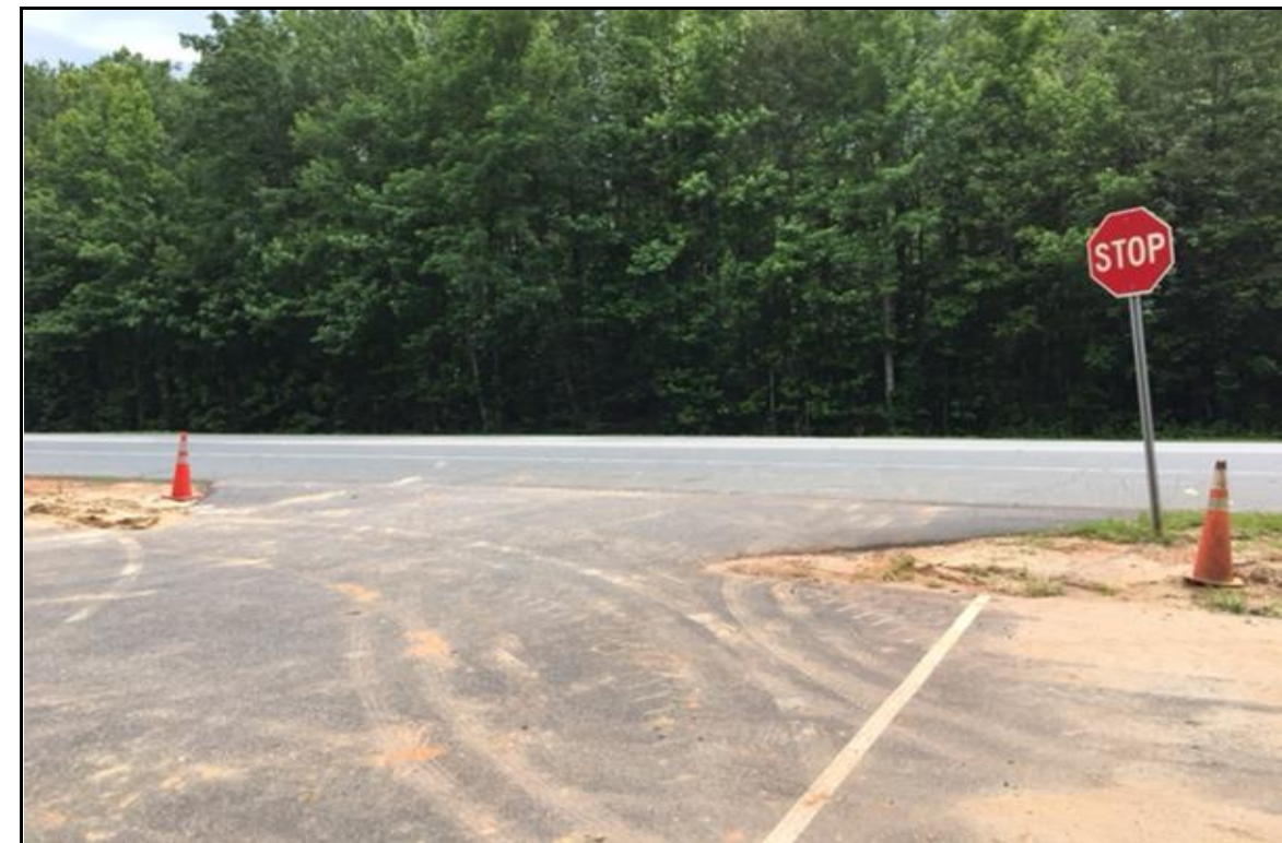
PHOTOGRAPH NO. 4: NORTH APPROACH TO END BENT NO.2 ON -RP_E- ALIGNMENT, LOOKING SOUTH
