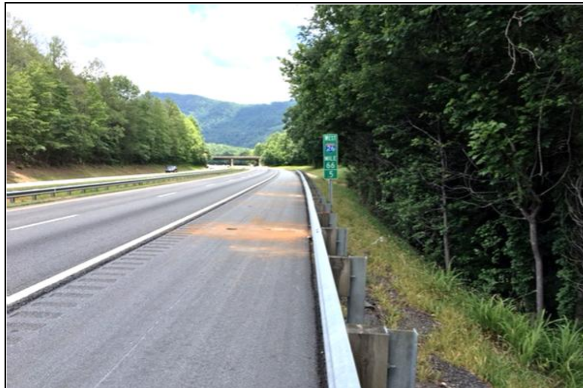
PHOTOGRAPH NO. 2: ON I-26 (WBL) -EL- ALIGNMENT OUTSIDE SHOULDER, EAST OF -RP_F- ALIGNMENT, LOOKING WEST
