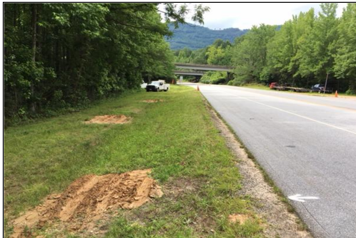
PHOTOGRAPH NO. 2: ON -E_CONN_REV-ALIGNMENT LEFT SHOULDER, SOUTH OF -RP_E- ALIGNMENT, LOOKING NORTH
