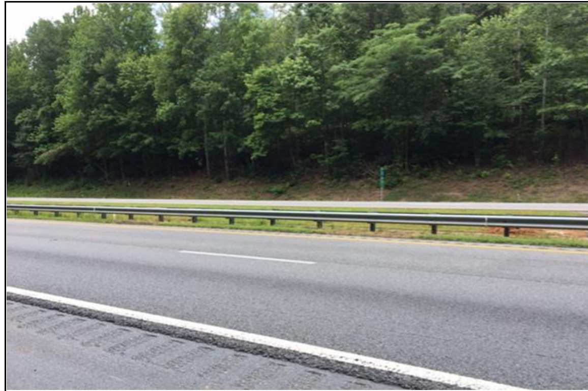
PHOTOGRAPH NO. 1: NORTH APPROACH TO END BENT NO. 1 ON -RP_F- ALIGNMENT, LOOKING SOUTH
