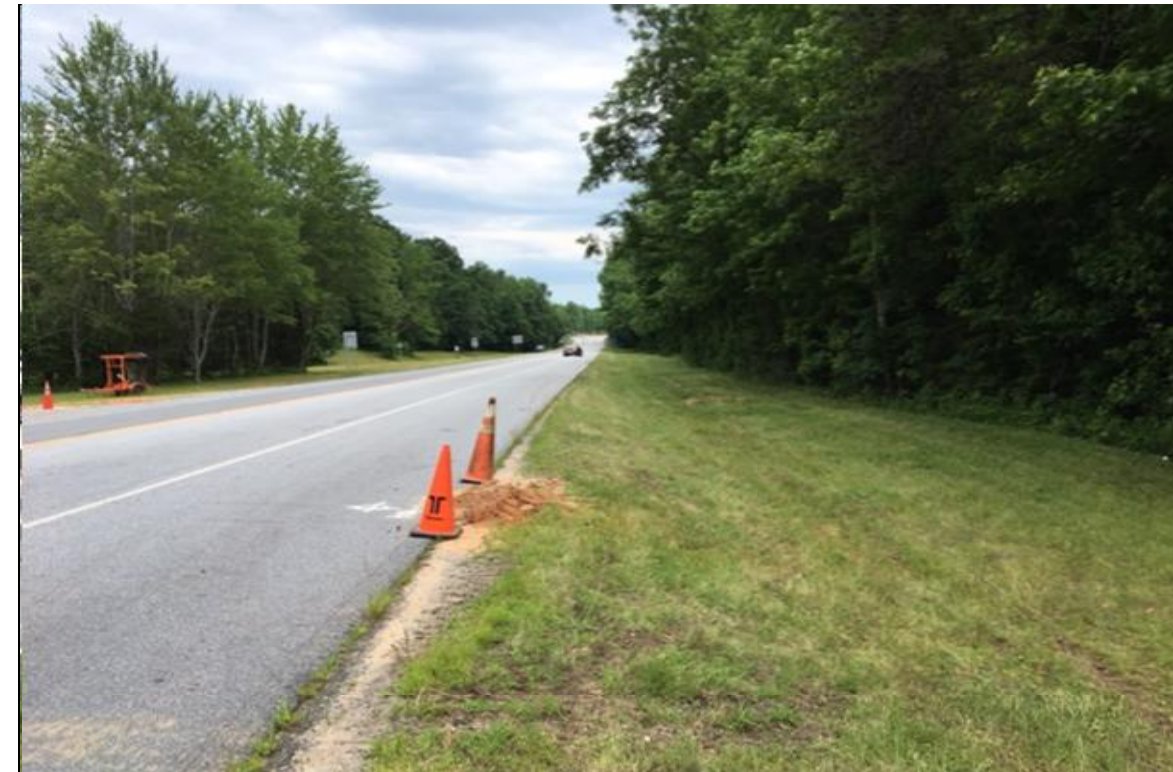
PHOTOGRAPH NO. 3: ON -E_CONN_REV-ALIGNMENT RIGHT SHOULDER, NORTH OF -RP_E- ALIGNMENT, LOOKING SOUTH
