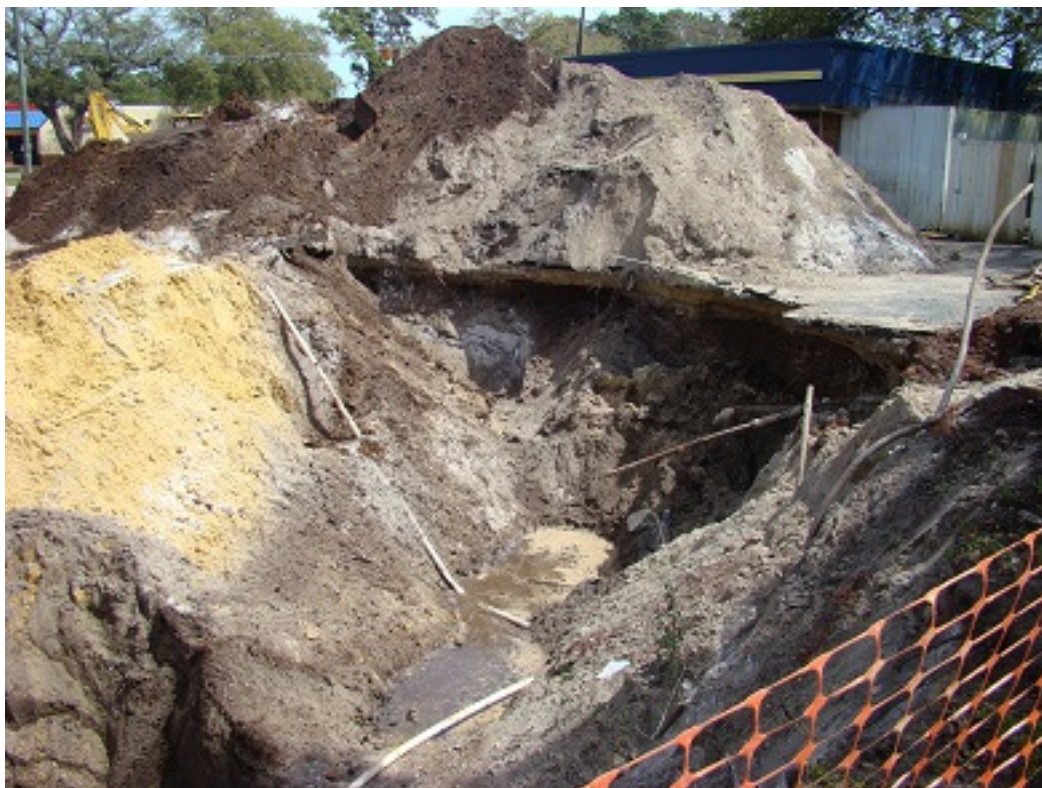
Photo 14: Begin backfilling, note steel UST vent pipes to the right, remedial system PVC pipe, and ground- water, facing southeast
