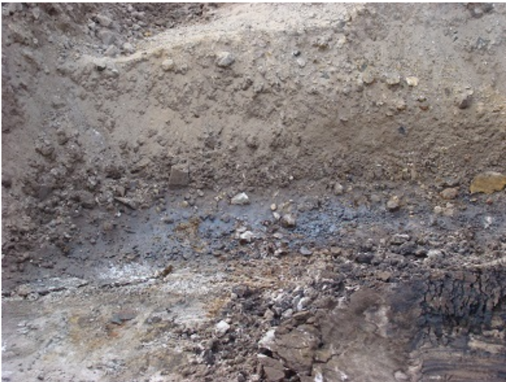
Photo 6: Stained soil beneath UST #3
