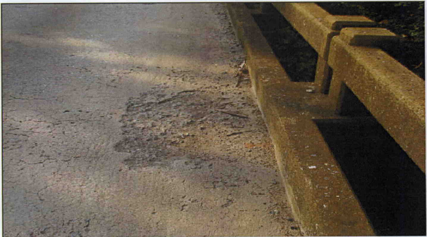
DECK DELAMINATION ALONG WEST CURB IN SPAN 2
