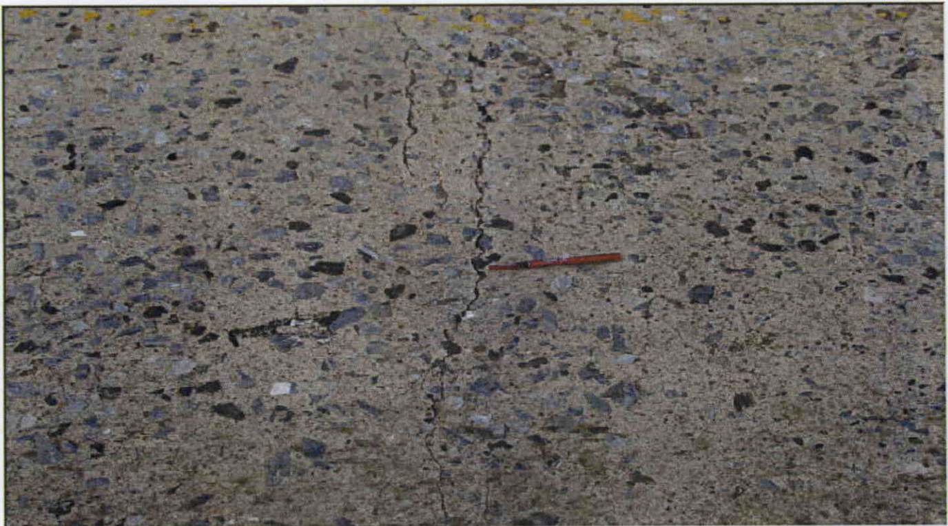
TRANSVERSE DECK CRACK AT MIDSPAN OF SPAN 1
