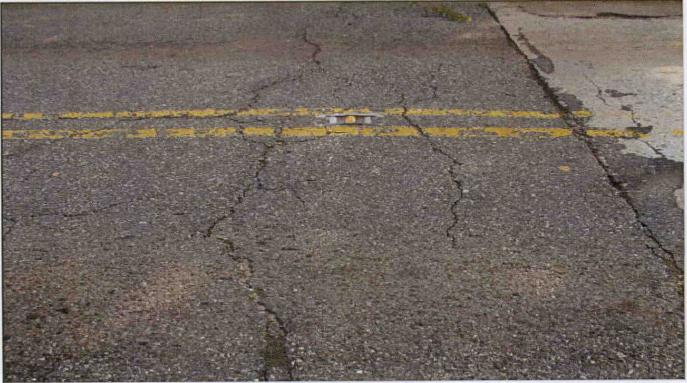
CRACKING ALONG NORTH APPROACH
