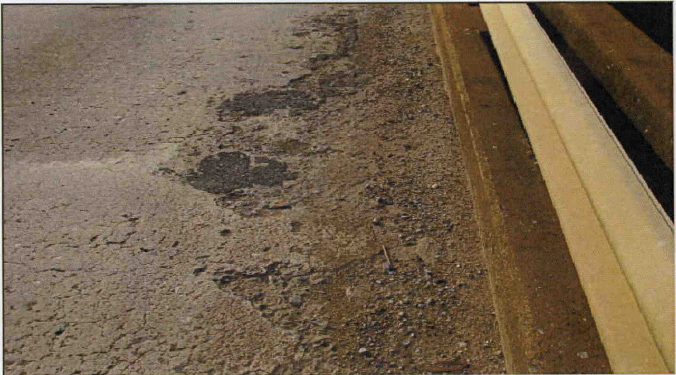
DECK DELAMINATION AT NORTHWEST CORNER
