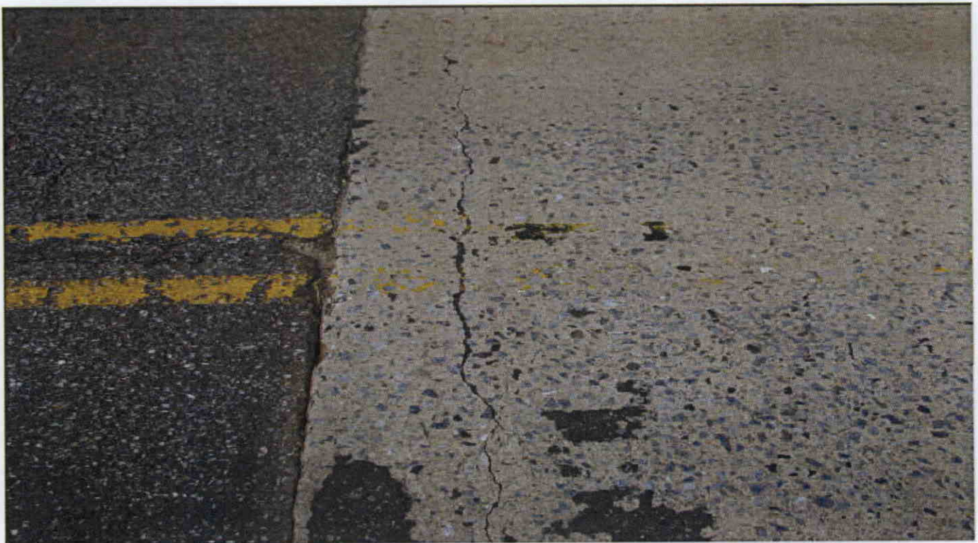
TRANSVERSE DECK CRACK AT SOUTH END OF BRIDGE
