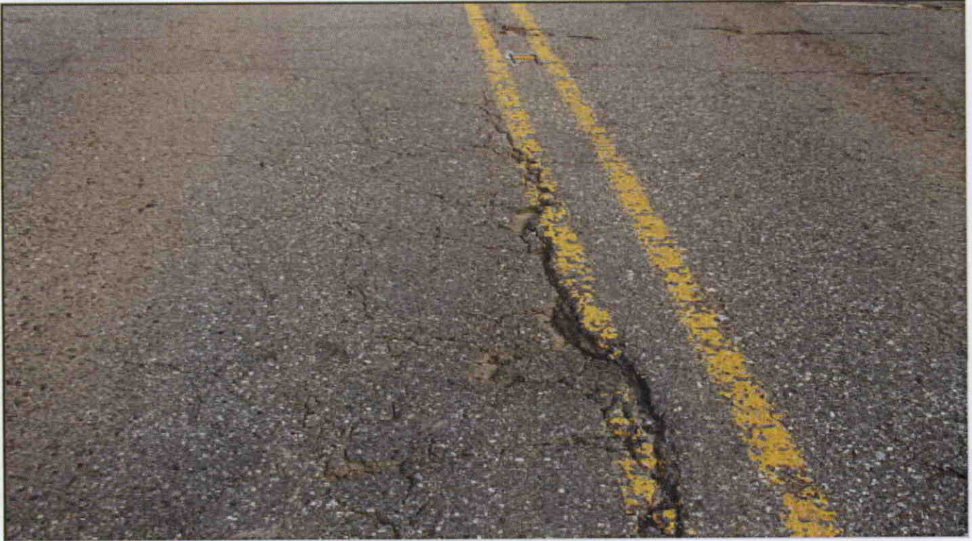
SETTLEMENT CRACKING IN SOUTH APPROACH
