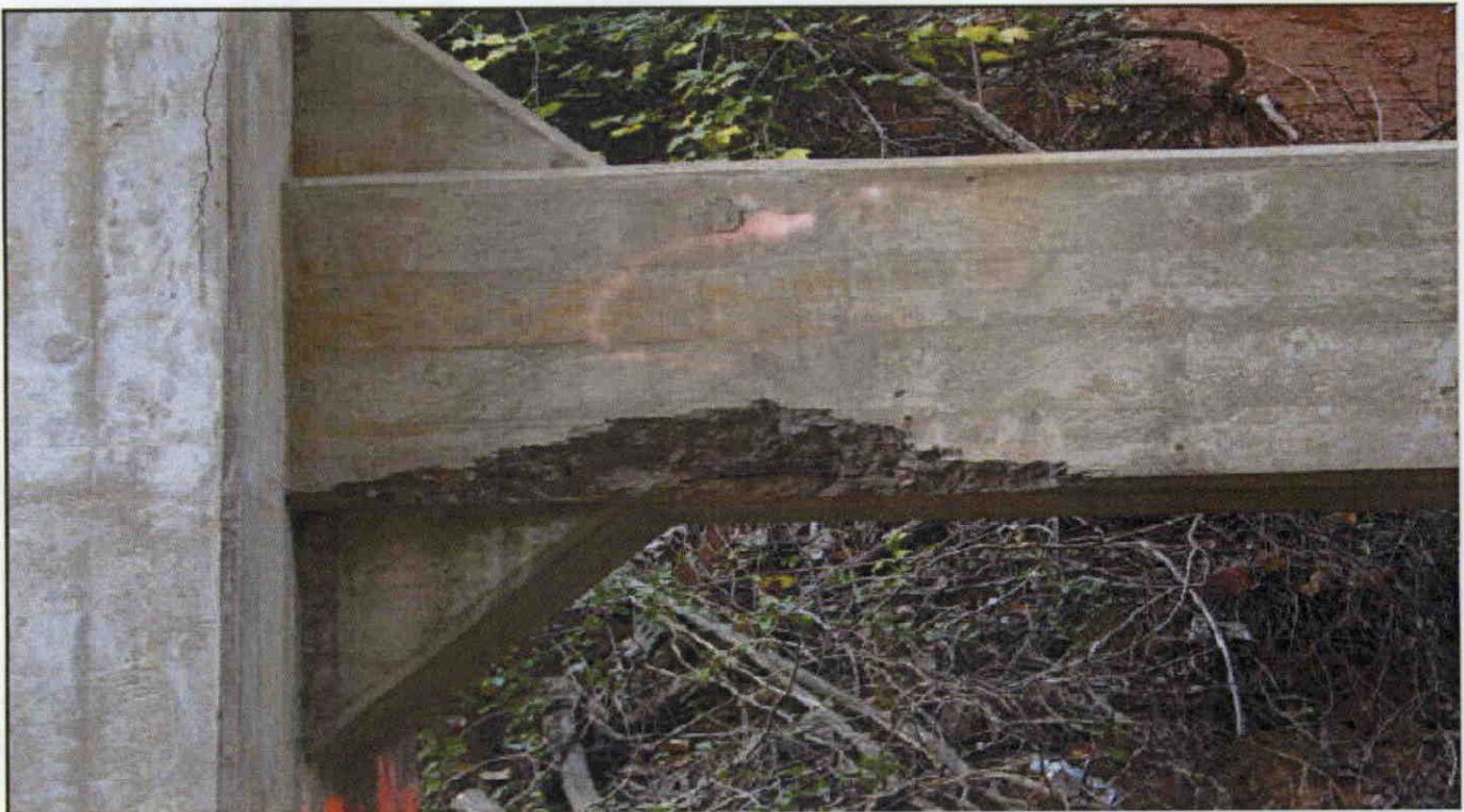
SPALLED NORTH FACE OF INTERIOR BENT LOWER STRUT
