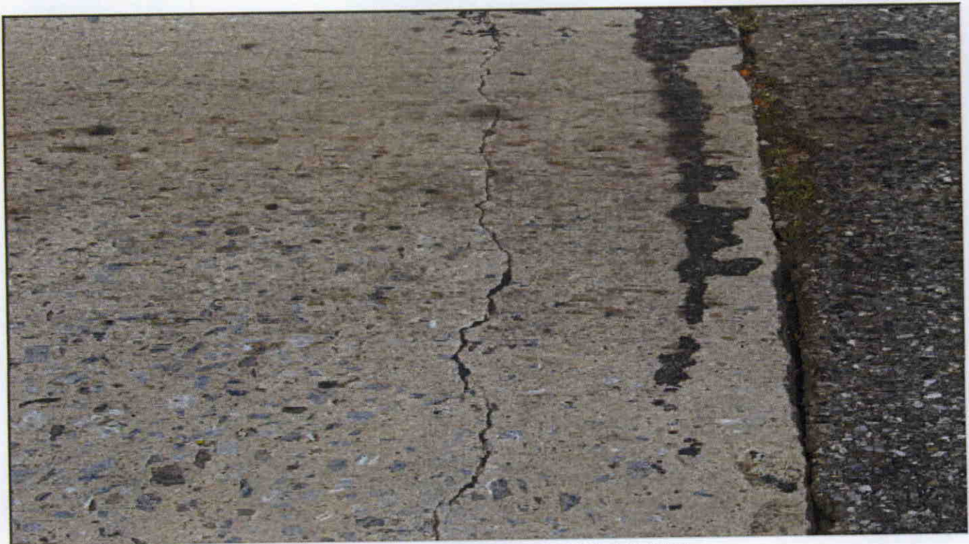
TRANSVERSE DECK CRACK AT NORTH END OF BRIDGE
