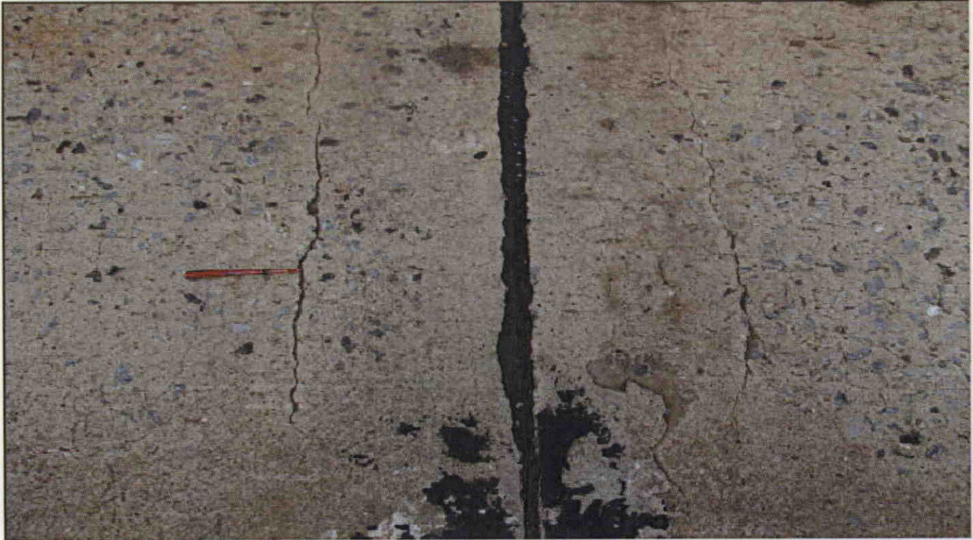
TRANSVERSE DECK CRACKS ALONG INTERIOR BENT JOINT
