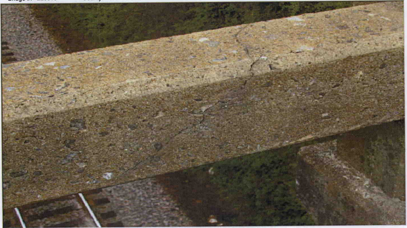
DIAGONAL CRACK ALONG WEST RAIL IN SPAN 2
