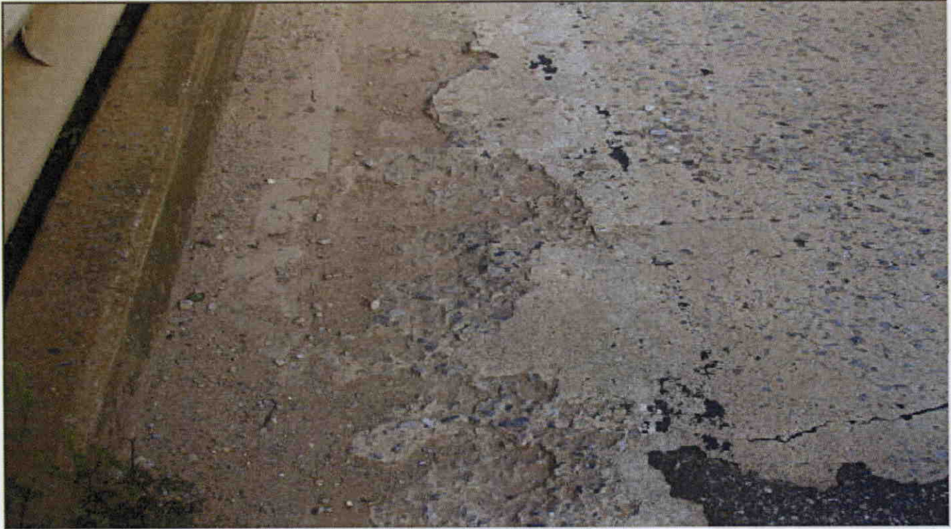
DECK DELAMINATION AT SOUTHWEST CORNER
