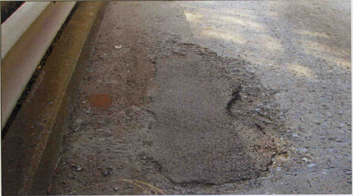
DECK DELAMINATION AT NORTHEAST CORNER
