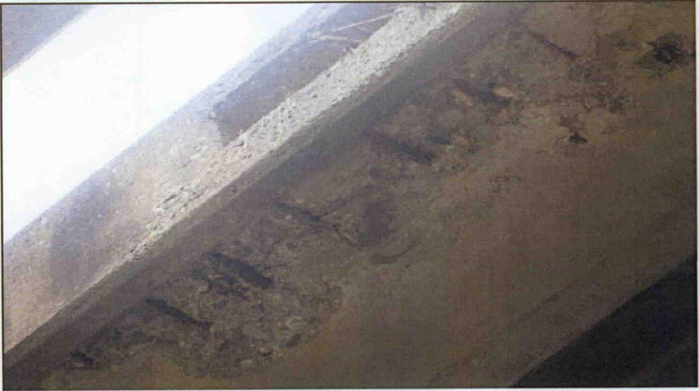
SPALLING ALONG WEST OVERHANG IN SPAN 2
