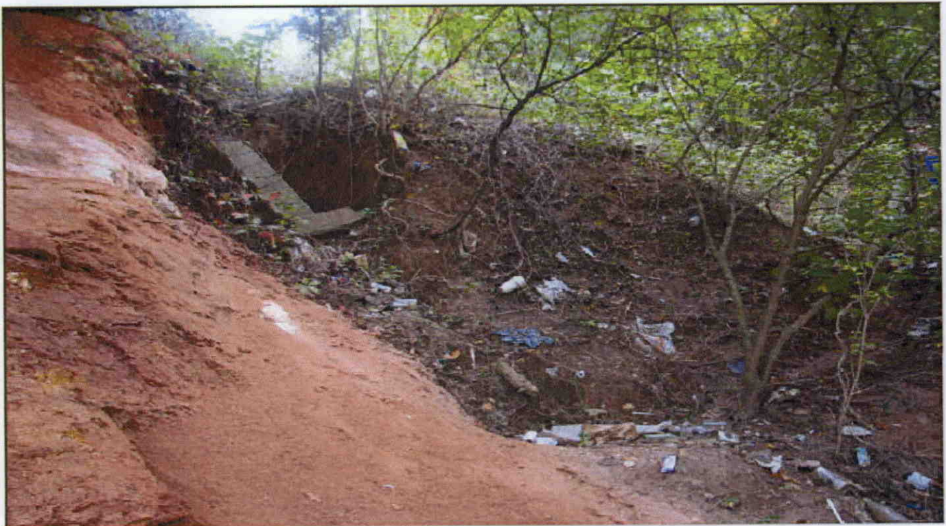
SLOPE EROSION AT SOUTHWEST CORNER UNDER SPAN 1
