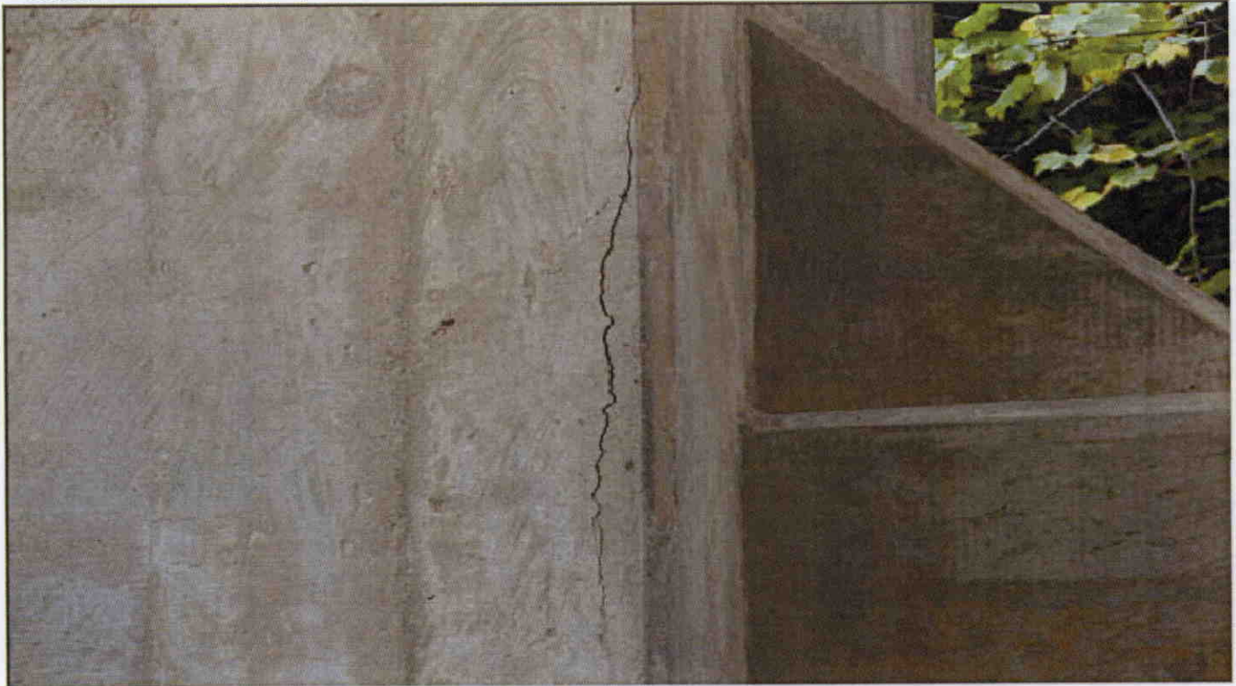
VERTICAL CRACK ON NORTH FACE OF INTERIOR BENT COLUMN 2
