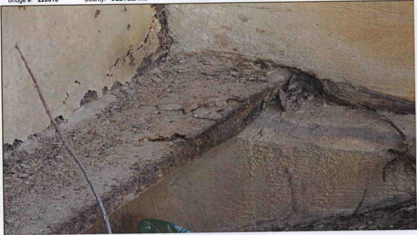
BEAM END RUST ON GIRDER 4 AT END BENT 2
