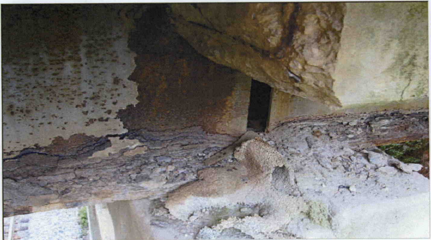
SECTION LOSS AT GIRDER 1 BEAM ENDS OVER BENT 1
