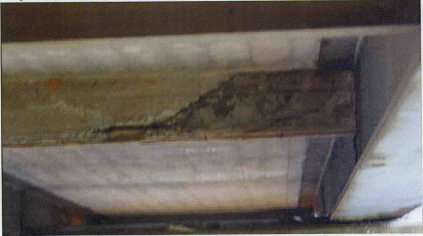
CRACKED END DIAPHRAGM IN BAY 3 OF SPAN 1 OVER BENT 1
