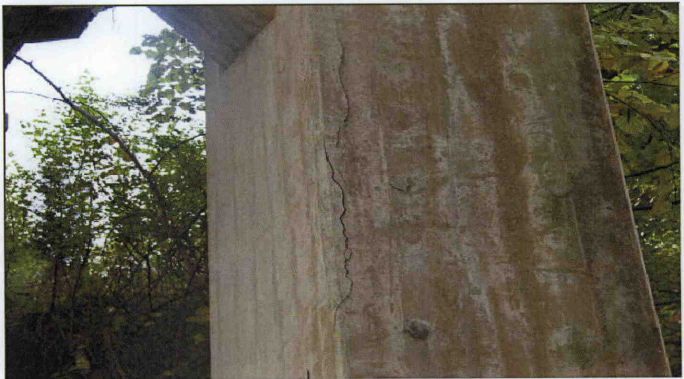
VERTICAL CRACK ON NORTH FACE OF INTERIOR BENT COLUMN 1
