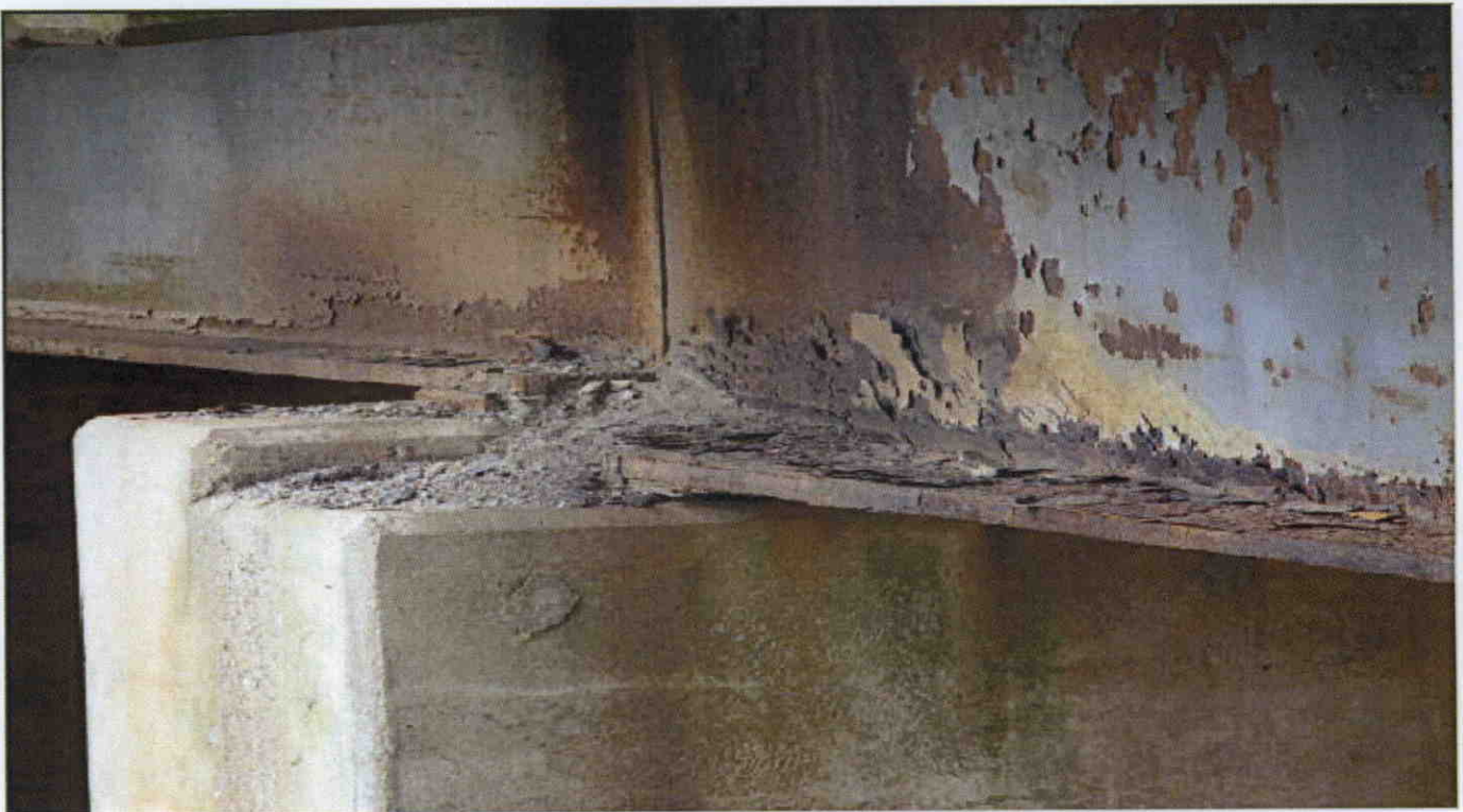
BEAM END RUST AT BENT 1 ON GIRDER 4
