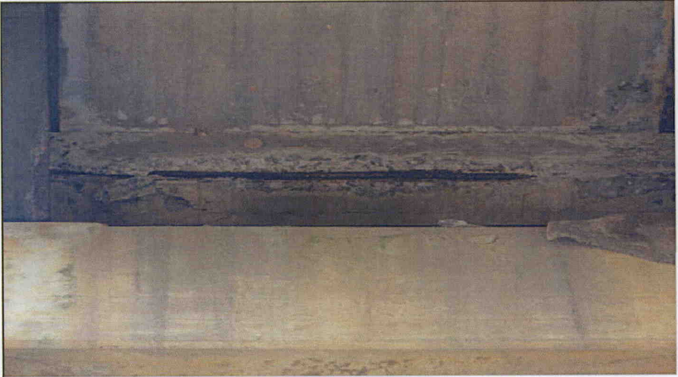
SPALLED END DIAPHRAGM IN BAY 2 OVER BENT 1
