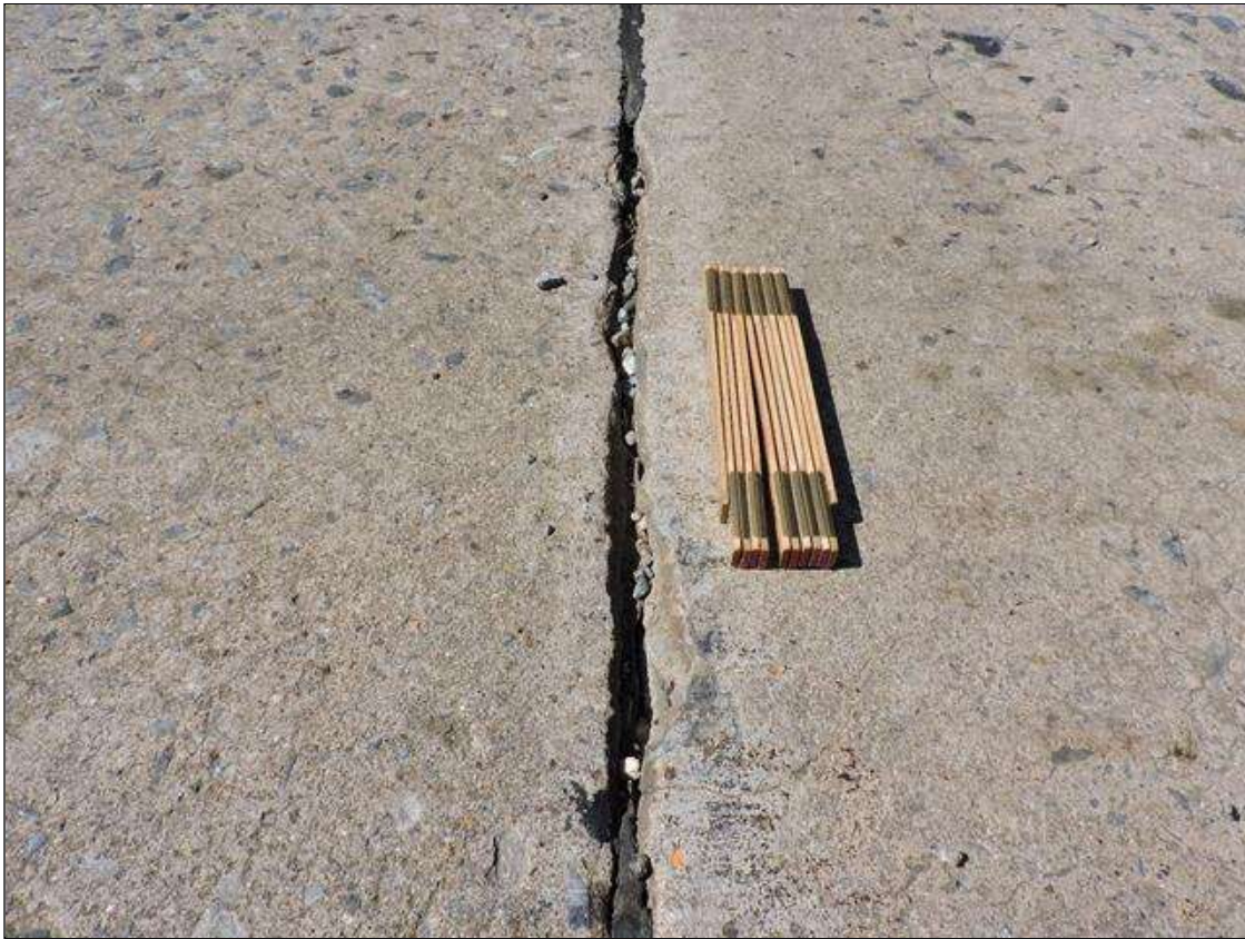
Expansion Joint 2: DETERIORATED JOINT MATERIAL ALONG BENT JOINT IN VARIOUS LOCATIONS THROUGHOUT, CONDITION IN SOUTHBOUND LANE SHOWN
