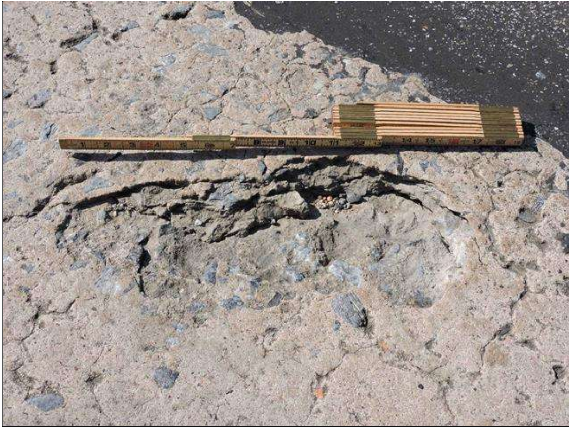
Span 2 Deck: 16" X 7" X 1" DEEP SPALL IN TOP OF DECK IN WHEEL LINE OF SOUTHBOUND LANE, APPROXIMATELY 8' FROM END BENT 2 FILL FACE
