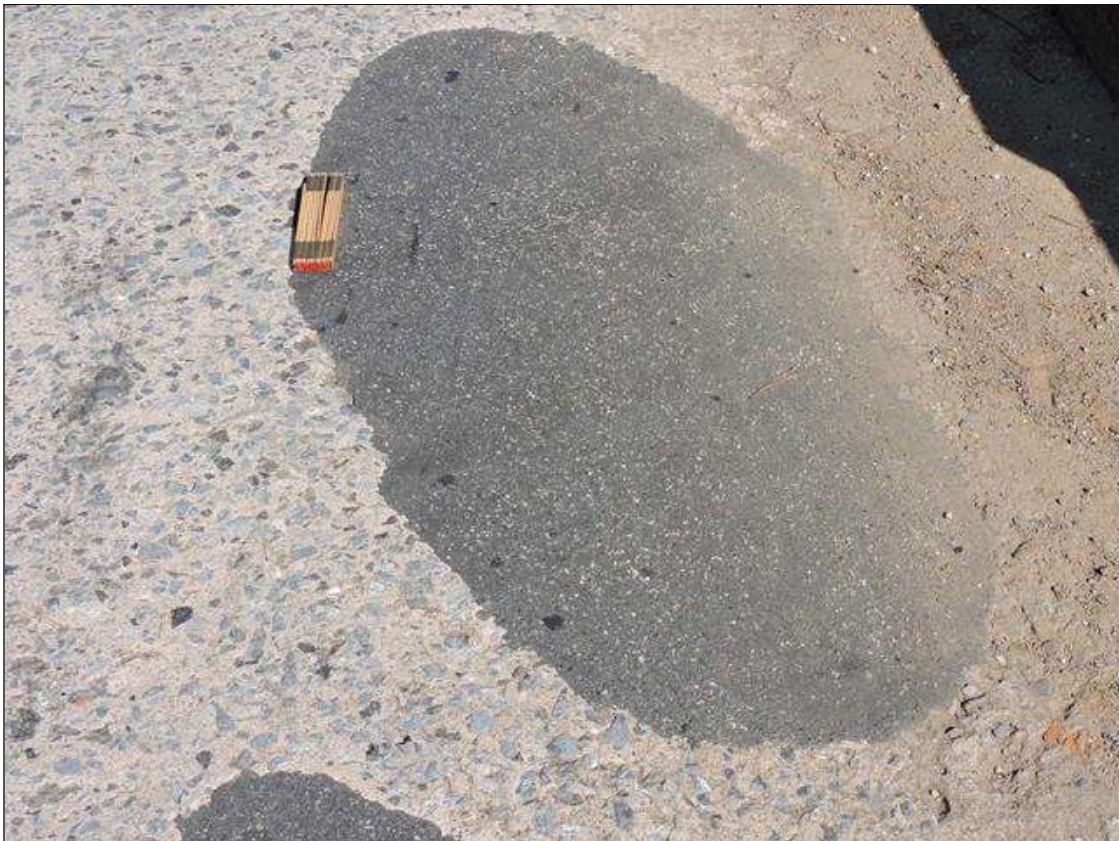
Span 2 Deck: 13 PATCHED AREAS UP TO 15' X 67" IN TOP OF DECK IN VARIOUS LOCATIONS THROUGHOUT, CONDITION IN NORTHBOUND LANE APPROXIMATELY 16' FROM END BENT 2 FILL FACE SHOWN
