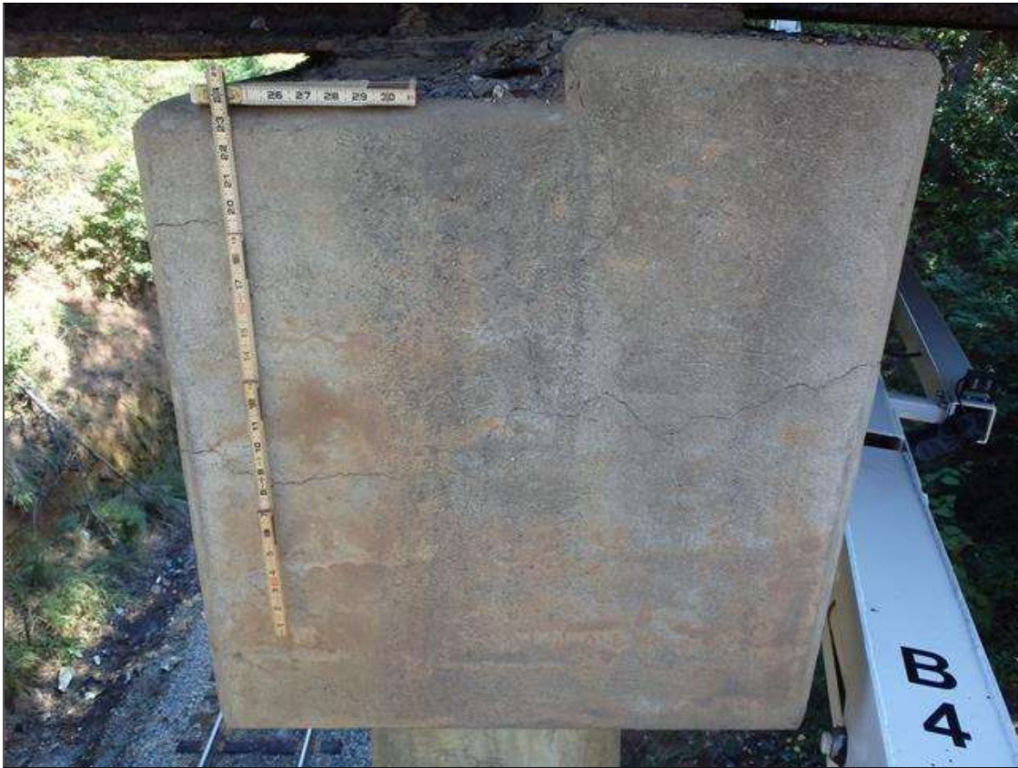
Bent 1 Cap 1: UP TO 0.04" MAP CRACKS IN BOTH ENDS OF CAP EXTENDING INTO ALL FACES, CRACKS IN LEFT END SHOWN
