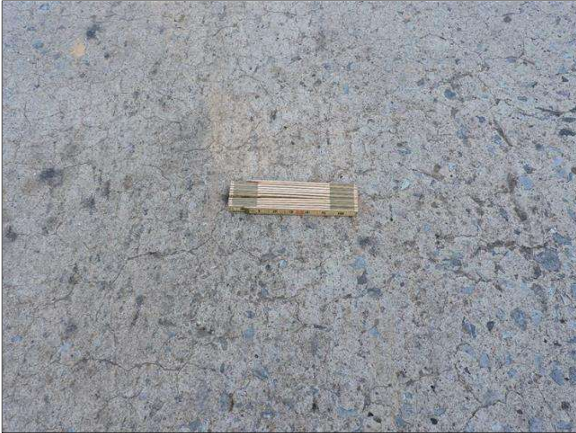
Span 2 Deck: UP TO 0.03" MAP CRACKS THROUGHOUT TOP OF DECK, CRACKS IN NORTHBOUND LANE APPROXIMATELY 8' FROM BENT SHOWN
