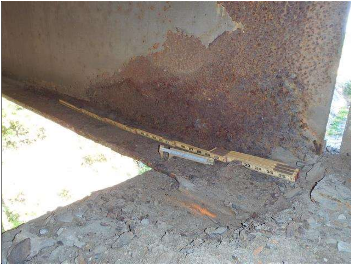
Span 2 Beam 4: SCALING AND PACK RUST ALONG BOTH FACES OF WEB AND BOTTOM FLANGE UP TO 58" LONG X 8" HIGH WITH UP TO 1/16" LOSS OF SECTION IN WEB AND 28" LONG X 3" WIDE DOWN TO 9/16" RESIDUAL FLANGE ALONG EDGES OF BOTTOM FLANGE AT FACE OF BENT BEARING, CONDITION ON LEFT SIDE SHOWN, PRIORITY MAINTENANCE
