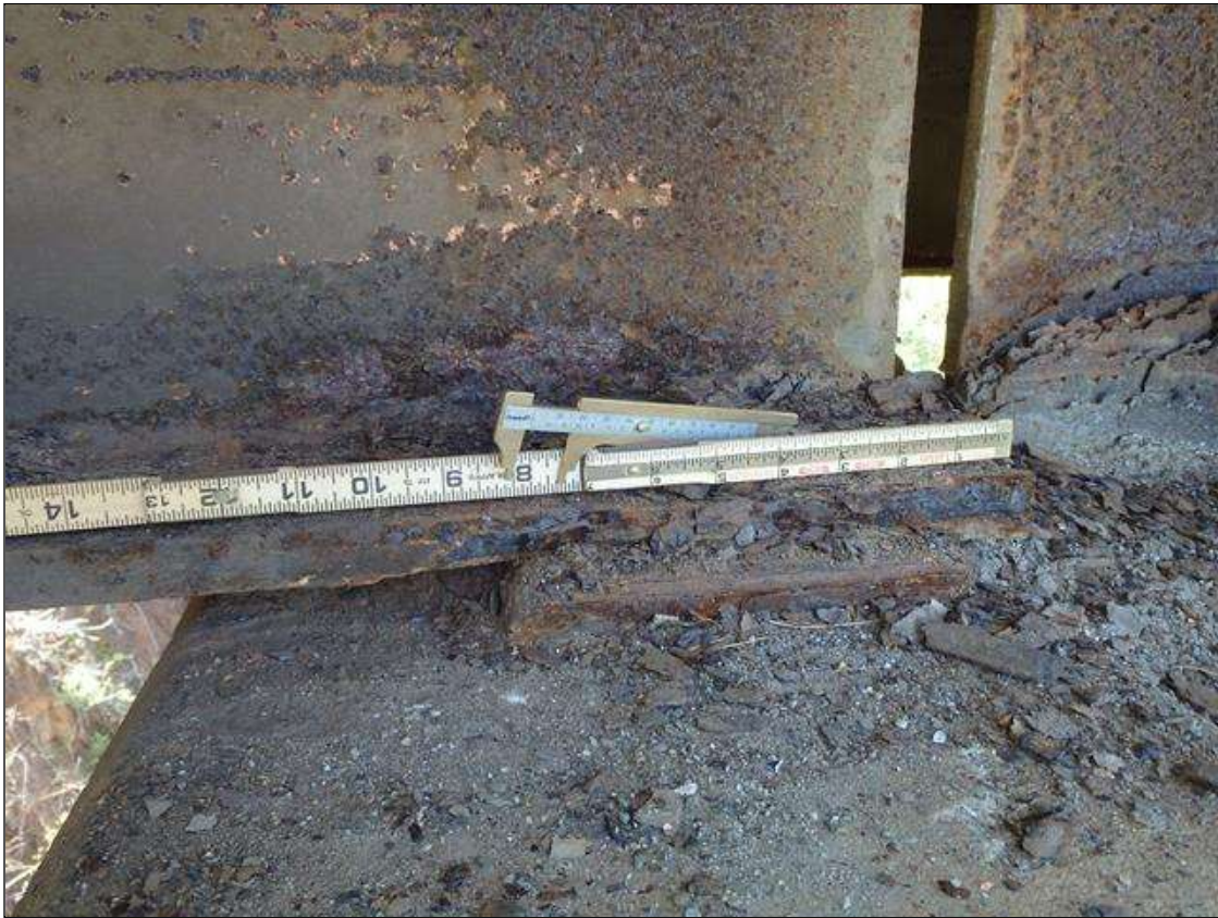
Span 1 Beam 4: SCALING AND PACK RUST ALONG BOTH FACES OF WEB AND BOTTOM FLANGE UP TO 12" LONG X 2" HIGH WITH NO MEASURABLE LOSS OF SECTION IN WEB AND 10" LONG X 2" WIDE DOWN TO 3/4" RESIDUAL FLANGE ALONG EDGES OF BOTTOM FLANGE AT BENT BEARING, CONDITION ON RIGHT SIDE SHOWN, PRIORITY MAINTENANCE
