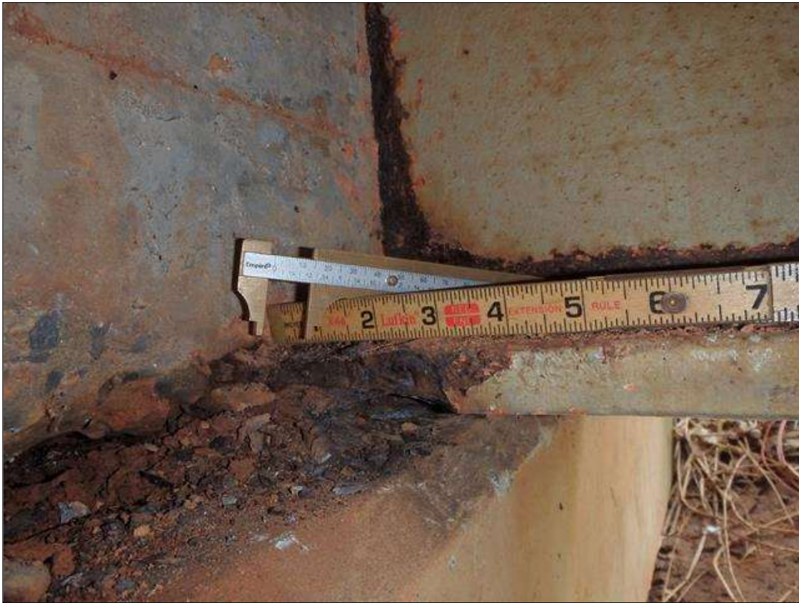
Span 1 Beam 1: SCALING AND PACK RUST ALONG BOTTOM FLANGE UP TO 6" LONG X FULL WIDTH DOWN TO 5/8" RESIDUAL FLANGE AT FACE OF END BENT 1 BEARING, CONDITION ON RIGHT SIDE SHOWN, PRIORITY MAINTENANCE
