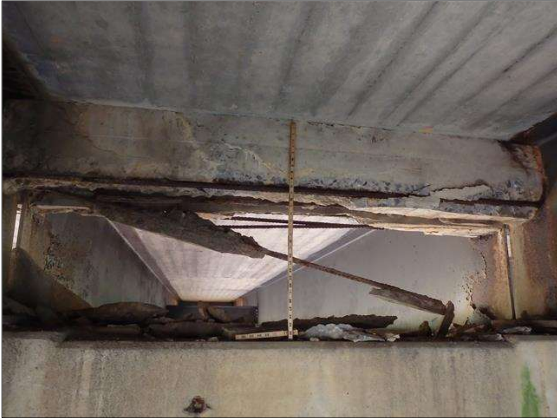
BENT DIAPHRAGMS: UP TO FULL LENGTH X FULL WIDTH X UP TO 6" DEEP SPALLS WITH EXPOSED REBAR IN DIAPHRAGMS, CONDITION IN BAY 2 OF SPAN 1 SHOWN
