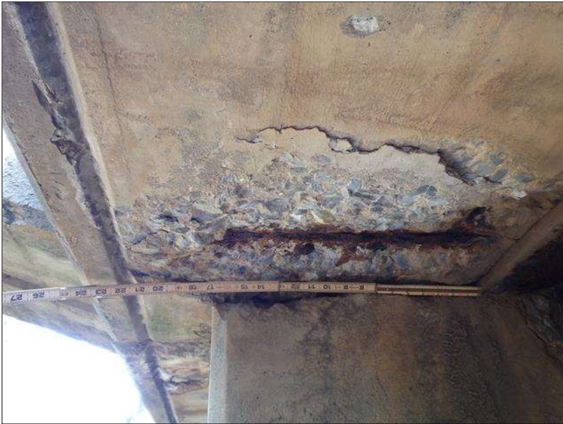
Span 1 Deck: UP TO 22" X 16" X 1 1/2" DEEP SPALLS WITH EXPOSED REBAR IN BOTTOM OF BOTH OVERHANGS ABOVE BENT, SPALL IN BOTTOM OF LEFT OVERHANG SHOWN
