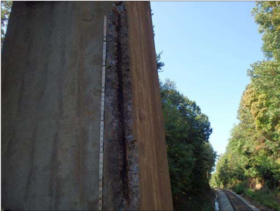
Bent 1 Pile 1: 55" X 6" X 2" DEEP SPALL WITH EXPOSED REBAR IN NORTHEAST CORNER OF COLUMN, APPROXIMATELY 16' FROM BOTTOM OF CAP, PRIORITY MAINTENANCE
