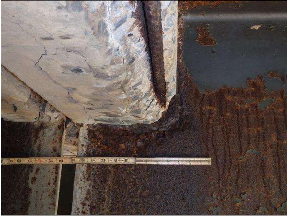
Span 2 Beam 3: SCALING AND PACK RUST IN BOTH FACES OF WEB UP TO 6" HIGH X 11" WIDE WITH UP TO 1/8" LOSS OF SECTION AROUND BENT DIAPHRAGM, CONDITION ON RIGHT SIDE SHOWN, PRIORITY MAINTENANCE
