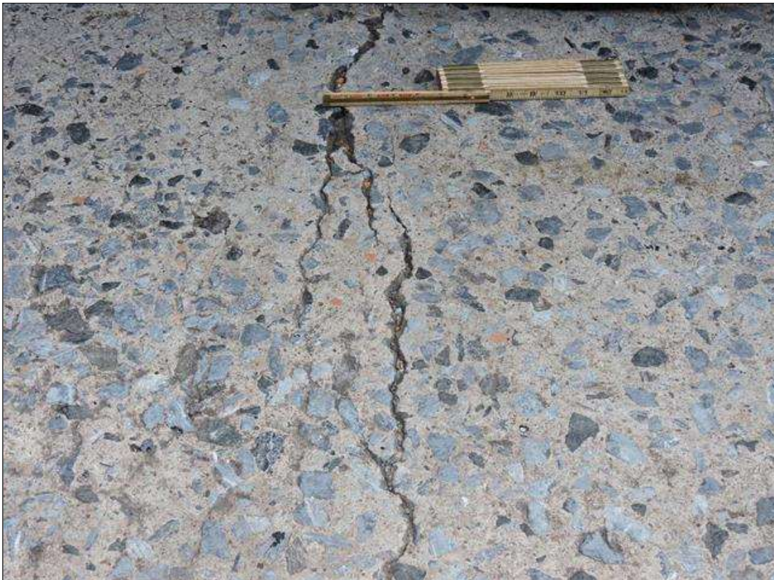
Span 1 Deck: UP TO 1/2" TRANSVERSE CRACKS AND UP TO 1/16" MAP CRACKS IN TOP OF DECK IN VARIOUS LOCATIONS THROUGHOUT, CRACKS NEAR MIDSPAN SHOWN
