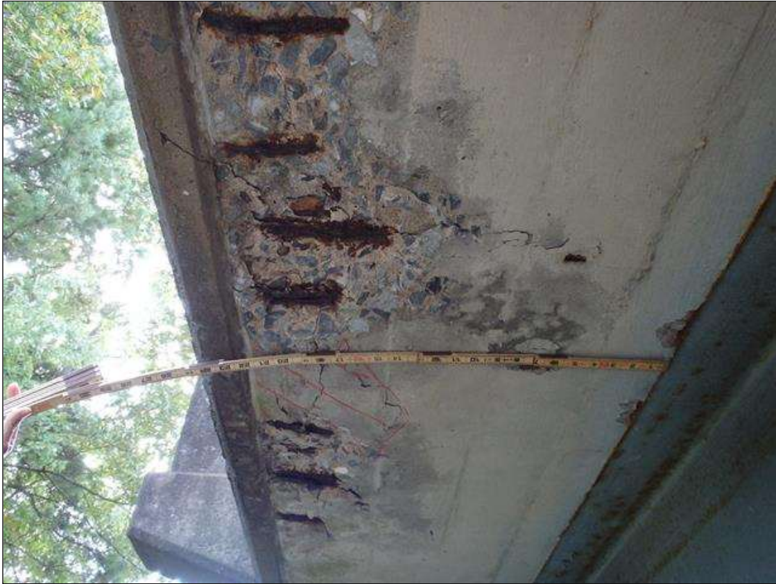
Span 1 Deck: UP TO 21" X 12" X 1 3/4" DEEP SPALLS WITH EXPOSED REBAR AND UP TO 9" X 9" AREAS OF DELAMINATION THROUGHOUT BOTTOM OF BOTH OVERHANGS, CONDITION IN BOTTOM OF RIGHT OVERHANG NEAR MIDSPAN SHOWN
