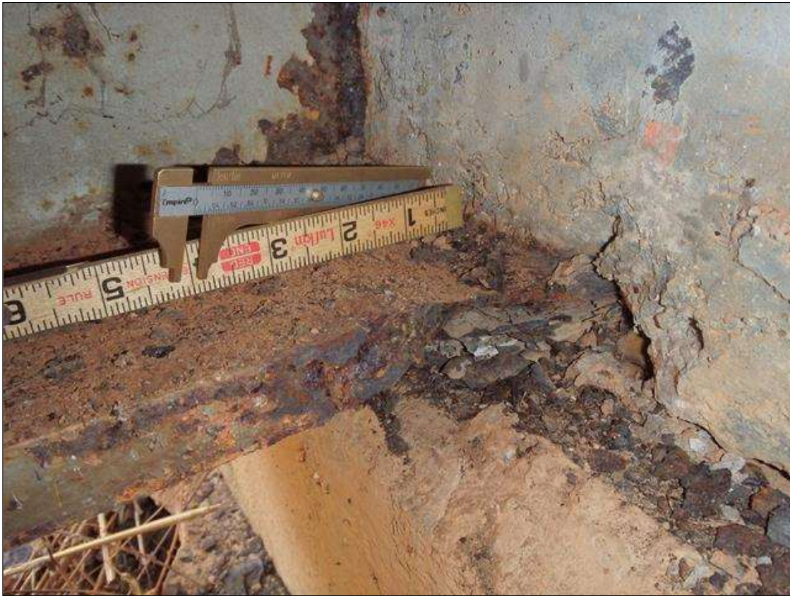
Span 2 Beam 1: SCALING AND PACK RUST ALONG BOTH EDGES OF BOTTOM FLANGE UP TO 4" LONG X 5" WIDE DOWN TO 1/4" RESIDUAL FLANGE AT FACE OF END BENT 2 BEARING, CONDITION ON RIGHT SIDE SHOWN, PRIORITY MAINTENANCE
