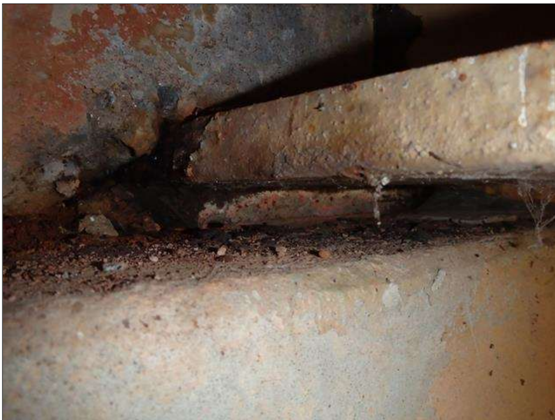
Span 1 Beam 3 Near Bearing: SURFACE CORROSION THROUGHOUT EXPOSED FACE OF BEAM 3 BEARING AT END BENT 1
