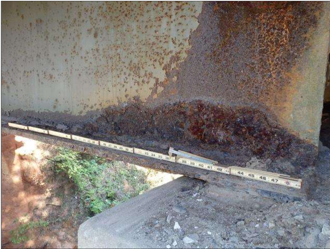
Span 2 Beam 1: SCALING AND PACK RUST ALONG BOTH FACES OF WEB AND BOTTOM FLANGE UP TO 55" LONG X 6" HIGH WITH UP TO 1/16" LOSS OF SECTION IN WEB AND 30" LONG X FULL WIDTH DOWN TO 1/2" RESIDUAL FLANGE AT FACE OF BENT BEARING, CONDITION ON LEFT SIDE SHOWN, PRIORITY MAINTENANCE
