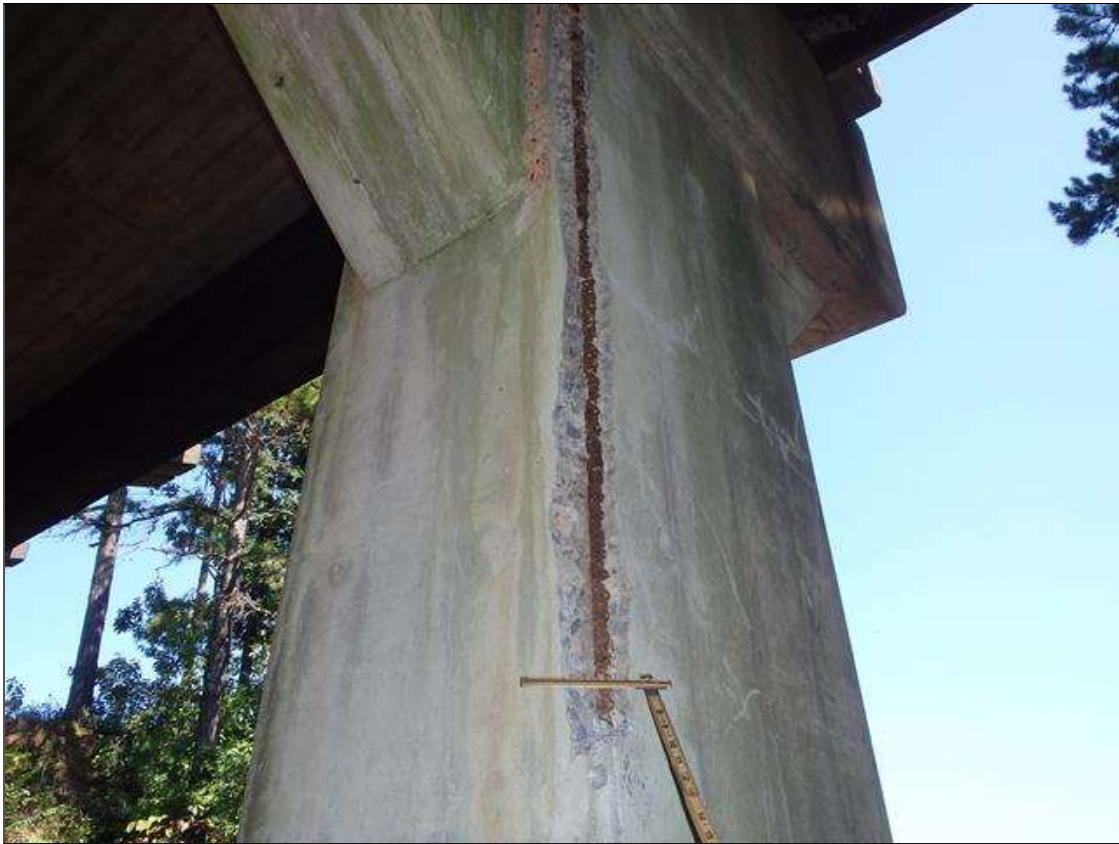
Bent 1 Pile 2: 66" X 4" X 2" DEEP SPALL WITH EXPOSED REBAR IN SOUTHWEST CORNER OF COLUMN AT BOTTOM OF CAP, PRIORITY MAINTENANCE
