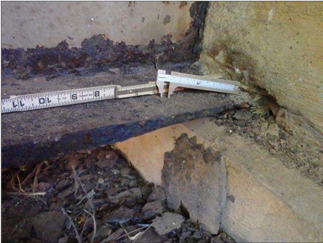
Span 2 Beam 4: SCALING AND PACK RUST ALONG BOTH EDGES OF BOTTOM FLANGE UP TO 9" LONG X 2" WIDE DOWN TO 5/16" RESIDUAL FLANGE AT FACE OF END BENT 2 BEARING, CONDITION ON RIGHT SIDE SHOWN, PRIORITY MAINTENANCE
