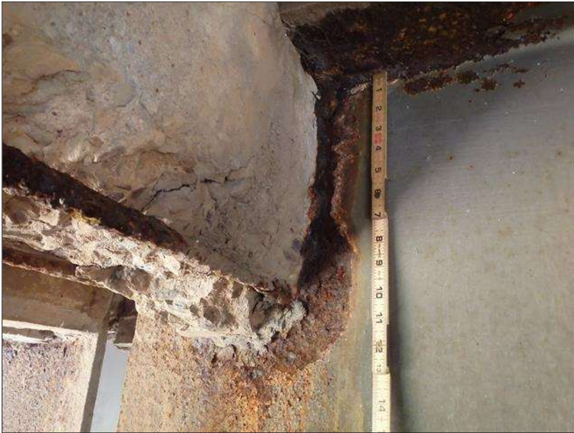
Span 1 Beam 2: SCALING AND PACK RUST IN BOTH FACES OF WEB UP TO 13" HIGH X 7" WIDE WITH UP TO 1/8" LOSS OF SECTION AROUND BENT DIAPHRAGM, CONDITION ON LEFT SIDE SHOWN, PRIORITY MAINTENANCE
