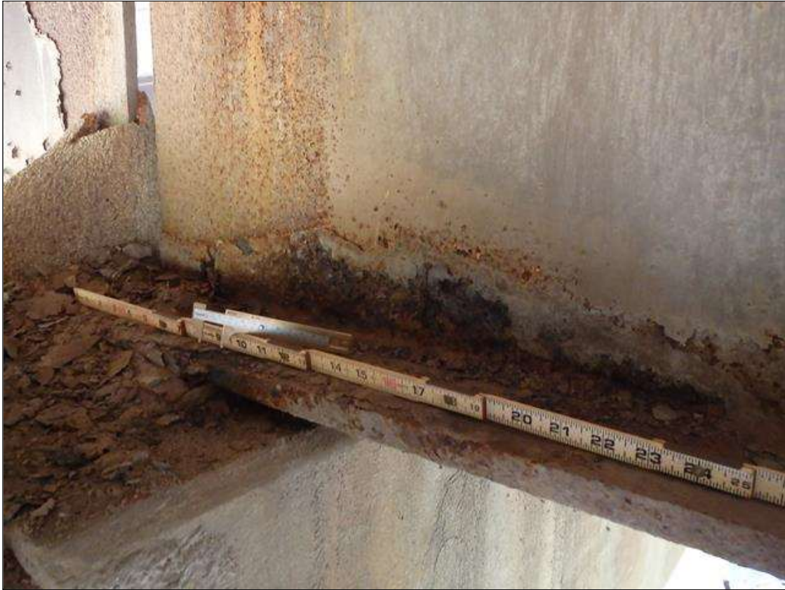
Span 1 Beam 2: SCALING AND PACK RUST ALONG BOTH FACES OF WEB AND BOTTOM FLANGE UP TO 20" LONG X 4" HIGH WITH NO MEASURABLE LOSS OF SECTION IN WEB AND 8" LONG X 2 1/2" WIDE DOWN TO 11/16" RESIDUAL FLANGE ALONG EDGES OF BOTTOM FLANGE AT FACE OF BENT BEARING, CONDITION ON LEFT SIDE SHOWN, PRIORITY MAINTENANCE
