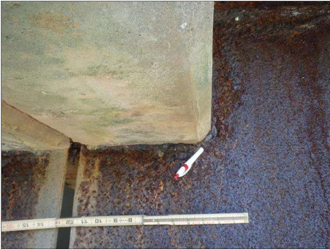
Span 2 Beam 4: SCALING AND PACK RUST IN BOTH FACES OF WEB UP TO 14" HIGH X 12" WIDE WITH UP TO 1/2" DIAMETER HOLES AROUND BENT DIAPHRAGM, CONDITION ON RIGHT SIDE SHOWN, PRIORITY MAINTENANCE
