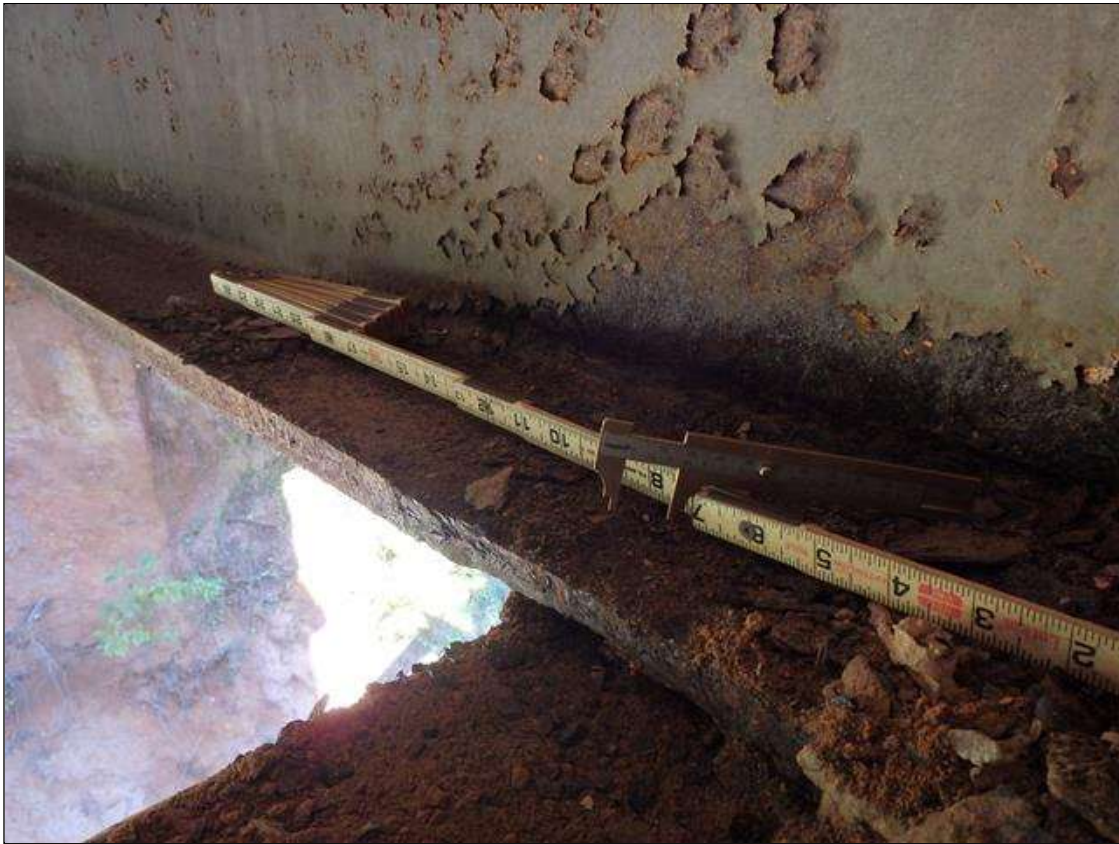
Span 2 Beam 2: SCALING AND PACK RUST ALONG BOTH FACES OF WEB AND BOTTOM FLANGE UP TO 18" LONG X 2" HIGH WITH NO MEASURABLE LOSS OF SECTION IN WEB AND 9" LONG X 2" WIDE DOWN TO 3/4" RESIDUAL FLANGE ALONG EDGES OF BOTTOM FLANGE AT FACE OF BENT BEARING, CONDITION ON LEFT SIDE SHOWN, PRIORITY MAINTENANCE
