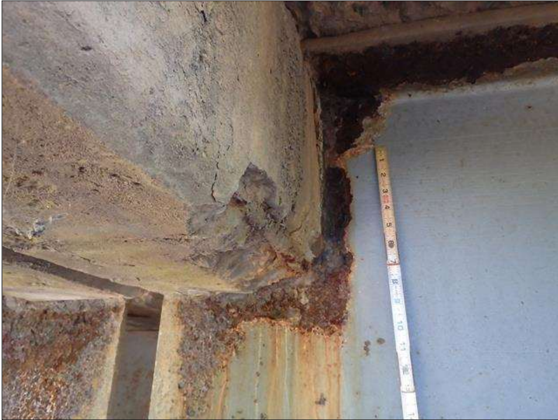
Span 1 Beam 1: SCALING AND PACK RUST IN BOTH FACES OF WEB UP TO 14" HIGH X 10" WIDE WITH UP TO 1/16" LOSS OF SECTION AROUND BENT DIAPHRAGM, CONDITION ON LEFT SIDE SHOWN, PRIORITY MAINTENANCE
