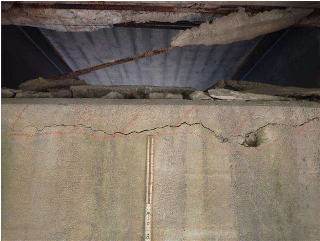
Bent 1 Cap 1: 56" X 6" X 3" AREA OF DELAMINATION AND UP TO 1/8" LONGITUDINAL AND HORIZONTAL CRACKS AND HAIRLINE MAP CRACKS THROUGHOUT TOP, BOTTOM AND SPAN 2 FACE OF CAP, CONDITION BENEATH BAY 2 SHOWN
