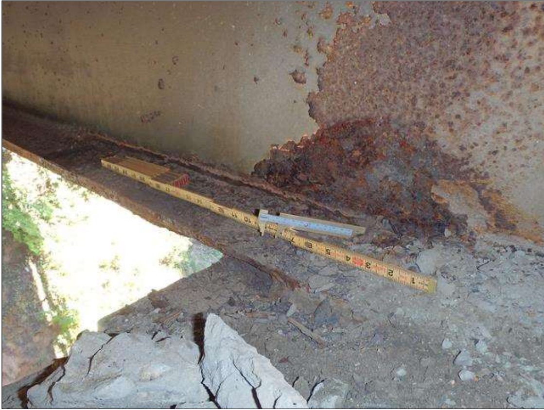
Span 2 Beam 3: SCALING AND PACK RUST ALONG BOTH FACES OF WEB AND BOTTOM FLANGE UP TO 34" LONG X 6" HIGH WITH UP TO 1/16" LOSS OF SECTION IN WEB AND 20" LONG X 3" WIDE DOWN TO 9/16" RESIDUAL FLANGE ALONG EDGES OF BOTTOM FLANGE AT FACE OF BENT BEARING, CONDITION ON LEFT SIDE SHOWN, PRIORITY MAINTENANCE
