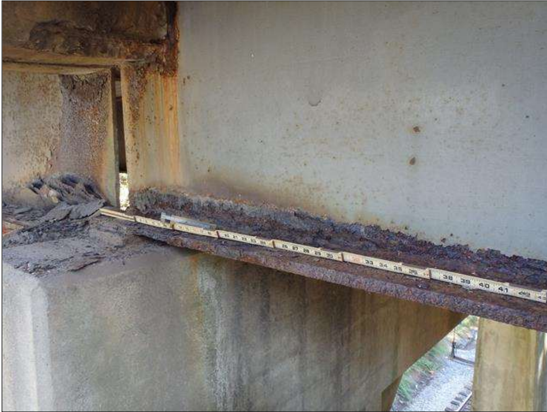
Span 1 Beam 1: SCALING AND PACK RUST ALONG BOTH FACES OF WEB AND BOTTOM FLANGE UP TO 102" LONG X 3" HIGH WITH UP TO 1/16" LOSS OF SECTION IN WEB AND 13" LONG X 3" WIDE DOWN TO 1/2" RESIDUAL FLANGE ALONG EDGES OF BOTTOM FLANGE AT FACE OF BENT BEARING, CONDITION ON LEFT SIDE SHOWN, PRIORITY MAINTENANCE
