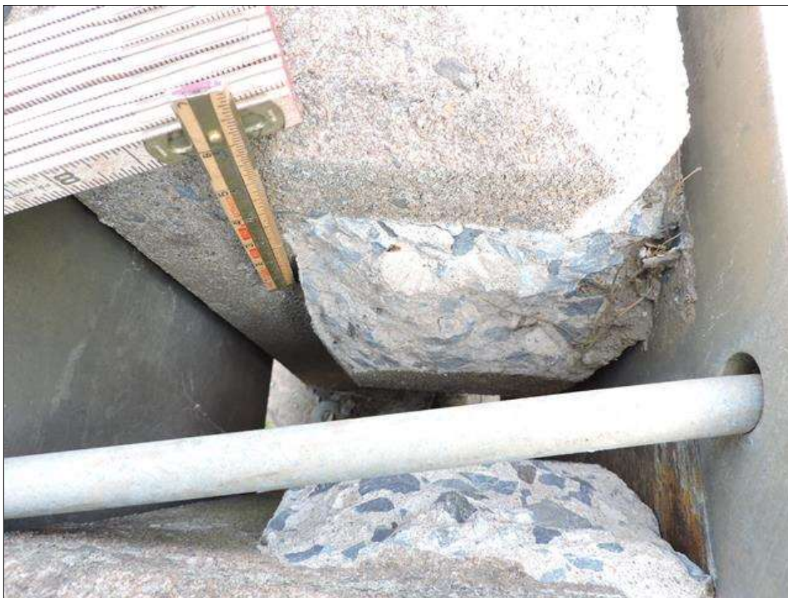
Span 1 Left Bridge Rail: TWO (2) SPALLS UP TO 7" X 5" X 2" DEEP IN ENDS OF RAIL, APPROXIMATELY 16' FROM END BENT 1
