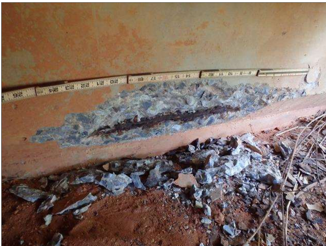
End Bent 1 Cap 1: 28" X 8" X 1 1/2" DEEP SPALL WITH EXPOSED REBAR IN FACE OF CAP TO RIGHT OF BEAM 1, PRIORITY MAINTENANCE
