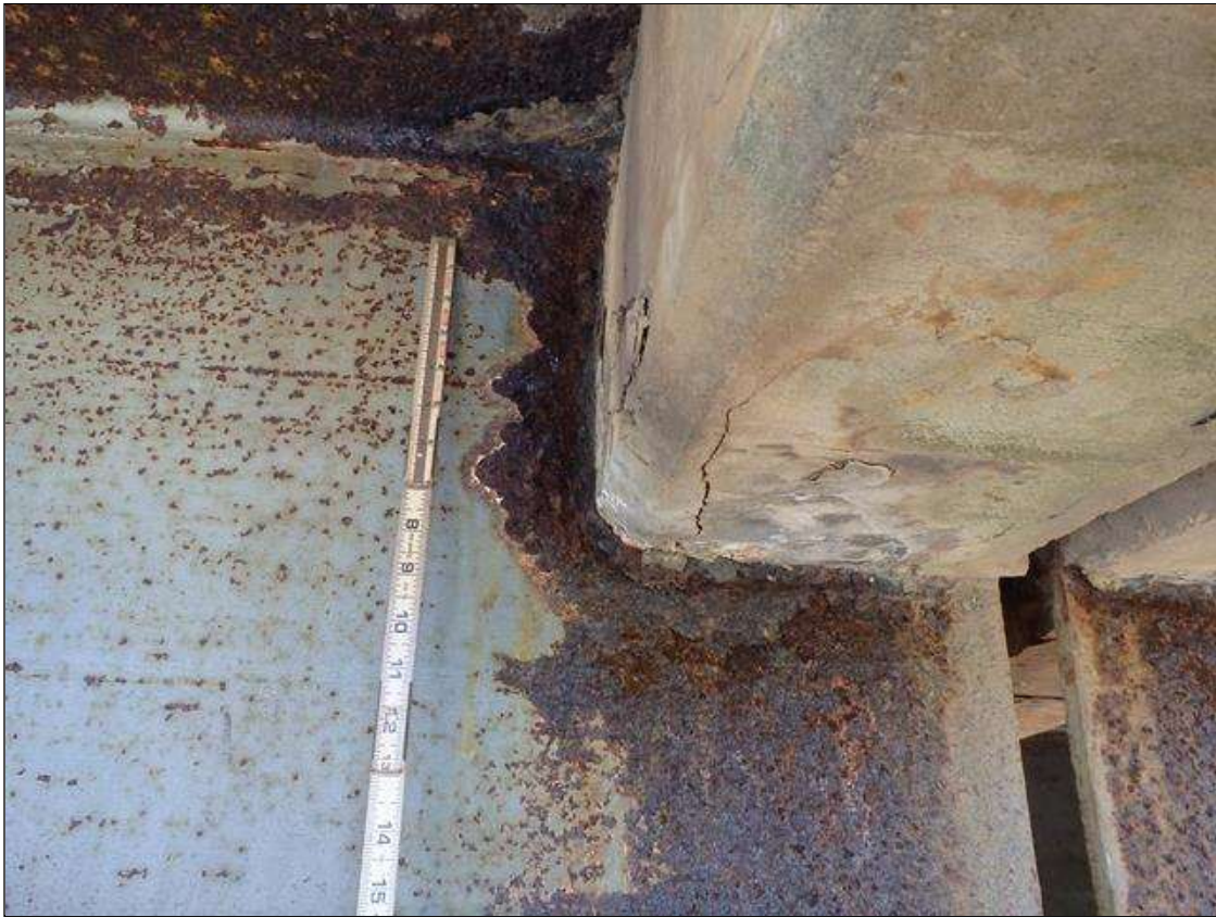
Span 1 Beam 4: SCALING AND PACK RUST IN BOTH FACES OF WEB UP TO 13" HIGH X 11" WIDE WITH UP TO 1/16" LOSS OF SECTION AROUND BENT DIAPHRAGM, CONDITION ON RIGHT SIDE SHOWN, PRIORITY MAINTENANCE
