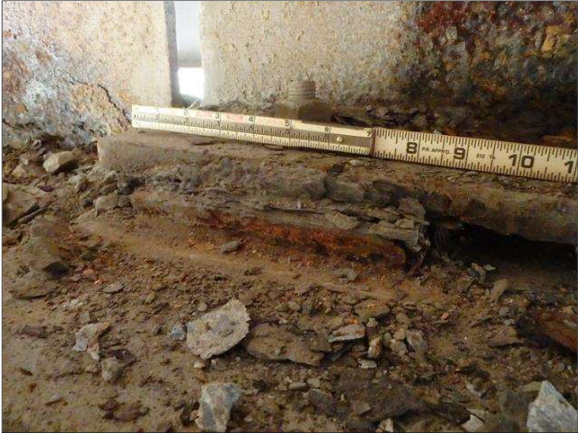
Span 1 Beam 3 Far Bearing: SCALING AND PACK RUST THROUGHOUT BEAM 3 BEARING AT BENT
