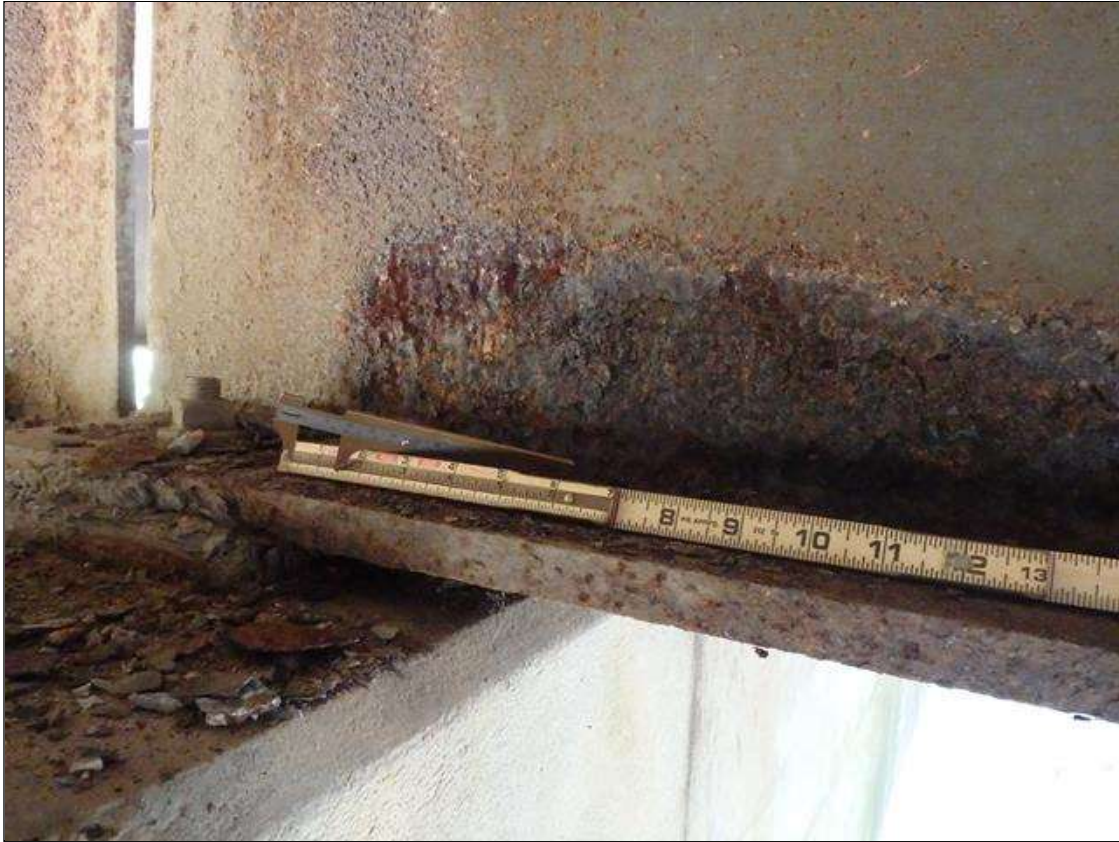
Span 1 Beam 3: SCALING AND PACK RUST ALONG BOTH FACES OF WEB AND BOTTOM FLANGE UP TO 48" LONG X 4" HIGH WITH NO MEASURABLE LOSS OF SECTION IN WEB AND 3" LONG X 2" WIDE DOWN TO 3/4" RESIDUAL FLANGE ALONG EDGES OF BOTTOM FLANGE AT FACE OF BENT BEARING, CONDITION ON LEFT SIDE SHOWN, PRIORITY MAINTENANCE
