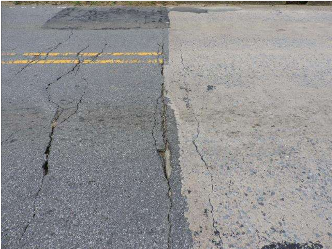
TRANSITION ALONG END BENT 1 FILL FACE, TRANSITION ALONG END BENT 2 FILL FACE SIMILAR
