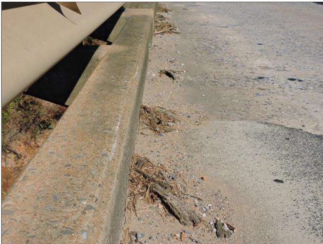
DIRT AND DEBRIS ACCUMULATION IN BOTH SHOULDERS, ACCUMULATION IN LEFT SHOULDER SHOWN
