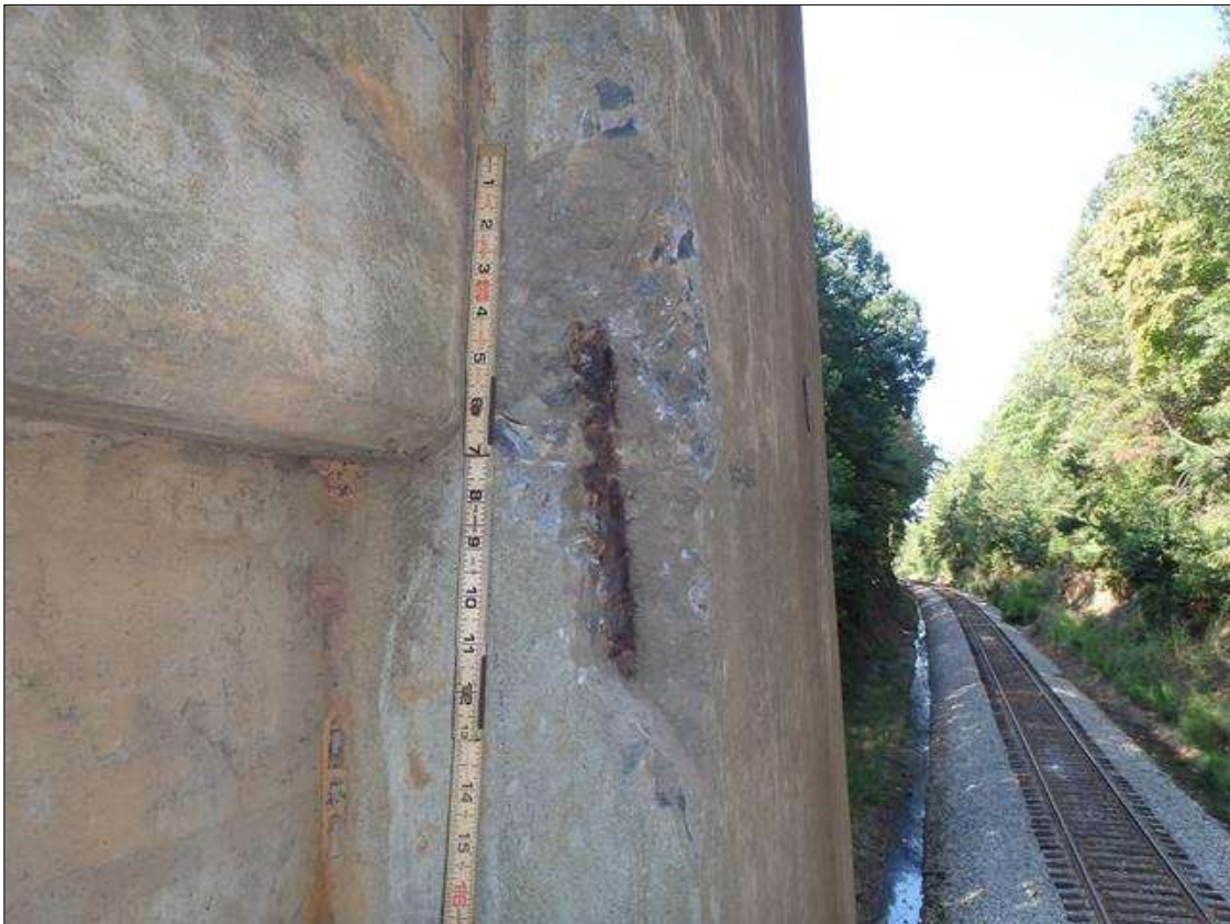
Bent 1 Pile 1: 18" X 7" X 2" DEEP SPALL WITH EXPOSED REBAR IN NORTHEAST CORNER OF COLUMN, APPROXIMATELY 13' FROM BOTTOM OF CAP, PRIORITY MAINTENANCE
