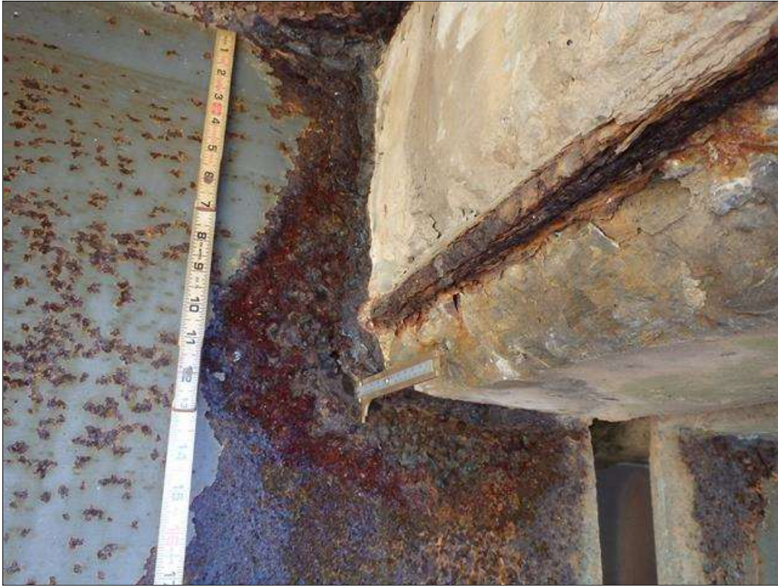
Span 2 Beam 1: SCALING AND PACK RUST IN BOTH FACES OF WEB UP TO 15" HIGH X 12" WIDE WITH 4" X 1/4" HOLE AROUND BENT DIAPHRAGM, CONDITION ON LEFT SIDE SHOWN, PRIORITY MAINTENANCE
