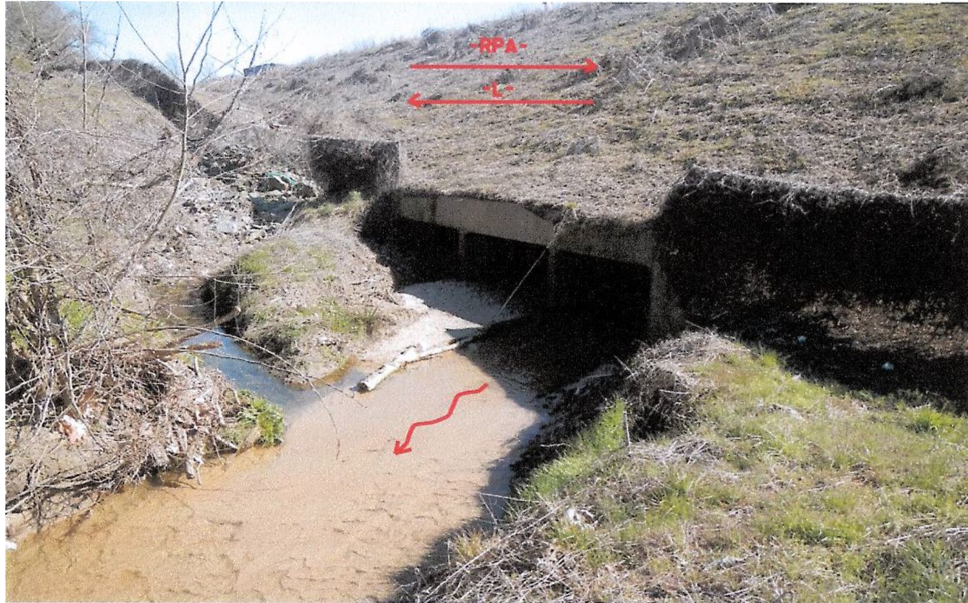
View Facing Southeast (Upstream) Along Tributary L-8 at Proposed -RPA- Culvert Location (Photo taken from BSR)
