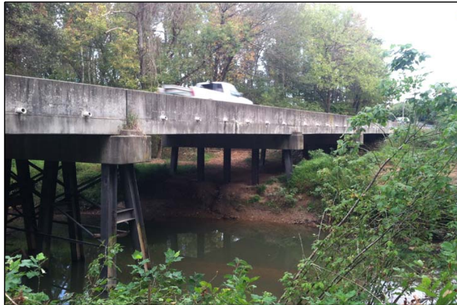
PHOTOGRAPH TAKEN FROM NEAR INTERIOR BENT 1 LOOKING UPSTATION AT EXISTING BRIDGE AND CHANNEL.
