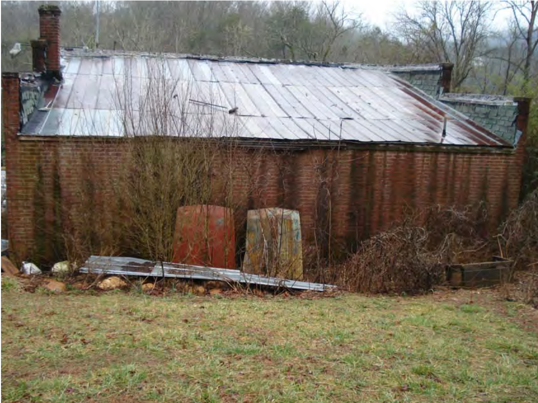
Photograph 2: View looking south at rear of former service station. No entrances or evidence of former bay doors, were observed.
