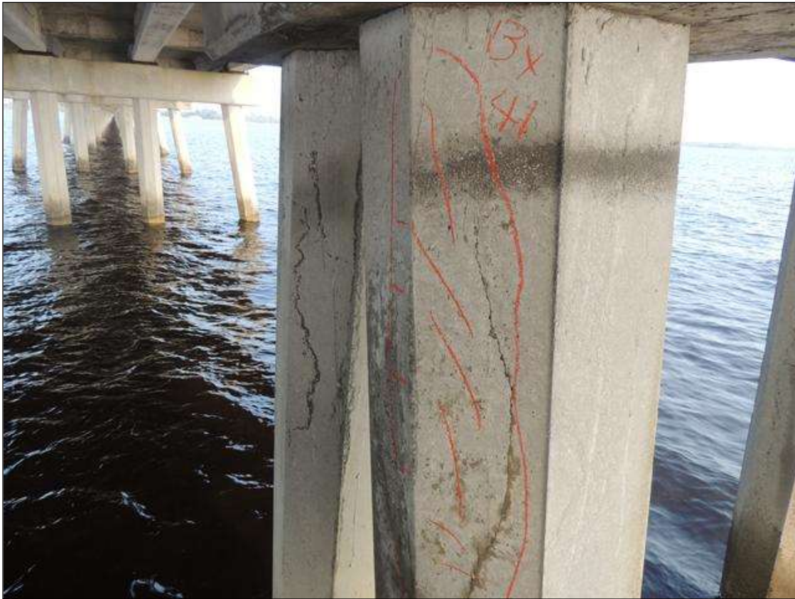
BENT 81 DELAMINATED AREA ON SOUTH FACE OF P3 UNDER BOTTOM OF CAP 13" X 41".
