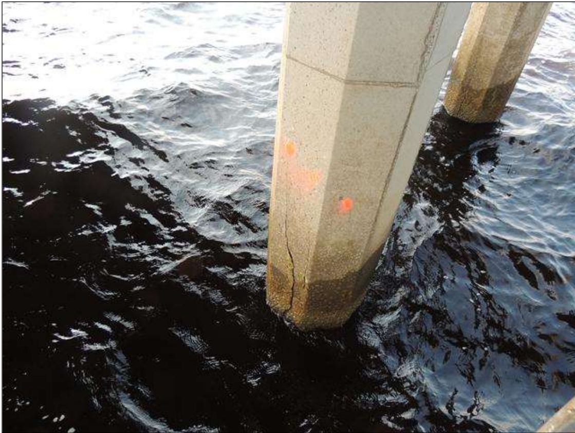
BENT 222 P3 CRACKED AND DELAMINATED AREA 42" FROM THE WATERLINE UP 22" AROUND THE PILE.
