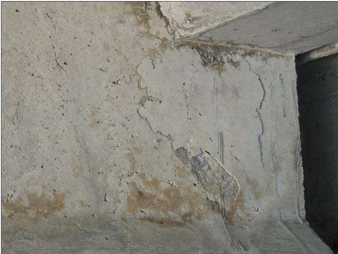
BENT 81 SPAN 82 SIDE DELAMINATED AREA AT THE LT END OF G2 8" X 9".
