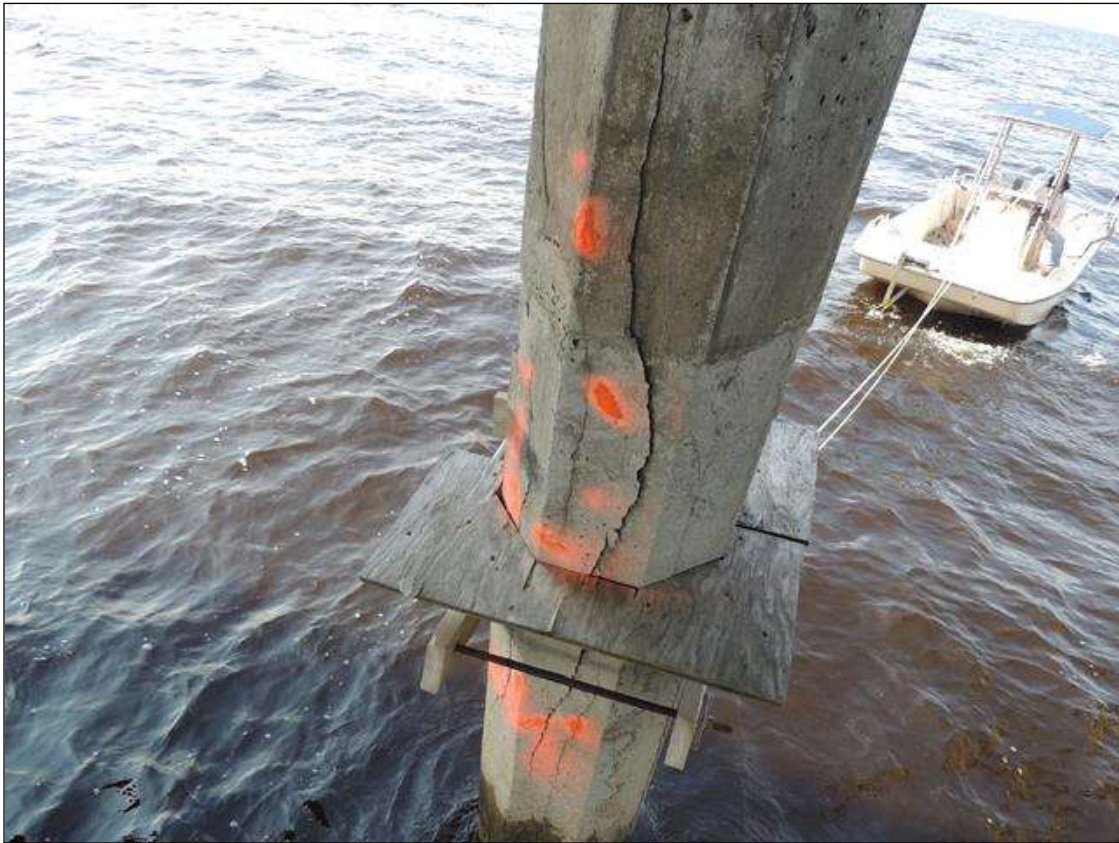
BEN 149 P4 ON THEW NE FACE HAS CRACKED , DELAMINATED AND SPALLED AREA FROM WL TO BOTTOM OF CAP 10' 3" AND 21" AROUND PILE.
