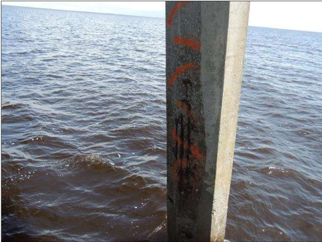
BENT 28 DELAMINATED AND SPALLED AREA ON NORTH FACE OF P4 FROM WL UP 10' 8" TO BOT OF CAP 18" WIDE CABLES EXPOSED PM
