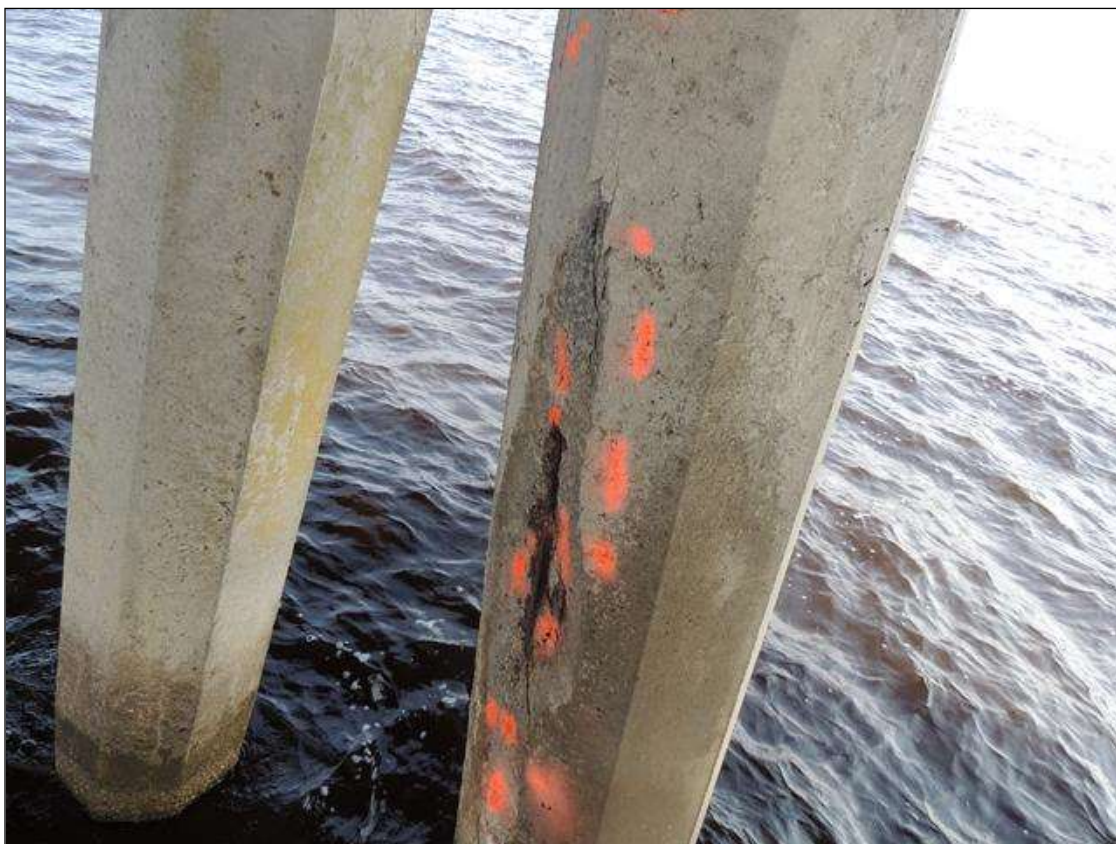
BENT 144 P2 CRACKED, SPALLED AND DELAMINATED AREA FROM THE BOTTOM OF CAP TO WL 9' 8" AND 23" AROUND PILE REBAR EXPOSED PM
