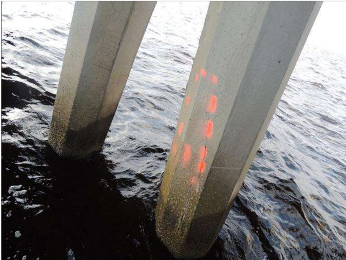
BENT 220 P4 CRACKED AND DELAMINATED AREA ON THE N FACE OF THE PILE 57" FROM THE WATERLINE UP 16" AROUND THE PILE.
