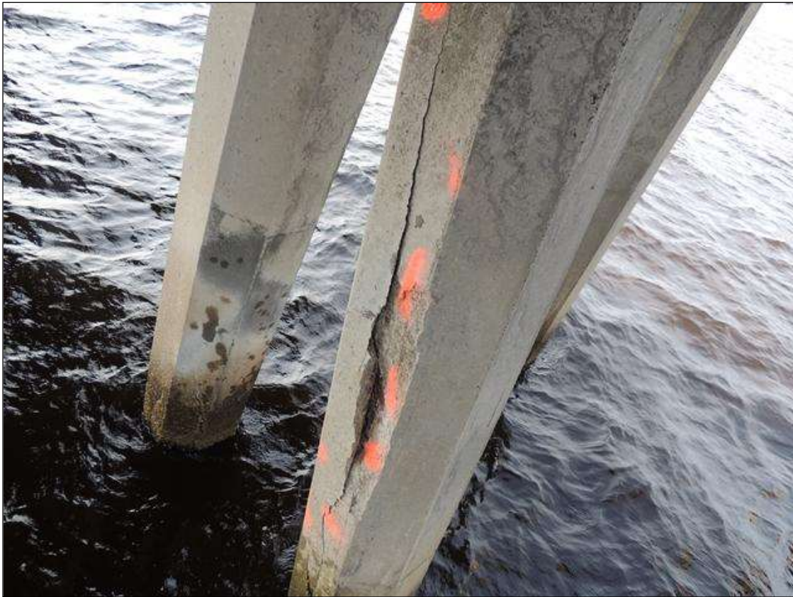
BENT 144 P4 CRACKED AND DELAMINATED AREA 20" AROUND THE PILE 9' 10" FROM THE BOTTOM OF THE CAP DOWN
