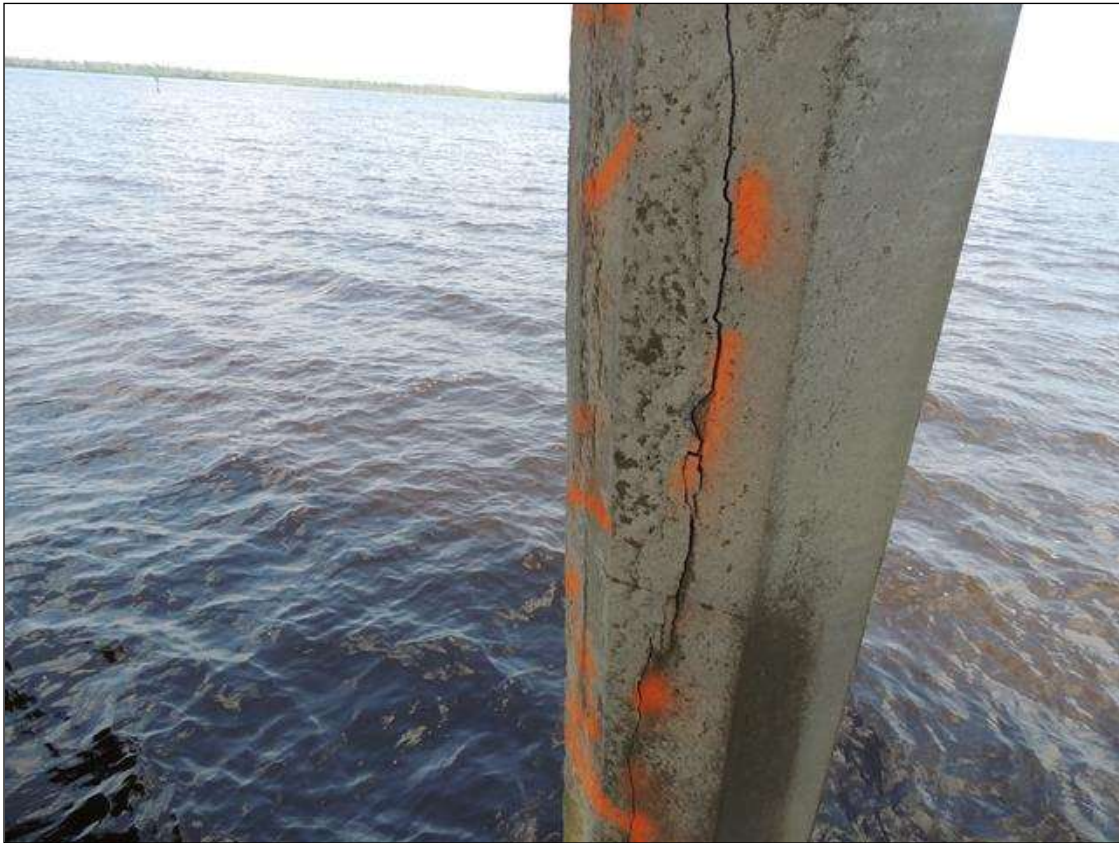
BENT 63 P1 IS CRACKED AND DELAMINATED ON SOUTH FACE FROM BOTTOM CAP TO WL 10' 8" X 21" AROUND PILE.
