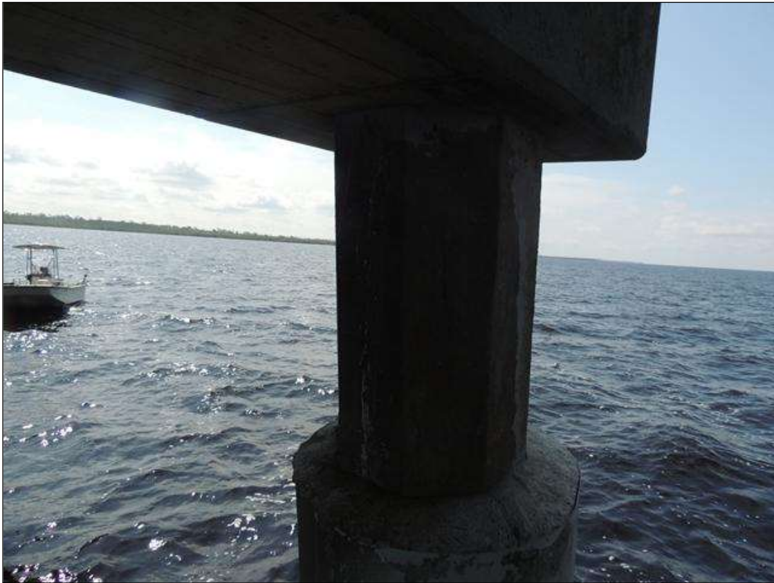
BENT 230 P4 CRACKED AND DELAMINATED AREA ABOVE THE REPAIR 39" FROM THE BOTTOM OF THE REPAIR TO THE CAP 25" AROUND THE PILE
