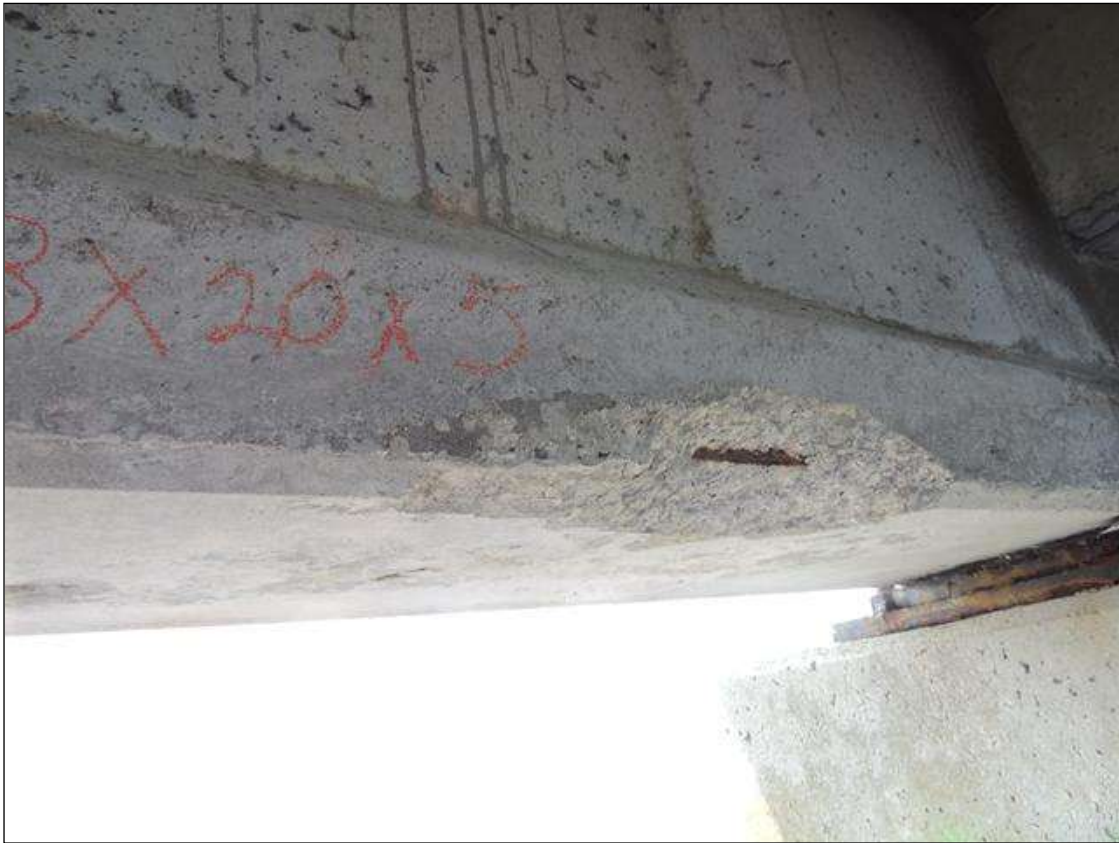
BENT 235 SPAN 236 SIDE SPALLED AREA ON LT SIDE OF G4 3" X 20" X 5" WITH CABLE EXPOSED 14" FROM BENT 235.
