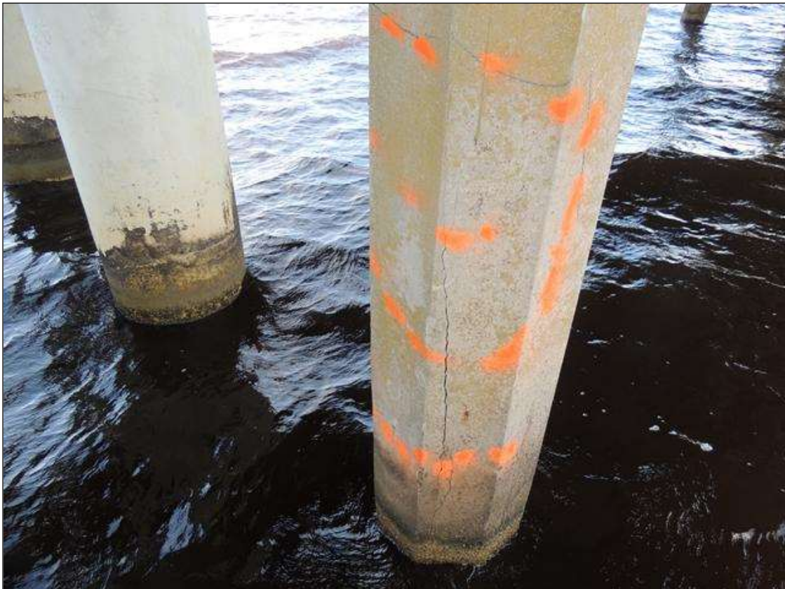
BENT 24 PILE 3 SW FACE IS CRACKED AND DELAMINATED STARTING 5' BELOW BOTTOM CAP EXTENDS TO WL 69" 28" AROUND PILE.
