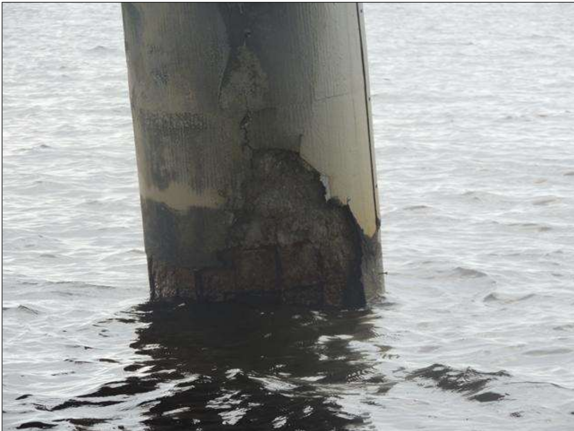
BENT 10 P4 CONCRETE REPAIRED AREA HAS FAILED AND HAS SOME EXPOSED REBAR.
