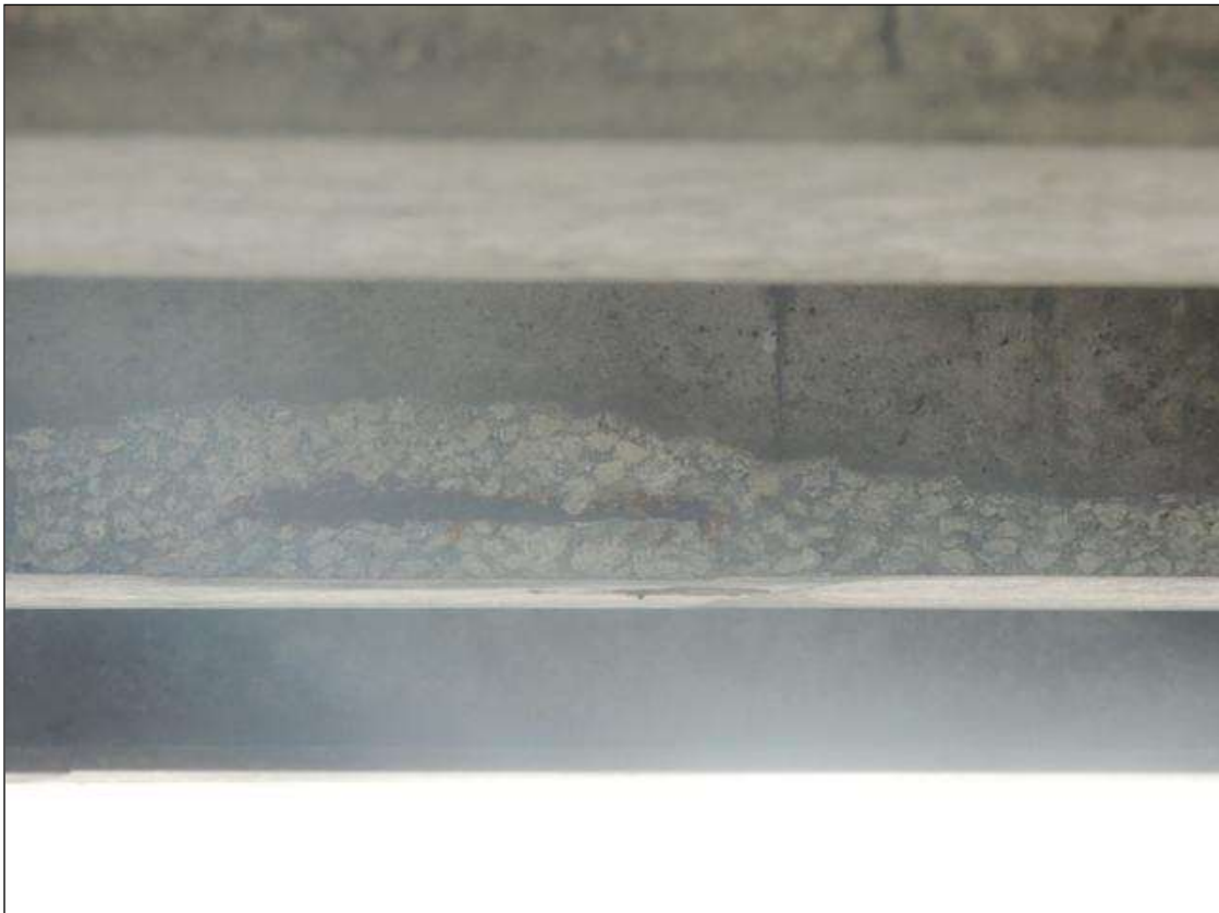
SPAN 4 LT BOTTOM SIDE OF G3 SPALLED ALONG BOTTOM EDGE 4" X 28" X 3" WITH EXPOSED CABLE NEAR MIDSPAN PM
