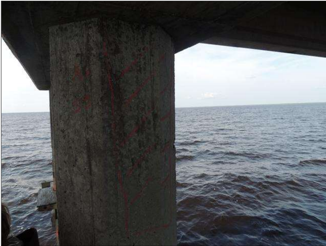
BENT 149 P3 CRACKED AND DELAMINATED AREA ON THE NORTH FACE OF THE PILE FROM BOTTOM OF CAP DOWN 33" X 16" AROUND PILE.
