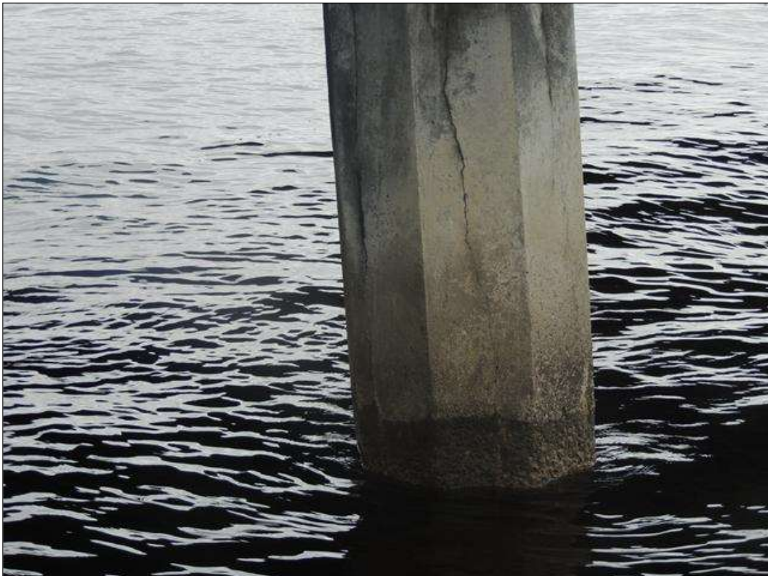
BENT 8 P4 CRACKED AND DELAMINATED AREA IN FACE OF PILE FROM WL TO BOTTOM OF CAP WITH P2 AND 3 SIMILAR.
