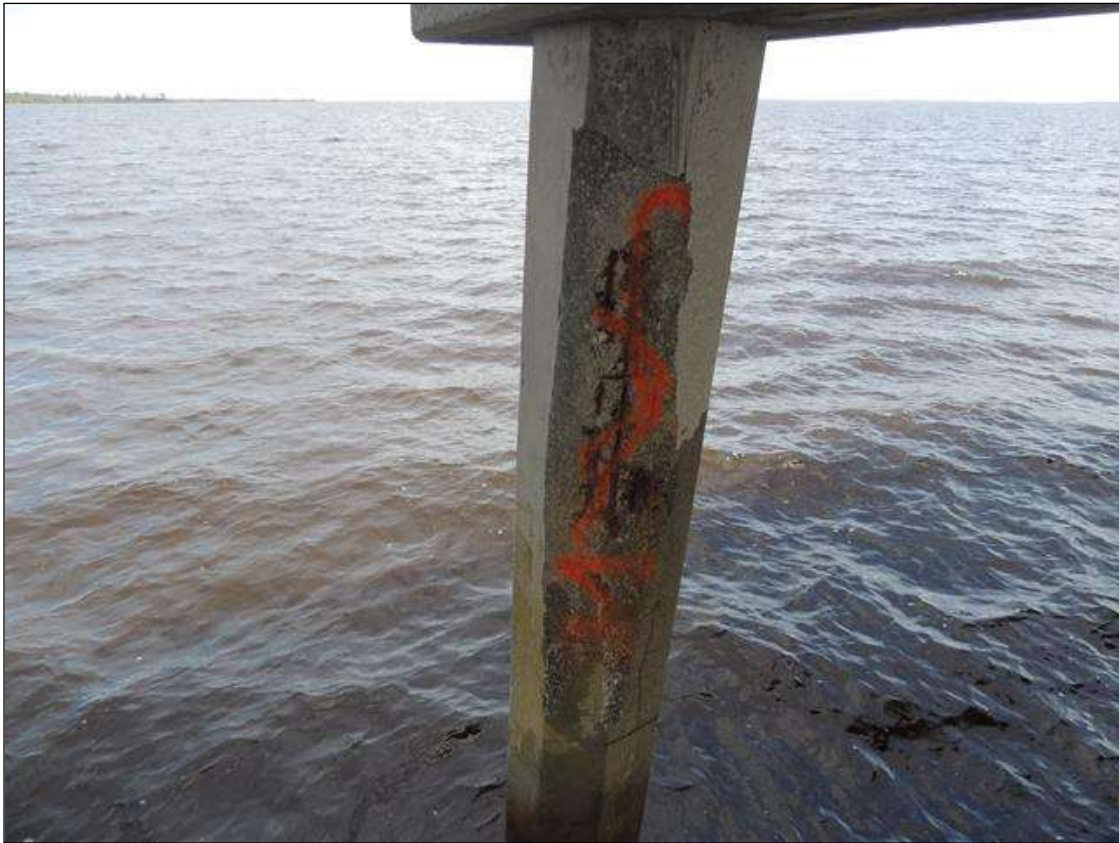
BENT 22 PILE 1 CR ACKED AND SPALLED AREA FROM WL TO BOTTOM OF CAP 11' X 16" AROUND PILE CABLES AND REBAR EXPOSED PM.
