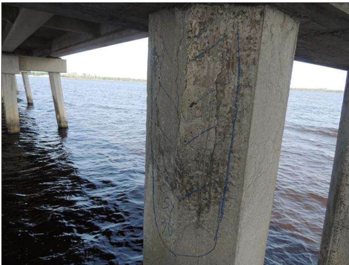
BENT 54 P2 CRACKED AND DELAMINATED AREA AROUND SE CORNER OF PILE FROM BOTTOM OF CAP DOWN 36" X 15" AROUND PILE.
