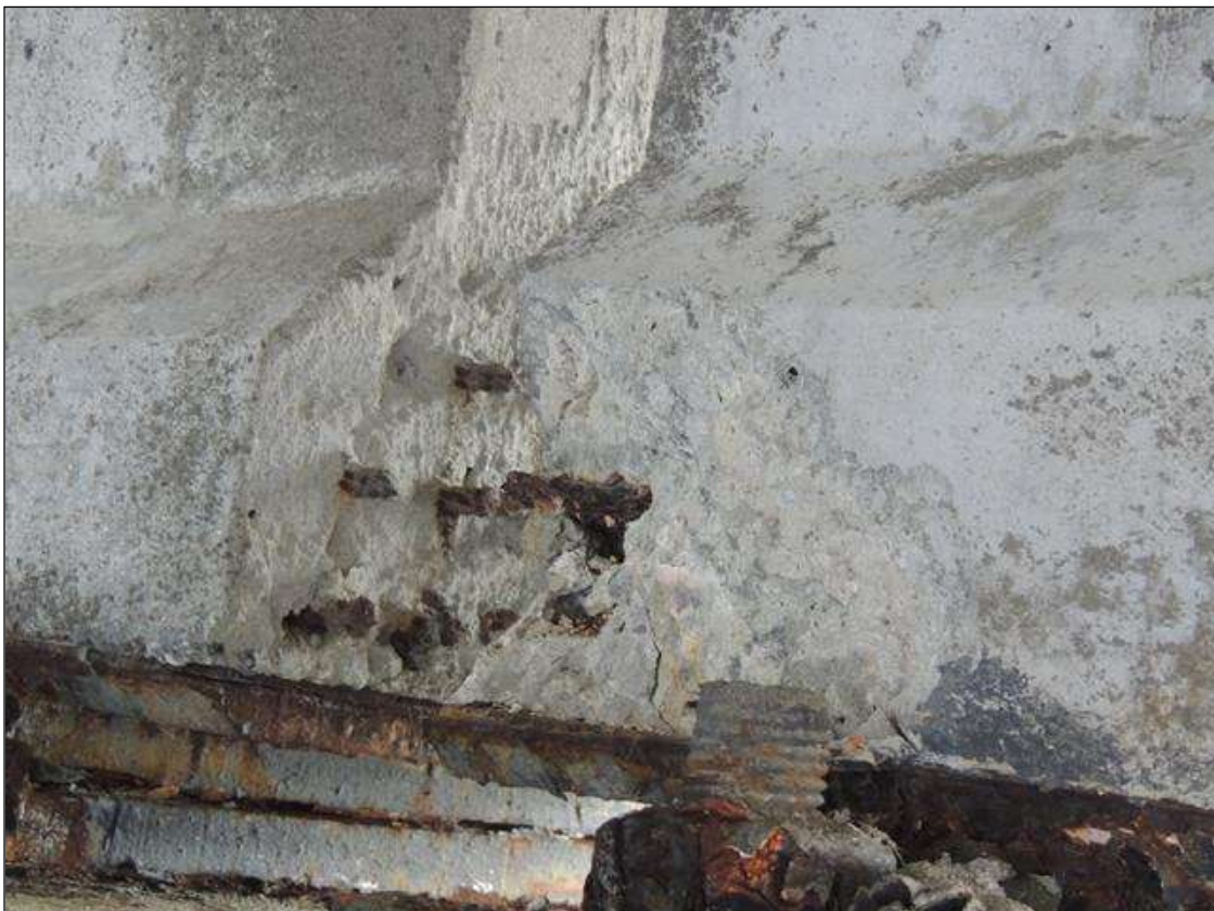
BENT 235 SPAN 235 SIDE SPALLED AREA ALONG THE BOTTOM LT END OF G4 7" X 9" X 3" DEEP CABLES EXPOSED PM.
