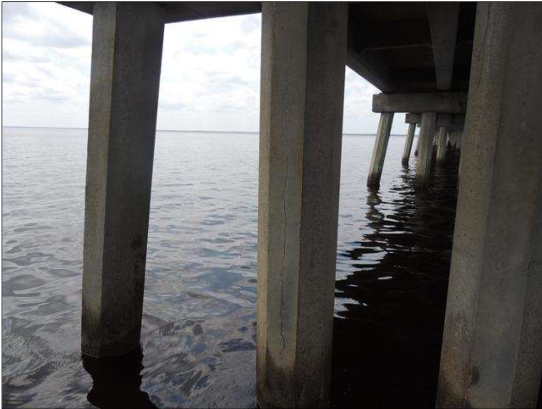
BENT 238 P4 VERTICAL CRACK IN THE EAST FACE OF PILE FROM BOT OF CAP TO WL CRACK AROUND 1/8" WIDE.
