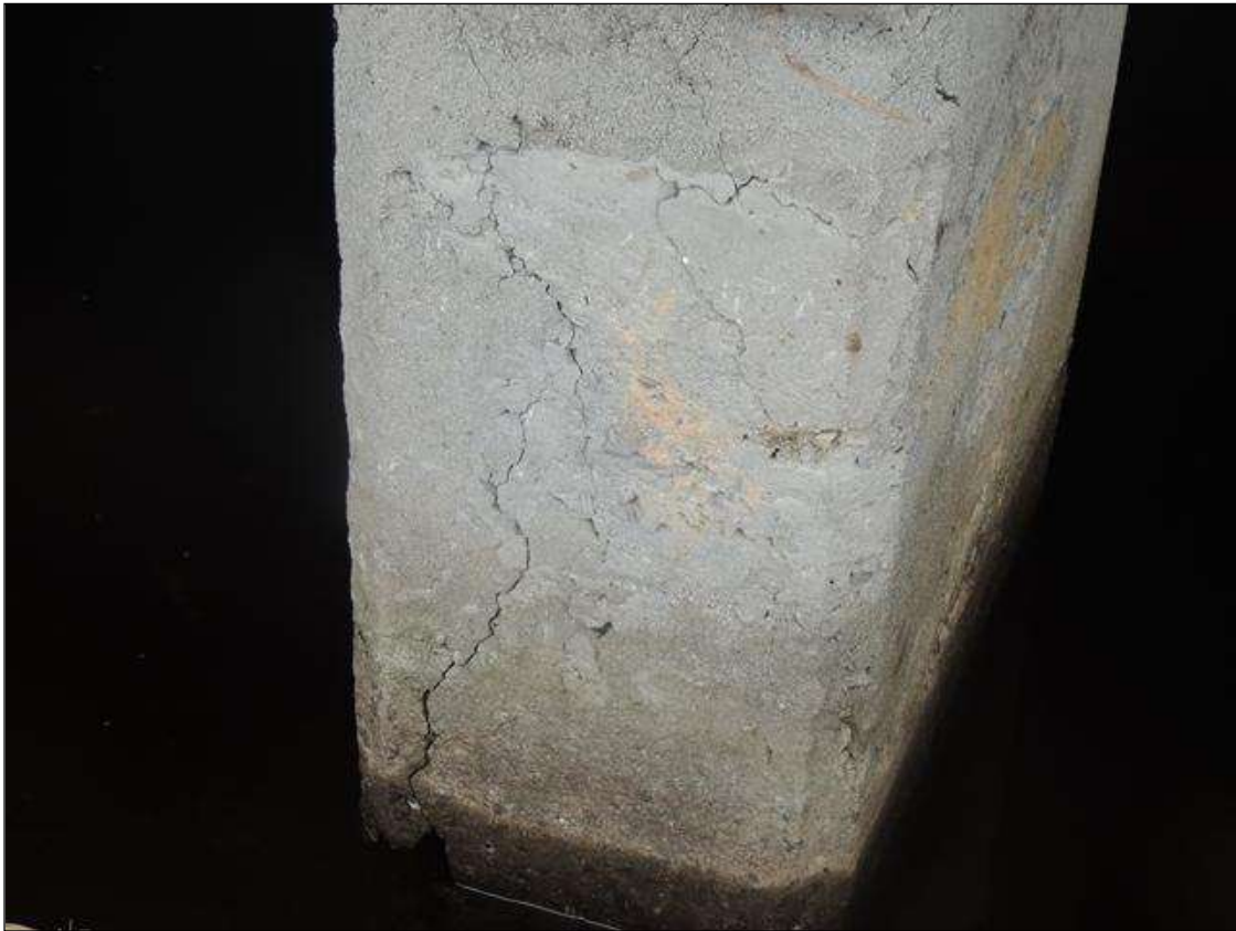
BENT 305 COL 4 CRACKED AND DELAMINATED ALONG RT OUTSIDE EDGE 12" W X 2' H .
