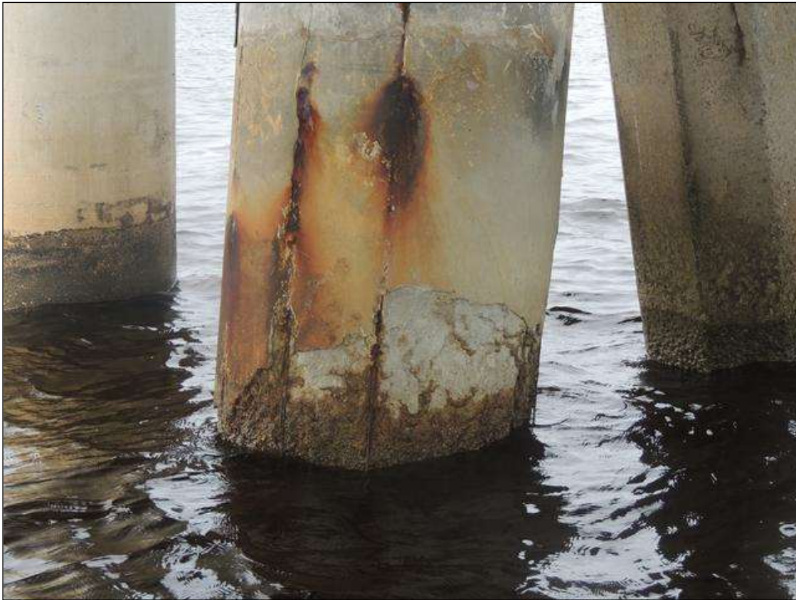
BENT 13 PILE 5 PATCHED AREA IS DETERIORATED AT WL AND HAS REBAR EXPOSED.
