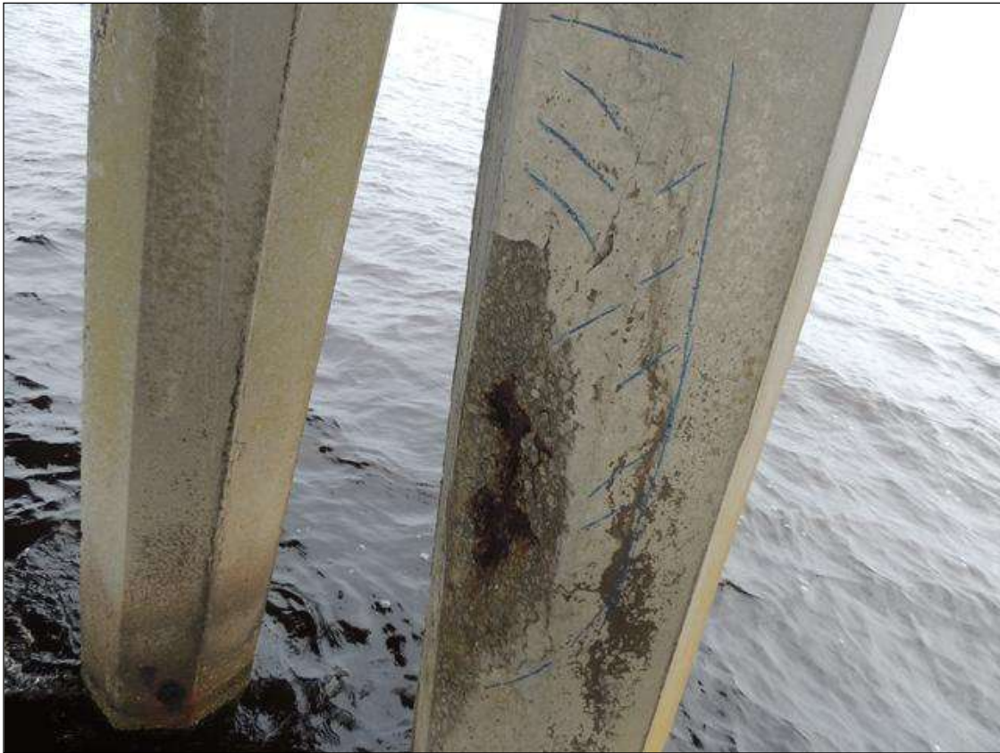
BENT 93 PILE 3 IS SPALLED AND DELAMINATED UNDER BOTTOM SUBCAP 1 STARTS 23" UNDER CAP 59" LONG X 17" W X 2" DEEP REBAR EXPOSED PM.
