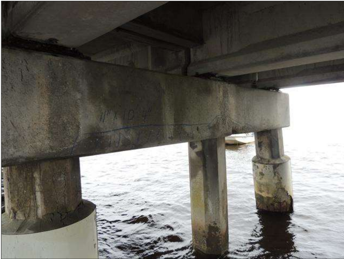
BENT 10 SPAN 10 SIDE DELAMINATED AND SPALLED AND CRACKED AREA ALONG THE BOTTOM FACE OF CAP FROM G2 TO RT SIDE G3 11" X 10' 4".
