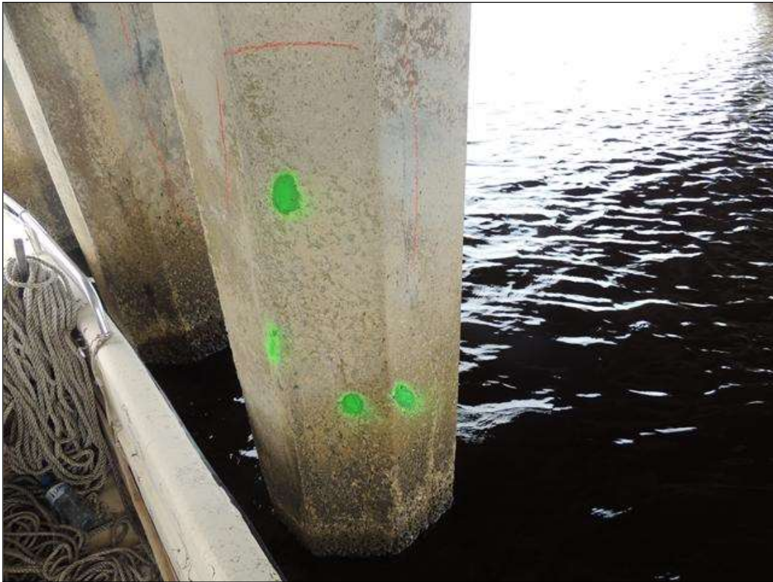
BENT 266 N EAST FACE OF P4 CRACKED AND DELAMINATED AREA FROM WL UP 52" X 18" AROUND PILE.
