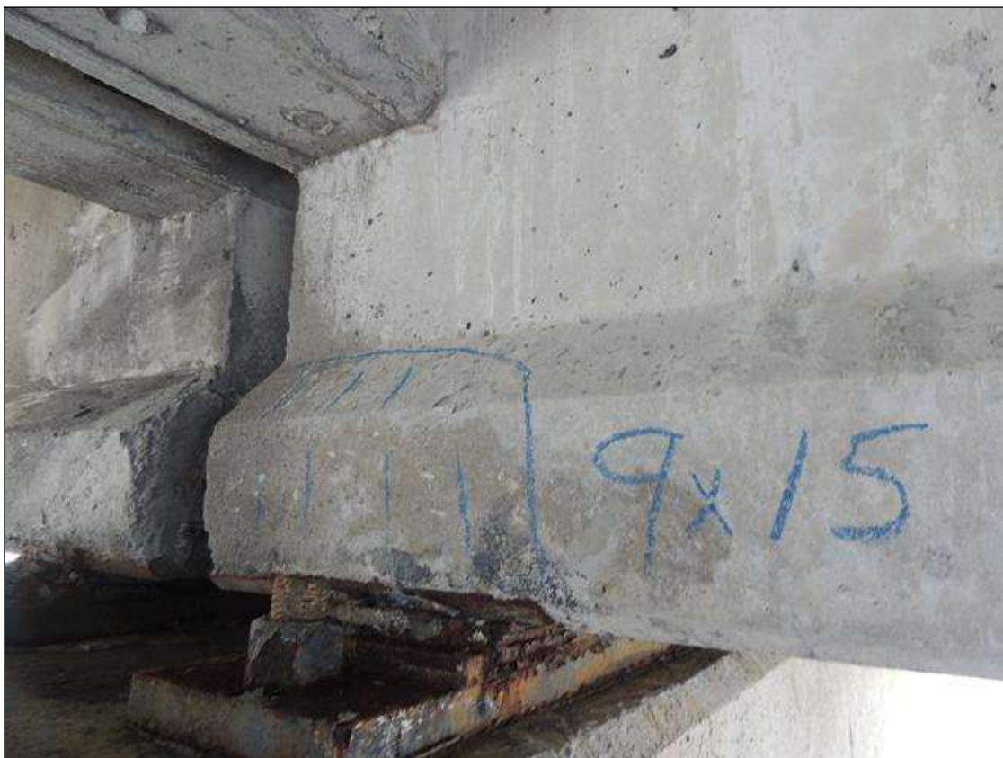
BENT 55 SPAN 55 SIDE CRACKED AND DELAMINATED AREA ALONG THE BOTTOM SIDE OF G3 9" X 15".
