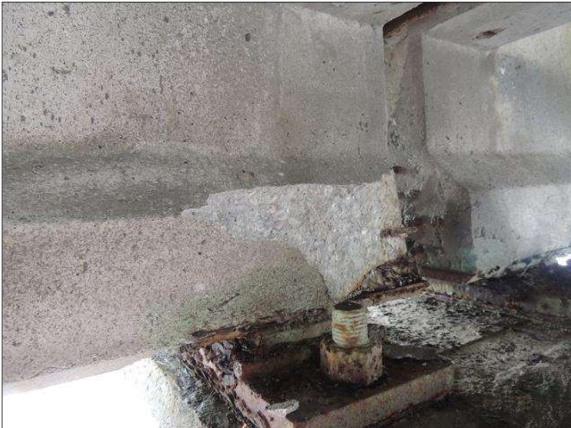
BENT 10 SPAN 10 SIDE SPALLED AREA ON THE RT SIDE OF G1 7" X 14" X 2" DEEP.
