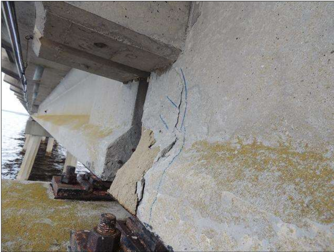
BENT 36 SPAN 36 SIDE PATCHED AND DELAMINATED AREA ALONG BOT LT END OF G1 18" H X 12" FROM END BACK.
