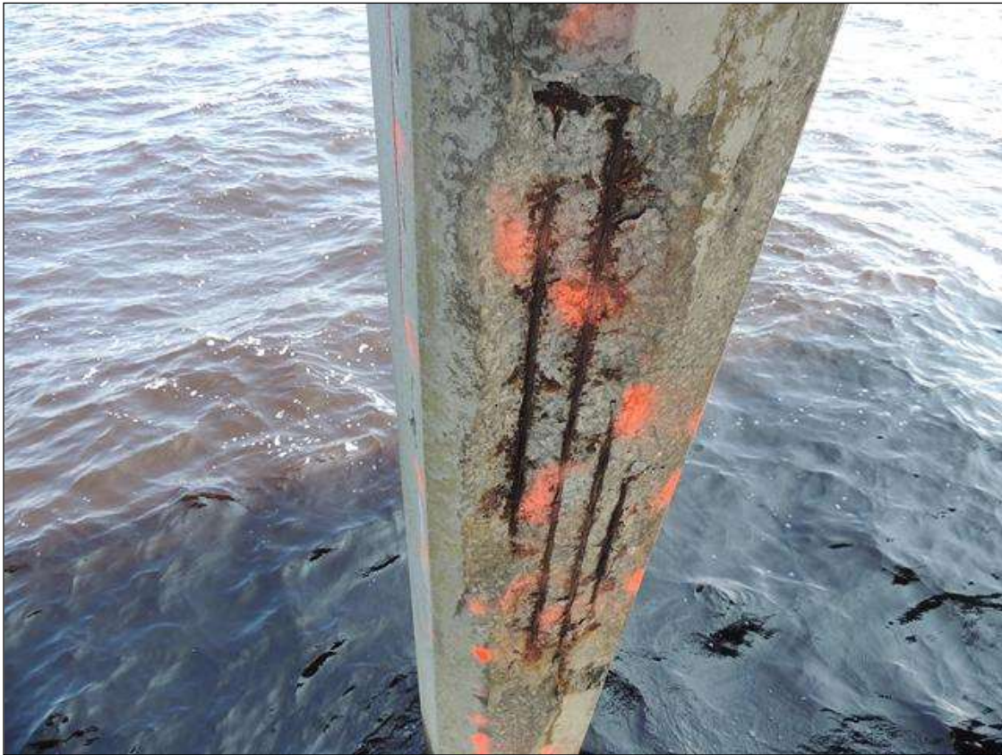
BENT 231 CRACKED SPALLED AND DELAMINATED AREA ALONG THE S FACE OF P1 10'2" FROM THE WATERLINE TO THE BOTTOM OF THE CAP 4 CABLES EXPOSED 3 BROKEN CABLE
