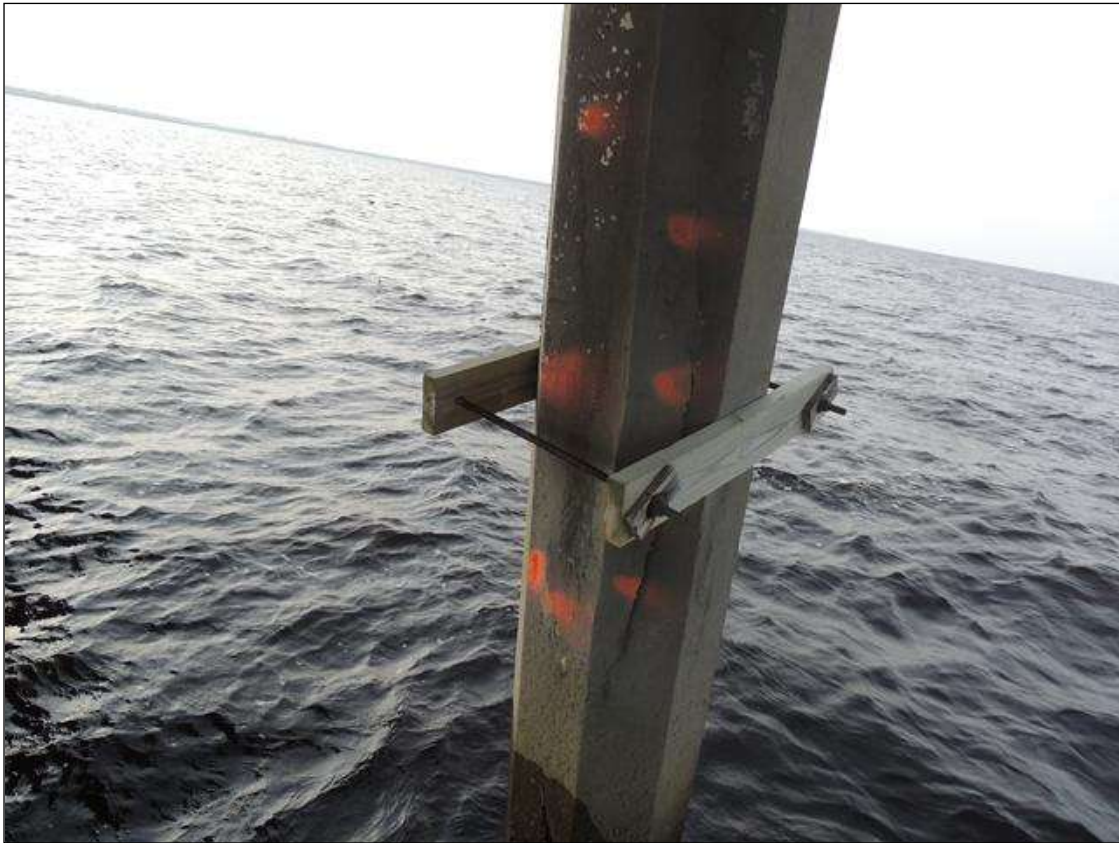
BENT 139 P4 CRACKED AND DELAMINATED AREA ON THE N FACE OF THE PILE 8' 1" FROM THE WATERLINE UP, 18" AROUND THE PILE
