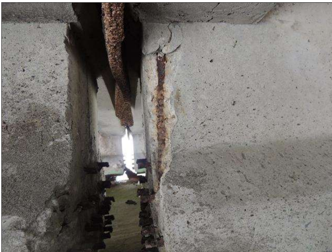
BENT 9 SPAN 9 SIDE SPALLED AREA ALONG END OF G3 4" W AND FROM DIAPHRAGM DOWN 10" X 1 1/2" DEEP REBAR EXPOSED.
