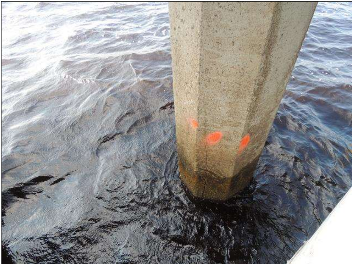
BENT 222 P4 CRACKED AND DELAMINATED AREA 30" FROM THE WATERLINE UP 18" AROUND THE PILE.
