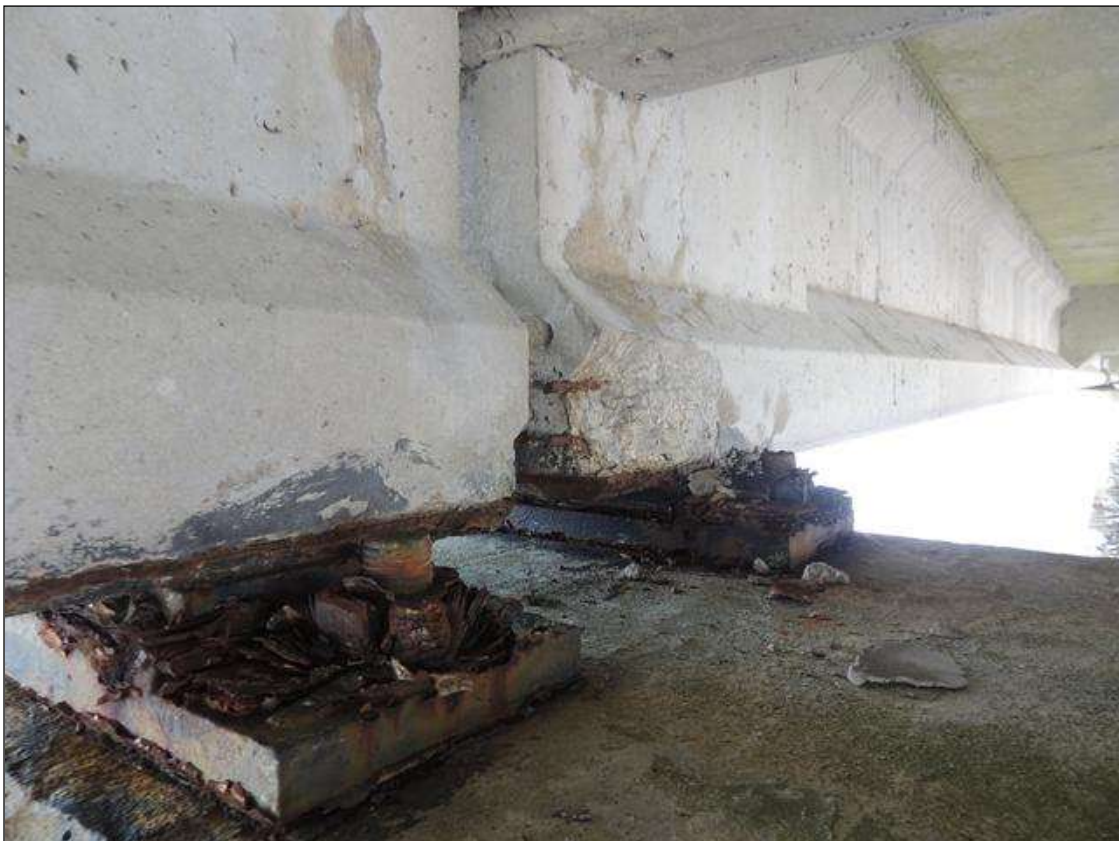
BENT 244 SPAN 245 SIDE SPALLED AREA ALONG THE LT BOTTOM SIDE OF G1 6" X 9" X 1 1/2" DEEP .
