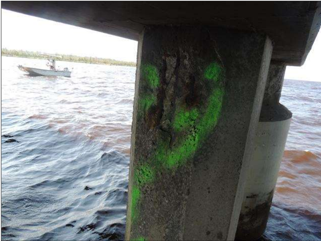
BENT 265 P5 CRACKED, SPALLED AND DELAMINATED AREA ON NORTH FACE OF PILE FROM BOTTOM CAP DOWN TO WL 75" X 18" AROUND PILE WITH 3 CABLES EXPOSE PM
