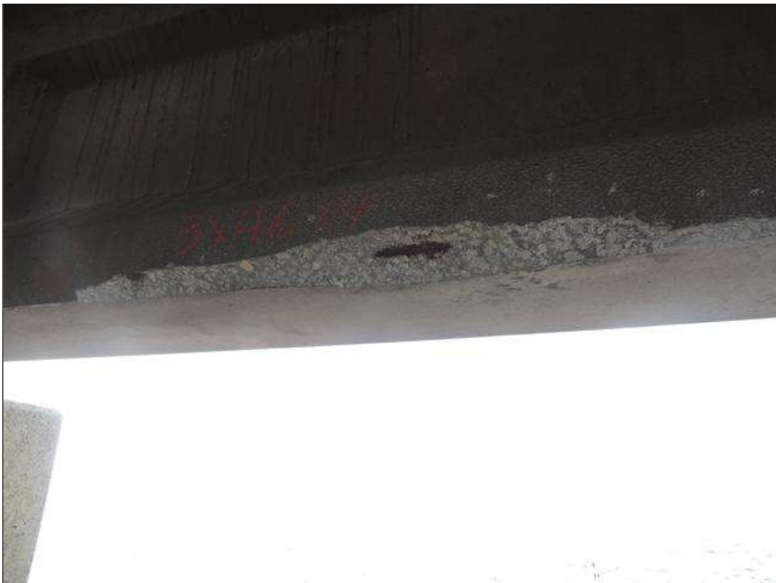
SPAN 144 SPALLED AREA ALONG THE BOTTOM LT SIDE OF G4 3' FROM BENT 144, 3" X 46" X 4"
