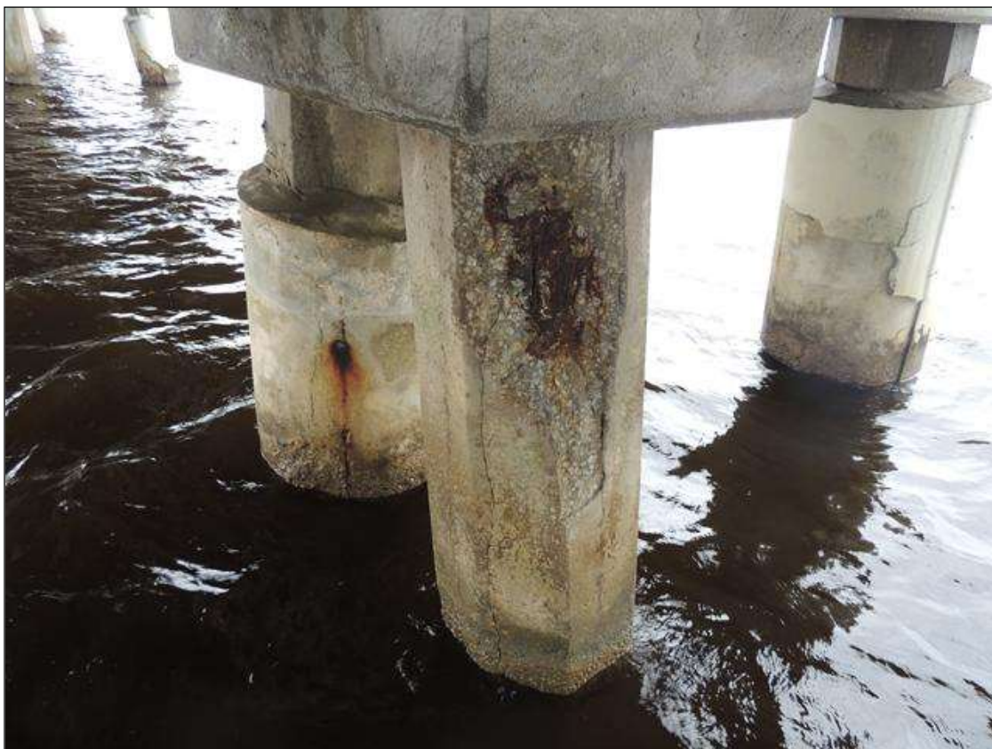
BENT 9 PILE HAS A CRACKED AND SPALLED AREA UNDER G3 17" X 39" X 3" DEEP WITH CABLES EXPOSED.
