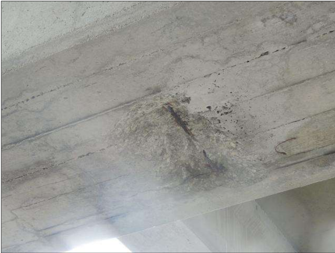
BENT 15 BOTTOM OF THE CAP BETWEEN P1 AND P2 IS SPALLED 18" X 24" X 4" DEEP WITH EXPOSED REBAR.
