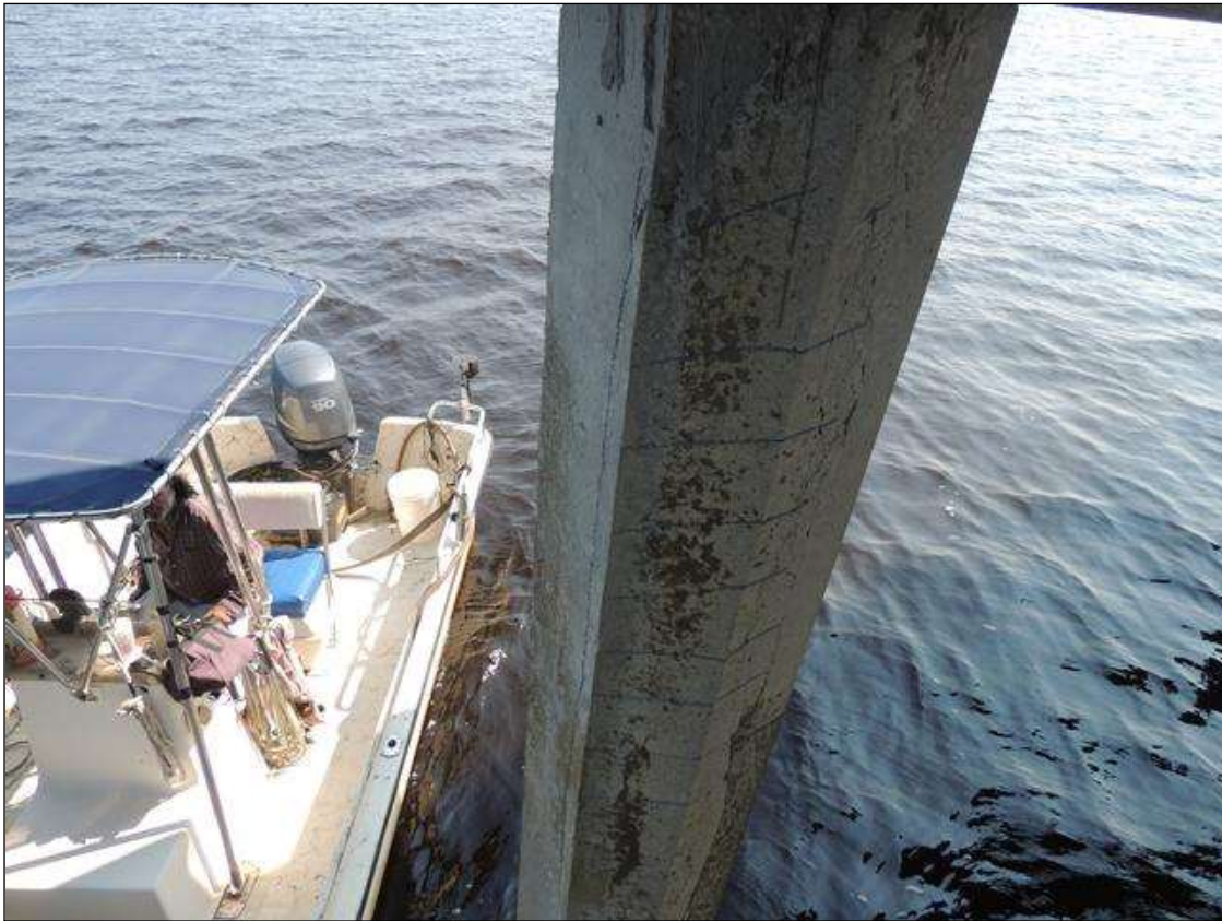
BENT 53 P1 CRACKED AND DELAMINATED AREA ON THE SOUTH FACE OF PILE FROM BOTTOM CAP TO WL 10' 6" X 17" AROUND PILE.
