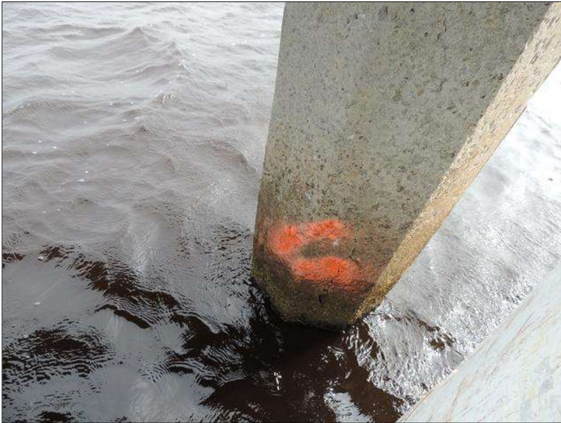
BENT 134 LARGE CRACK AND DELAMINATED AREA ON THE N FACE OF P4 28" FROM WL UP AND 14" AROUND PILE.
