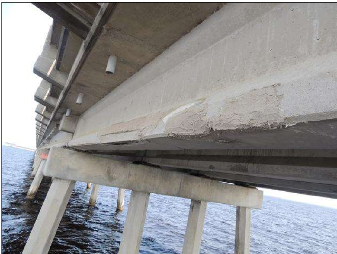
SPAN 147 SCATTERED PATCHED AREAS ALONG BOTOM R SIDE OF G4.
