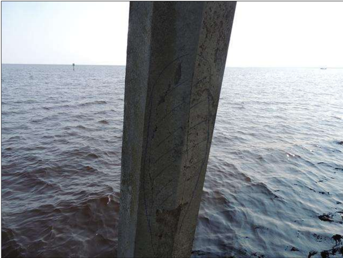
BENT 52 P1 CRACKED AND SPALLED AND DELAMINATED AREA ON SOUTH FACE OF PILE STARTS 33" BELOW BOT CAP AND EXTENDS 68" X 17" W X 1 3/4" DEEP.
