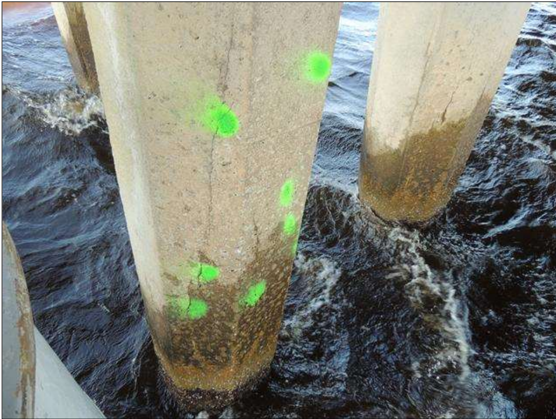
BENT 260 P5 CRACKED AND DELAMINATED AREA FROM THE WATER LINE UP 50" AND 18" AROUND PILE ON NORTH SIDE..
