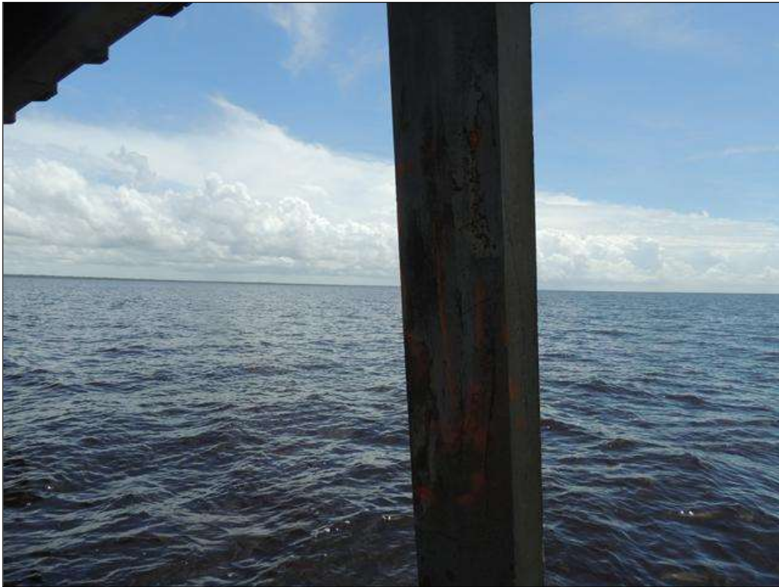
BENT 24 P4 CRACKED AND DELAMINATED AREA FROM THE BOT OF CAP DOWN 8' 3" 29" AROUND PILE.
