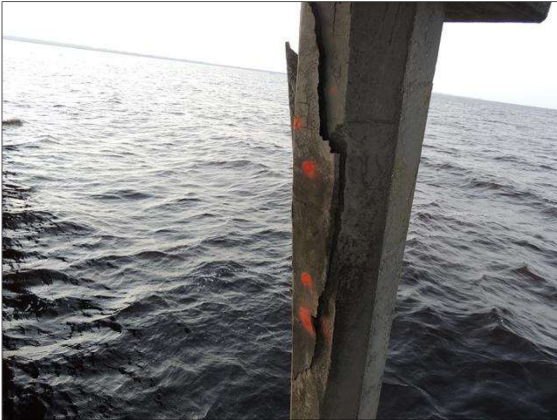
BENT 140 P6 CRACKED, SPALLED, AND DELAMINATED AREA, 10' X 6" FROM THE BOTTOM OF CAP TO WL, 26" AROUND THE PILE, REBAR AND CABLES EXPOSED
