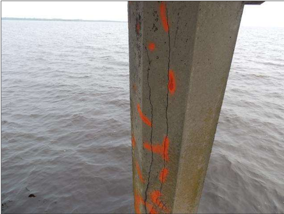
BENT 98 PILE 1 CRACKED AND DELAMINATED AREA ON THE SOUTH FACE OF PILE FROM BOTTOM CAP DOWN 75" X 18" AROUND PILE.
