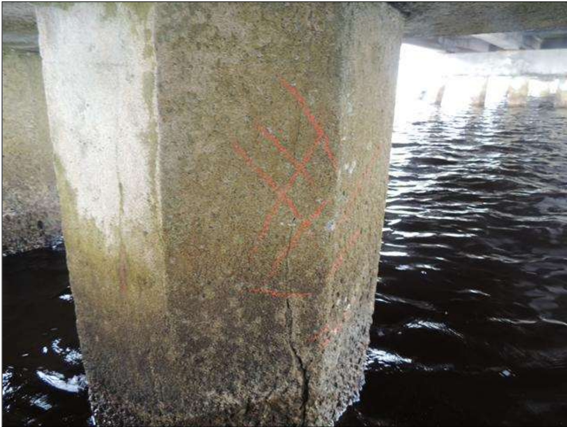
BENT 270 P3 CRACKED AND DELAMINATED AREA 14" AROUND PILE AND 27" FROM TOP TO WL WITH PILES 1,2,5 AND 6 SIMILAR.
