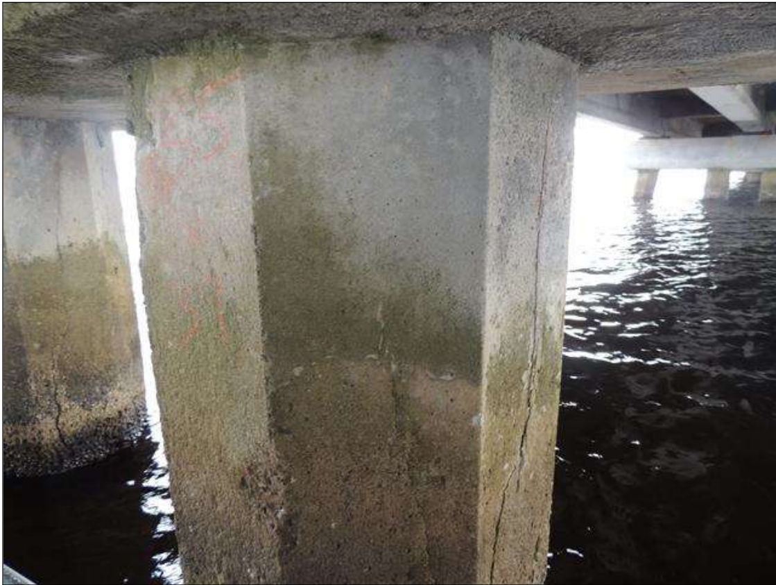
BENT 269 P3 CRACKED AND DELAMINATED FROM TOP DOWN TO WL 32" AROUND PILE AND 39" DOWN PILES 1 AND 2 AND 4 AND 5 SIMILAR.
