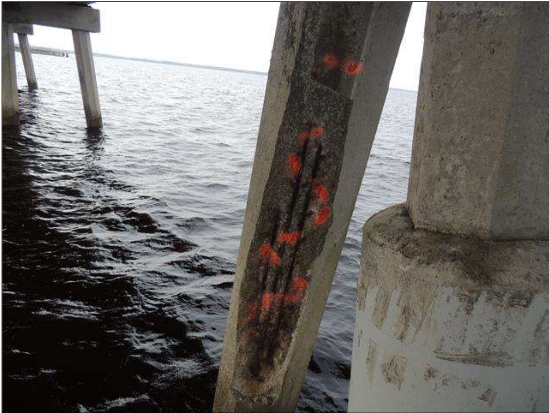
BENT 132 P2 IS CRACKED AND DELAMINATED AND SPALLED FROM THE BOTTOM OF SUBCAP TO WL 124" AND 15" AROUND PILE 3 CABLES EXPOSED PM.
