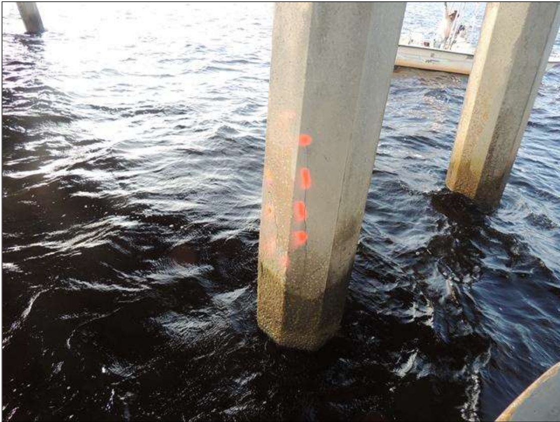
BENT 213 P3 CRACKED AND DELAMINATED AREA ON THE N FACE OF THE PILE, 55" FROM THE WATERLINE UP 14" AROUND THE PILE
