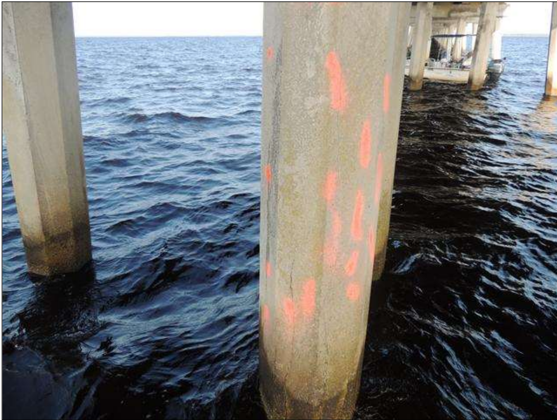
BENT 216 P5 CRACKED AND DELAMINATED AREA ALONG THE E FACE OF THE PILE 78" FROM THE WATERLINE UP 32" AROUND THE PILE
