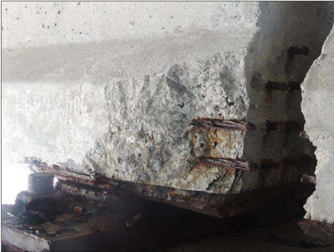
BENT 217 SPAN 218 SIDE SPALLED AREA ALONG THE BOTTOM LT END OF G2 8" X 10" X 2" DEEP CABLE EXPOSED PM.
