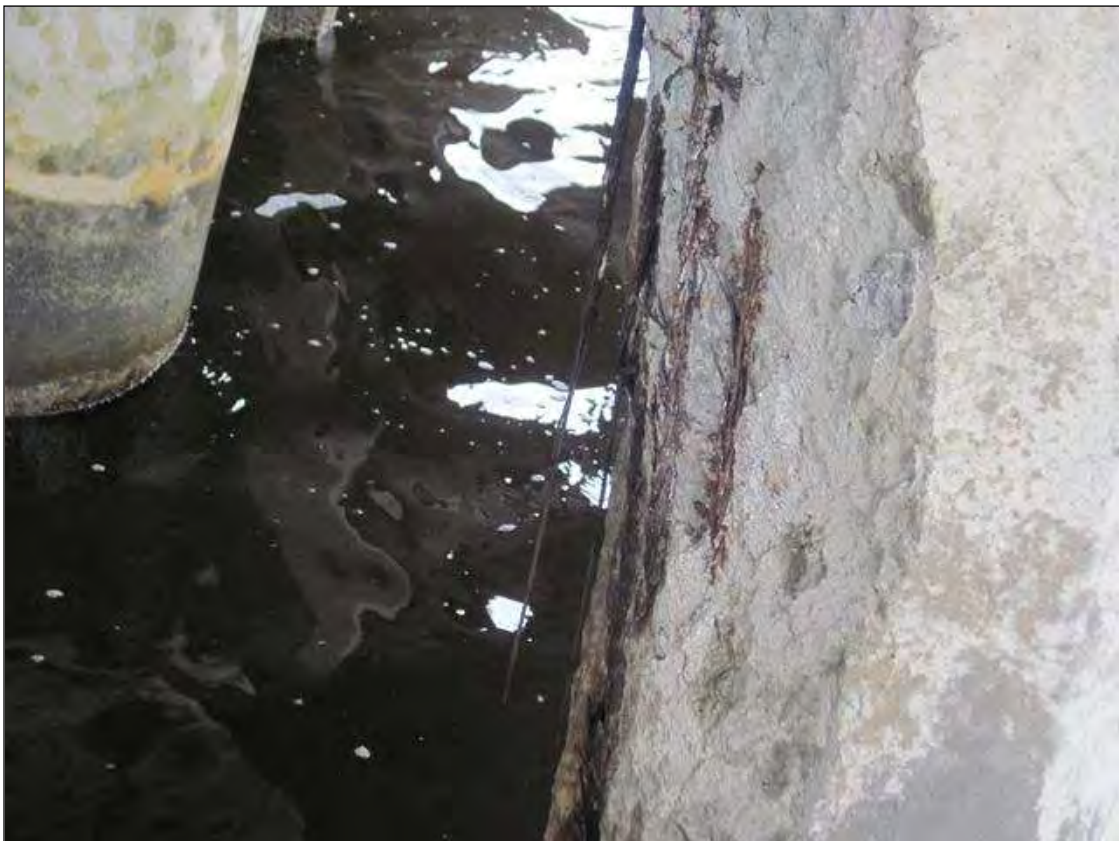
REST BENT 2, P-10, SPALLED W/ EXPOSED STRANDS (50%-100% LOSS) FROM CAP TO W/L, FACES 1,2,7,8.
