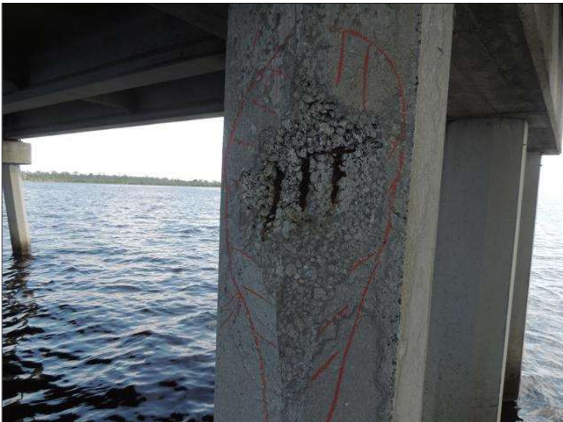
BENT 246 P2 SPALLED AND DELAM AREA ON THE NORTH FACE OF PILE STARTS 7" BELOW BOT OF CAP GOES DOWN 37" X 17" AROUND PILE W 3 CABLES EXPOSED PM
