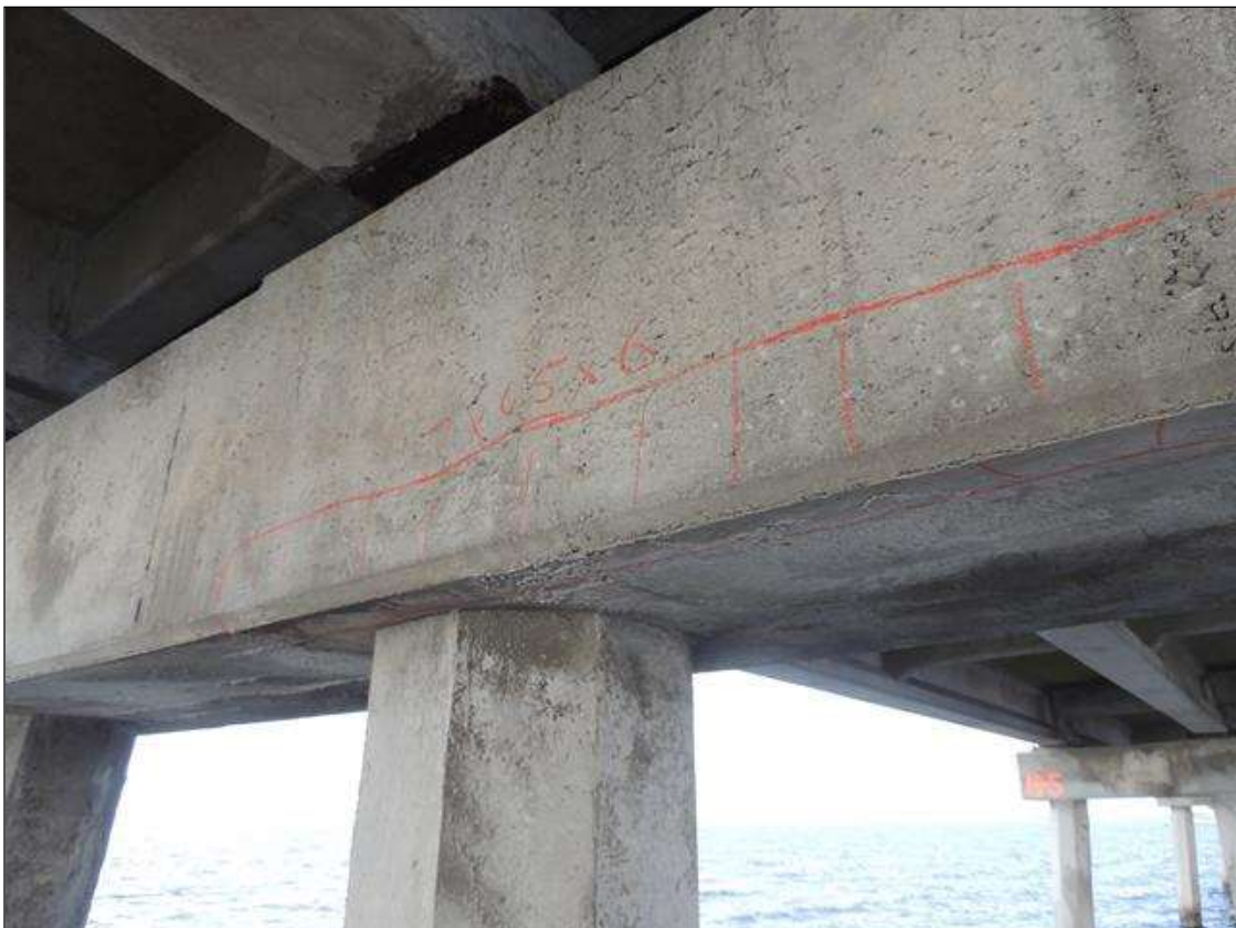
BEN 146 SPAN 147 SIDE CRACKED AND DELAMINATED AREA ALONG THE BOTTOM FACE AND BOTTOM OF THE CAP UNDER G3 7' X 65" X 12" UNDER BOTOM.
