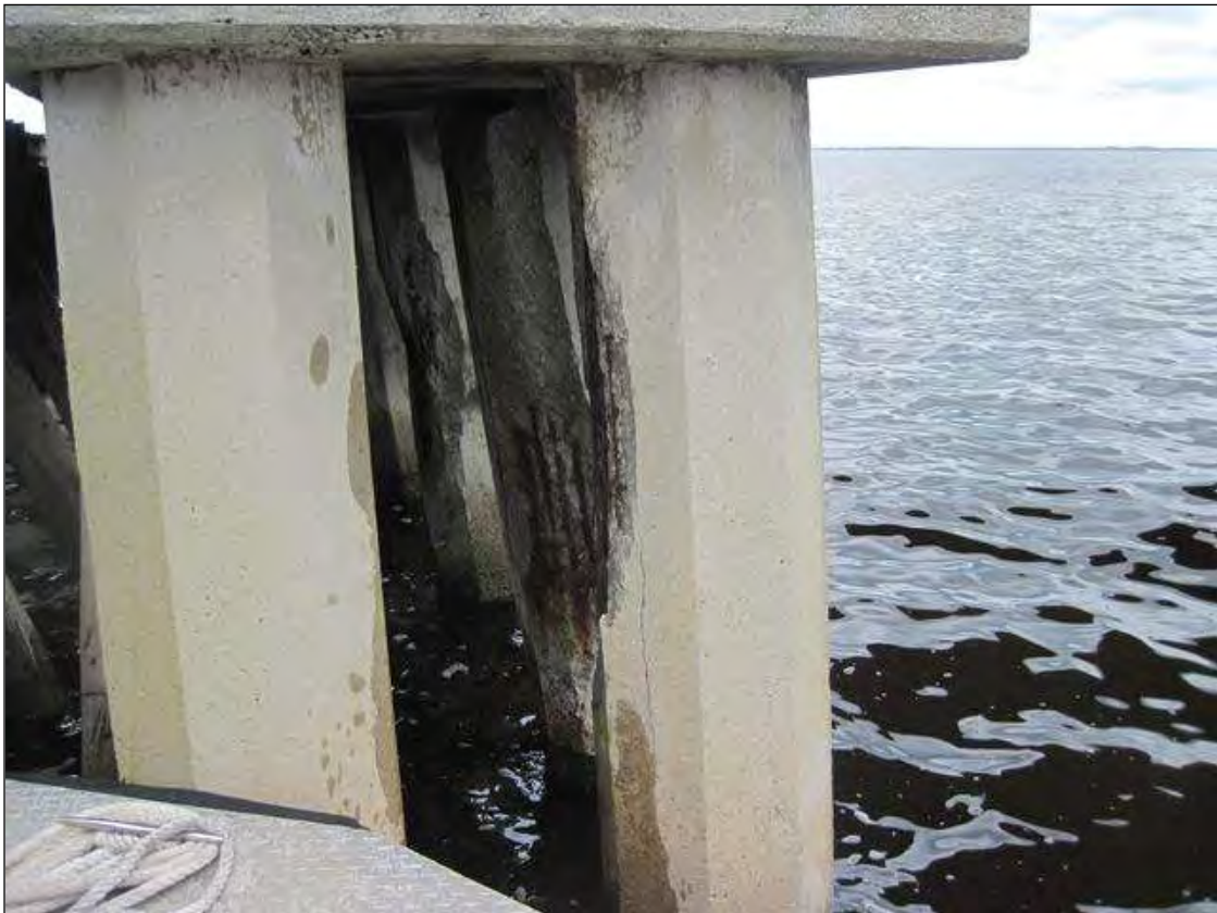
REST BENT 2, P-14, SPALLED W/ EXPOSED STRANDS (50%-100% LOSS) FROM CAP TO W/L, FACES 1,2,8.
