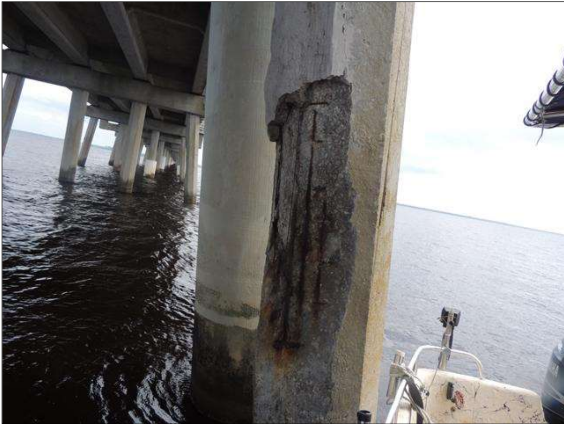
BENT 116 CRACKED AND SPALLED AND DELAMINATED AREA ON P7 WITH CABLES EXPOSED 6' 6" H X 28" AROUND PILE PM
