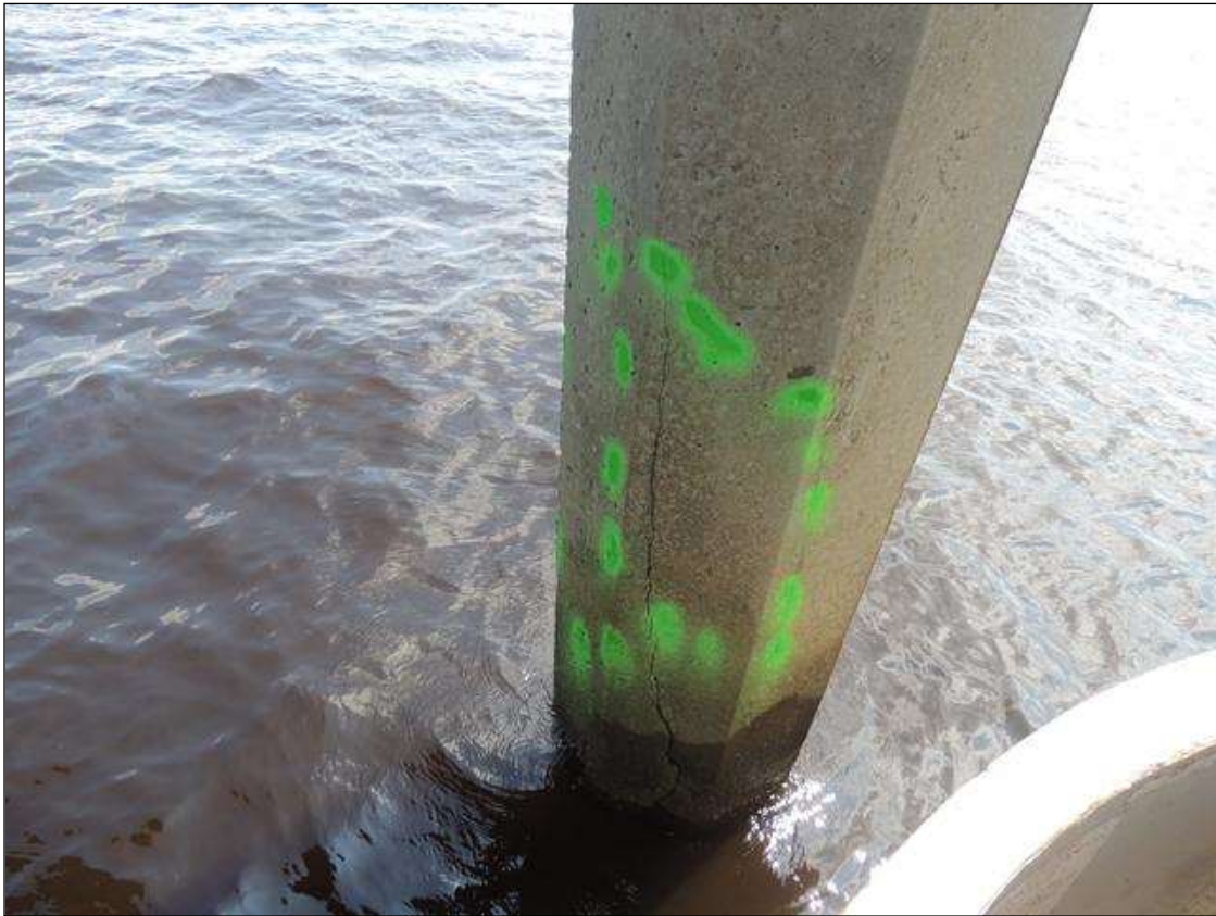
BENT 244 P6 CRACKED AND DELAMINATED AREA ALONG NE FACE FROM WL UP 41" X 21" AROUND PILE.
