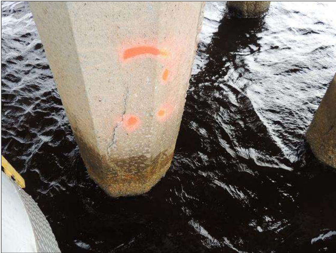
BENT 136 P3 CRACKED AND DELAMINATED AREA ON THE N FACE OF PILE FROM WL UP 41" X 16" AROUND PILE.
