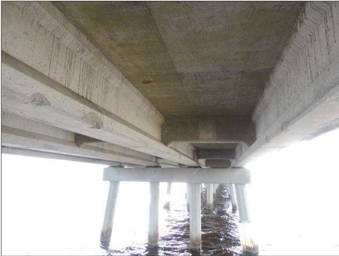
SPAN 147 SCATTERED SURFACE SPALLED AREAS ON BOOM EDGES OF G2 , G3 AND G4 .
