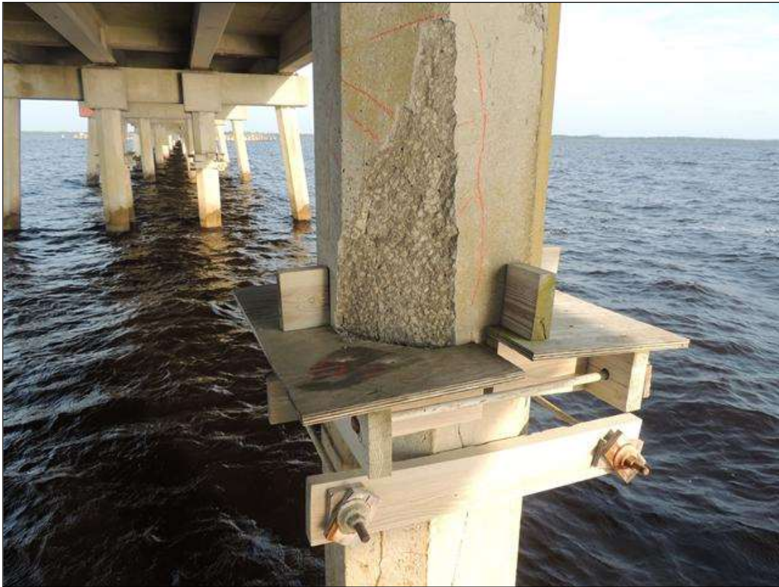
BENT 137 PILE 2 CRACKED AND DELAMINATED AREA ON THE NE FACE OF THE PILE 18" AROUND, 9' 2" FROM THE WATERLINE UP
