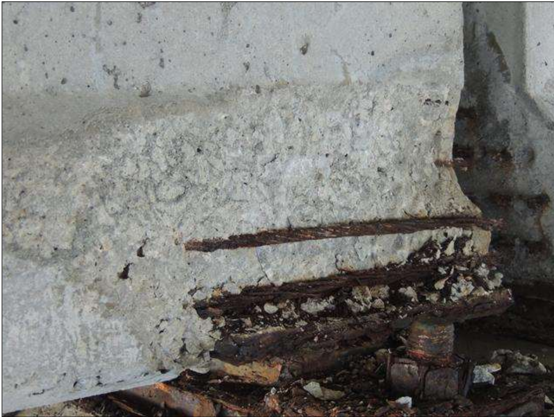
BENT 240 SPAN 241 SIDE SPALLED AREA ALONG THE LT BOTTOM END OF G2 10" X 24" L X 2 1/2" DEEP CABLES EXPOSED PM.
