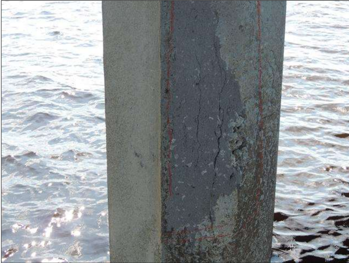
BENT 249 P3 PATCHED AREA IS CRACKED AND DELAM AND HONEYCOMBED STARTING 55" BELOW BOT OF CAP GOES 30" DOWN AND 14" WIDE ON NORTH FACE.
