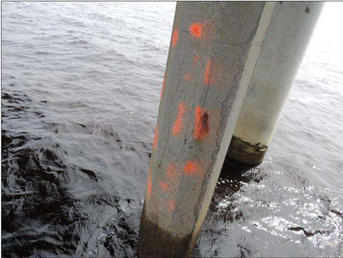
BENT 126 PILE 3 CRACKED AND DELAMINATED AREA ON THE N FACE OF PILE STARTS 3' ABOVE WL AND GOES UP 4' AND 16" AROUND PILE.
