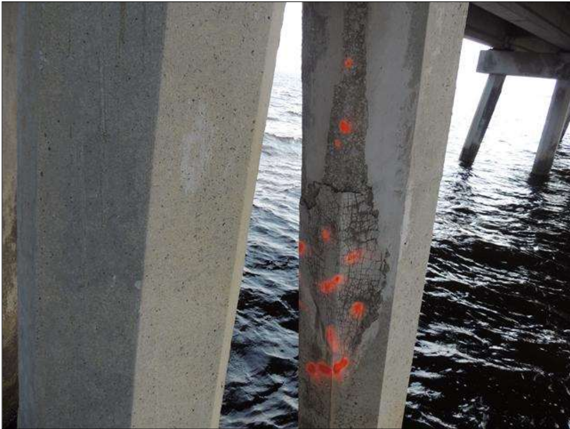
BENT 148 P5 IS CRACKED , DELAM AND SPALLED ON THE WEST FACE FROM BOTTOM OF CAP DOWN 72" AND 21" AROUND PILE.
