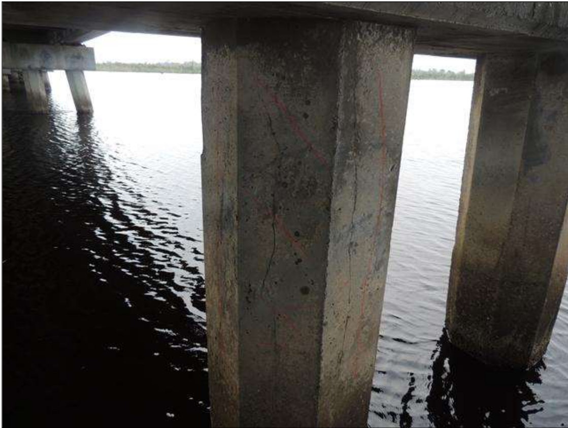
BENT 266 CRACKED AND DELAMINATED AREA ON THE WEST FACE OF PILE FROM BOT CAP TO WL 75" X 18" AROUND PILE.
