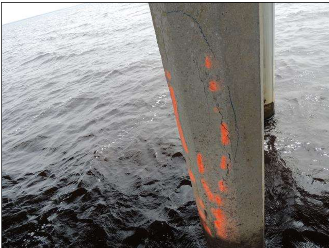
BENT 125 PILE 3 IS CRACKED AND DELAMINATED ON N FACE OF PILE FROM THE WL UP 90" .
