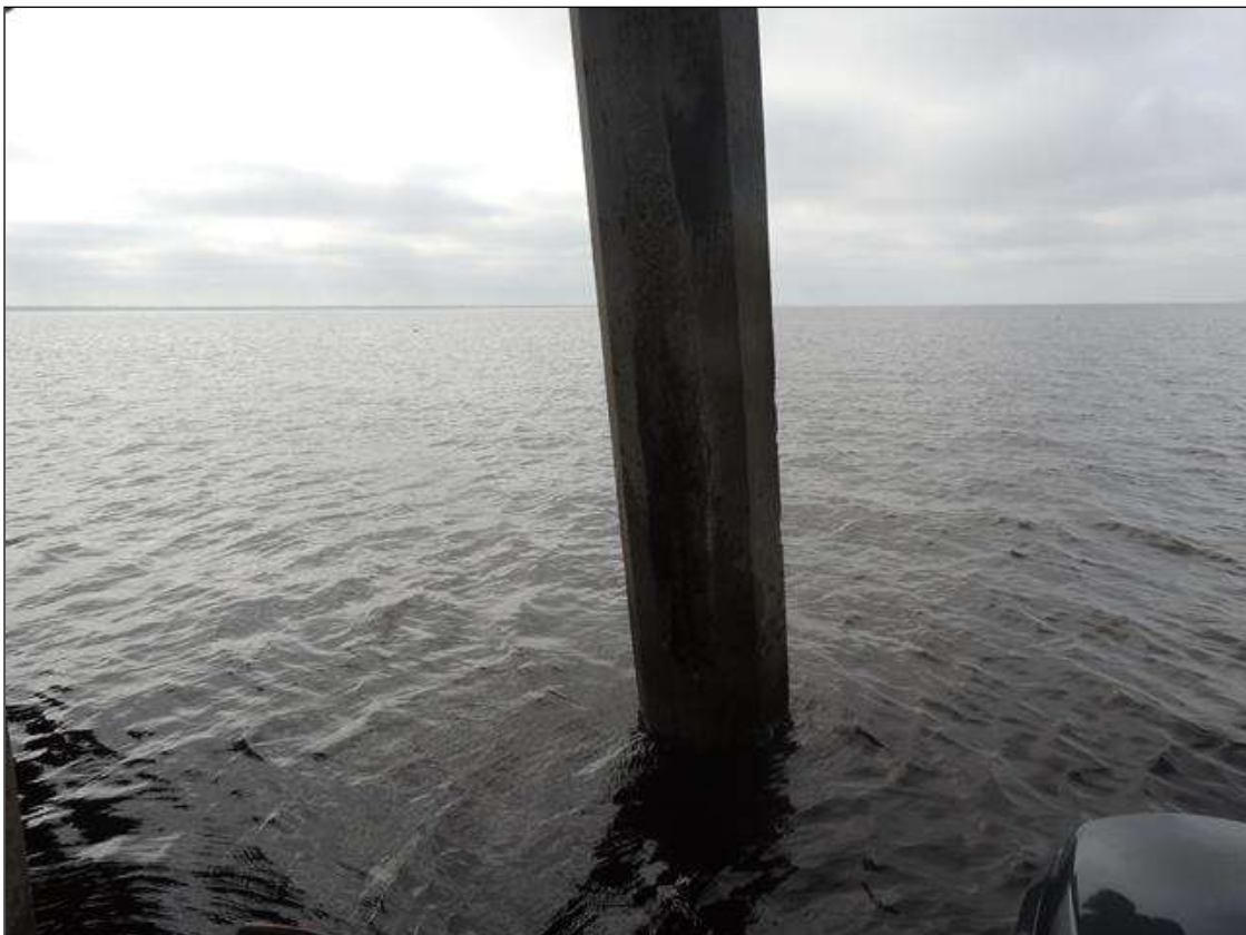
BENT 14 P4 SPALLED AREA FROM BOTTOM OF CAP TO WL 108" X 14" WIDE REBAR EXPOSED PM
