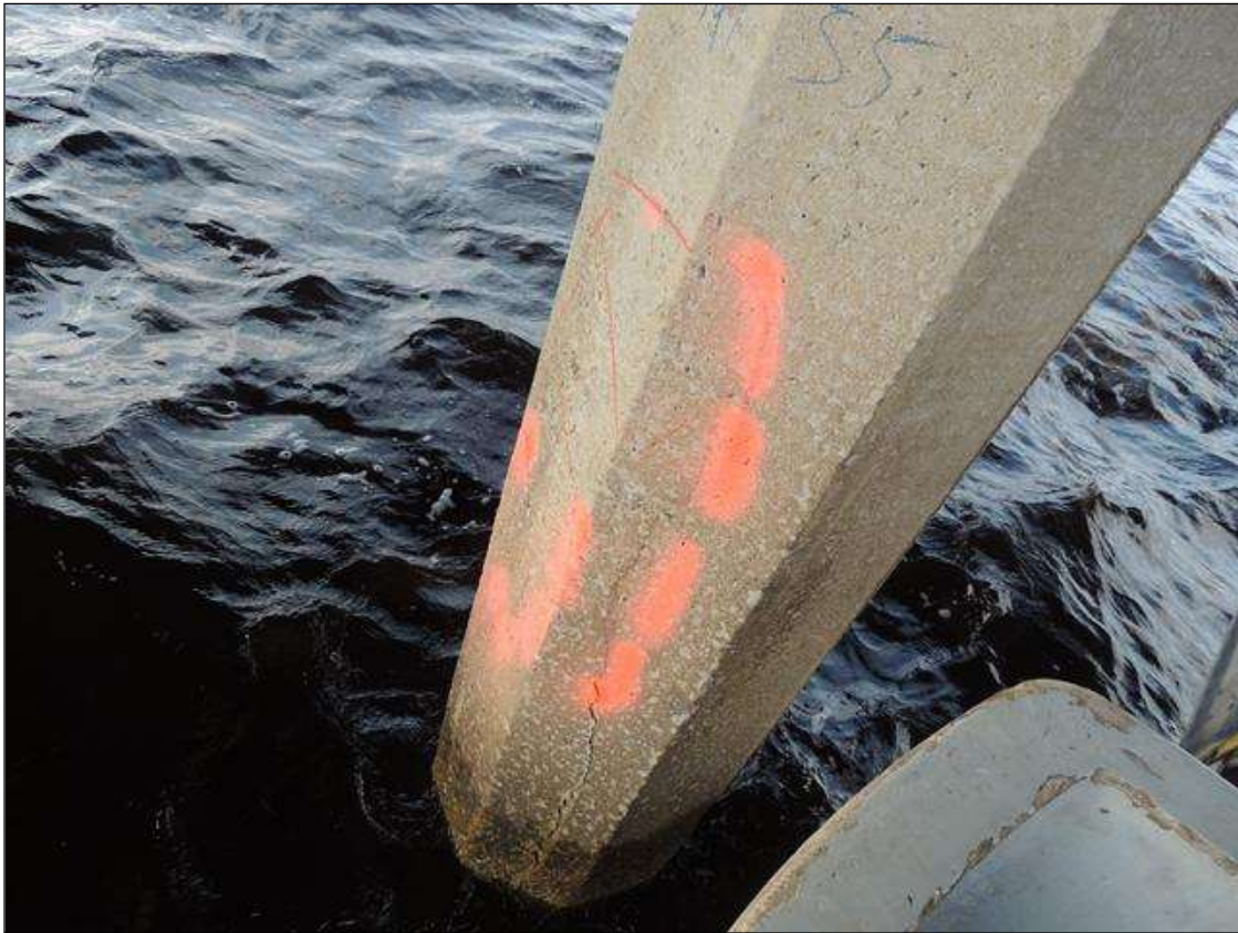
BENT 221 P2 CRACKED AND DELAMINATED AREA ON THE N FACE OF THE PILE 55" FROM THE WATERLINE UP 14" AROUND THE PILE.
