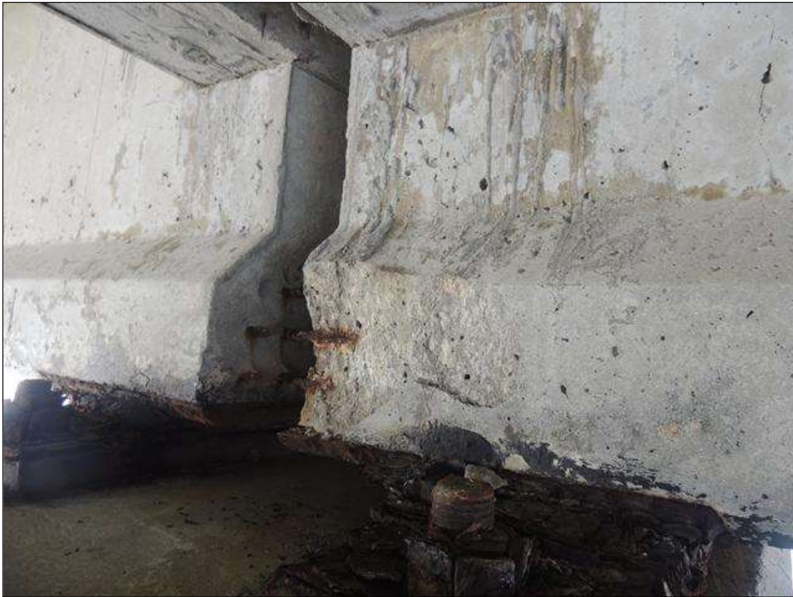
BENT 222 SPAN 222 SIDE SPALLED AREA ALONG THE LT BOTTOM END OF G3 7" X 9" X 2" DEEP CABLE EXPOSED PM.
