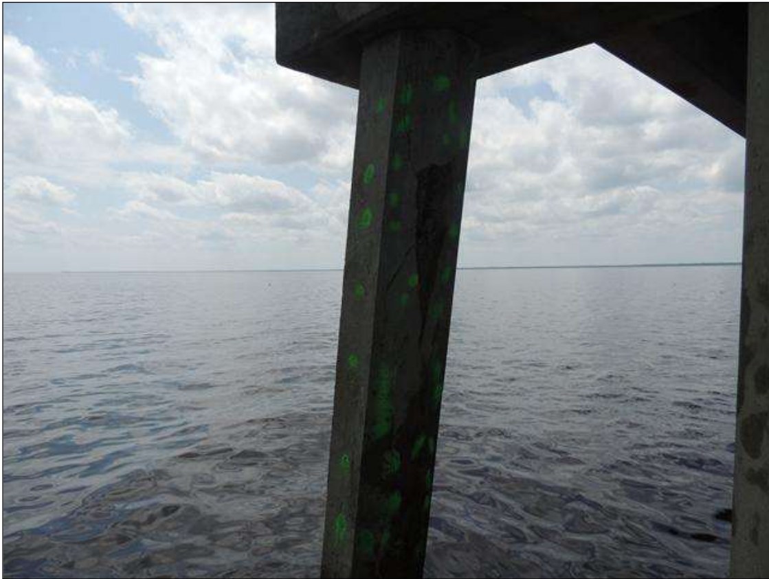
BENT 237 P5 CRACKED, DELAM, SPALLED AREA FROM BOT CAP TO WL 10' 4" X 25" AROUND PILE WITH 2 CABLES EXPOSED AND 3" DEEP NORTH FACE PM.
