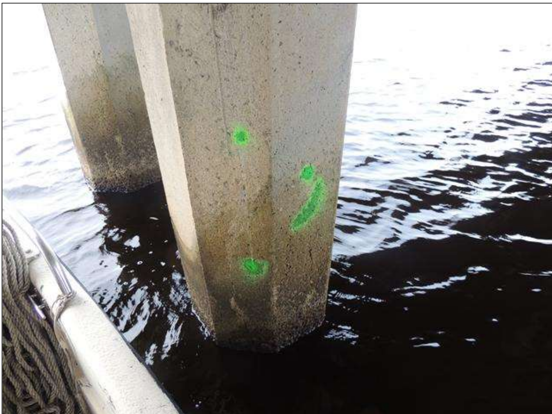
BENT 267 P5 CRACKED AND DELAMINATED AREA ON SPAN 268 SIDE FROM WL UP 48" X 16" AROUND PILE.
