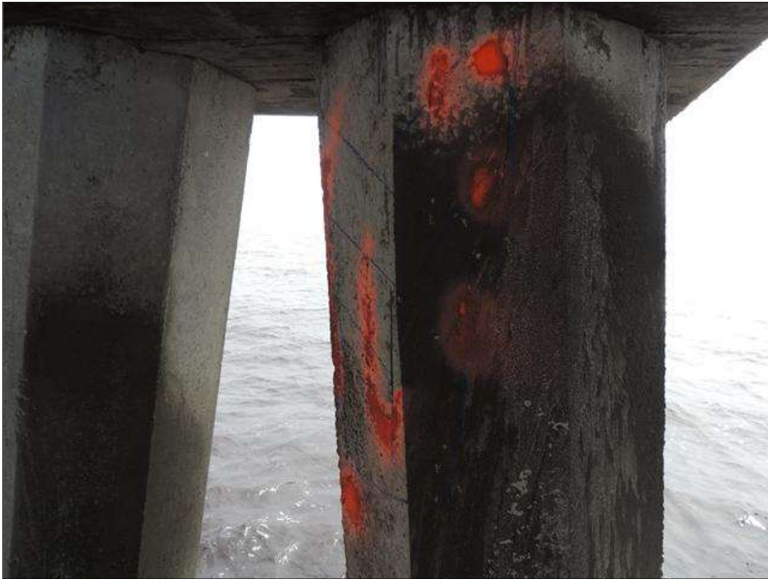
BENT 128 PILE 4 DELAMINATED AREA ON THE N FACE OF THE PILE FROM BOTTOM OF CAP DOWN 29" X 15" AROUND PILE.
