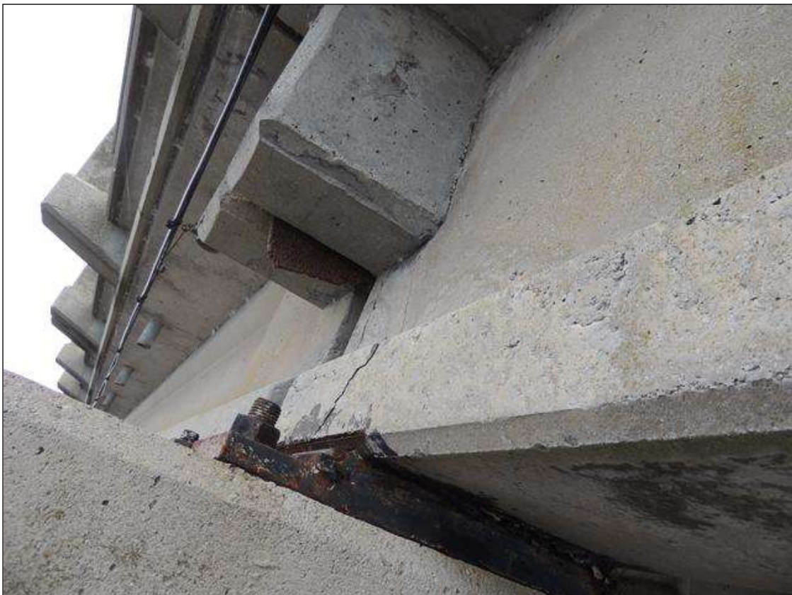
BENT 70 LT END OF G1 IS CRACKED AND DELAMINATED 17" H X 12" FROM END BACK.
