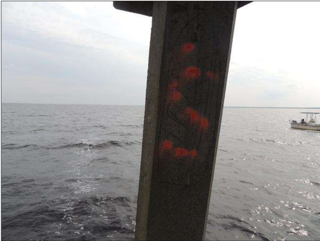
BENT 134 PILE 4 HAS DELAMINATED AREA STARTING 10" BELOW BOTTOM OF CAP AND GOES DOWN 44" X 16" AROUND PILE.
