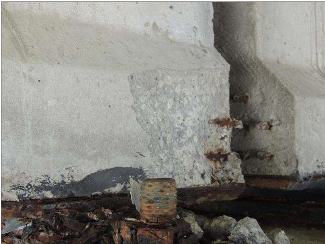
BENT 134 SPAN 134 SIDE SPALLED AREA ALONG THE BOTTOM RT END OF G3 7" X 9" X 1 1/2" DEEP.
