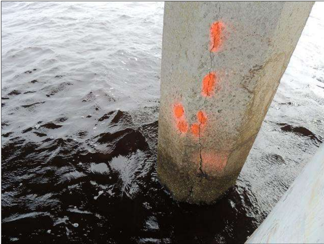
BENT 134 LARGE CRACK AND DELAMINATED AREA ON THE N FACE OF P3 48" FROM WL UP AND 12" AROUND PILE.
