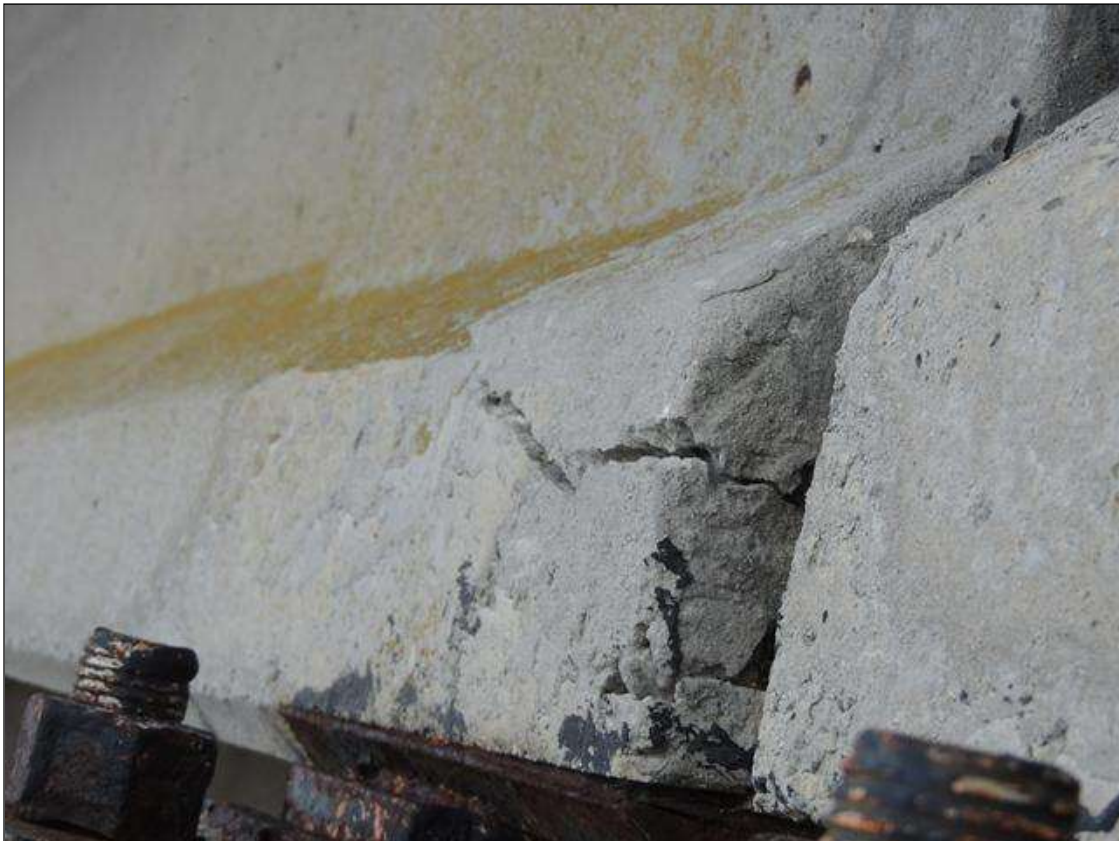
BENT 67 SPAN 68 SIDE BOTTOM LT END OF G1 IS CRACKED AND DELAMINATED 9" X 10".
