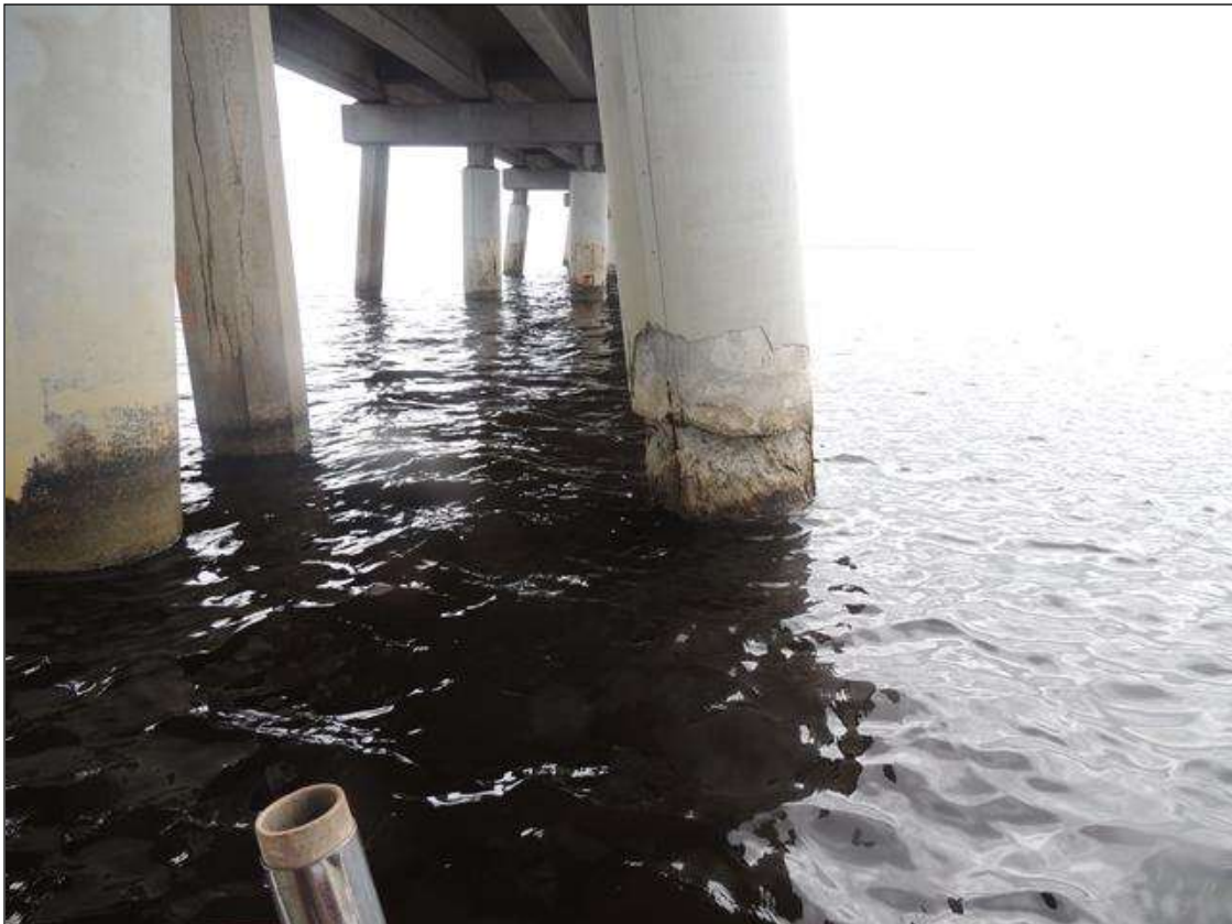
BENT 17 HAS REPAIRED AREA THAT HAS SPALLED 4" DEEP ALL AROUND PILE FROM WL UP 2'.
