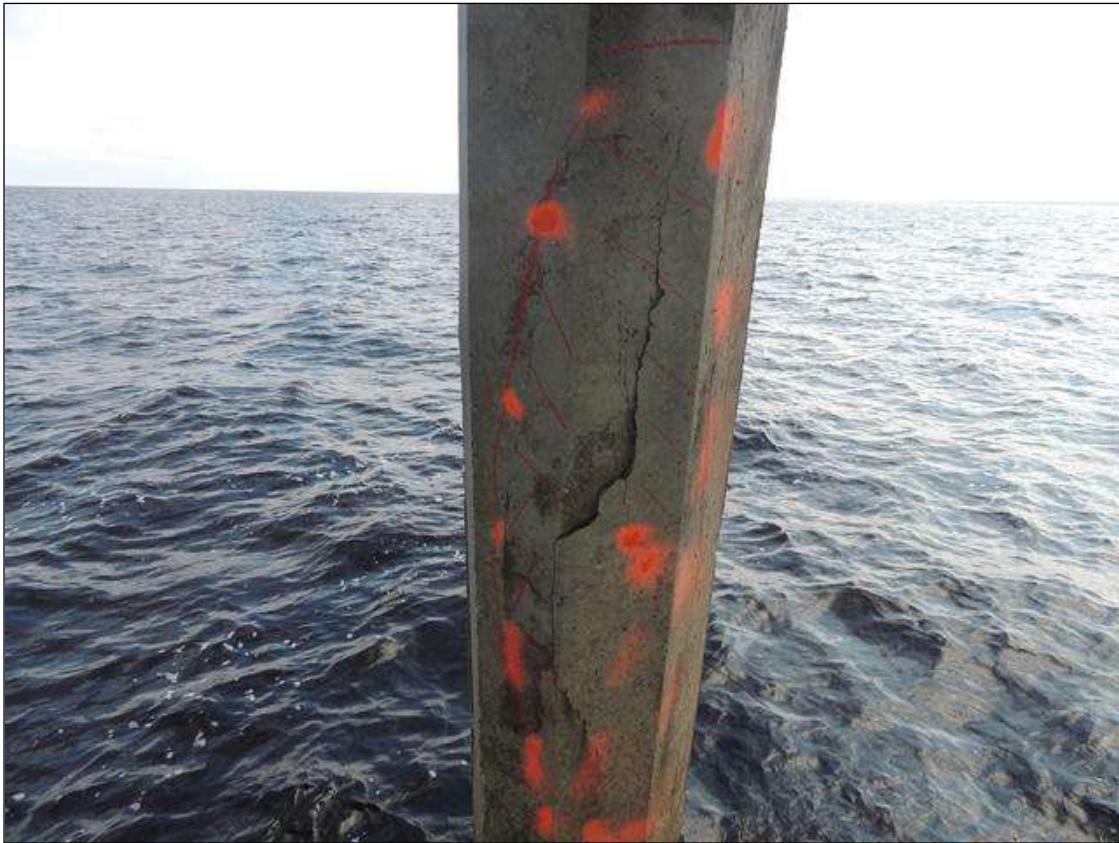
BENT 221 P1 SPALLED CRACKED AND DELAMINATED AREA ALONG THE S FACE OF THE PILE 101" FROM THE WATERLINE UP 21" AROUND THE PILE.
