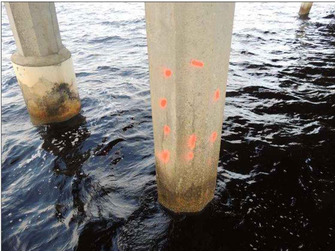
BENT 218 P3 CRACKED AND DELAMINATED AREA 58" FROM THE WATERLINE UP 20" AROUND THE PILE.
