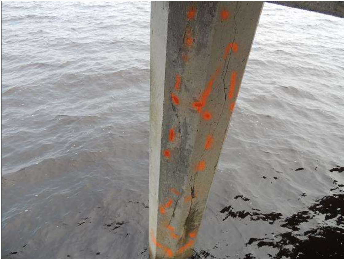
BENT 101 PILE 1 IS CRACKED AND DELAMINATED AND SURFACE SPALLED AREA SOUTH FACE FROM BOTTOM OF CAP DOWN 11' 5" X 23" AROUND PILE.
