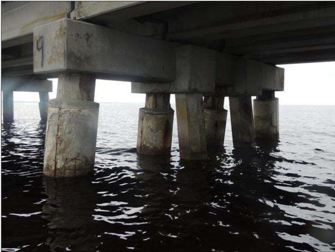
BENT 10 THE CASING AROUND REPAIRED PILES IS BREAKING OFF AROUND PILE.AND MISSING IN SPOTS.
