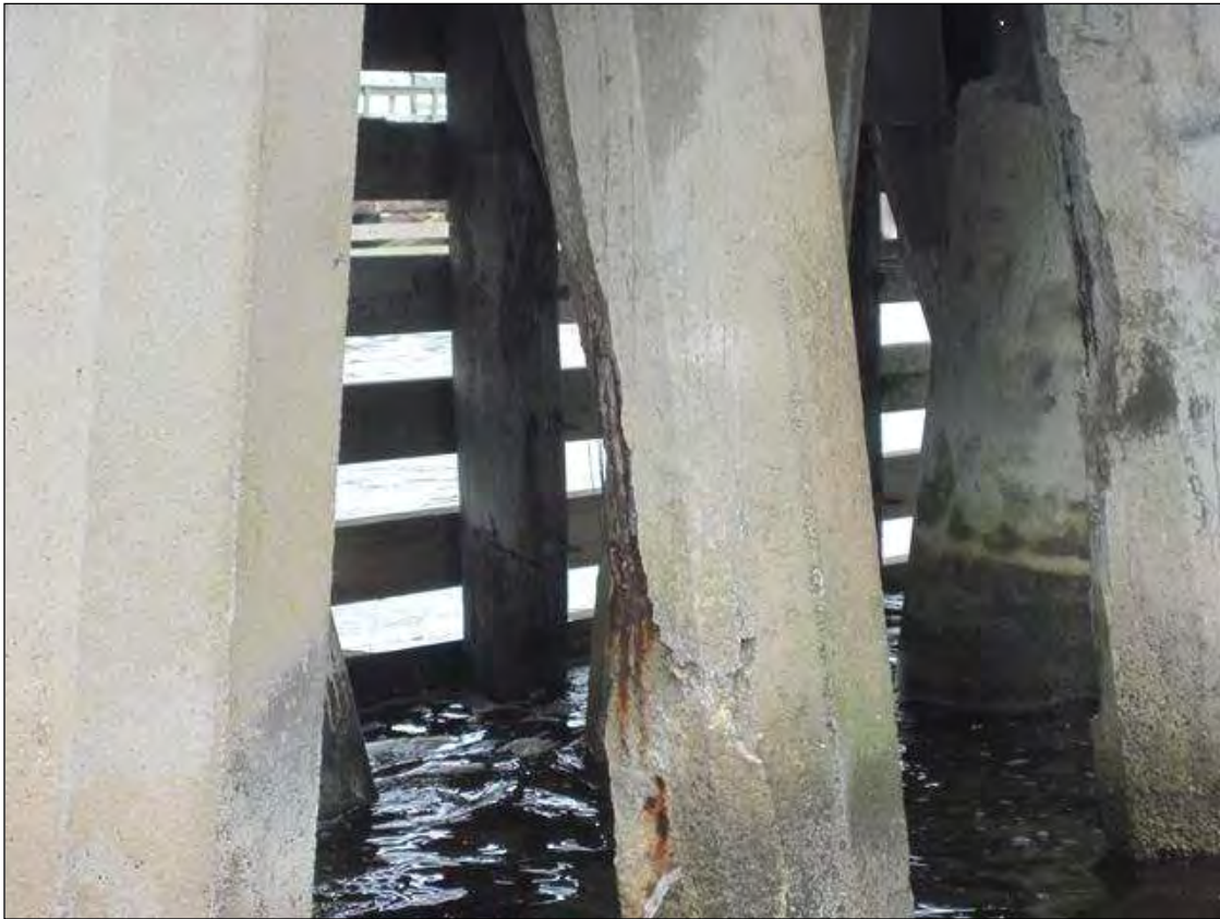
REST BENT 2 PILES POOR
