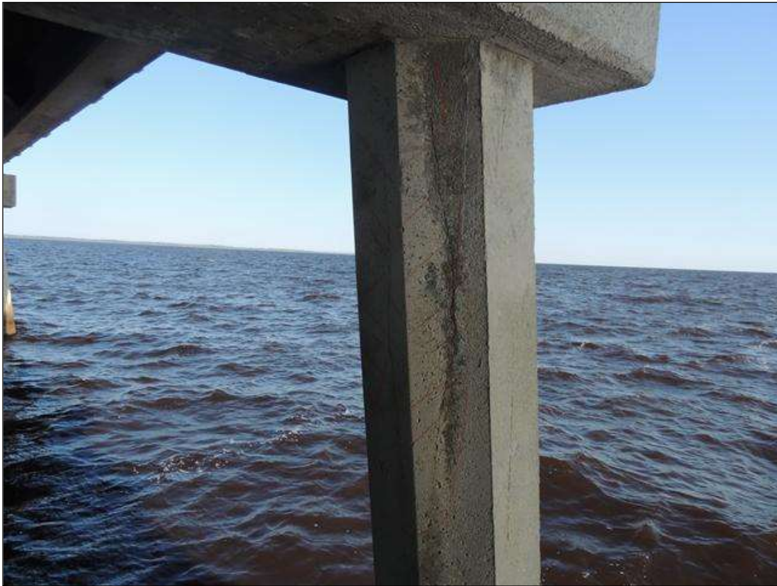
BENT 260 PILE 1 CRACKED AND DELAMINATED AREA FROM THE BOTTOM OF CAP DOWN 58" AND 18" AROUND PILE ON SOUTH FACE.
