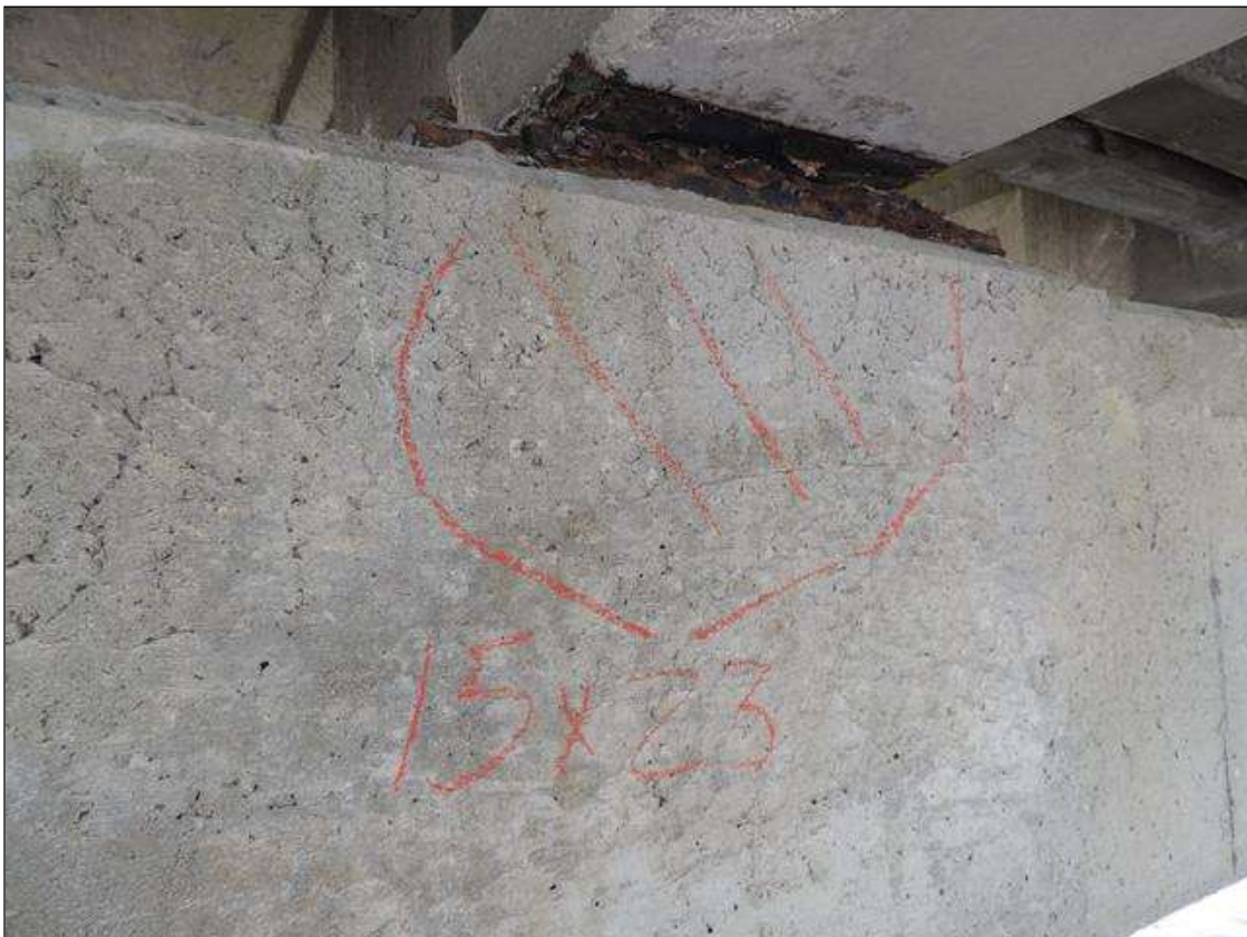
BENT 167 SPAN 167 SIDE CRACKED AND DELAMINATED AREA ALONG THE CAP UNDER G3 15" X 23"
