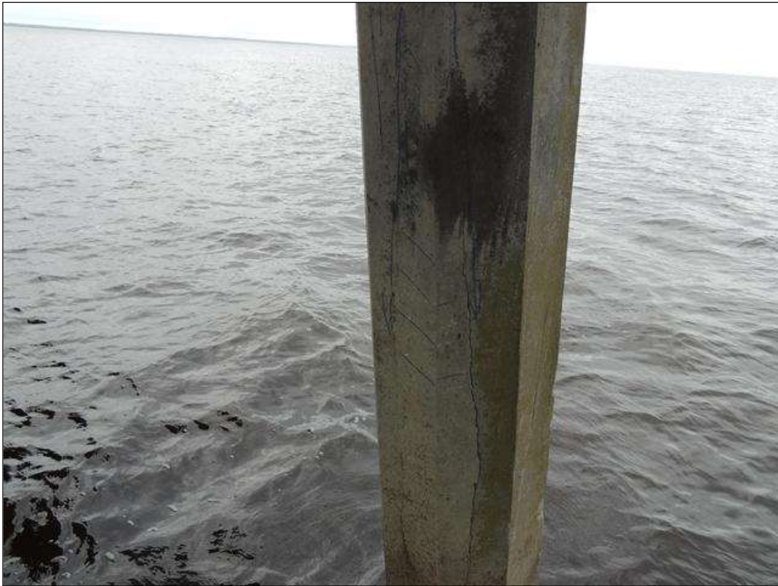
BENT 14 CRACKED AND DELAMINATED AREA ON THE NW SIDE OF PILE 4 STARTS 10" BELOW CAP AND GOES DOWN 8' 4" X 12" WIDE.
