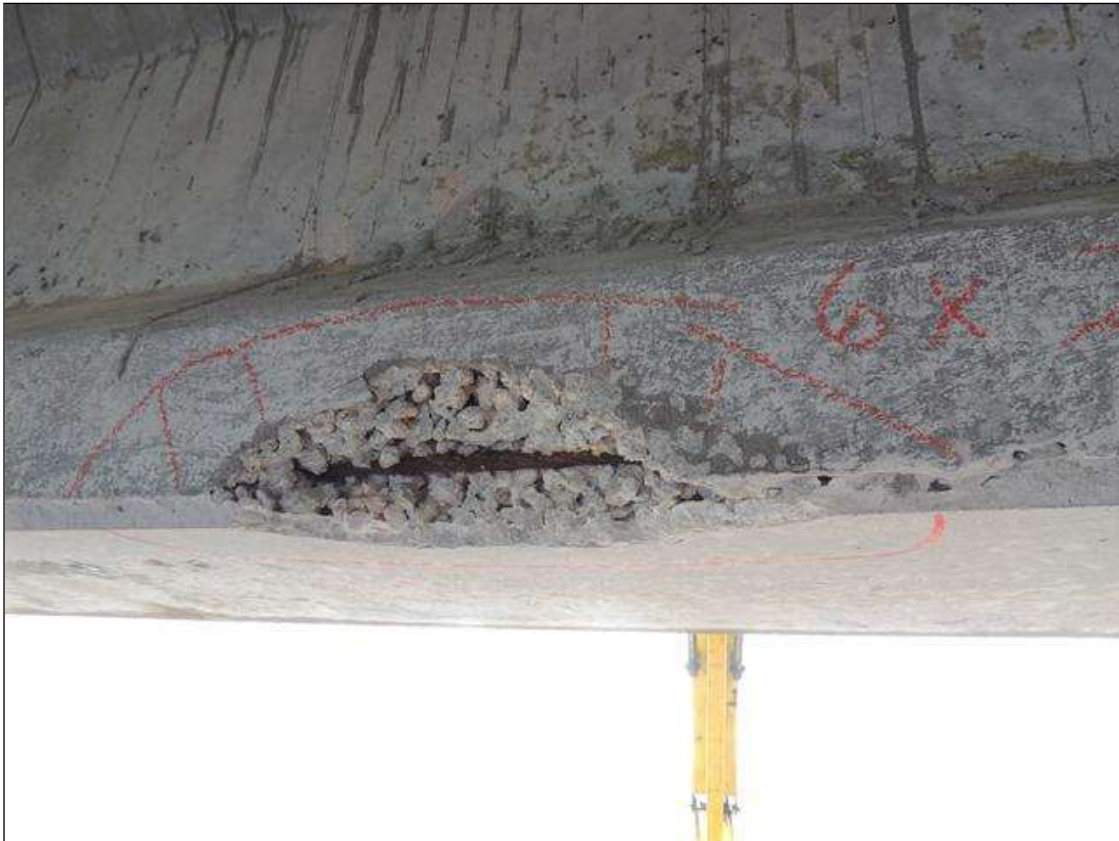
SPAN 233 SPALLED AND HONEYCOMBE AREA ALONG LT SIDE G4 11' FROM BENT 232 6" X 23" X 4" DEEP WITH CABLES EXPOSED PM
