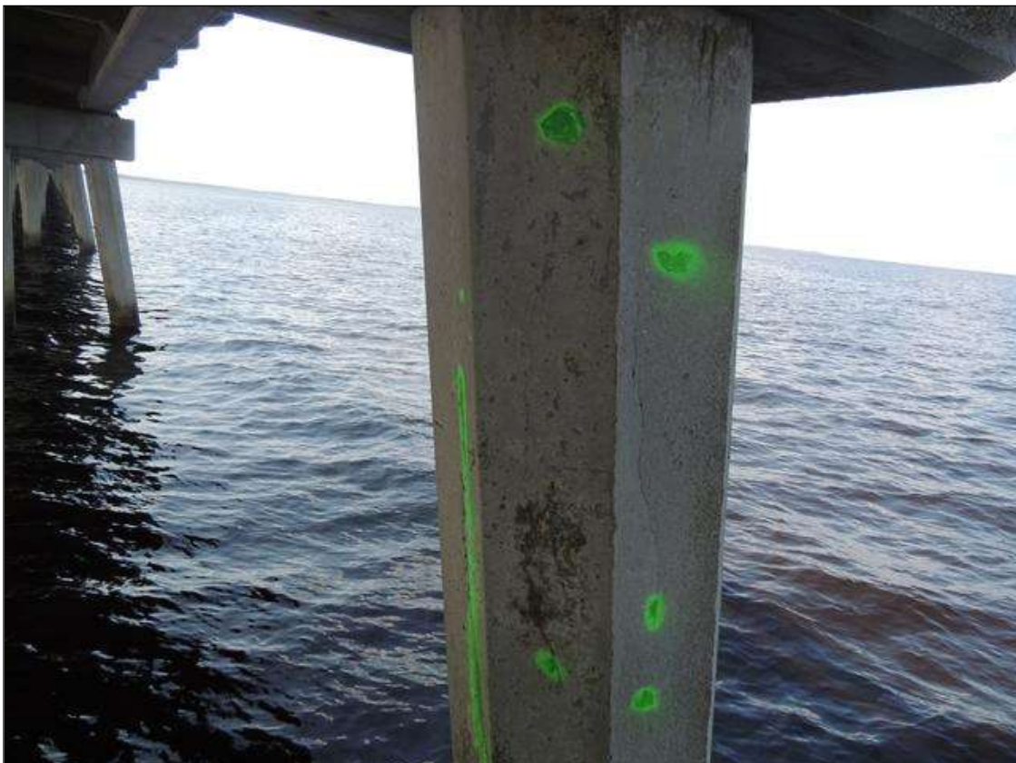
BENT 244 P1 CRACKED AND DELAMINATED AREA ALONG SE FACE OF PILE FROM BOTTOM OF CAP DOWN 61" X 16" AROUND PILE.
