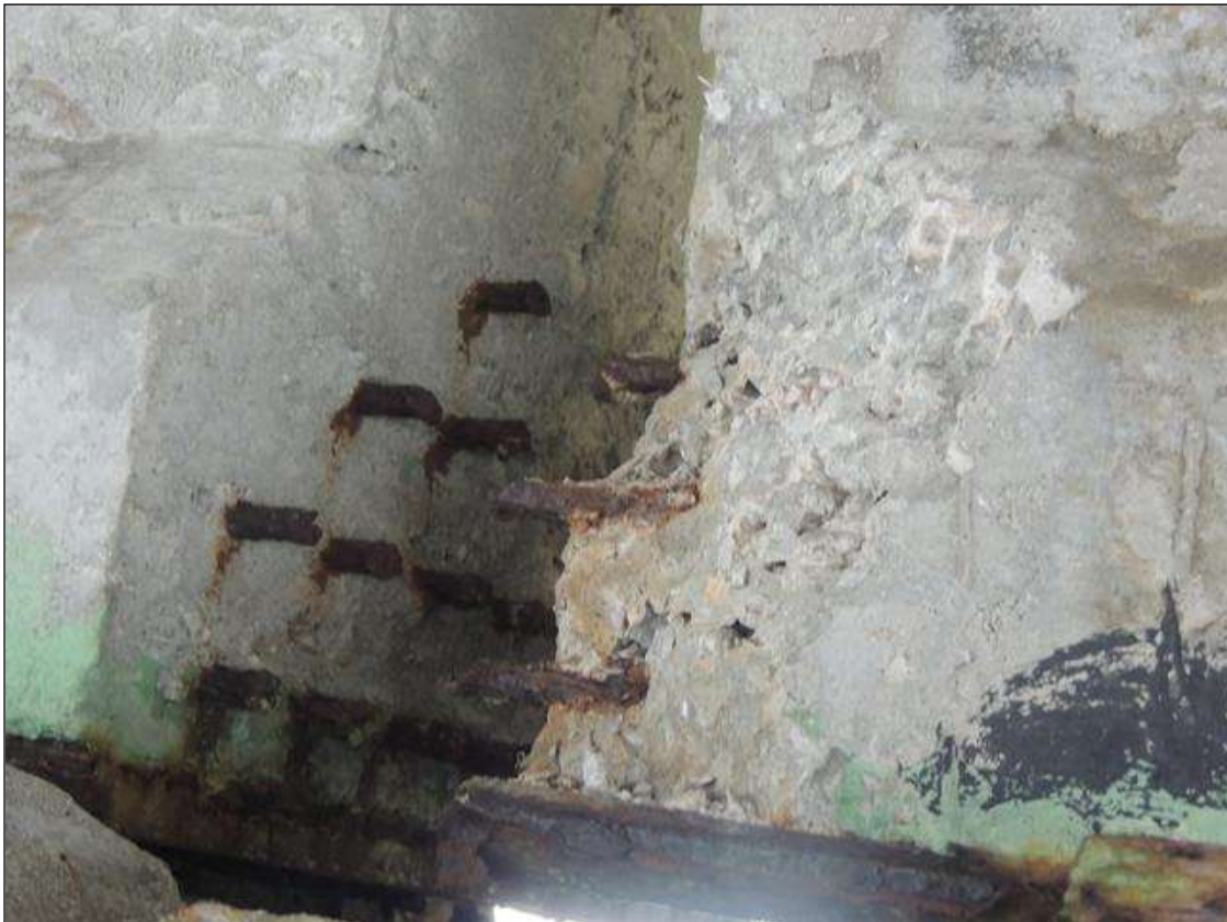
BENT 22 SPAN 22 SIDE SPALLED AREA ALONG BOTTOM LT END OF G2 4" X 9" X 2" DEEP CABLE EXPOSED.
