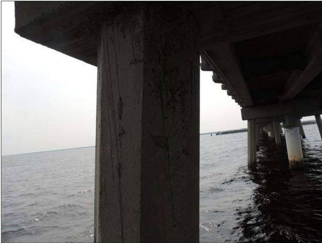
BENT 132 CRACKED AND DELAMINATED AREA ON THE NORTH FACE OF P6 FROM BOTTOM OF CAP DOWN 49" X 12" AROUND PILE.
