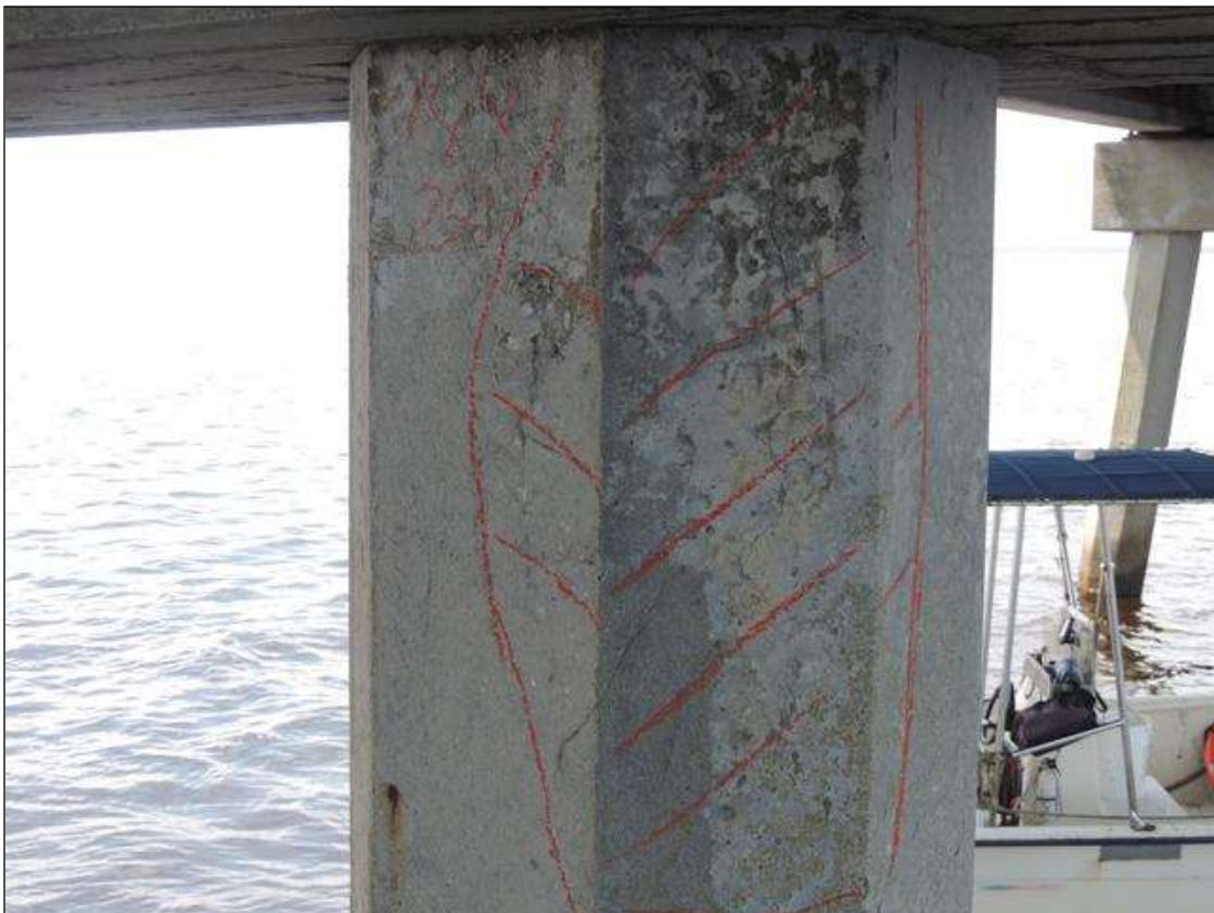
BENT 235 CRACKED AND DELAMINATED AREA ALONG THE TOP FACE OF PILE 2 ON NE FACE 18" X 28".
