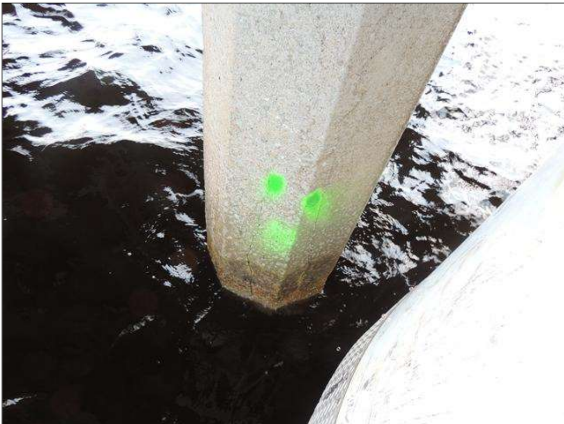
BENT 234 CRACKED AND DELAMINATED AREA ON PILE 2 FROM WL UP 36" AND 24" AROUND PILE.
