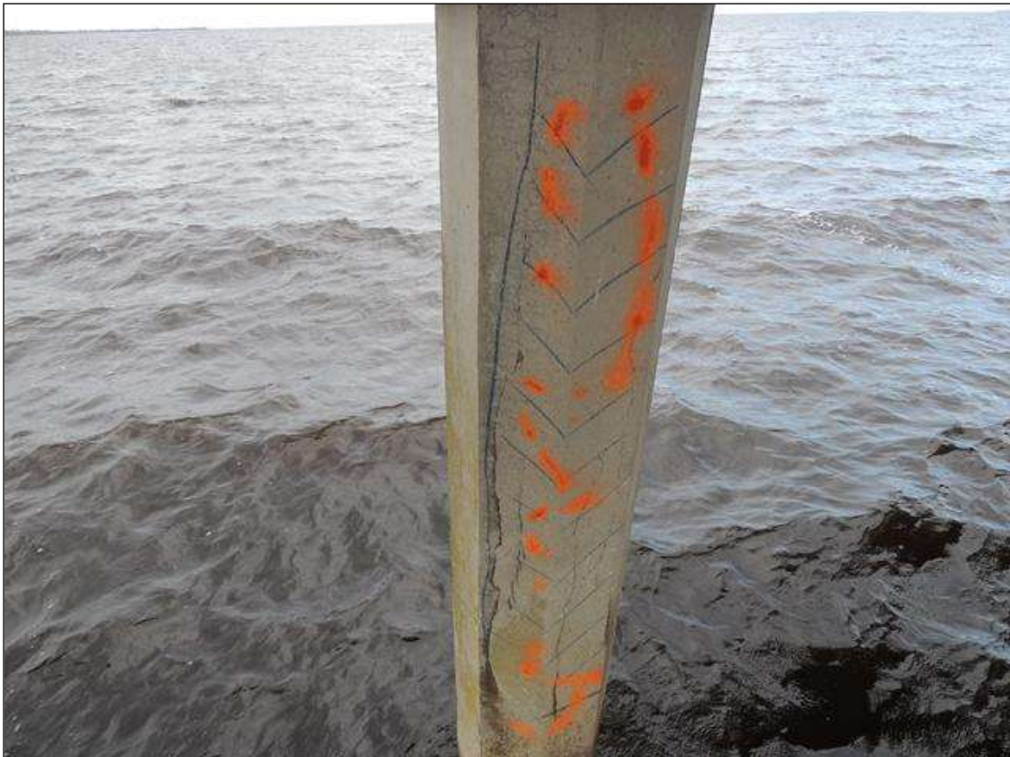
BENT 36 P1 SOUTH FACE CRACKED AND DELAMINATED AREA FROM WL UP TO BOT OF CAP 10' 4".
