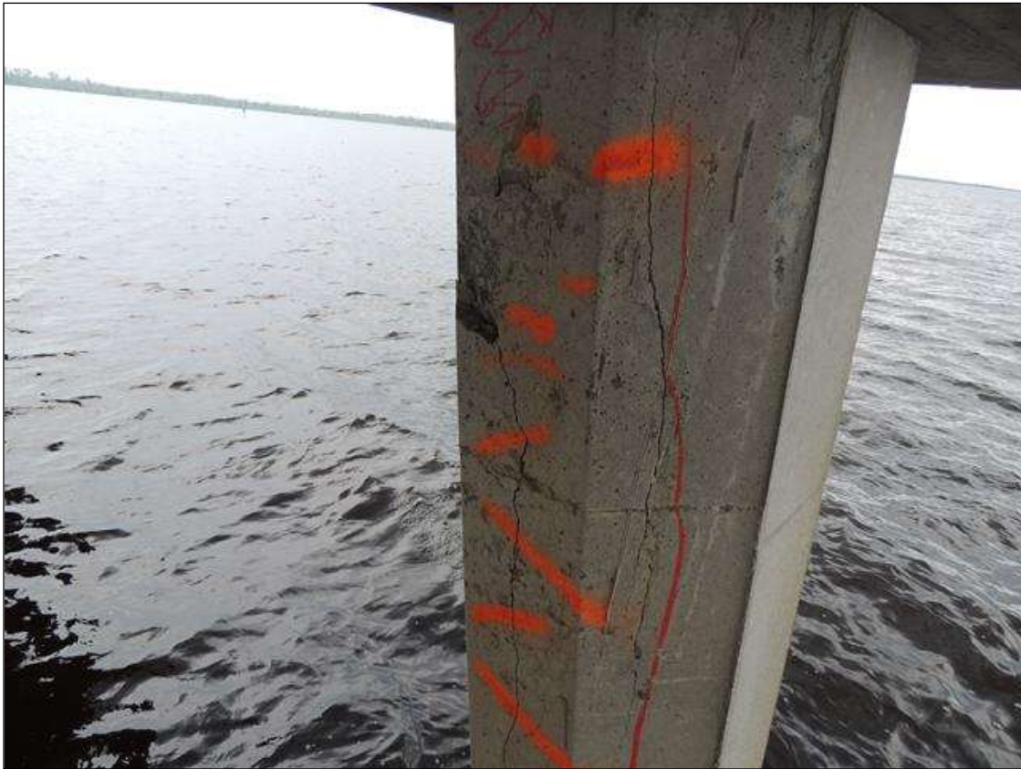
BENT 69 PILE 1 CRACKED AND DELAMINATED AREA ON SOUTH FACE OF PILE FROM BOTTOM OF CAP DOWN 63" X 22" AROUND.
