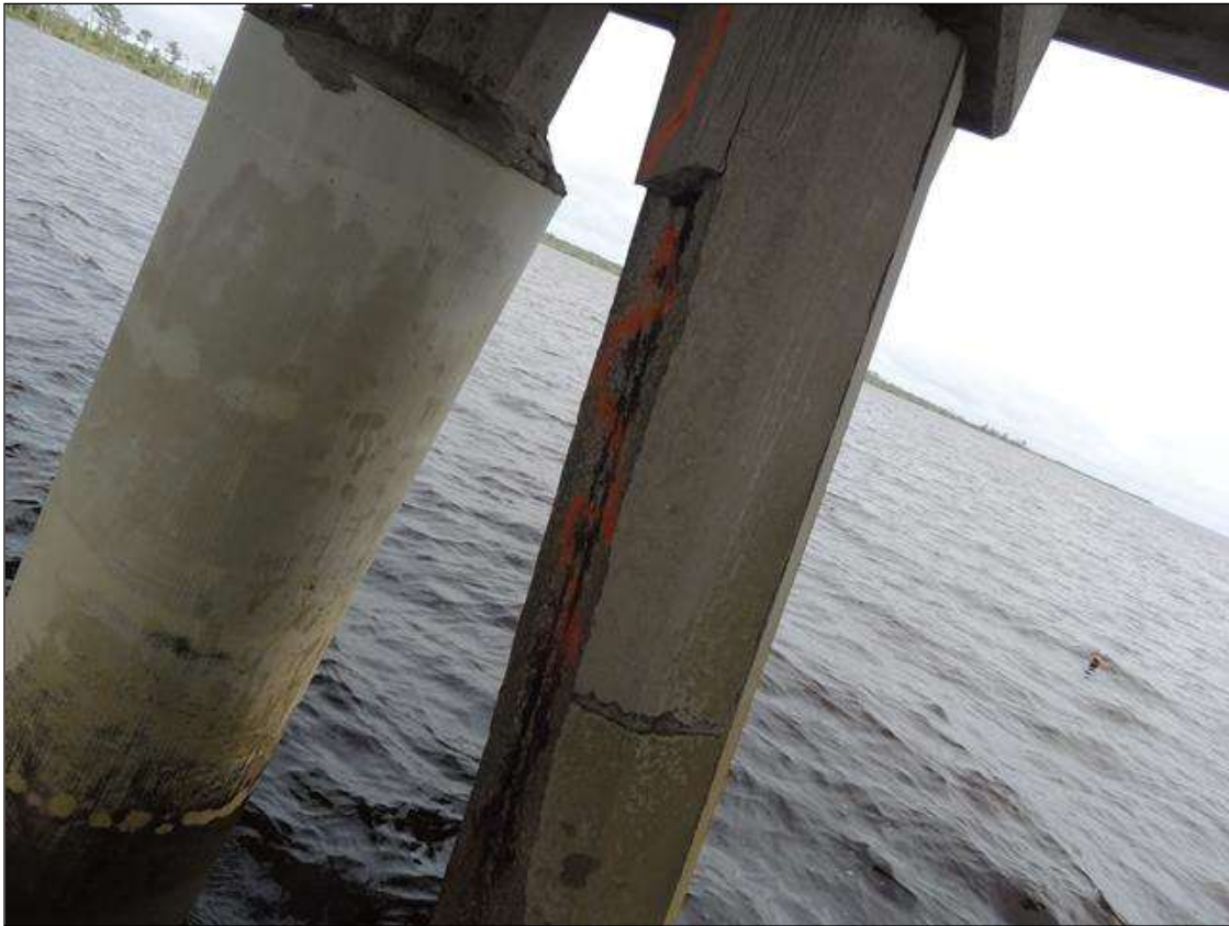
BENT 17 PILE 3 UNDER SUBCAP 1 HAS SAPLLED AREA 10' 2" LONG X 2 1/2" DEEP ON SW SIDE WITH CABLES EXPOSED AND BROKEN.PM
