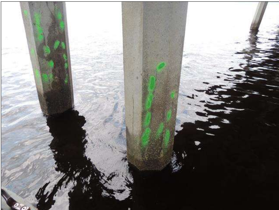
BENT 237 P4 CRACKED AND DELAMINATED AREA FROM THE WL UP 50" X 14" AROUND PILE ON NE FACE.
