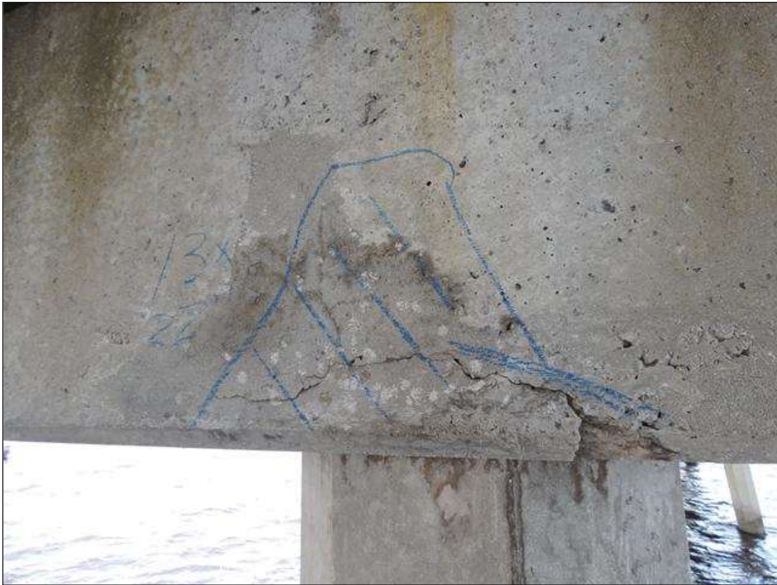
BENT 24 SPAN 25 SIDE CRACKED AND DELAMINATED AREA IN FACE OF CAP UNDER G2 13" X 22",,
