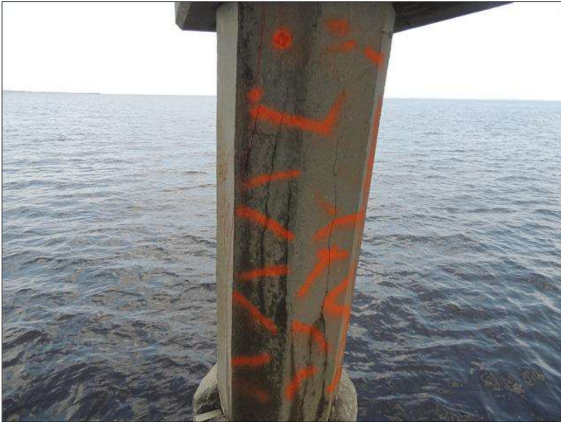
BENT 66 PILE 1 CRACKED AND DELAMINATED AREA ABOVE THE PILE REPAIR FROM BOTTOM OF CAP DOWN 70" X 32" AROUND PILE.
