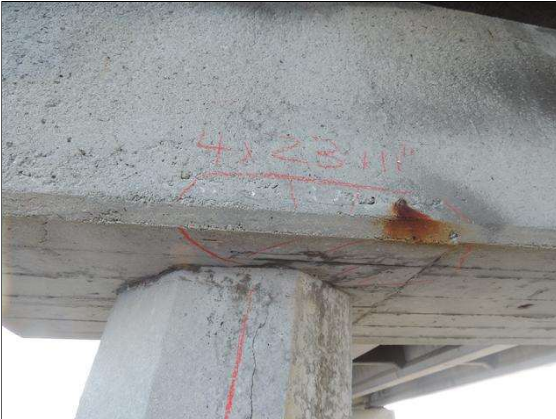
BENT 231 SPAN 231 SIDE CRACKED AND DELAMINATED AREA ALONG THE BOTTOM FACE OF THE CAP AT P1 4" X 23" X 11" UB.
