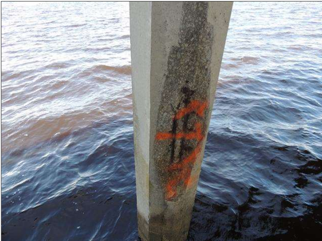
BENT 25 SOUTH FACE OF P1 SPALLED AND CRACKED AND DELAMINATED AREA STARTS 1' BELOW BOT OF CAP AND GOES DOWN TO WL 9' X 16" AROUND X 2" DEEP CABLES PM
