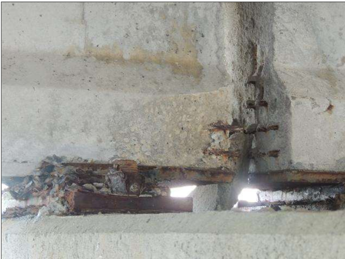
BENT 138 SPAN 138 SIDE SPALLED AREA ALONG THE BOTTOM RT END OF G1 7" X 11" 1 1/2" DEEP
