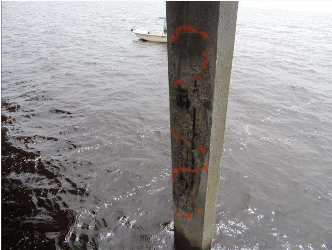
BENT 120 PILE 6 IS CRACKED, DELAMINATED AND SPALLED FROM BOTTOM CAP DOWN 127" AND 18" W WITH 3 CABLES EXPOSED. PM
