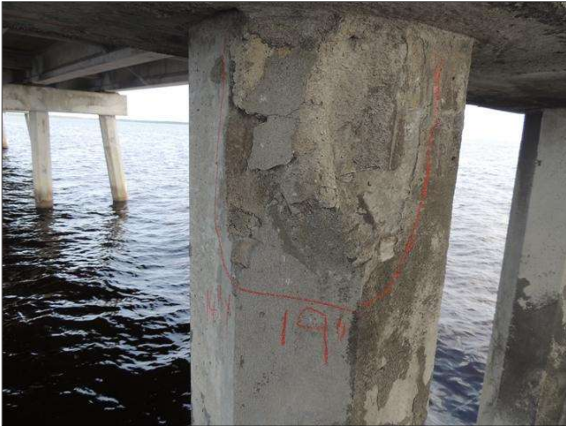
BENT 166 P3 EAST FACE SPALLED AND DELAMINATED AREA 19" FROM THE BOTTOM OF THE CAP DOWN X 18" AROUND X 2" DEEP
