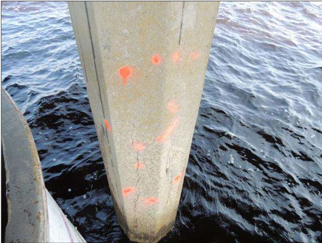
BENT 231 P2 CRACKED AND DELAMINATED AREA ON THE SE FACE OF THE PILE 75" FROM THE WATERLINE UP 30" AROUND THE PILE
