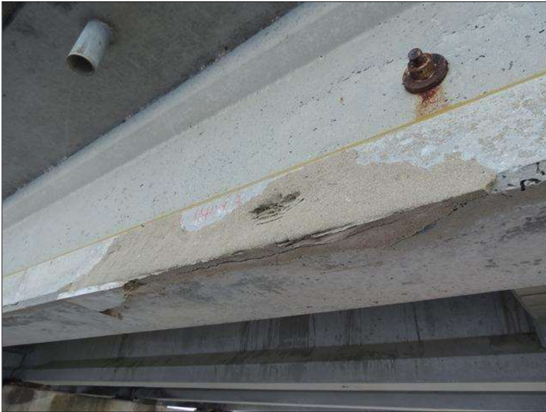
SPAN 246 PATCHED AREA ALONG THE LT BOTTOM SIDE OF G1 6" X 44" X 3".
