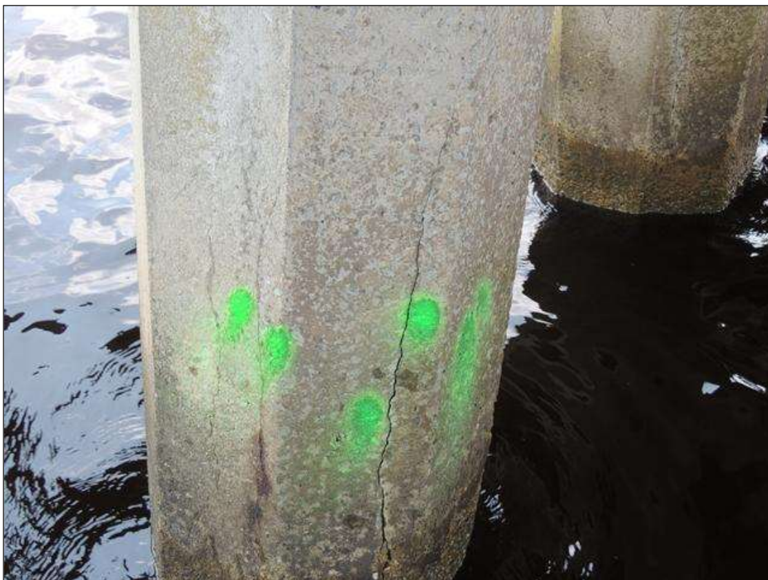
BENT 237 CRACKED AND DELAMINATED AREA ON P5 ON NE FACE FROM WL UP 46" AND 29" AROUND PILE.
