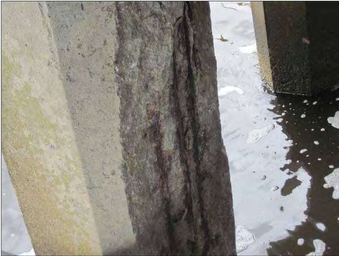
REST BENT 2, P-12, SPALLED W/ EXPOSED STRANDS (50%-100% LOSS) FROM CAP TO W/L, FACES 1,2,3,6,7,8.
