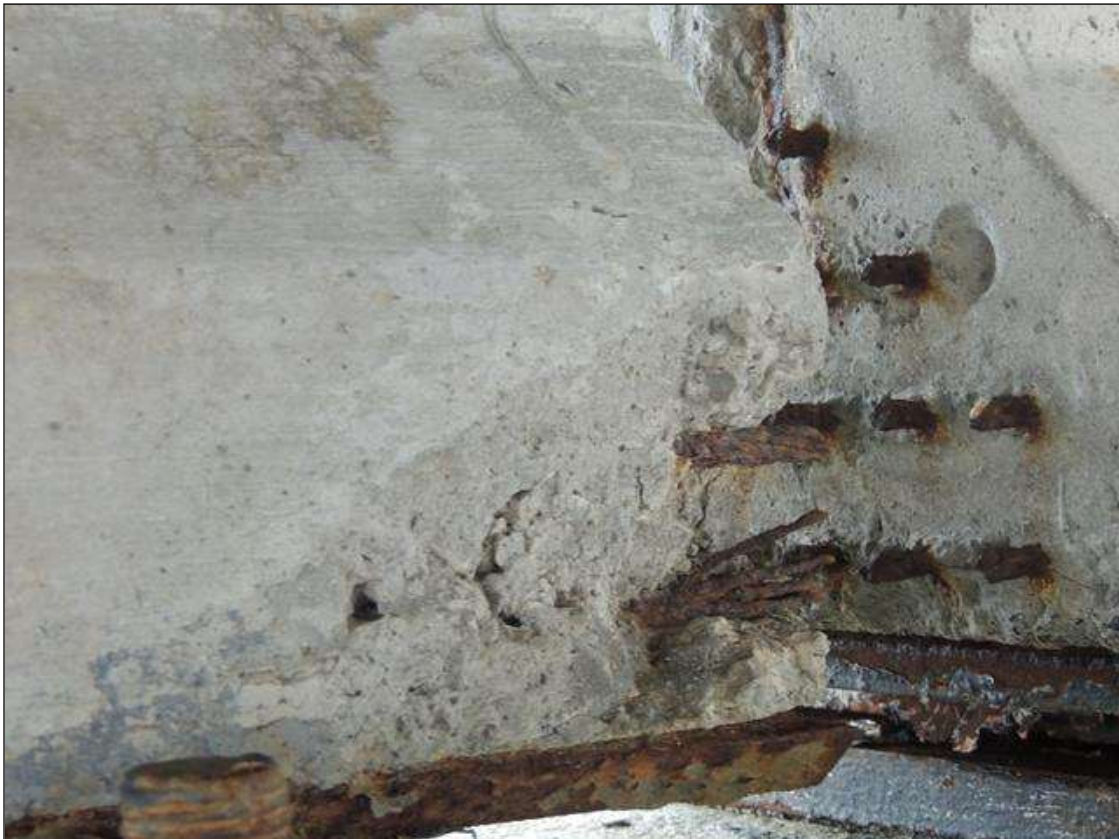
BENT 65 SPAN 65 SIDE SPALLED AREA ON THE BOTTOM RT END OF G1 6" X 8" X 2" DEEP
