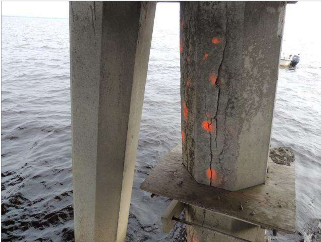
BENT 136 P4 LARGE CRACKED AND DELAMINATED AREA FROM BOTTOM OF CAP TO WL 10' X 28" AROUND PILE ON N FACE.
