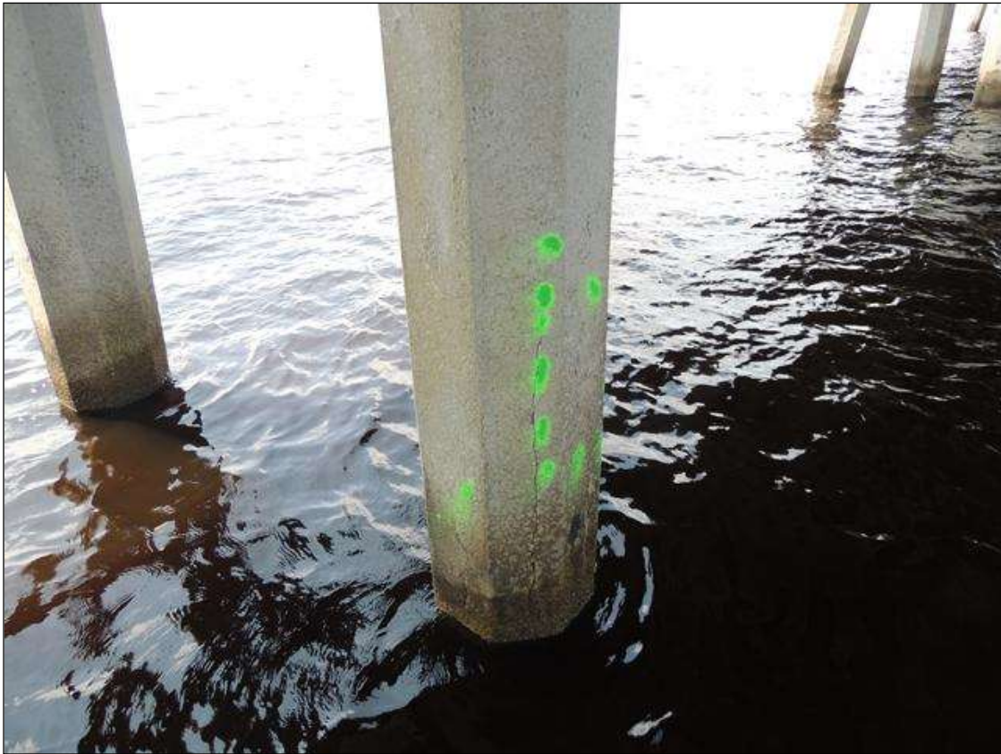
BENT 234 CRACKED AND DELAMINATED AREA ON PILE 3 FROM THE WL UP 53" X 28" AROUND PILE.
