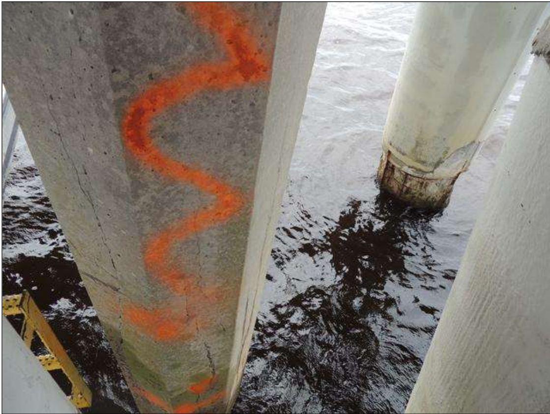
BENT 17 P5 UNDER SUBCAP 2 IS HEAVILY CRACKED AND DELAMINATED 10' 2" LONG X 33" AROUND PILE ON WEST SIDE.PM
