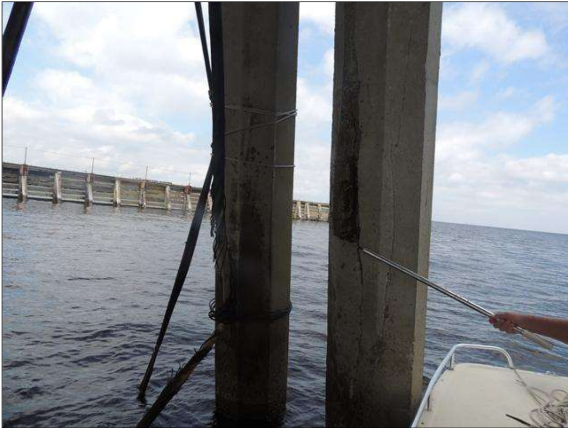
BENT 116 P2 DELAMINATED AND CRACKED AND SPALLED AREA WITH 3 CABLES EXPOSED 9' 4" H X 24" AROUND PILE ON SOUTH FACE.PM
