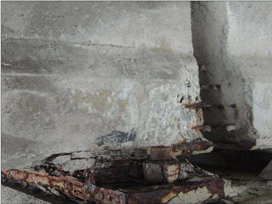
BENT 132 SPAN 133 SIDE SPALLED AREA ALONG THE BOTTOM LT END OF G2 8" X 9" X 2" DEEP CABLE EXPOSED PM.
