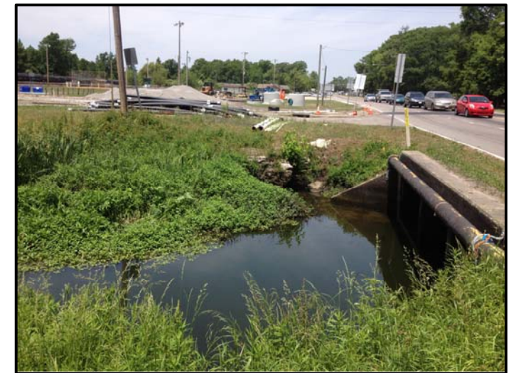
View of Inaccessible Drainage Area and Debris
