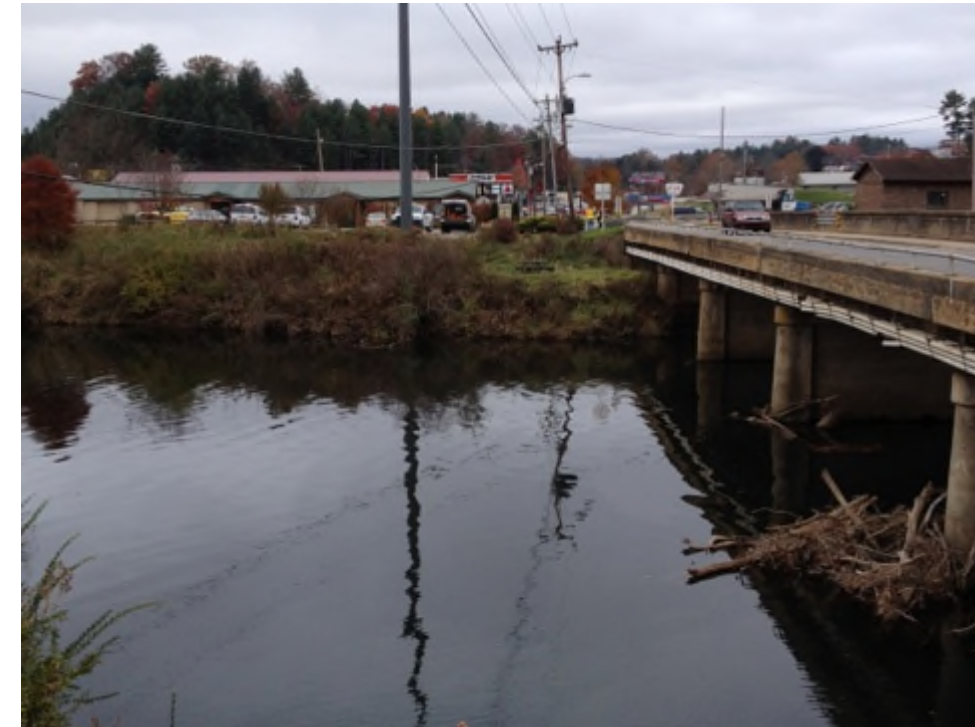
Photograph No. 2: This photograph was taken from proposed End Bent No. 2 right of the US 441 -L- alignment, looking South along the proposed bridge alignment
