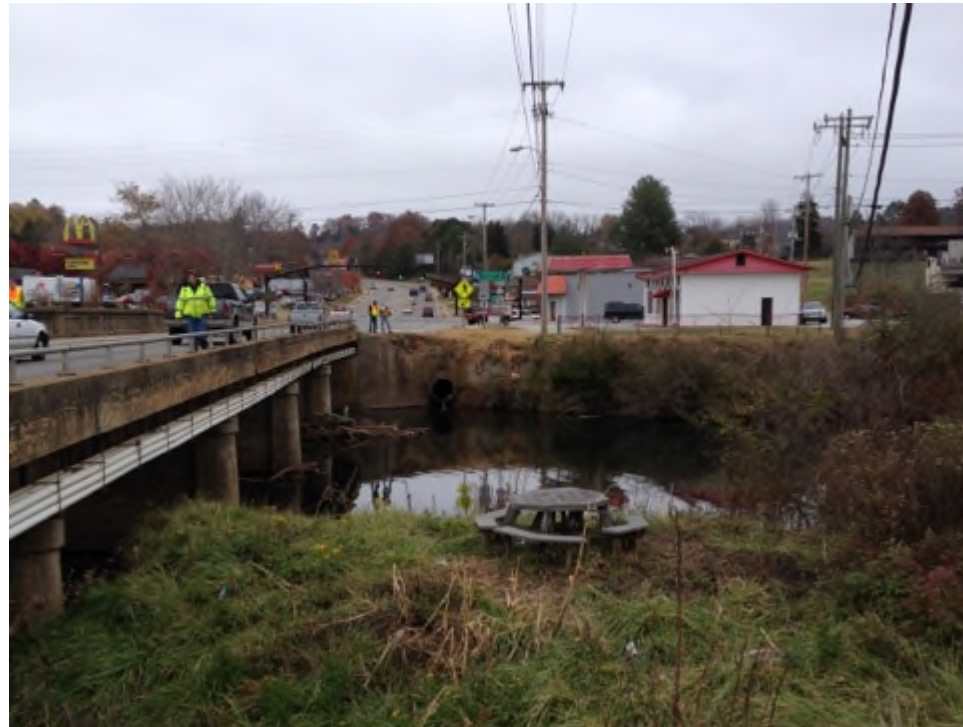
Photograph No. 1: This photograph was taken from proposed End Bent No. 1 right of the US 441 -L- alignment, looking North along proposed bridge alignment
