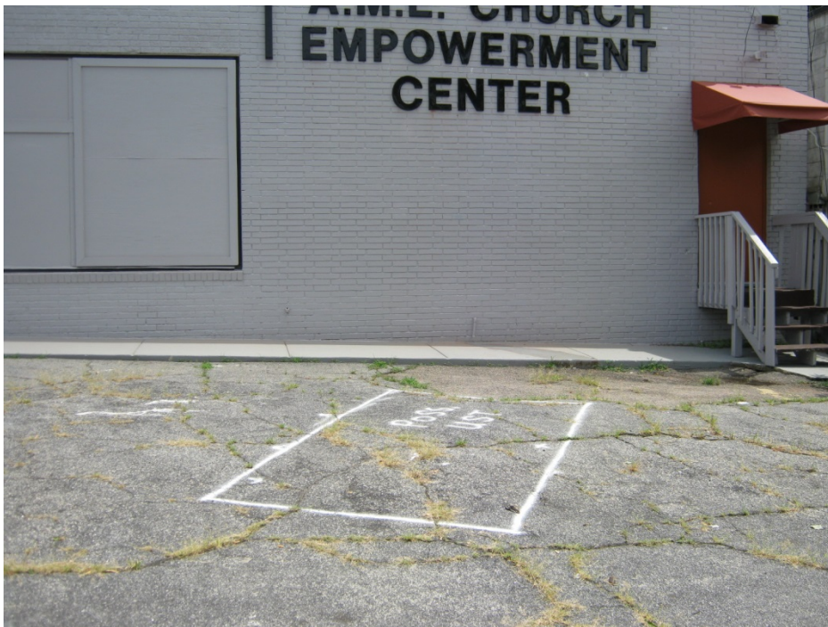
Photo #4: A view of the Possible UST location adjacent to the structure, facing east.
