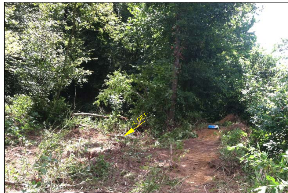
PHOTOGRAPH TAKEN FROM NEAR END BENT 2 OF THE DETOUR STRUCTURE LOOKING DOWNSTATION ALONG -LDET-
