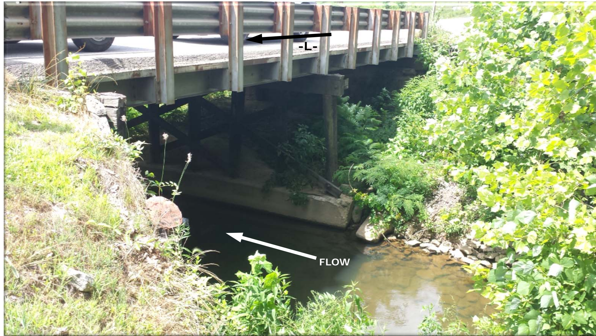
PHOTOGRAPH 1: BRIDGE 169 ON SR 1148 (-L-) OVER GUM CREEK (LOOKING WEST FROM NORTH SIDE).
