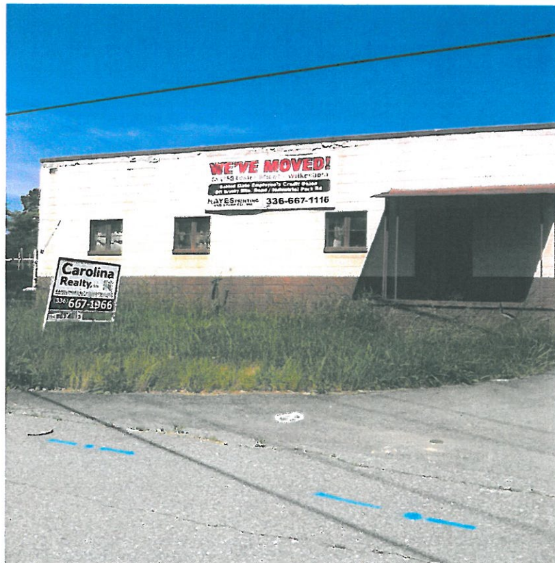
Photograph 2 – View of the portion of the structure formally utilized by Hayes Printing.
