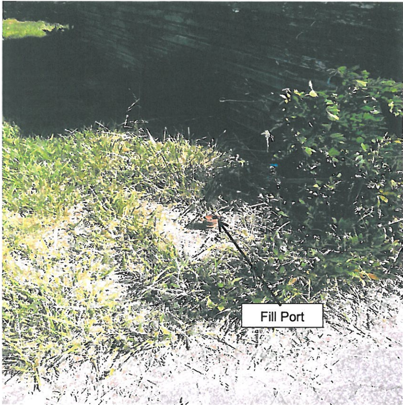
Photograph 9 – View of a fill port observed on the western side of the structure.
