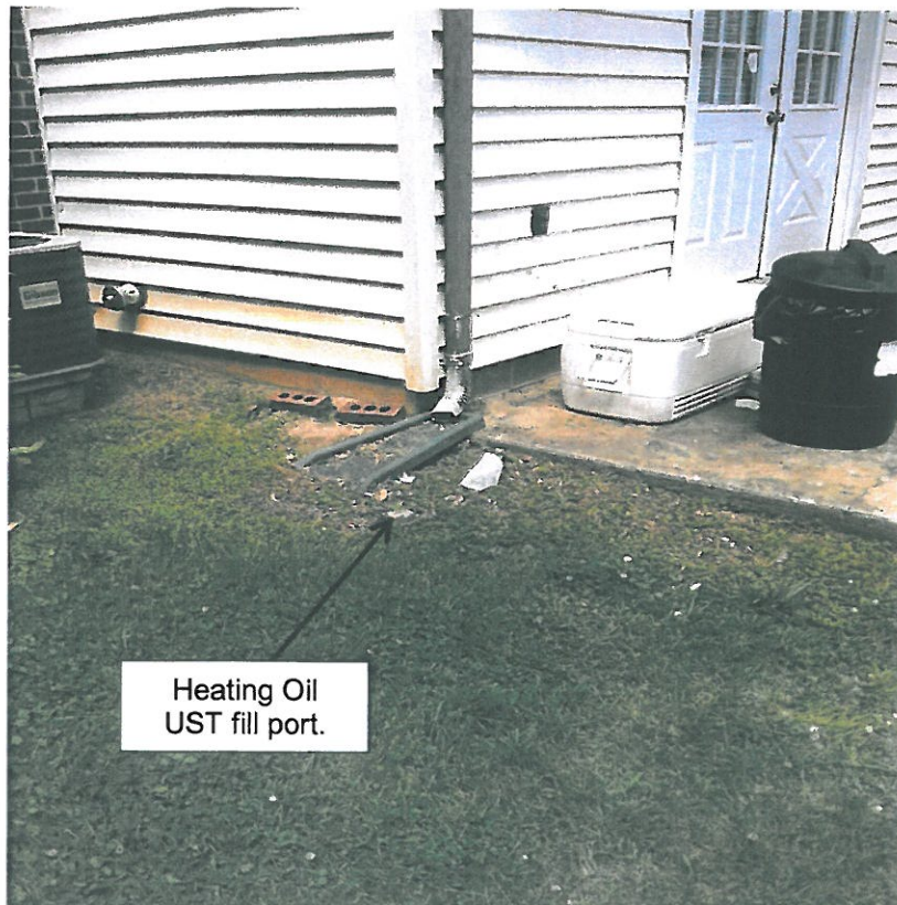
Photograph 8 – View of a heating oil UST fill port.
