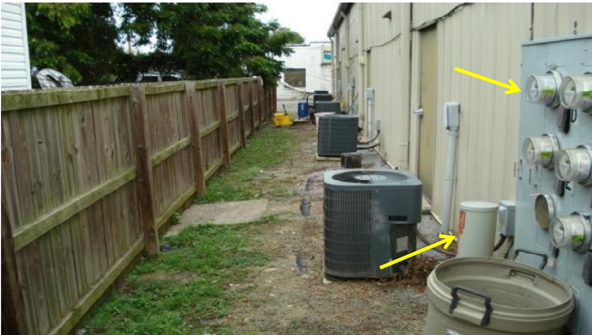
Telephone pedestal and electric meters at rear of 1301 West 14 th Avenue
