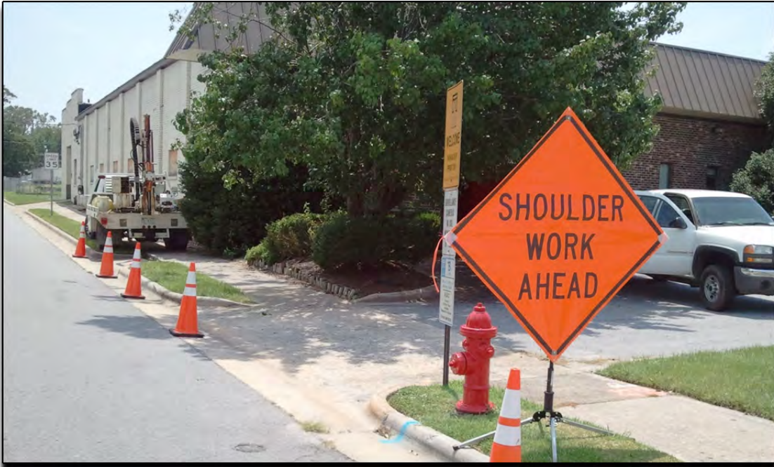
From near corner of W. 10 th St. and S. Washington St. looking South down S. Washington St, probing at proposed catch basin number 1021 (DPT-01) location.
