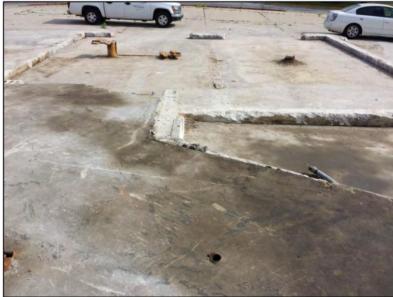
Looking north from southern portion of former building. UST fill port in foreground and hydraulic lift cylinders in background.
