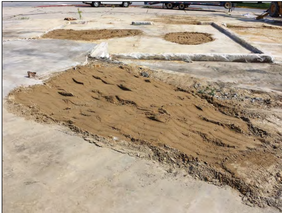
Looking north from southern portion of former building. Backfilled UST excavation in foreground and backfilled hydraulic lift cylinder excavations in background.
