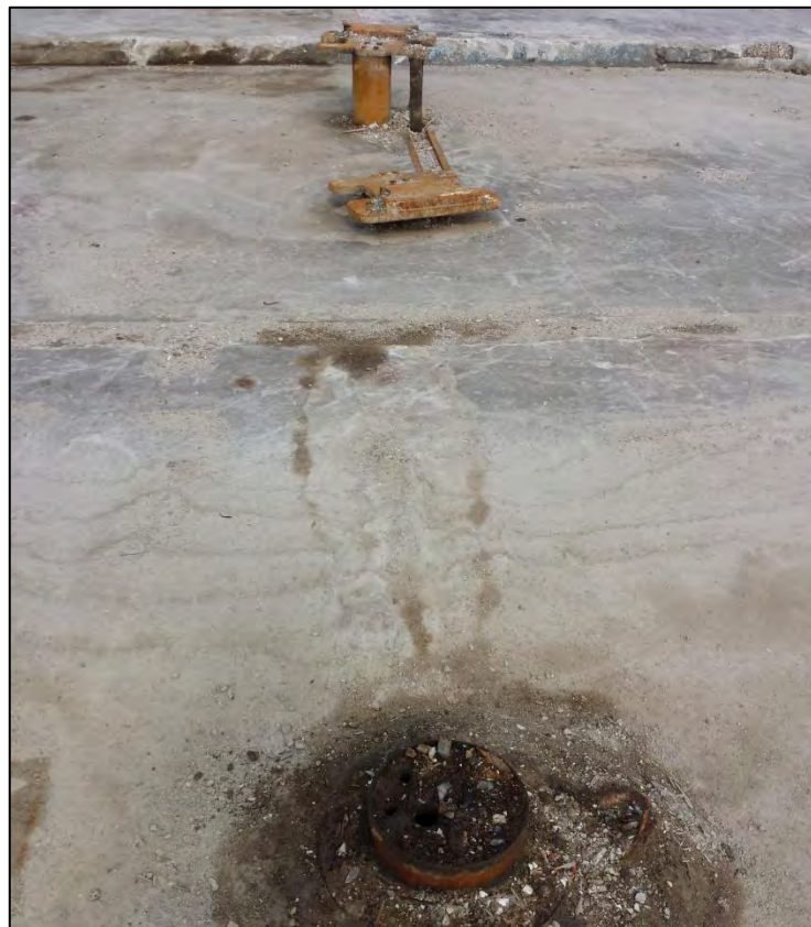
Looking west from eastern portion of former building. Single post (eastern most) hydraulic lift cylinder in foreground and dual post (western most) hydraulic lift cylinders in background.
