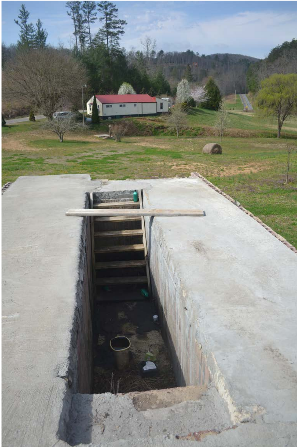
Photograph 3: View of oil change pit at the site. Oil staining, oil containers, oil filters and plastic trash can containing oil can be seen in photograph in base of pit. View is to the southwest.
