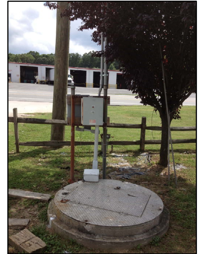
Photograph of steel well cover and well system at west end of survey area.
