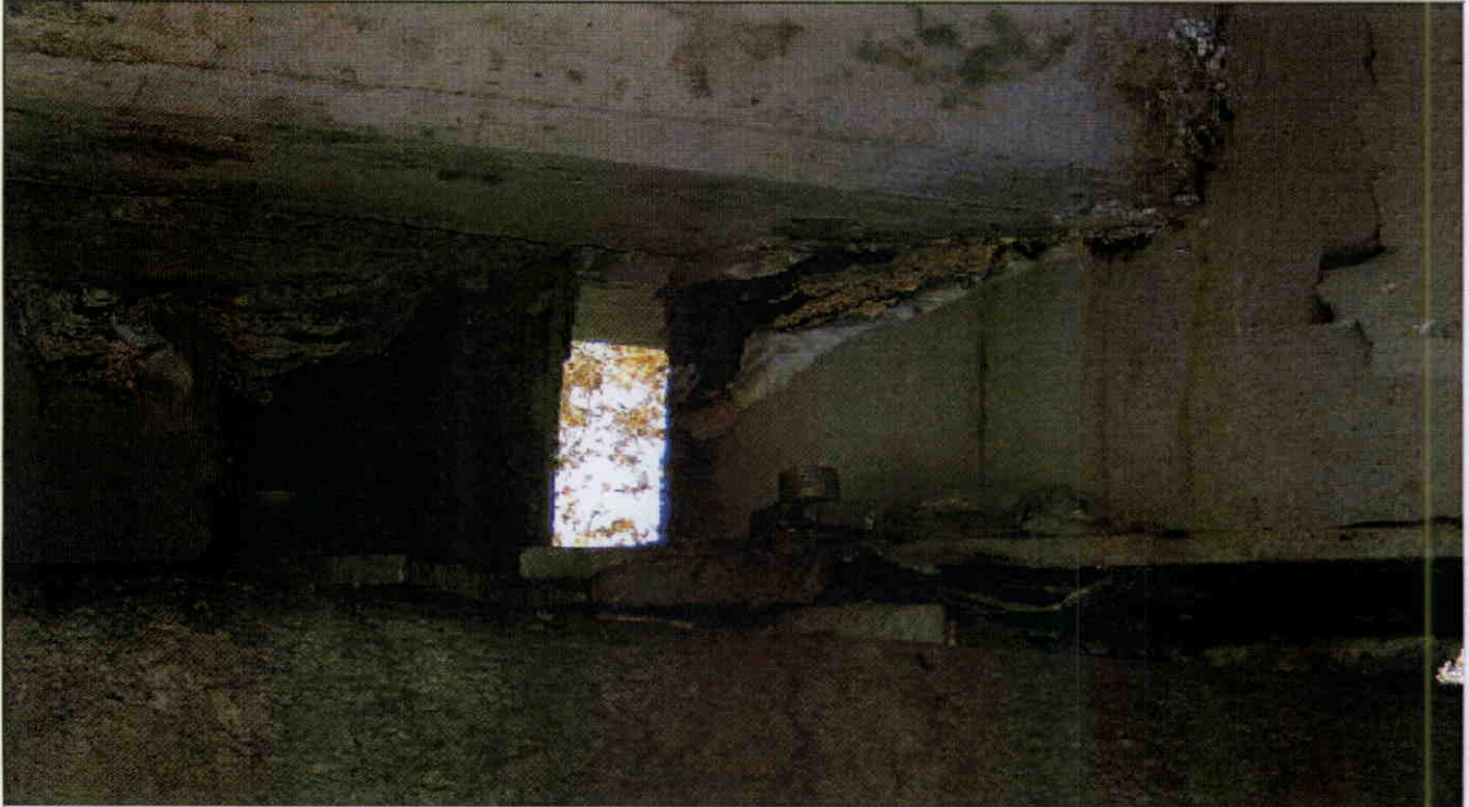
RUST IN ENDS OF BEAM 1 SPAN 4 AND SPAN 5 AT BENT 4
