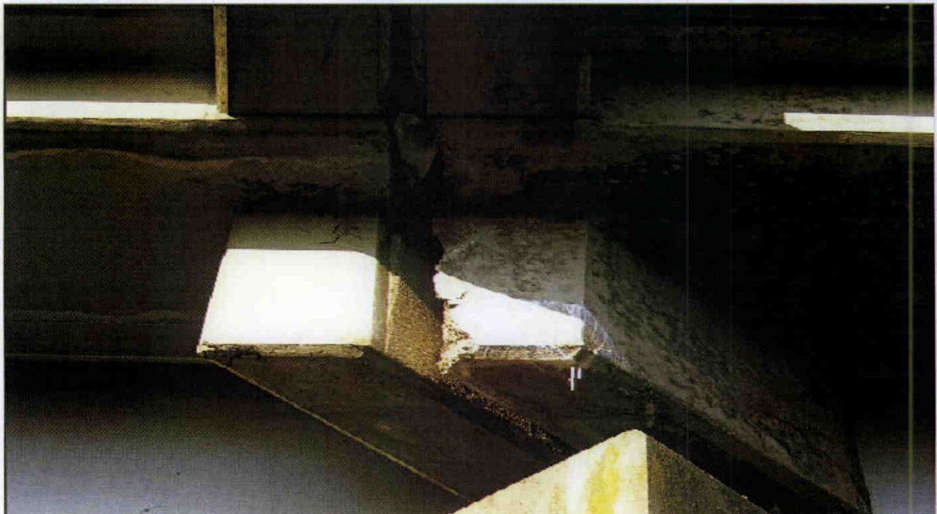
CRACKED AND SPALLED RIGHT OVERHANG DIAPHRAGM AT BENT 2
