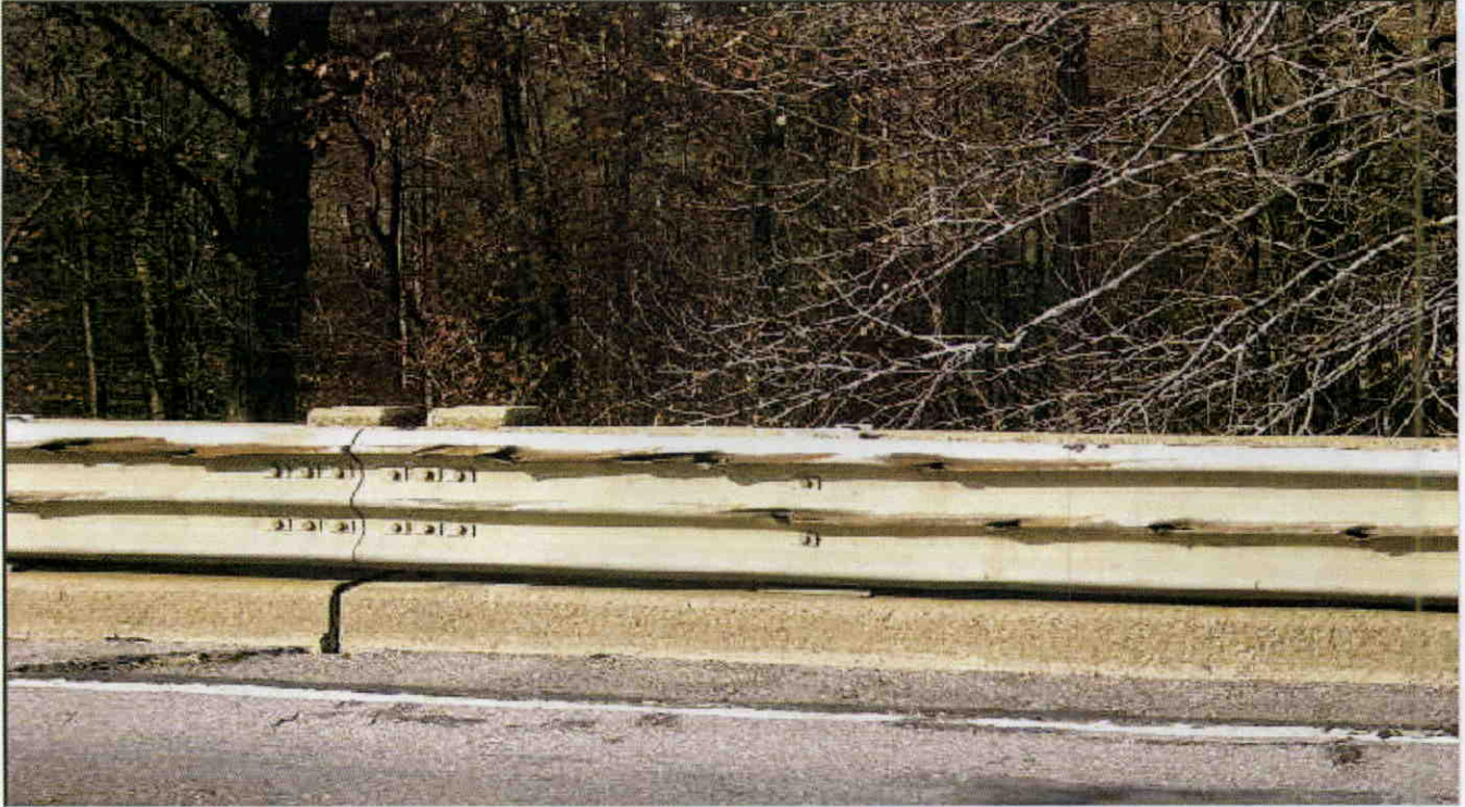
SCRAPE DAMAGE IN LEFT SIDE GUARDRAIL
