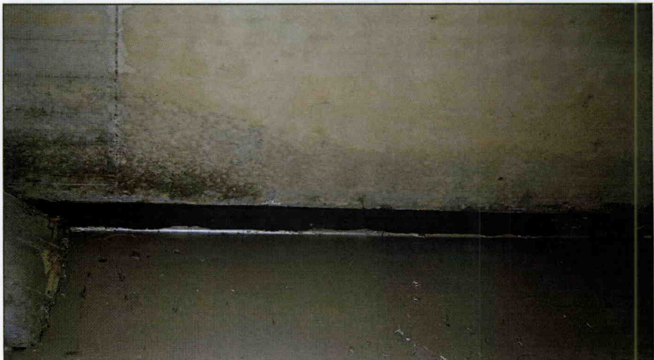
RUST IN TOP FLANGE OF BEAM 1 SPAN 5
