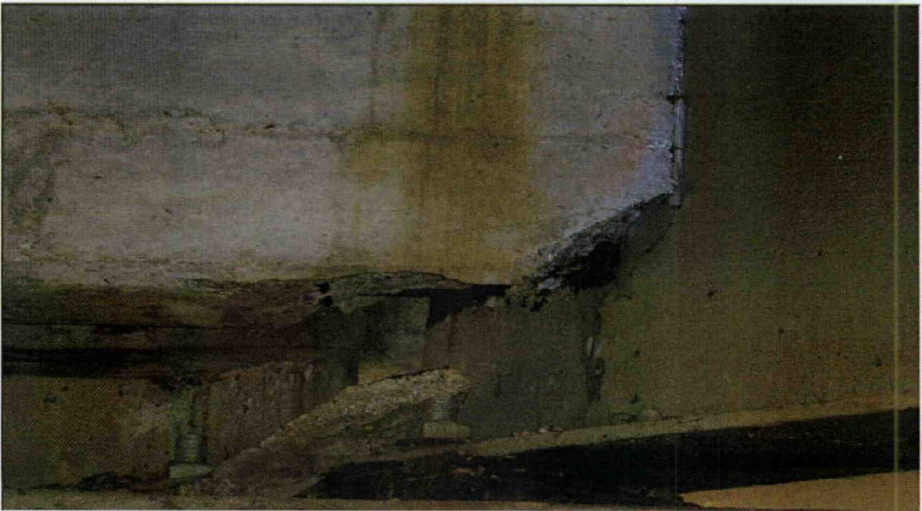
SPALL IN BAY1 SPAN 1 DIAPHRAGM OTHERS SIMILAR
