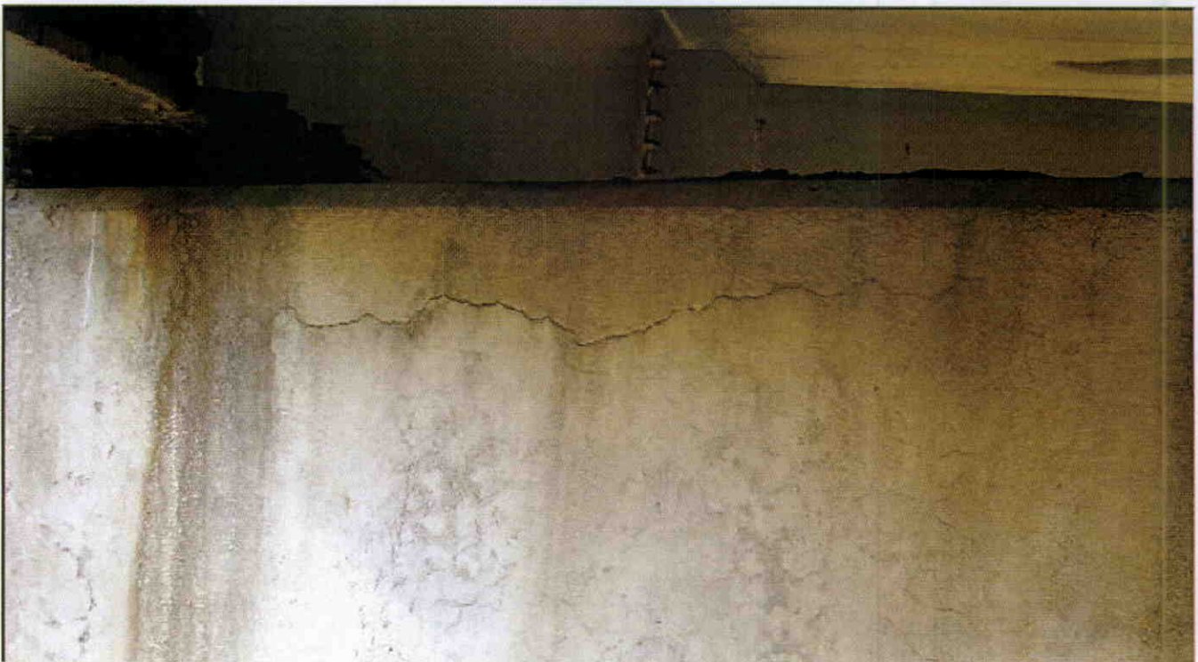
CRACK IN SPAN 5 SIDE OF BENT 4
