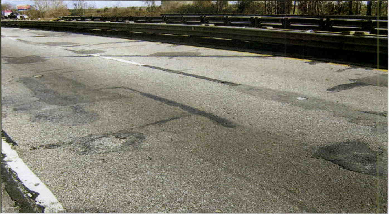
MISSING ASPHALT AND PATCHES IN WEARING SURFACE IN WEARING SURFACE IN OF SPAN 1
