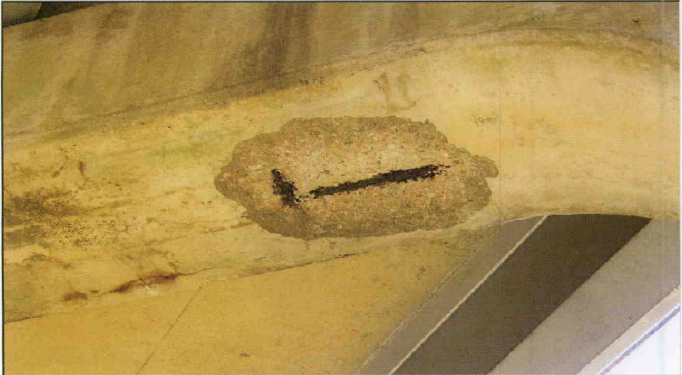
SPALL WITH EXPOSED REBAR IN BOTTOM OF CAP OF BENT 3 BETWEEN COLUMN 2 AND COLUMN 3
