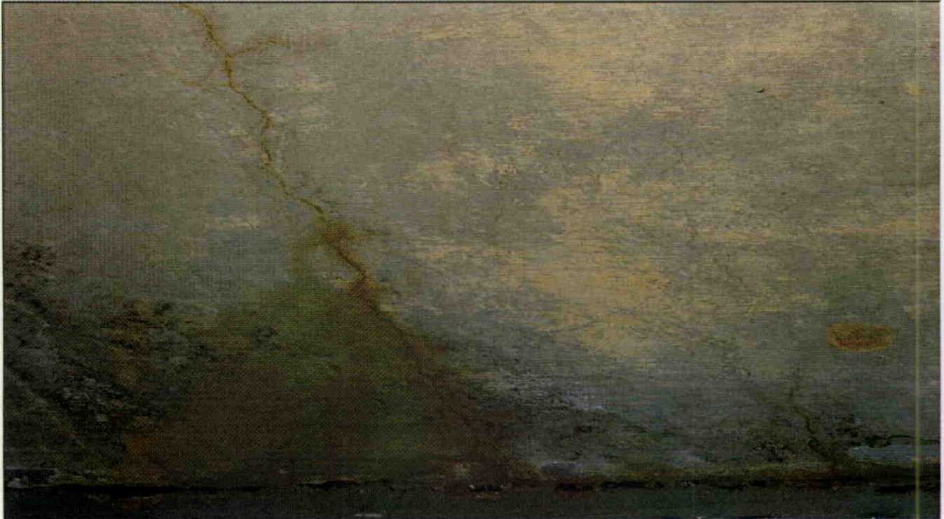
TRANSVERSE CRACK IN BOTTOM OF DECK OF BAY 1 SPAN 1
