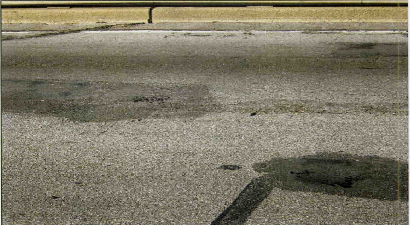
CRACKS AND PATCHES IN WEARING SURFACE IN WEARING SURFACE OF SPAN 5
