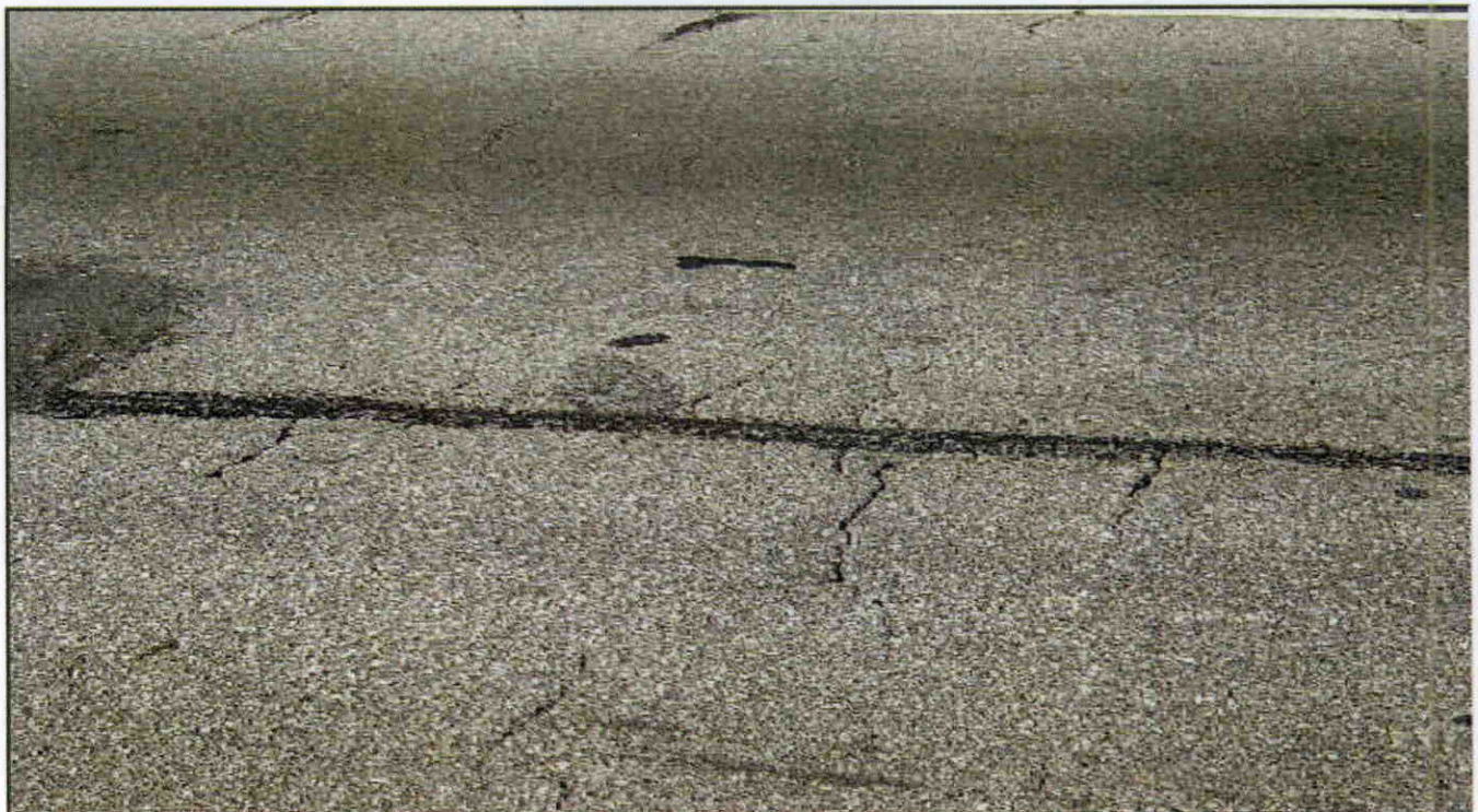
CRACKS PATCHES IN WEARING SURFACE AND VOIDS IN ASPHALT WEARING SURFACE OF SPAN 4
