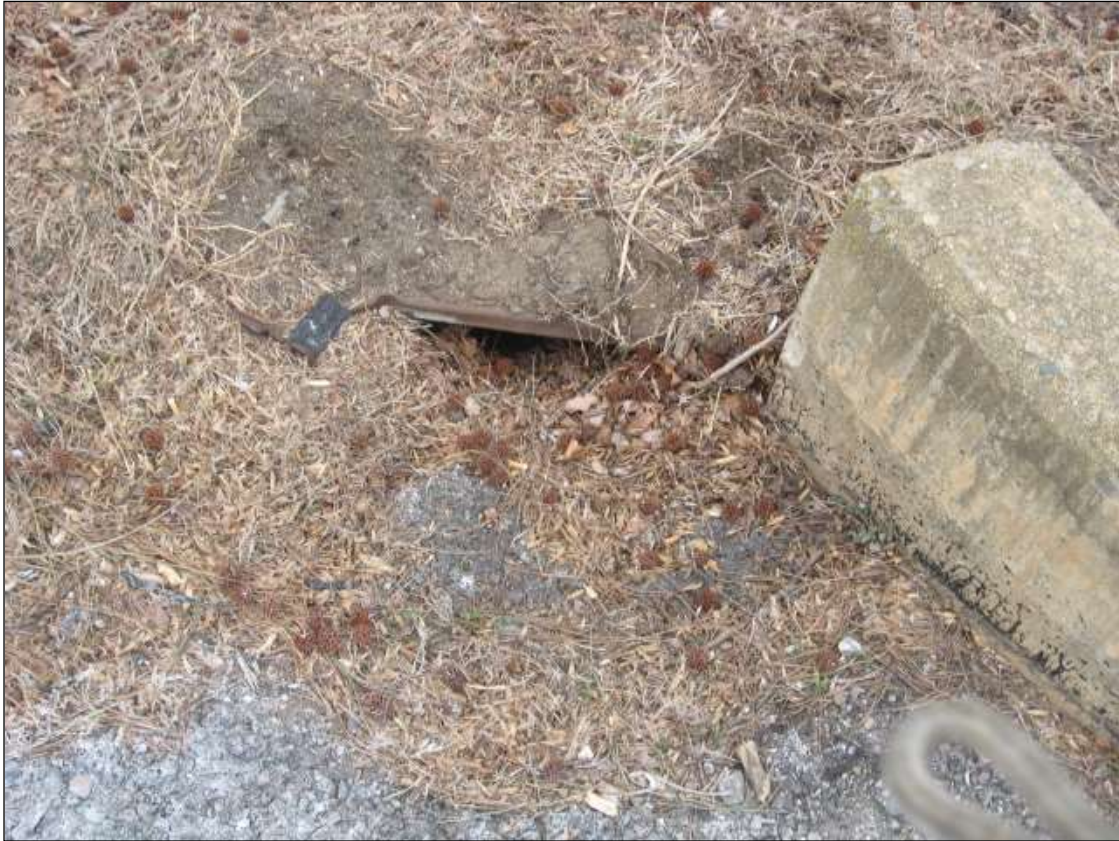
DRAIN BLOCKED WITH DIRT AND DEBRIS @ SOUTH WEST CORNER
