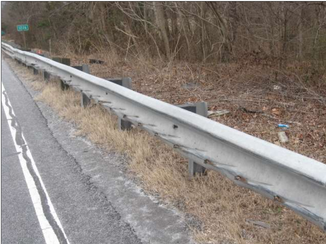
DAMAGED GUARDRAIL @ WEST SIDE THROUGH OUT BRIDGE
