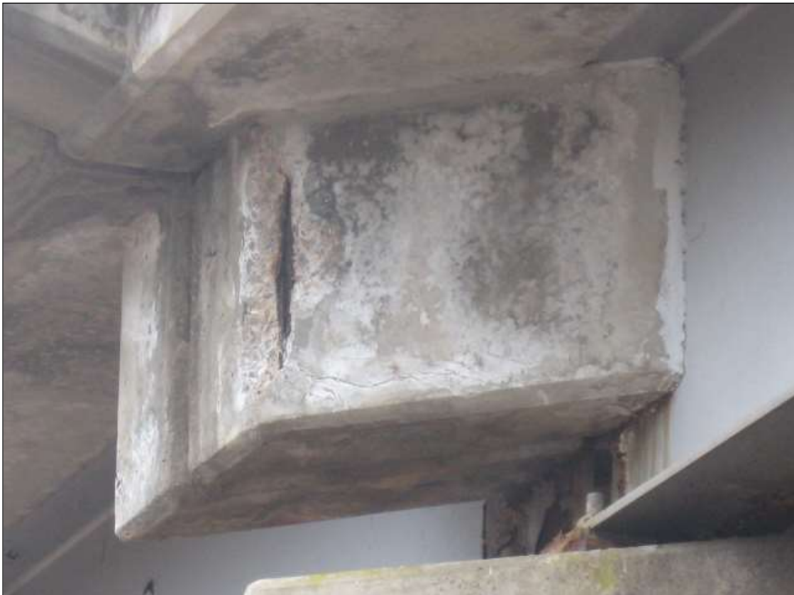
SPALL IN DIAPHRAGM OVER INTERIOR BENT 1 RIGHT SIDE WITH EXPOSED STEEL
