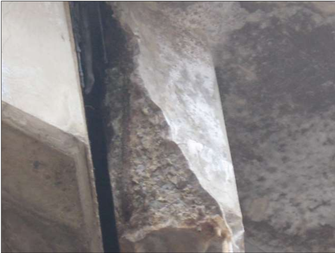
SPALL IN DIAPHRAGM WITH EXPOSED STEEL OVER INTERIOR BENT 2 RIGHT SIDE
