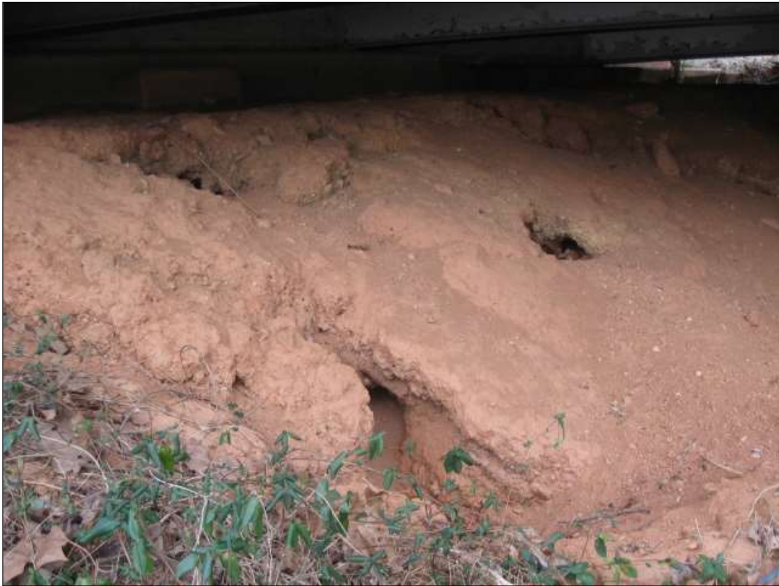
RODENT HOLES IN SLOPE @ END BENT 2
