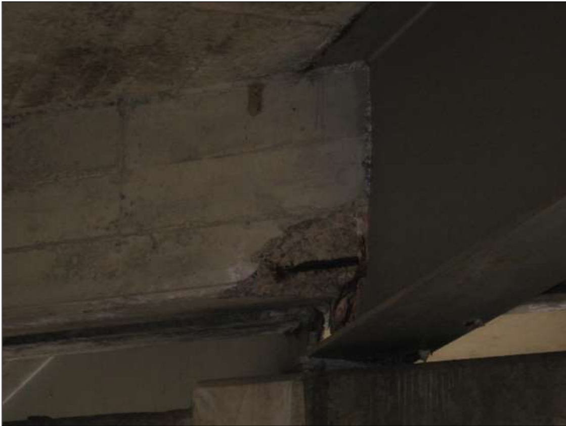
SPALL IN DIAPHRAGM WITH EXPOSED STEEL OVER INTERIOR BENT 3 SPAN 4 SIDE BAY 2
