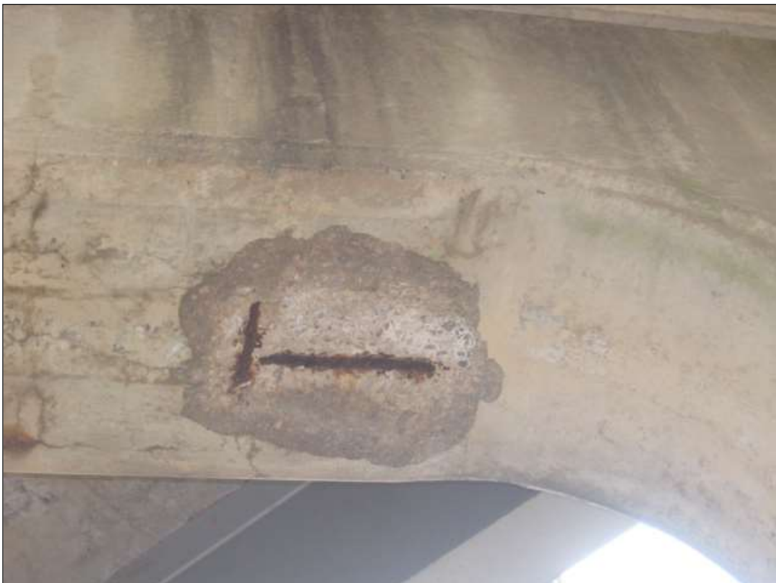
SPALL IN BOTTOM OF CAP WITH EXPOSED STEEL @ INTERIOR BENT 3 BETWEEN COLUMN 2 AND COLUMN 3 ( 10 IN DIAMETER X 2 IN DEEP )
