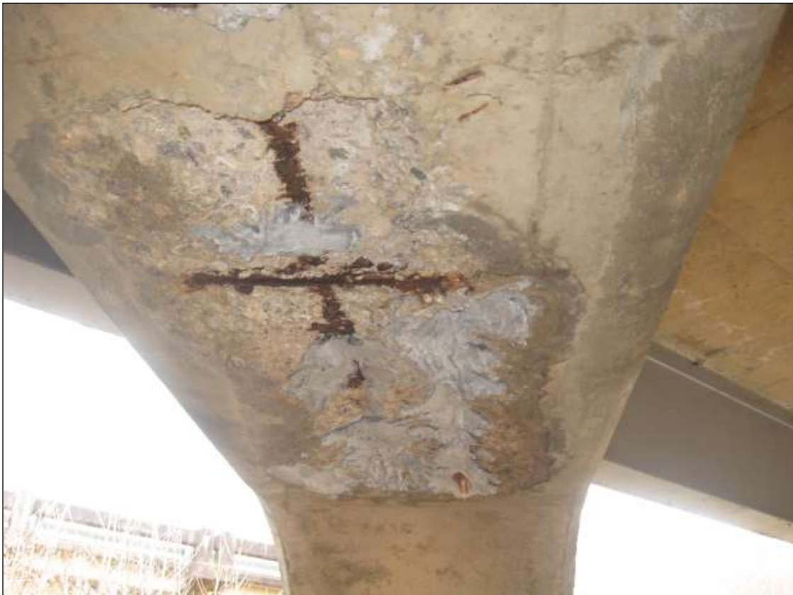
SPALL UNDER BOTTOM OF CAP WITH EXPOSED STEEL @ INTERIOR BENT 4 BETWEEN COLUMN 2 AND COLUMN 3 ( 4FT LONG X 2FT WIDE X 3 IN DEEP )
