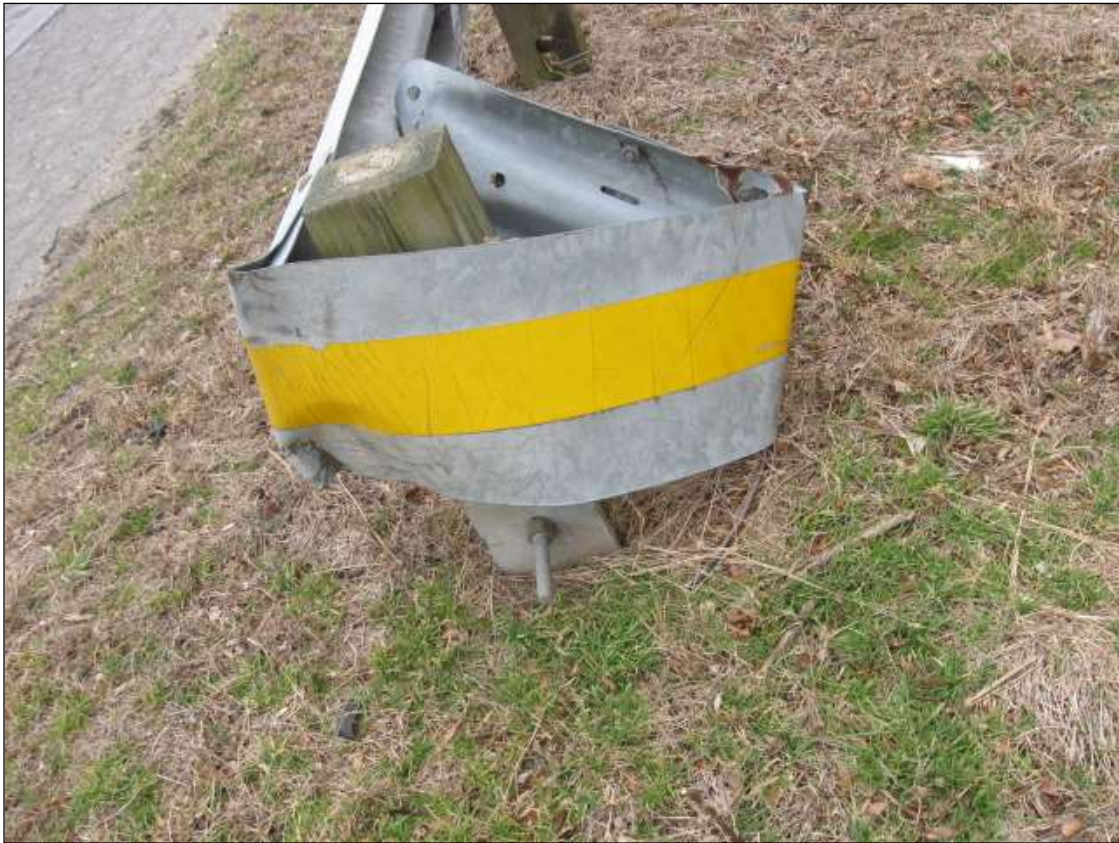
DAMAGED GUARDRAIL TERMINAL @ NORTH WEST CORNER
