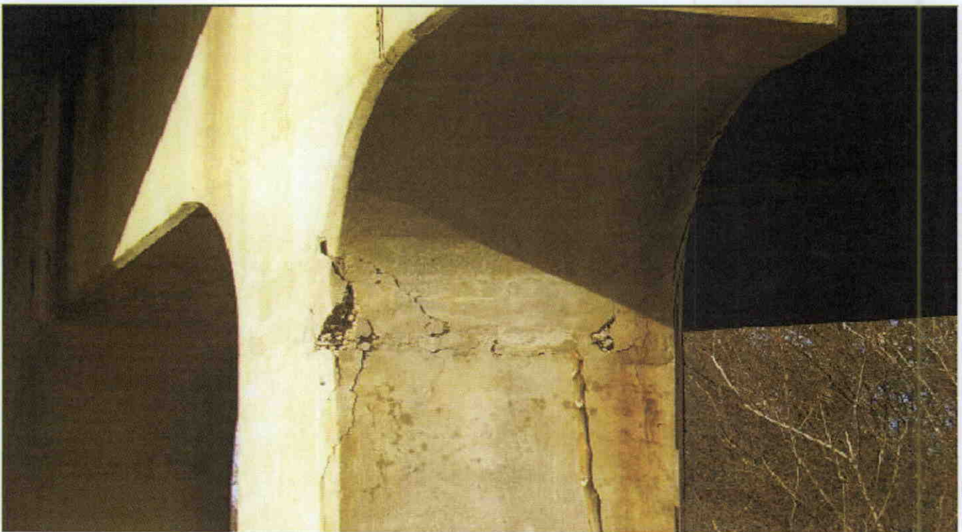
SPALLS CRACKS AND DELAMINATION IN RIGHT SIDE OF COLUMN 3 BENT 3
