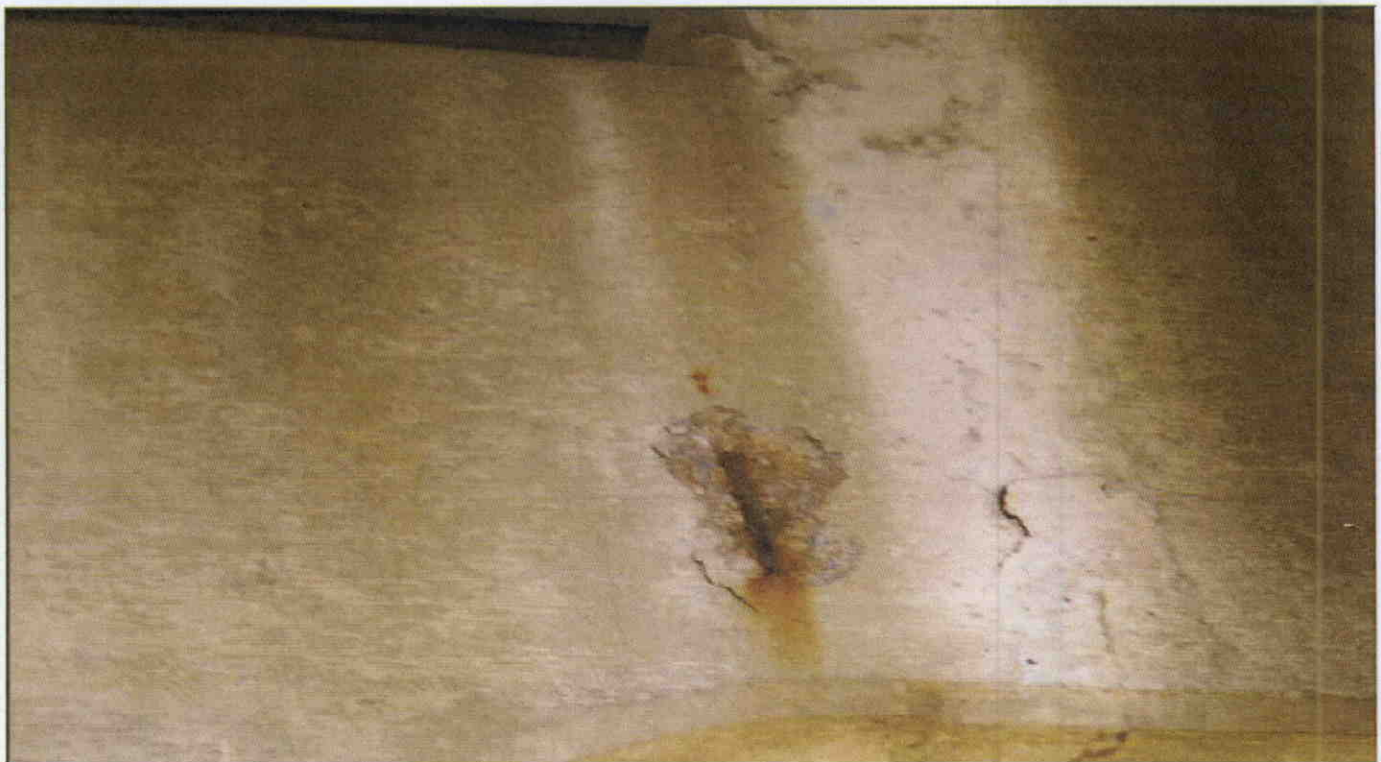
SPALL WITH EXPOSED REBAR IN FACE OF SPAN 3 SIDE OF BENT 3 AT BEAM 3
