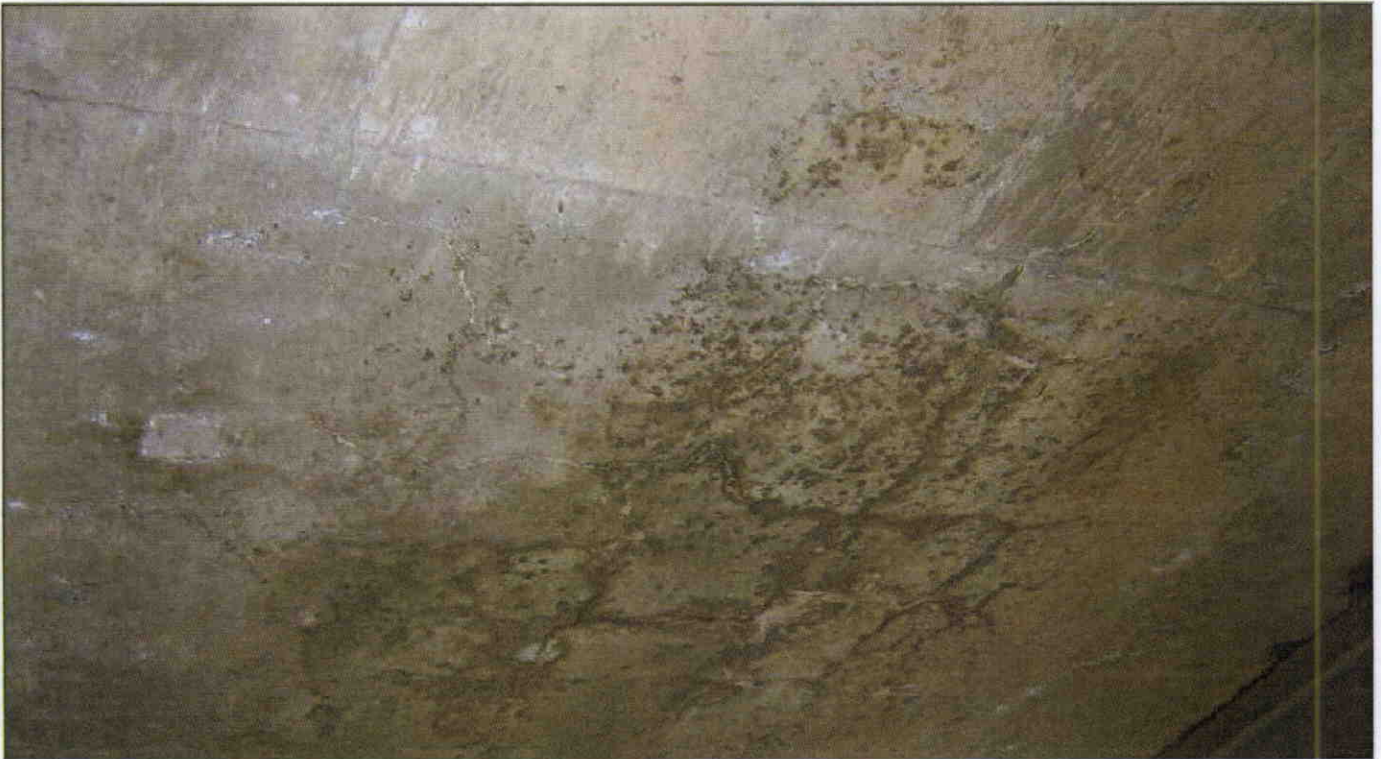
CRACKS WITH EFFLO LEAKAGE IN BOTTOM OF DECK BAY 3 SPAN 1
