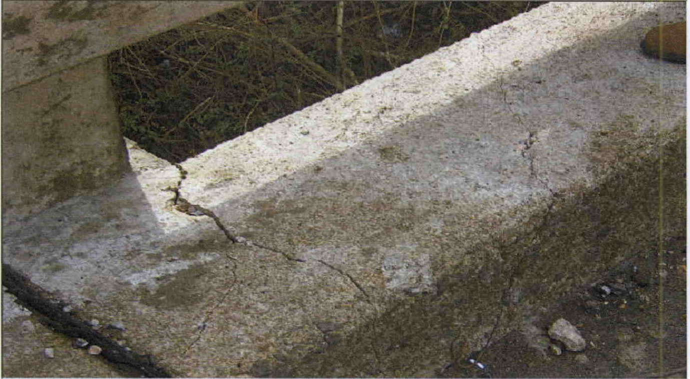
CRACKED CURB AT RIGHT SIDE OF SPAN 2 AT BENT 2
