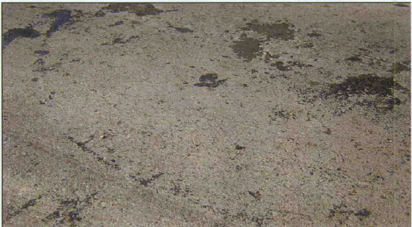
MAP CRACK IN TOP OF DECK SPAN 4
