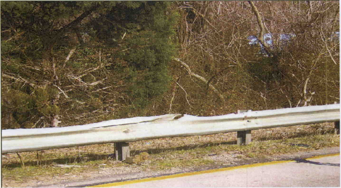
GUARDRAIL DAMAGE AT LEFT SIDE OF APPROACH 1
