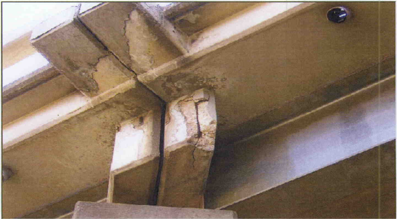
SPALL WITH EXPOSED REBAR IN LEFT DIAPHRAGM AT BENT 2
