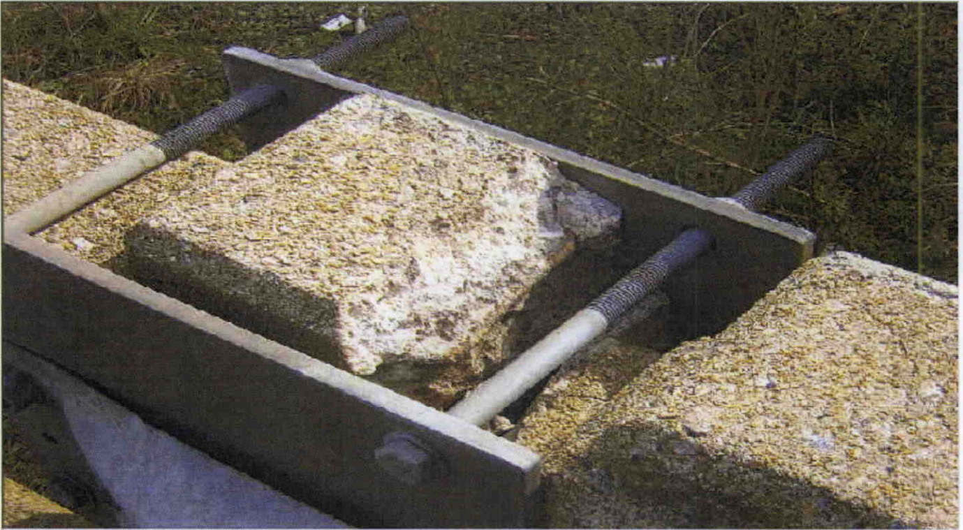
SPALL IN GUARDRAIL POST AT RIGHT SIDE ATTACHMENT END BENT 1
