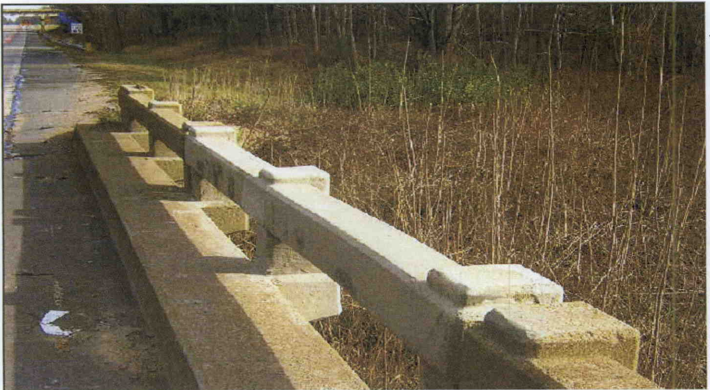
GUARDRAIL REPAIR AT RIGHT SIDE OF SPAN 4
