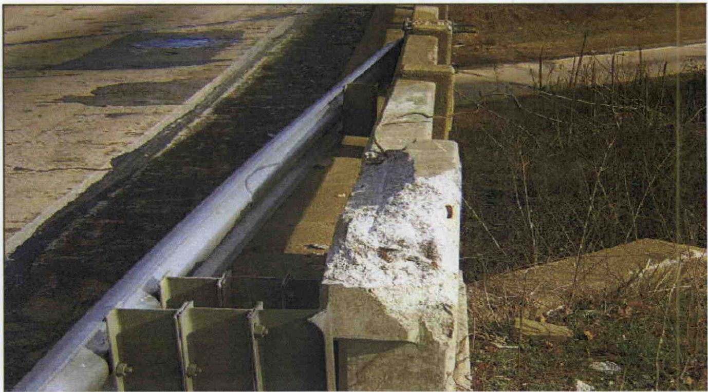
COLLISION DAMAGE AT RIGHT ENDPOST OF END BENT 1
