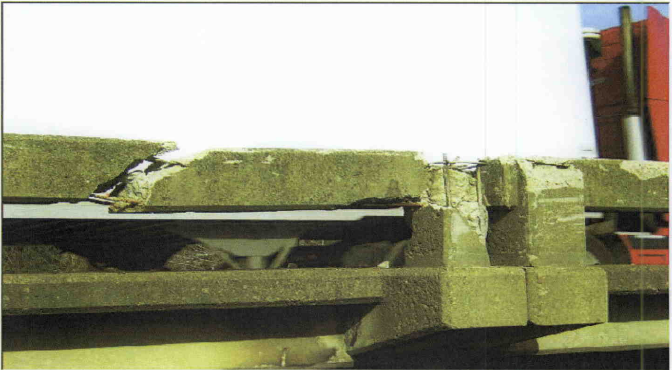
GUARDRAIL DAMAGE AT RIGHT SIDE OF SPAN 1 AT BENT 1
