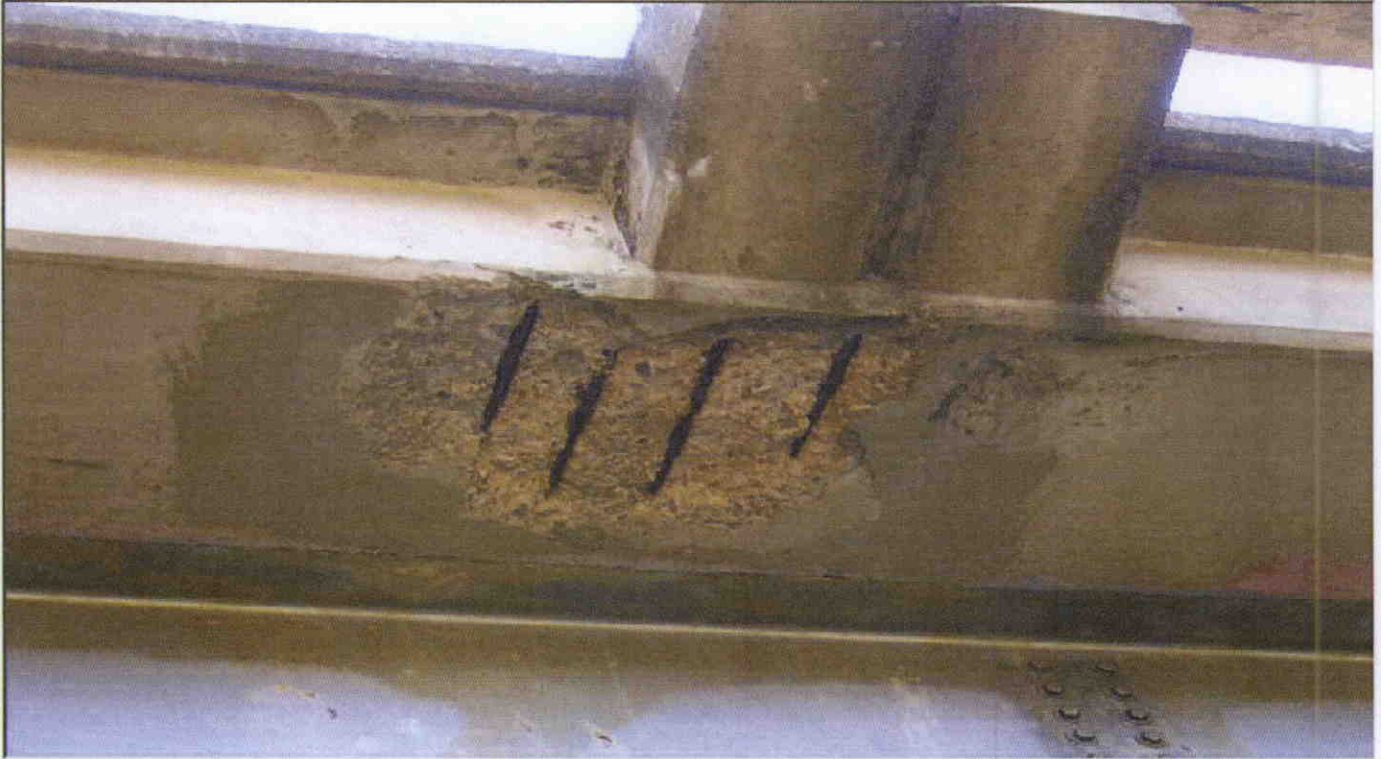
SPALL WITH EXPOSED REBAR IN BOTTOM OF LEFT OVERHANG SPAN 2
