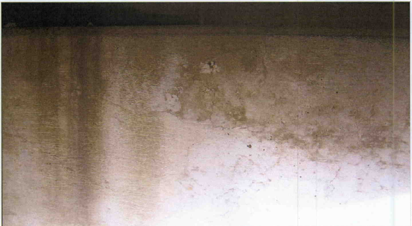
HAIRLINE CRACKS IN SPAN 1 SIDE FACE OF BENT 1 BAY 3
