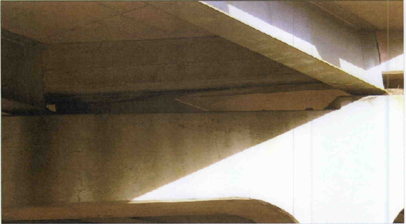
LONGITUDINAL CRACK IN FACE OF SPAN 3 SIDE OF BENT 3 CAP AT BAY 3
