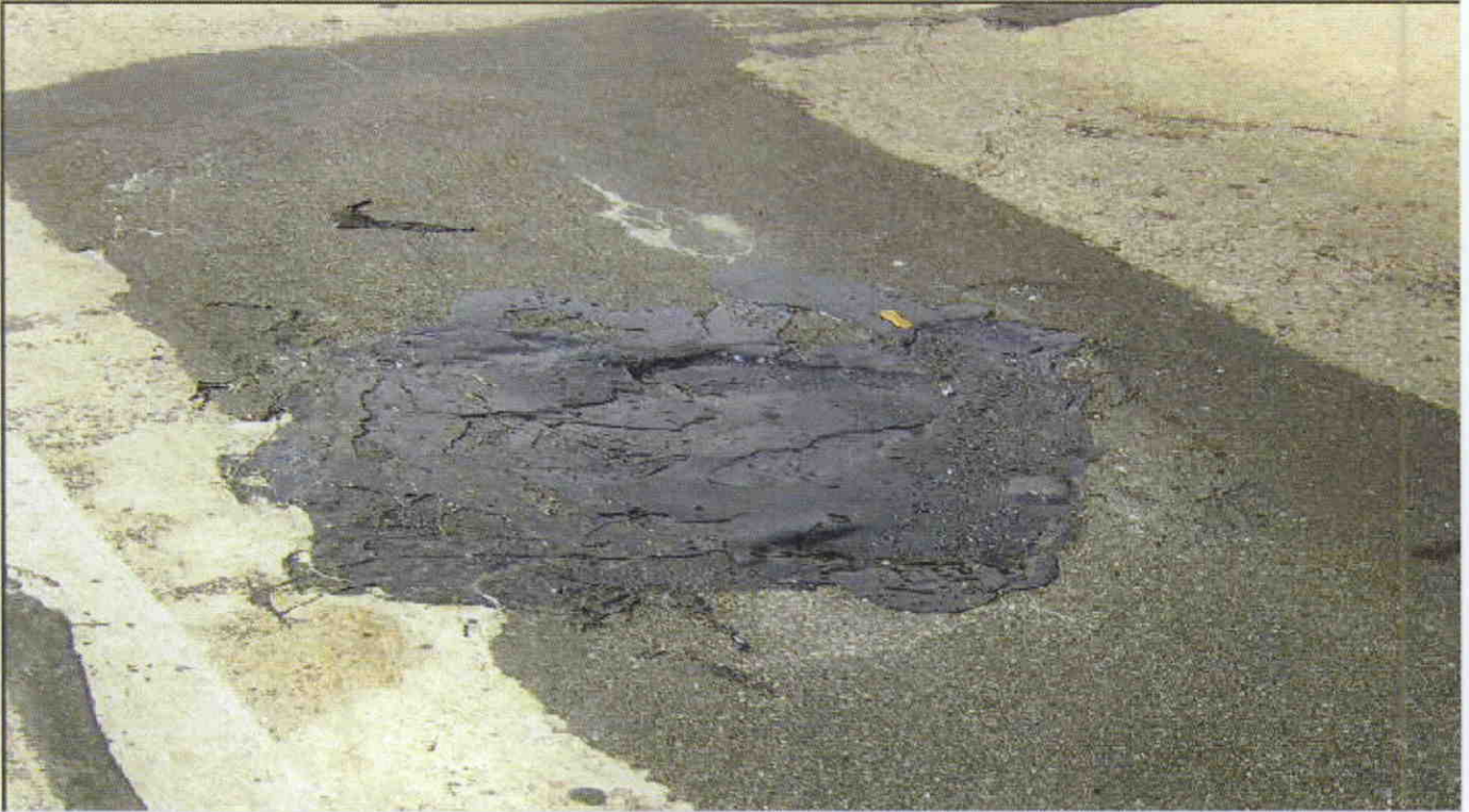
PATCH AND SETTLEMENT IN TOP OF DECK SPAN 1
