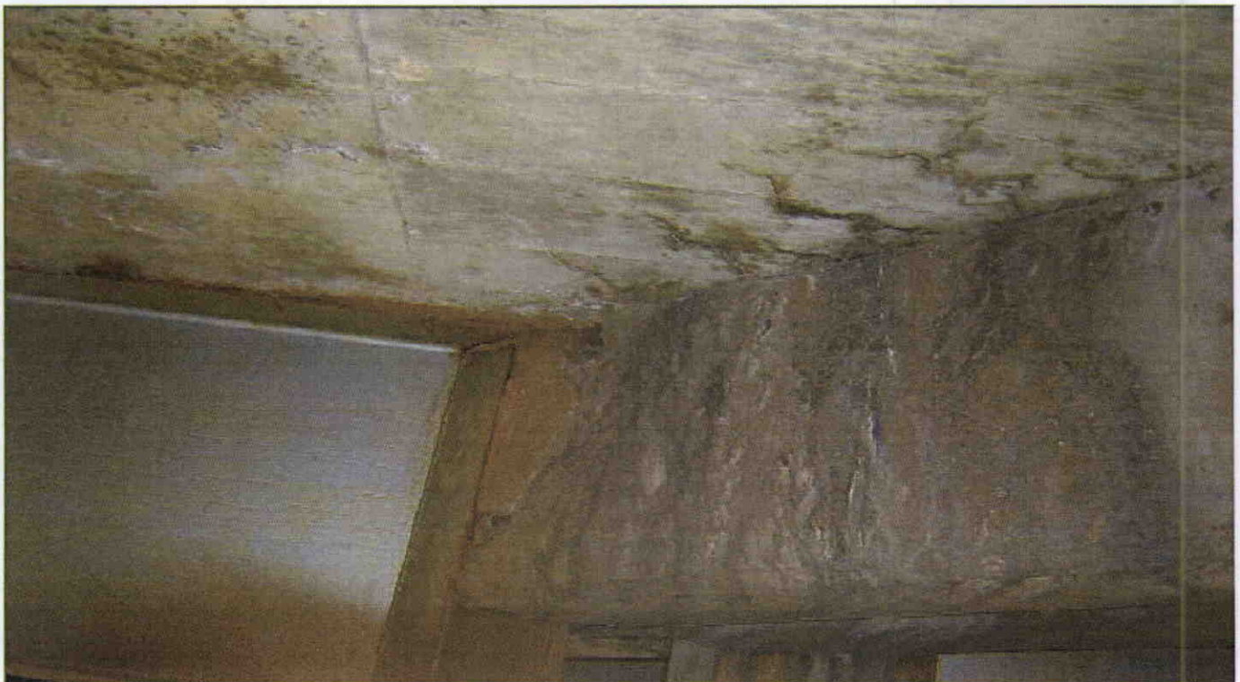
CRACKS AND SPALLS IN BAY 3 DIAPHRAGM OF SPAN 1 AT BENT 1
