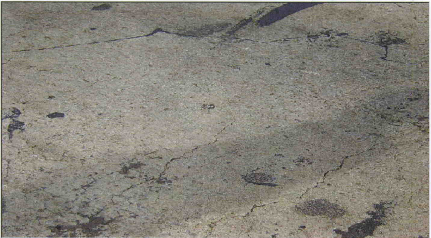
TRANSVERSE CRACKS IN TOP OF DECK SPAN 1
