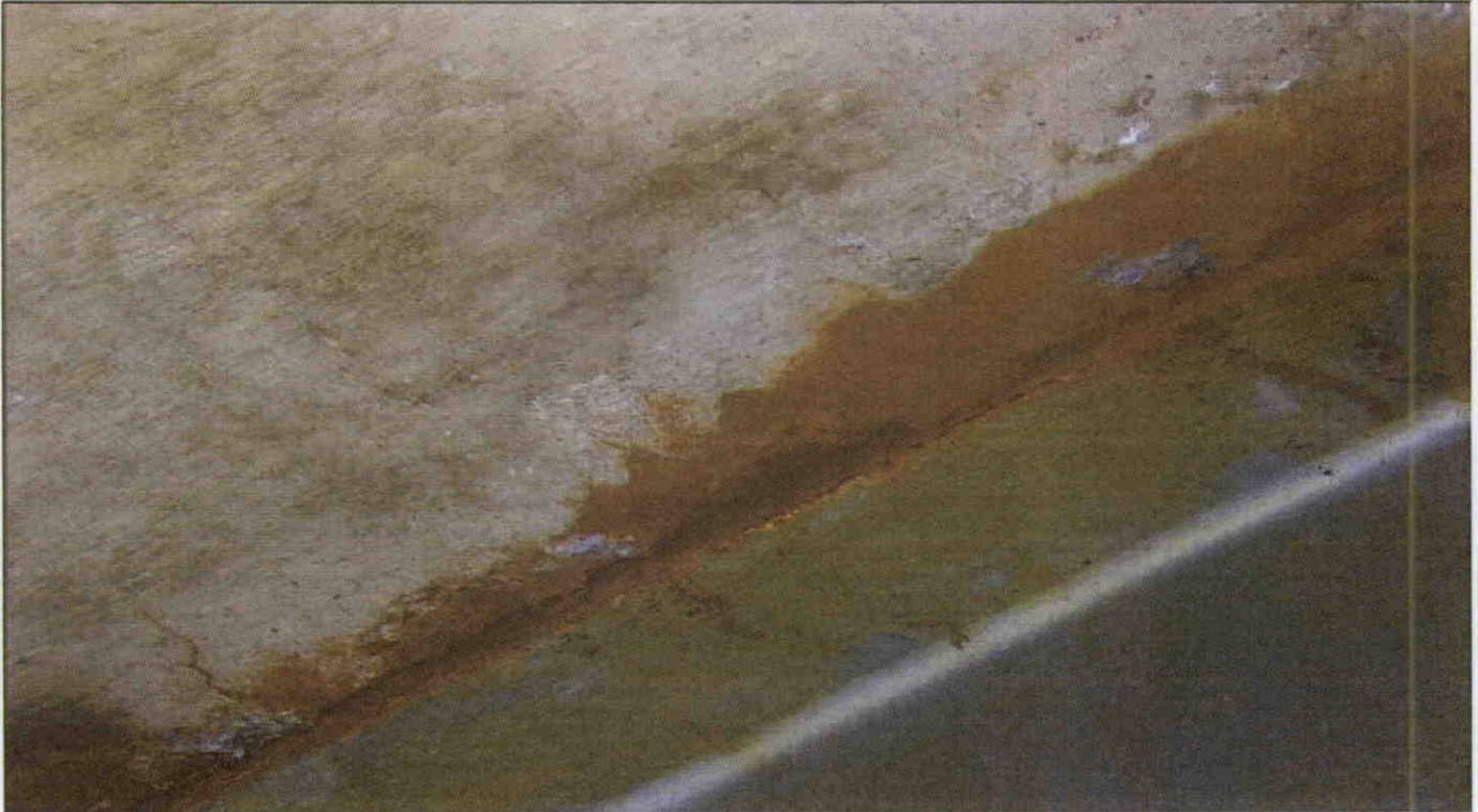
RUST POWDER STAIN IN BOTTOM OF DECK AT BEAM 3 SPAN 1 AT BENT 1
