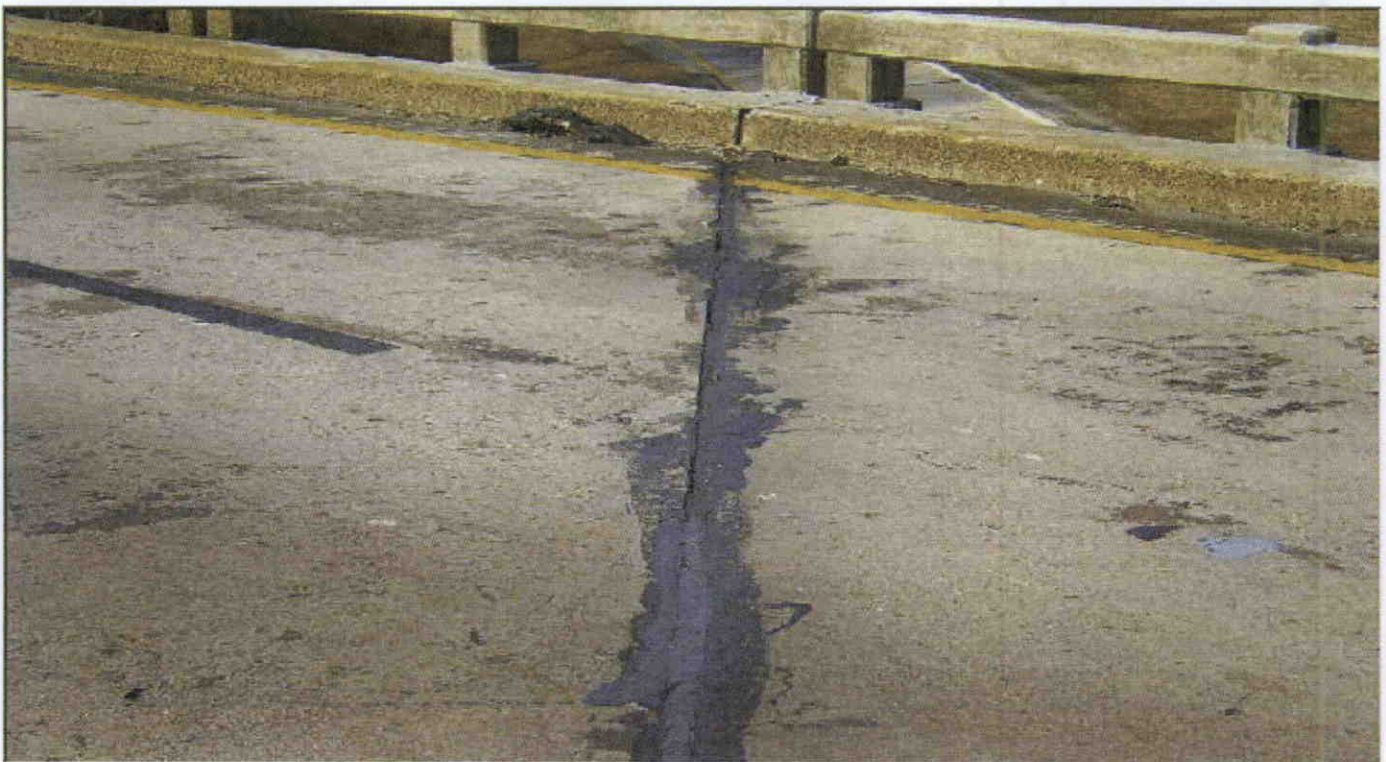
JOINT IN TOP OF DECK OVER BENT 2
