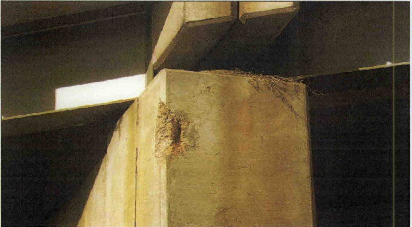
SPALL WITH EXPOSED REBAR IN RIGHT END OF BENT 3 CAP
