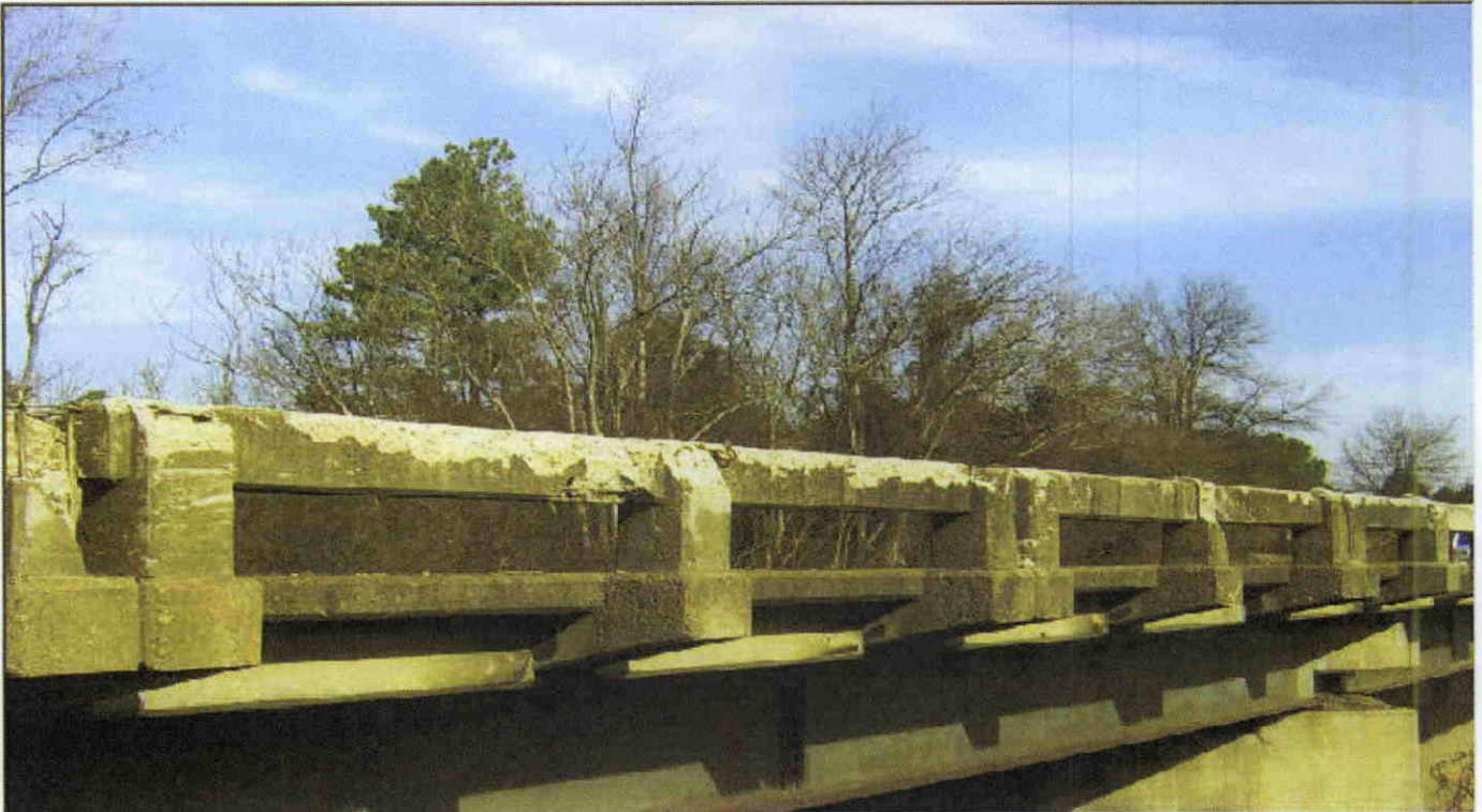
GUARDRAIL DAMAGE AT RIGHT SIDE OF SPAN 2
