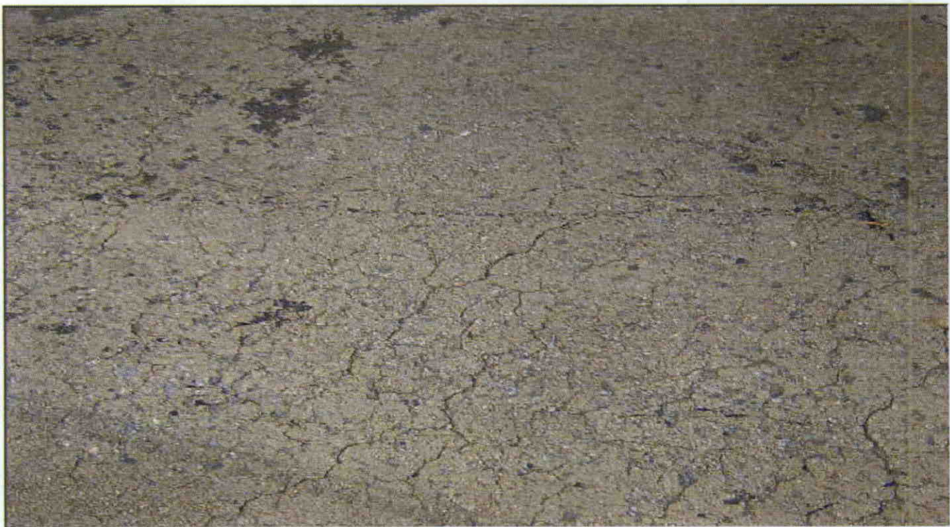
MAP CRACKS AND SCALING WITH EXPOSED COARSE AGGREGATE IN TOP OF DECK SPAN 2
