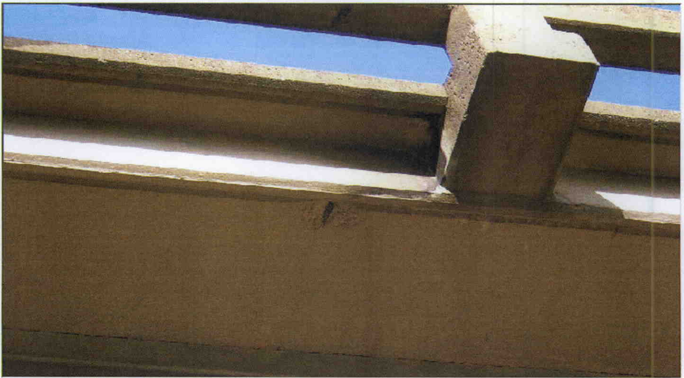
SPALL WITH EXPOSED REBAR IN BOTTOM OF RIGHT OVERHANG SPAN 3
