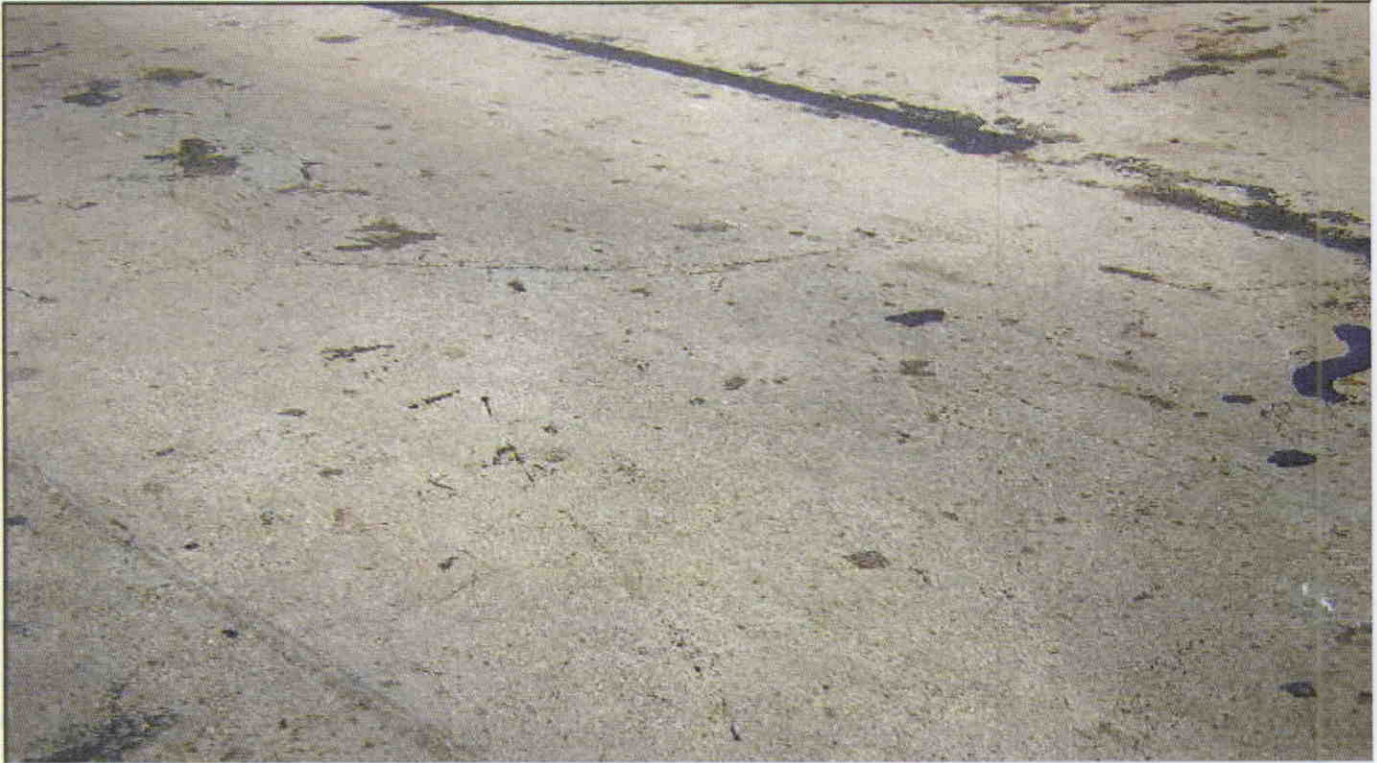
TRANSVERSE AND MAP CRACKS AND SCALING WITH EXPOSED COARSE AGGREGATE IN TOP OF DECK SPAN 3
