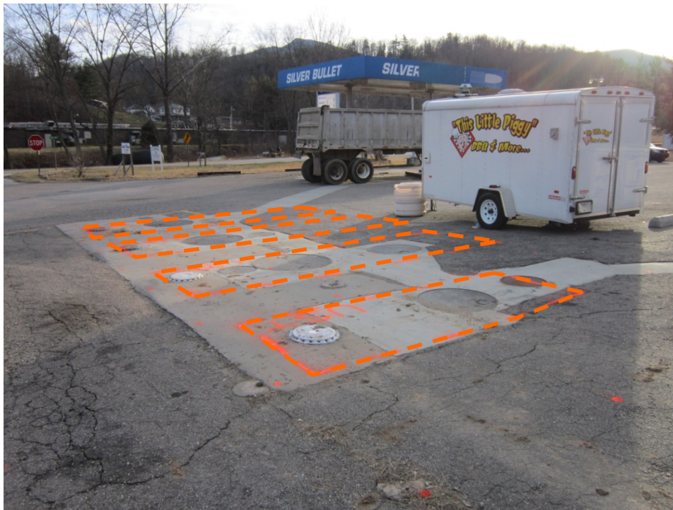
Parcel 12 (William Young Property), looking southwest. Photo shows approximate marked locations of known UST Nos. 1 through 4 near the southeast corner of the building.
