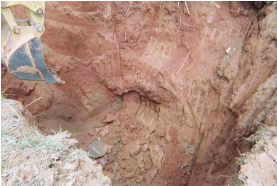
Photograph 2: Excavating pit to remove potentially contaminated soil (note stained soil at far end of excavation).
