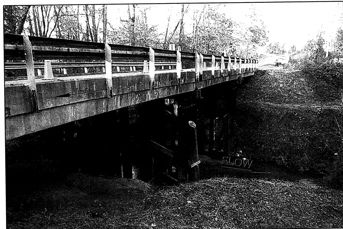
PHOTO TAKEN FROM NEAR THE END BENT 2 LOOKING DOWNSTATION FROM THE RIGHT OF THE BRIDGE.
