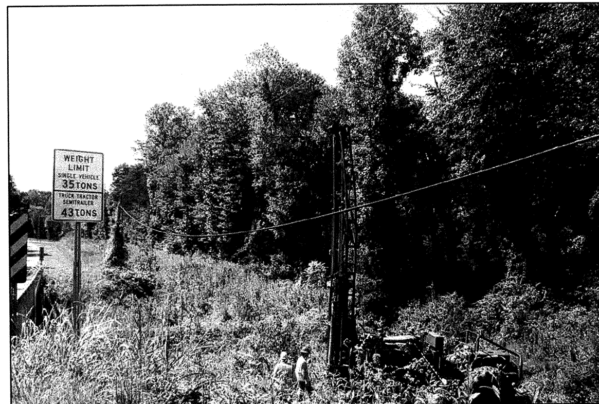
PHOTO TAKEN FROM NEAR END BENT 2 LOOKING AT EB2 (-LDET-) BEING DRILLED.
