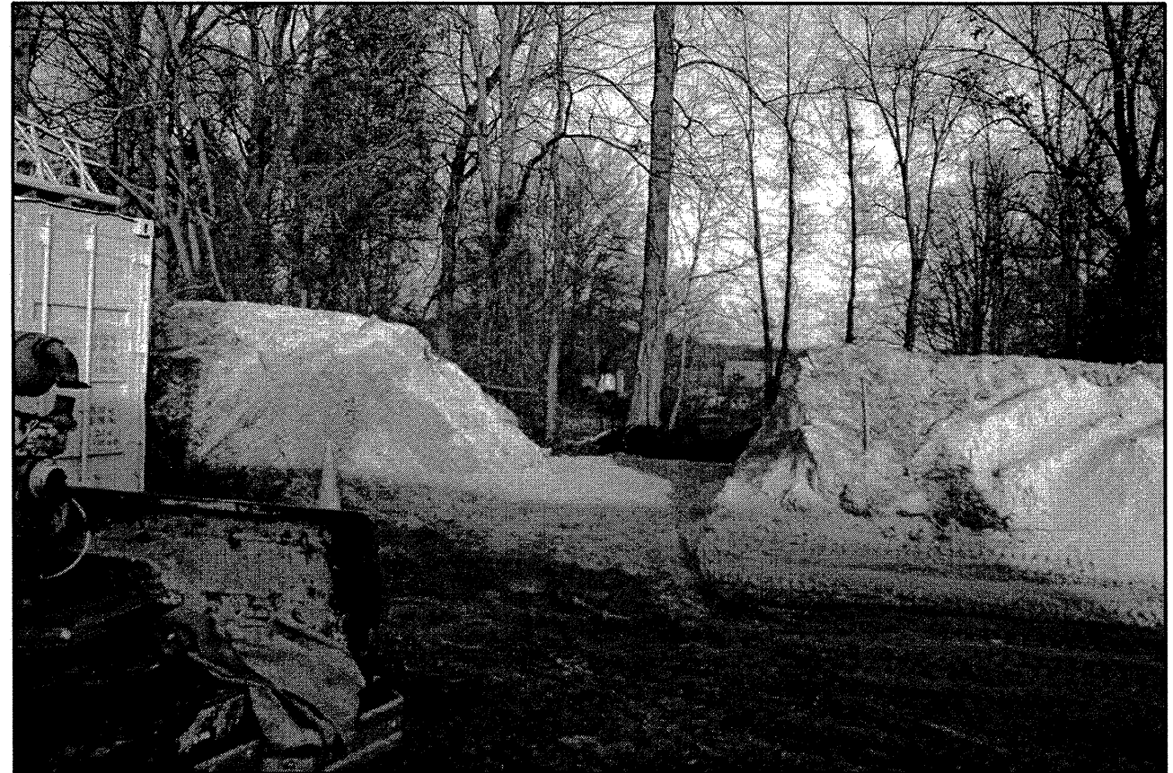
PHOTO TAKEN FROM NEAR END BENT 2, LOOKING DOWNSTATION (ALONG -L-) TOWARD B1-A. AS SHOWN ABOVE, EXCAVATION WAS REQUIRED TO ACCESS BORINGS B1-A AND B1-B. BORING EB2-A IS SHOWN BY TRAFFIC CONE.
