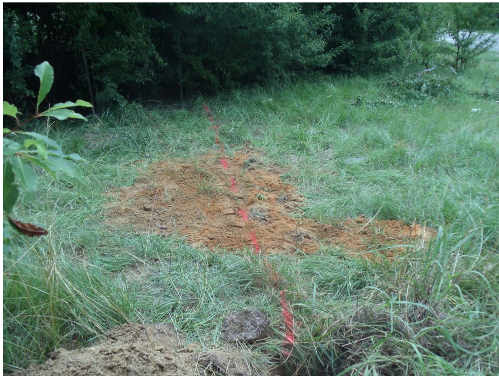
Buried section of vent pipe was traced with Fisher Gemini-3 to wooded area east of building
