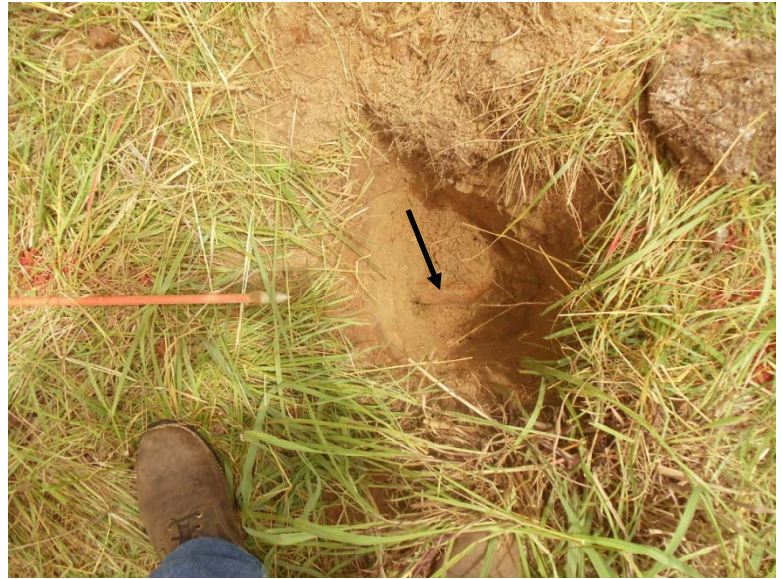
Buried section of vent pipe (arrow) excavated 6 feet east of building at depth of 1.4 feet.
