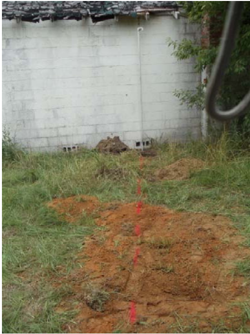
Vertical vent pipe at building and buried section of pipe traced to east
