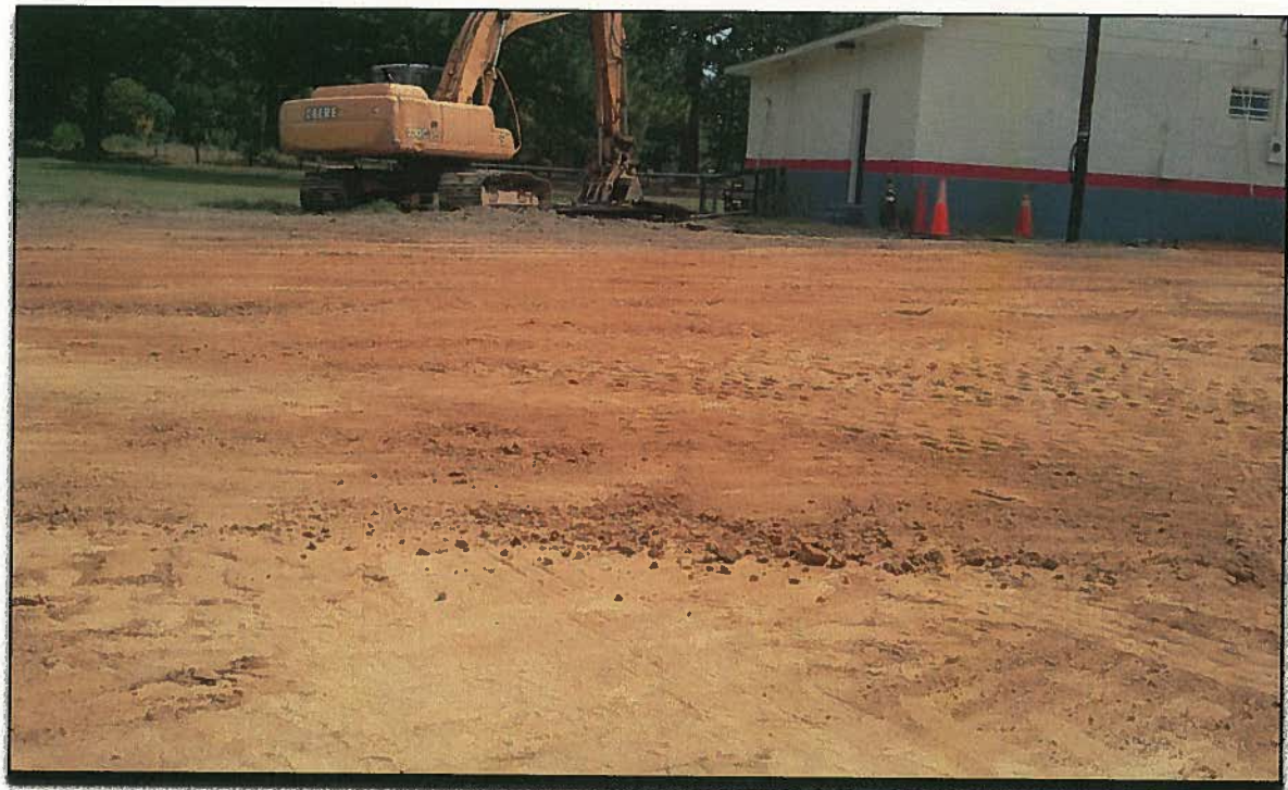
Looking East across former UST basin from near John Nunnery Rd. after backfilling, compaction, and finish grading.
