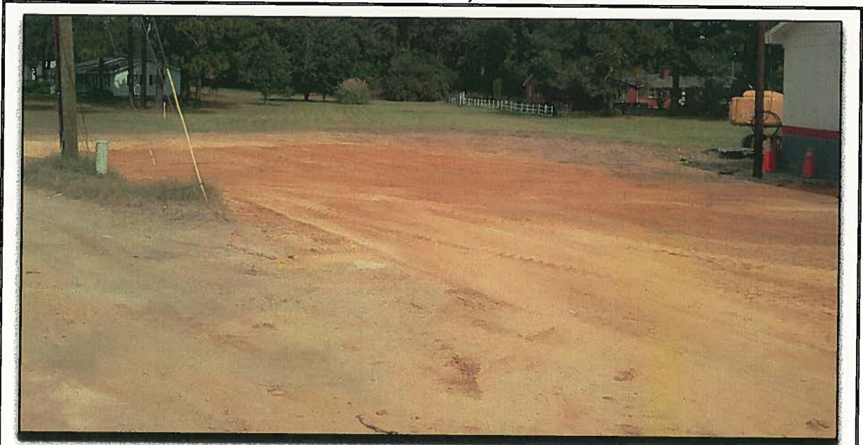
Looking Northeast across former UST basin and lines excavation from near John Nunnery Rd. and NC 24 after backfilling, compaction, and finish grading.
