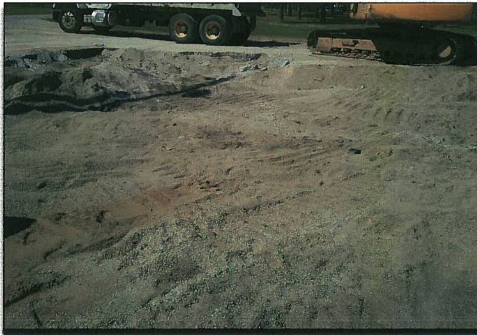
From Southeast side of UST Basin looking Northwest across excavation backfilled with "native" stone.
