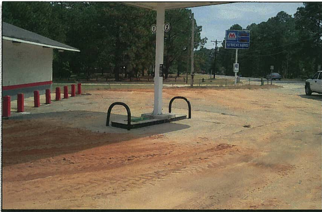
Looking East from near John Nunnery Rd. after backfilling, compaction, and finish grading.
