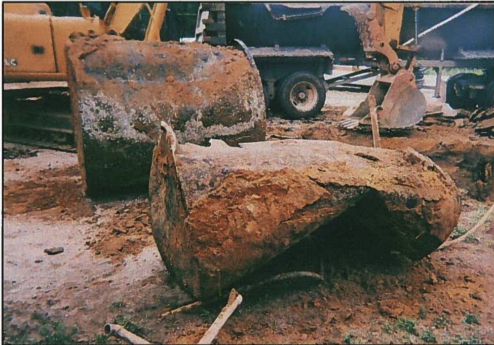
Looking Southeast, UST #4 and UST #5 (in foreground) removed from excavation (in background on right).
