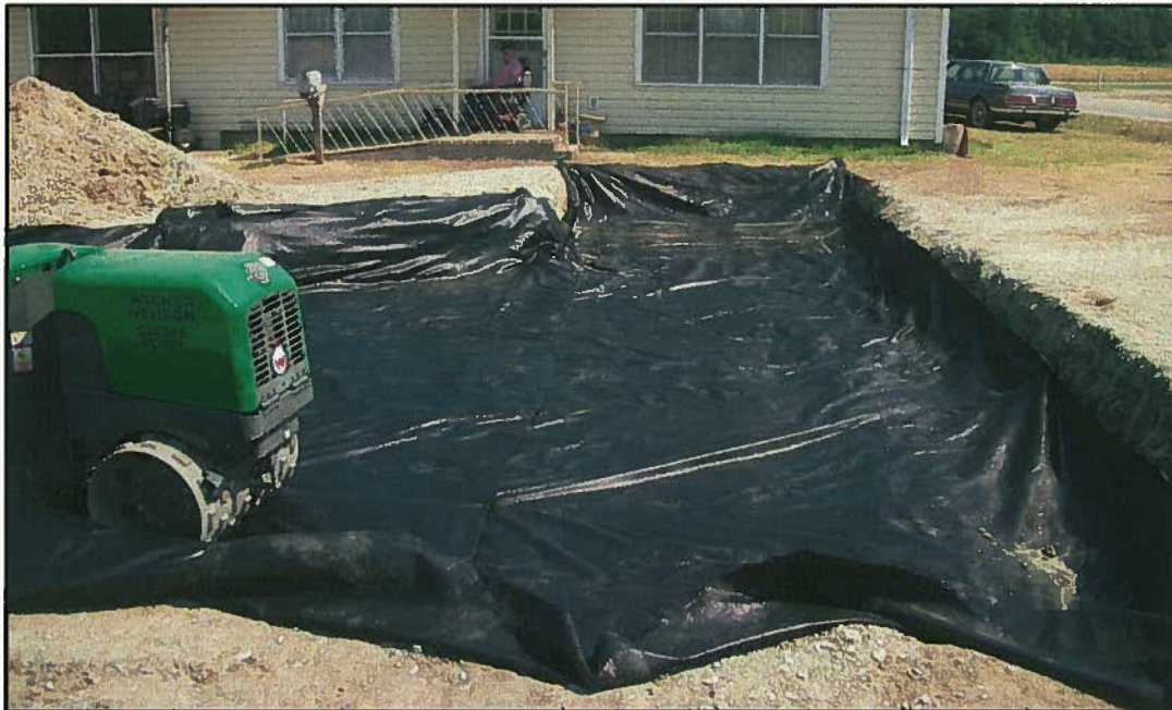
Looking North across UST #3, UST #2, and UST #1 excavation following removal of two (2) feet of unsuitable "pumping" fill and placing geotextile fabric.
