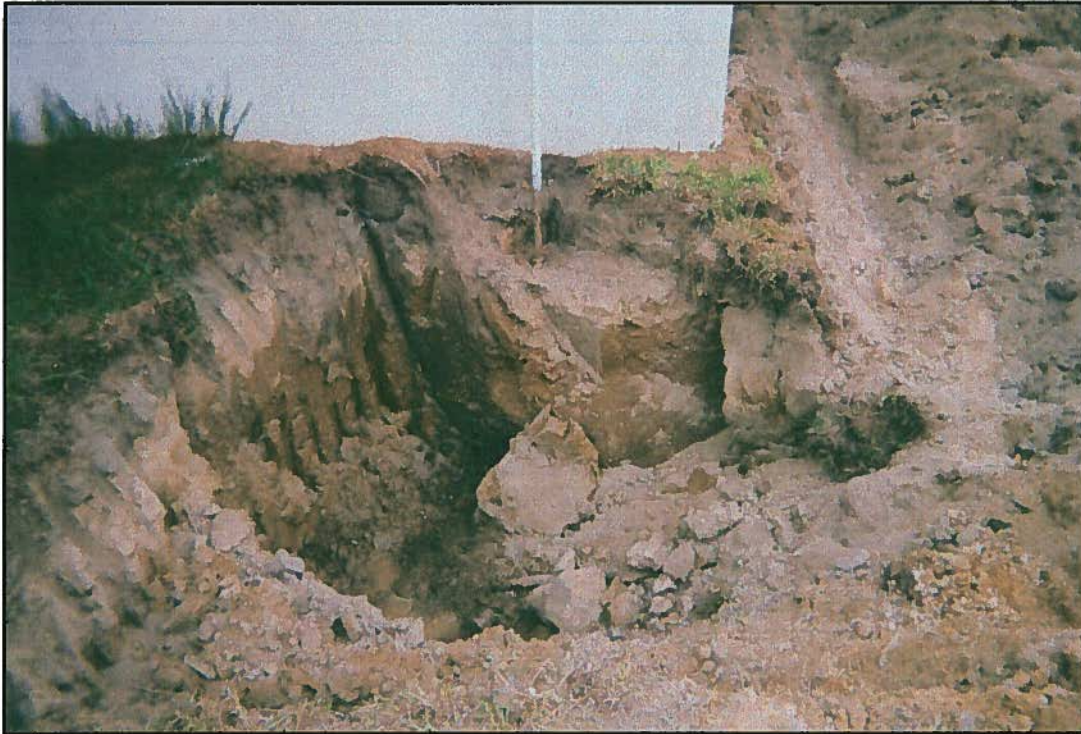
July 6, 2011 – Looking east at southwest corner of building and suspected UST location following excavation investigation.
